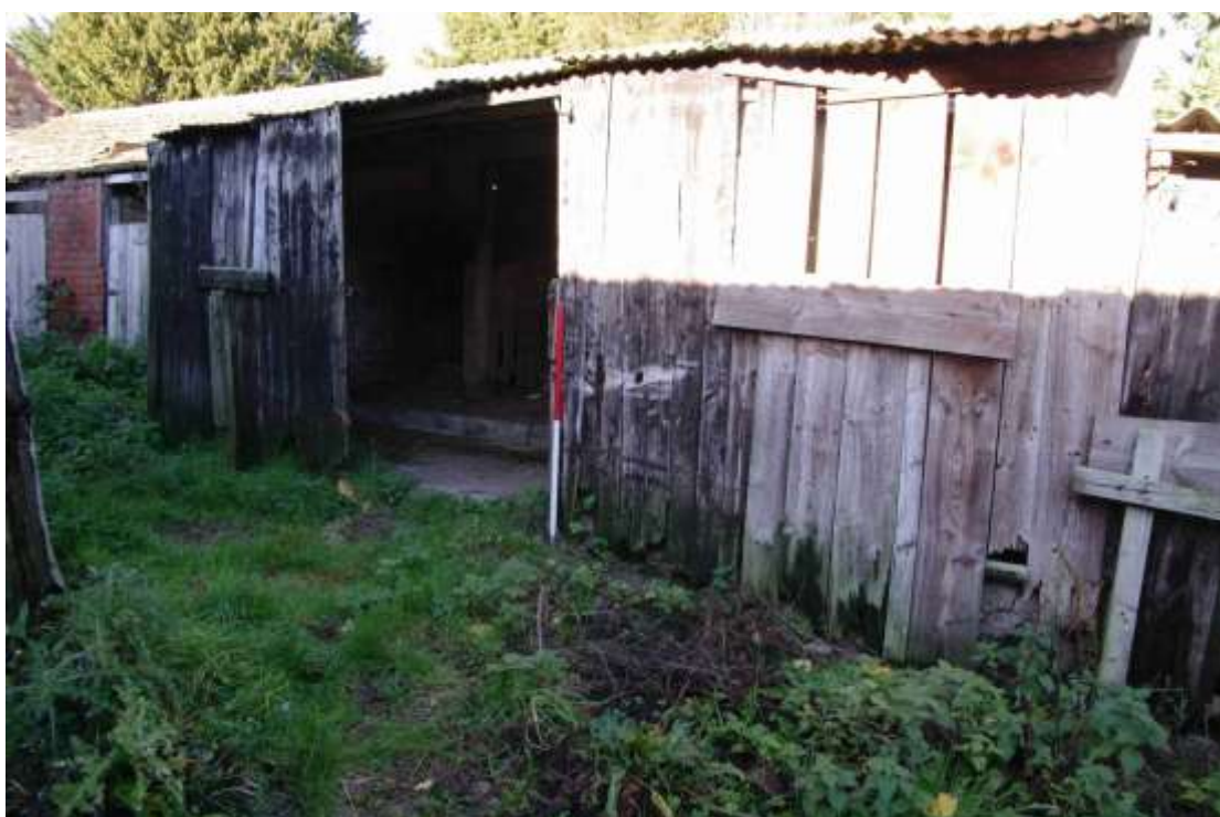
Figure 14: Shed 2 south facing elevation Looking north-west. 1m scale. Shed 1 on left, Shed 3 on right
