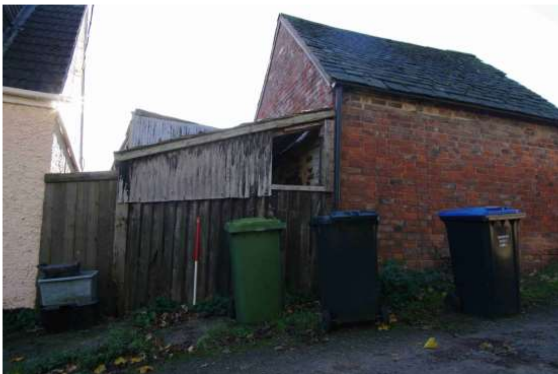
Figure 23: Sheds 4 and 5 north facing elevations Looking south-west. 1m scale. Shed 4 on right, Shed 5 on left
