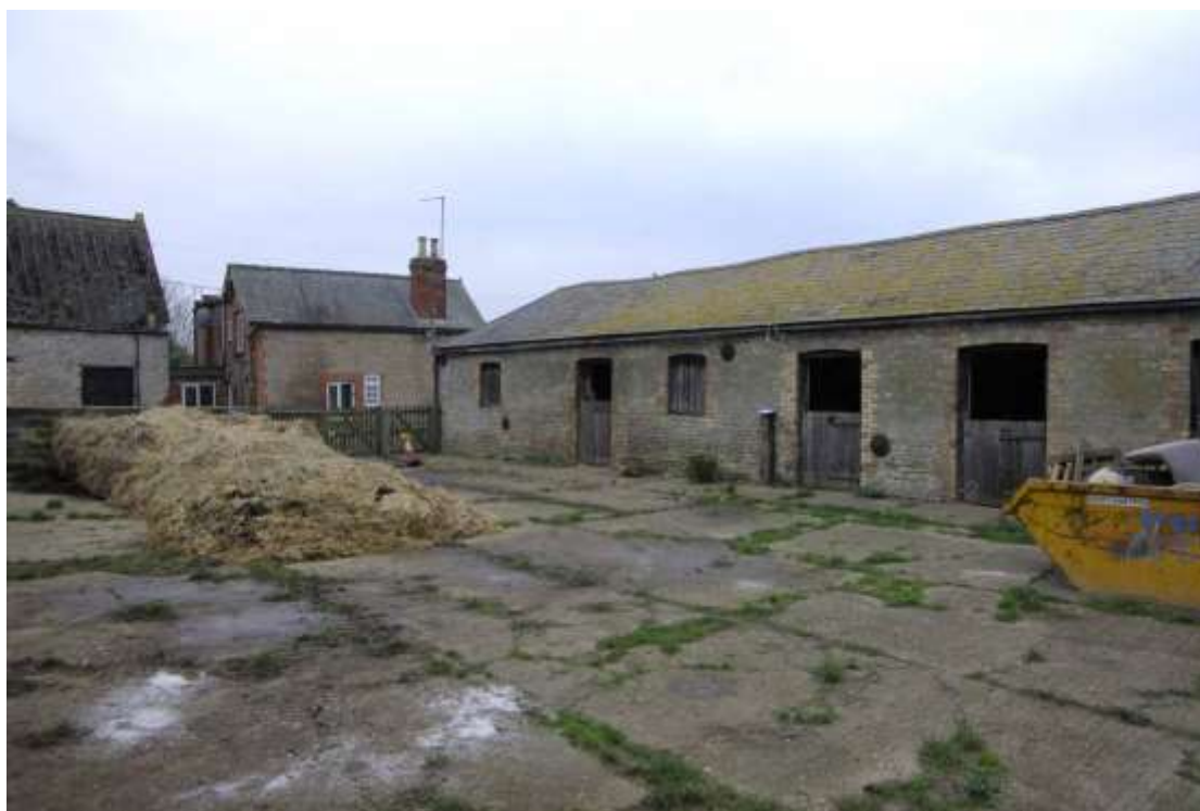
Figure 12 Main courtyard and west range Gatepost to left of centre doorway indicates location of original dividing wall. Looking south west
