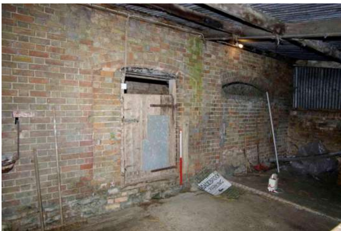
Figure 19 Ground floor of west facing elevation of hayloft Looking south east. 1m scale
