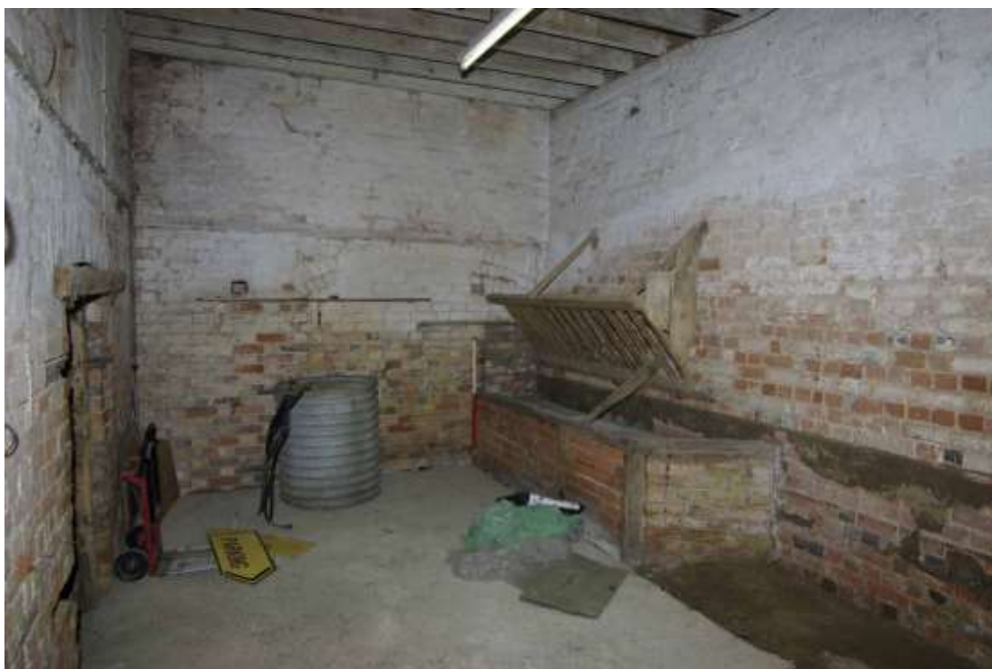
Figure 21 Hayloft building, ground floor western room (tack room) Looking north east. 1m scale
