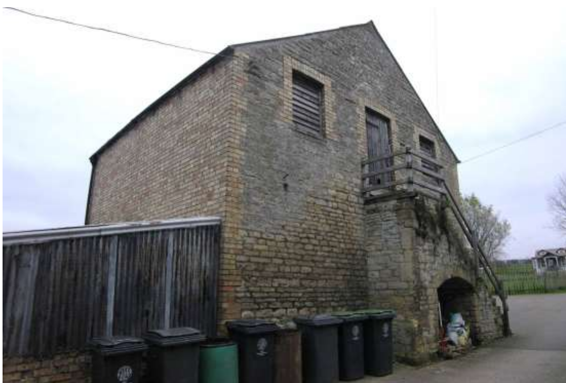
Figure 17 South facing elevation Looking north east. Corrugated lean-to on left. 1m scale
