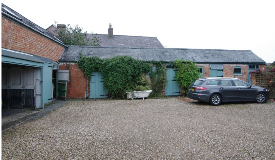
Figure 31 East range, west facing elevation Looking east. Brick joint to left of 1m scale
