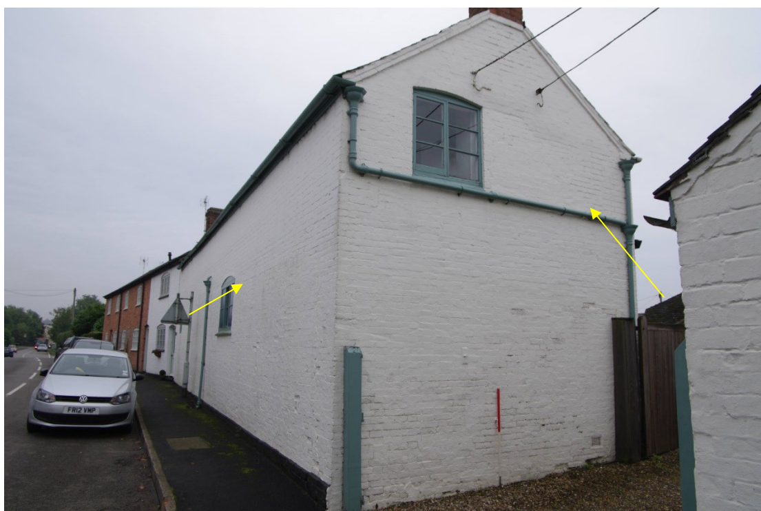
Figure 23 North range stables, west facing elevation Looking south-east. 1m scale. Arrows point to original wall and gable height
