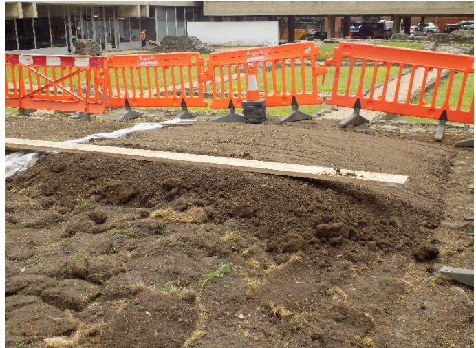
b. Building up the gradient of the slope and soil levels to a minimum of 150mm above the floor
