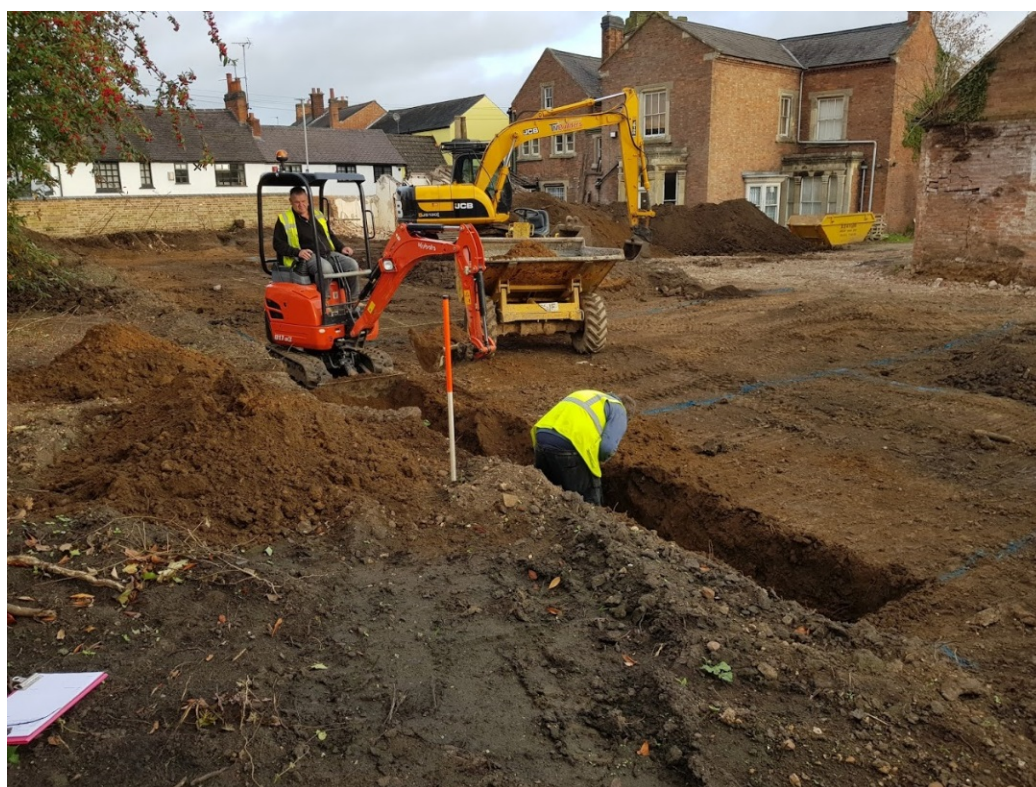
Figure 7: Visit 2. Work began excavating the trenches for the foundations on the marked out areas. The ground proved to be very hard in places.
