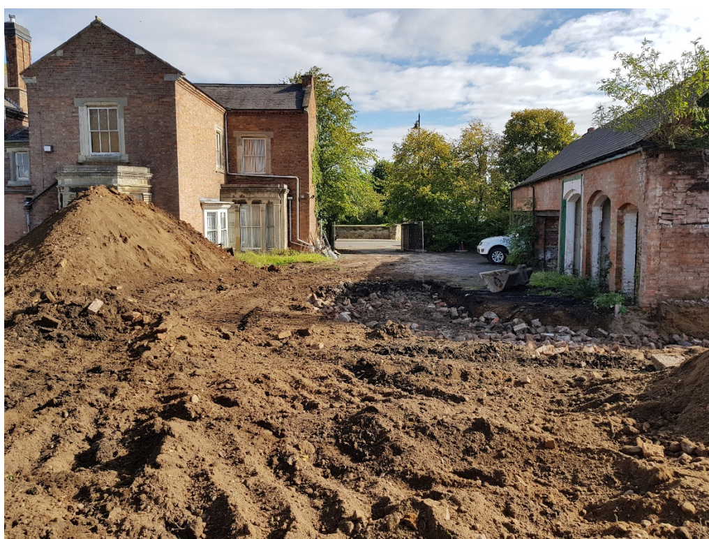
Figure 4: Visit 1. Looking east towards the front entrance. The area which had been excavated and filled with hard-core rubble is visible.
