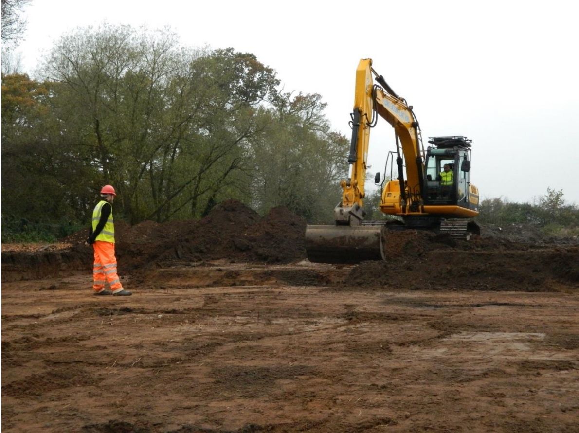
Figure 2: View of the machining underway, removing the topsoil to create an open-area excavation
