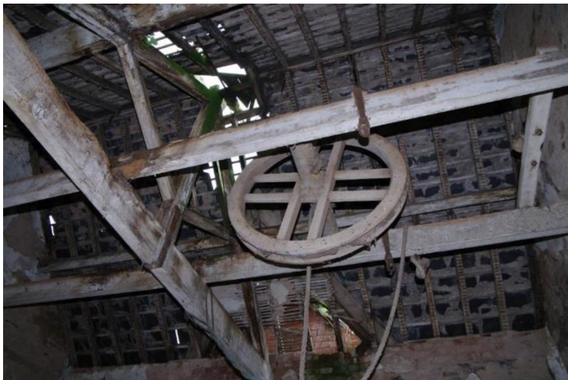
Figure 37 Building B north room, pulley wheel in roof Also note remnants of laths and plaster on the underside
