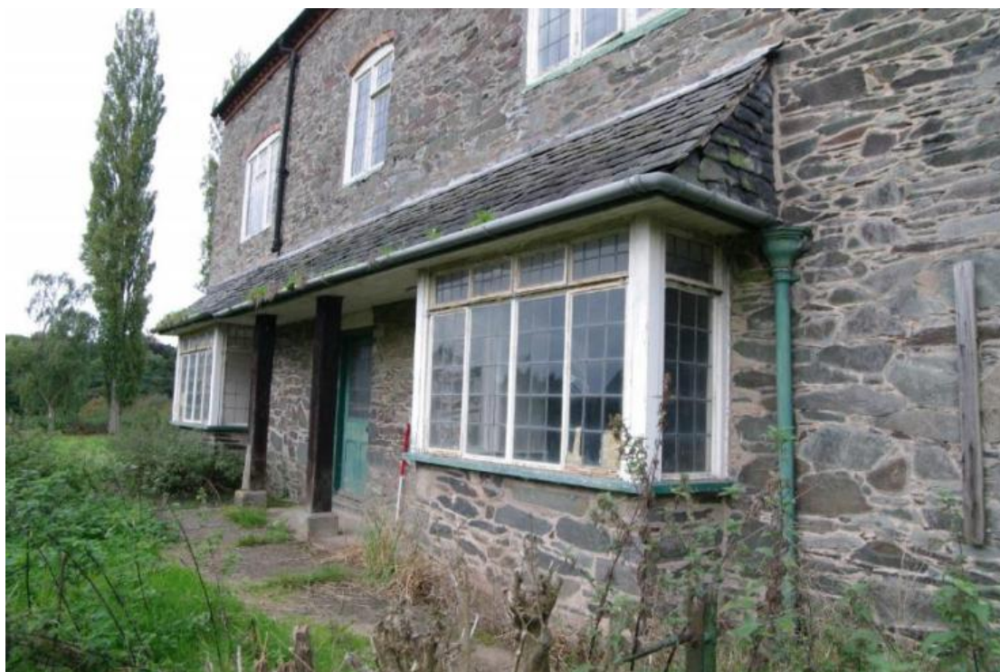
Figure 100 Main House east-facing elevation ground floor bay windows Looking south-west. 1m scale
