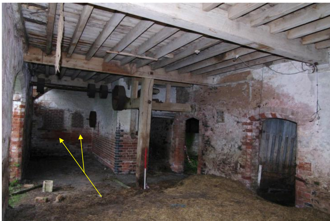
Figure 31 Building B ground floor south room Looking north-east. 1m scale. Blocked windows on north wall shown with arrows
