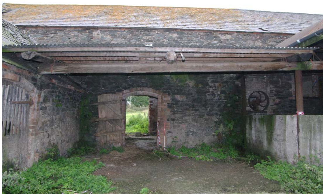
Figure 25 Building B south end of east-facing elevation Looking west. 1m scale. Building C on left
