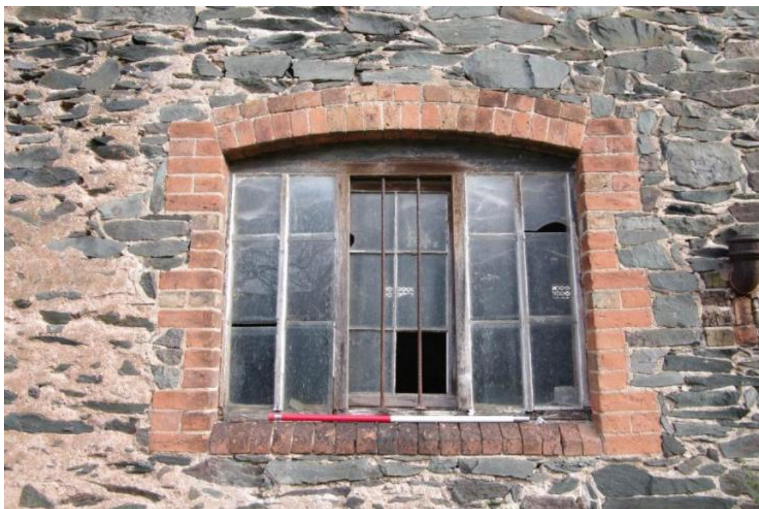
Figure 71 Building F south facing elevation ground floor window detail Looking north. 1m scale
