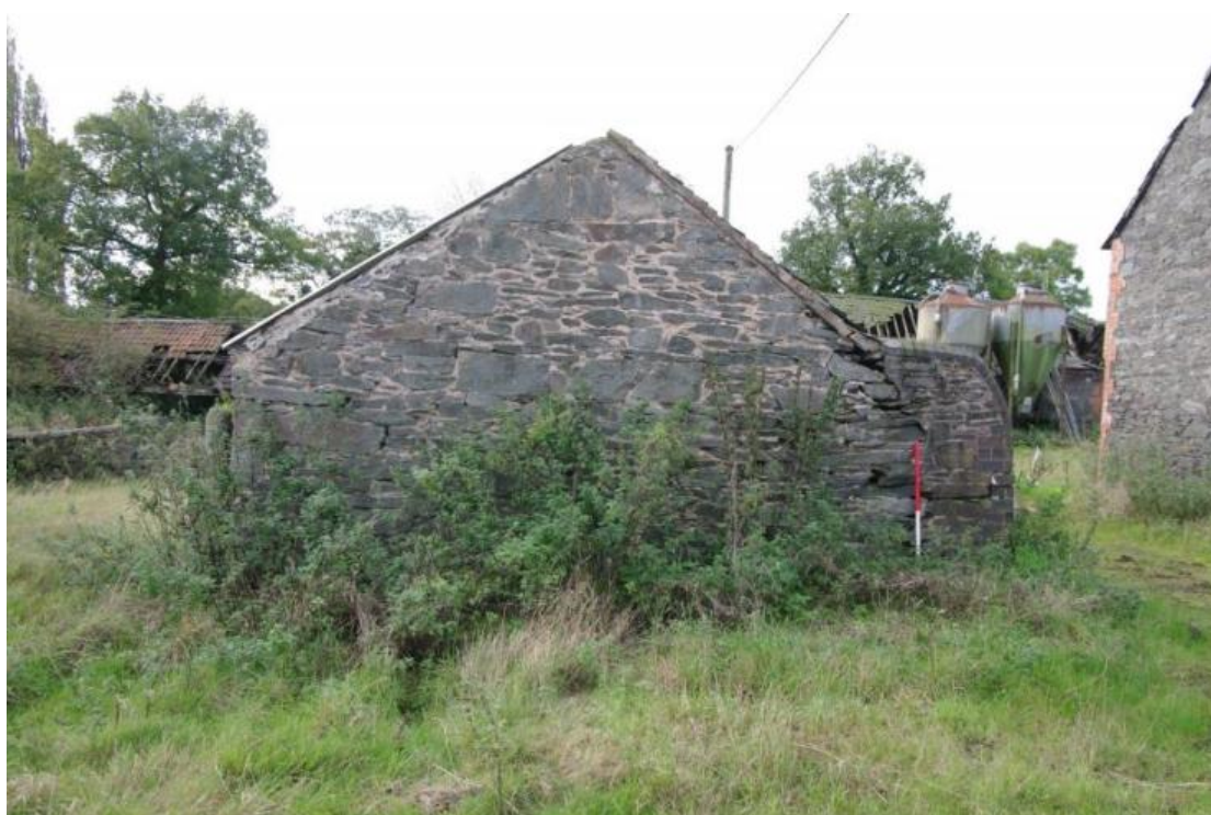
Figure 52 Building D north facing gable end Looking south. 1m scale. Gable end of Building A on right
