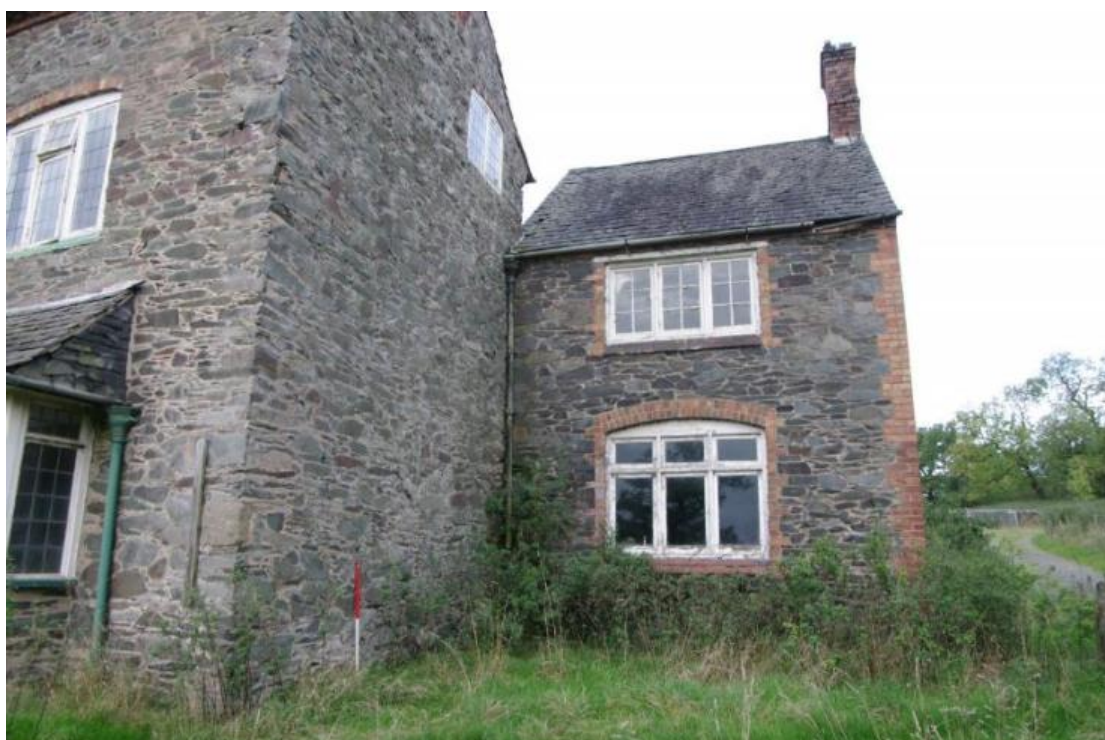
Figure 103 East-facing elevation of extension on north-west corner of house Looking south-west. 1m scale
