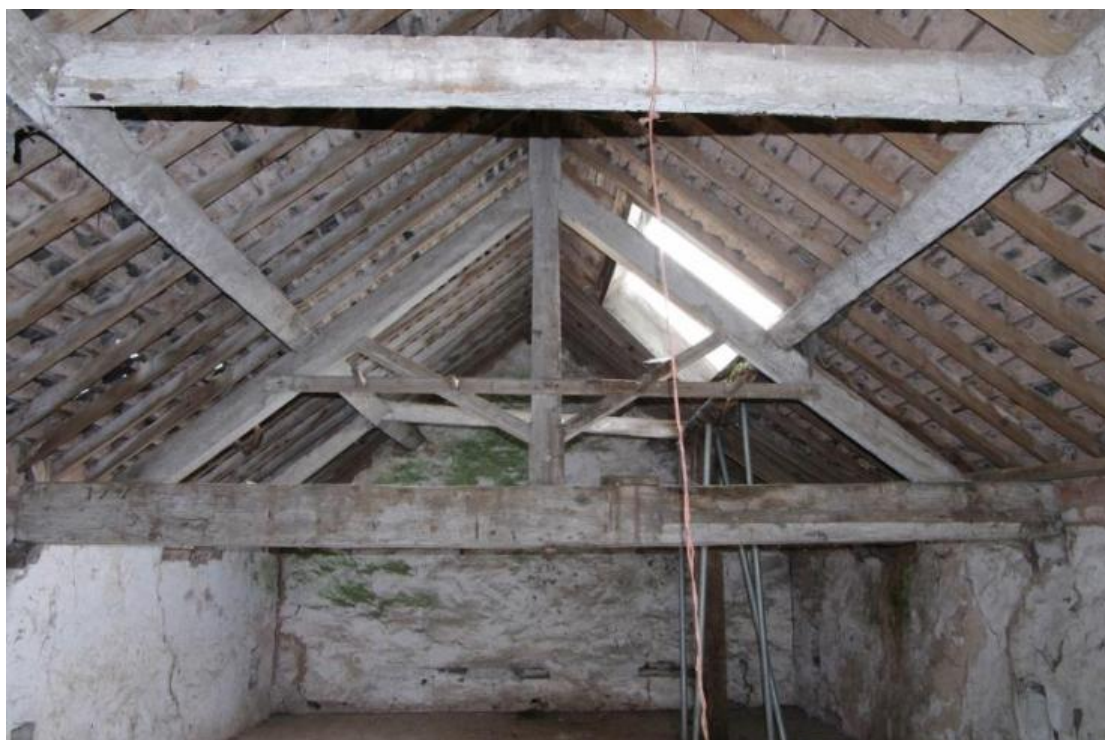
Figure 74 Building F first floor and roof detail Looking east. Note saddle tree attached to centre post
