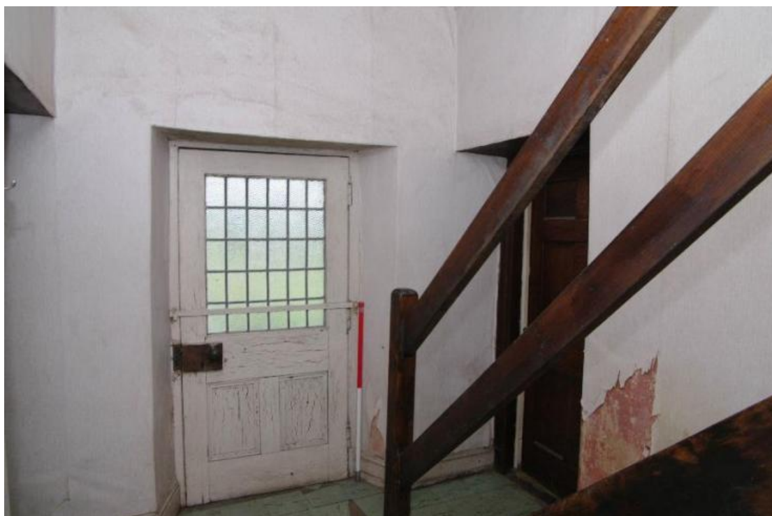
Figure 121 Front door in hall Looking south-east. 1m scale. Door to Room 8 on right
