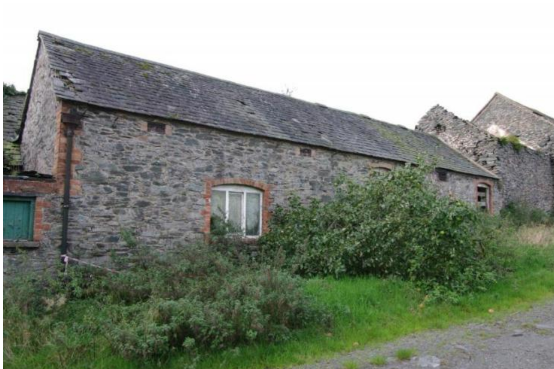
Figure 76 Building G north-facing elevation Looking south-west. Building F on far right of picture
