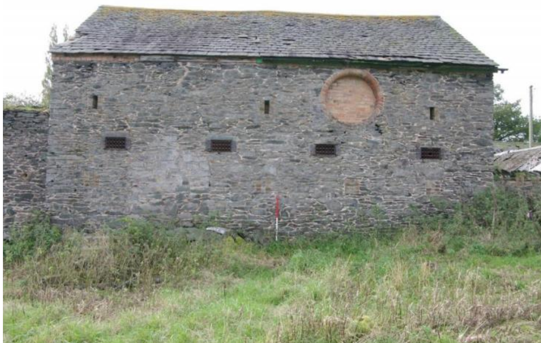
Figure 66 Building F north-facing elevation Looking south. 1m scale. Note blocked vents at ground floor level
