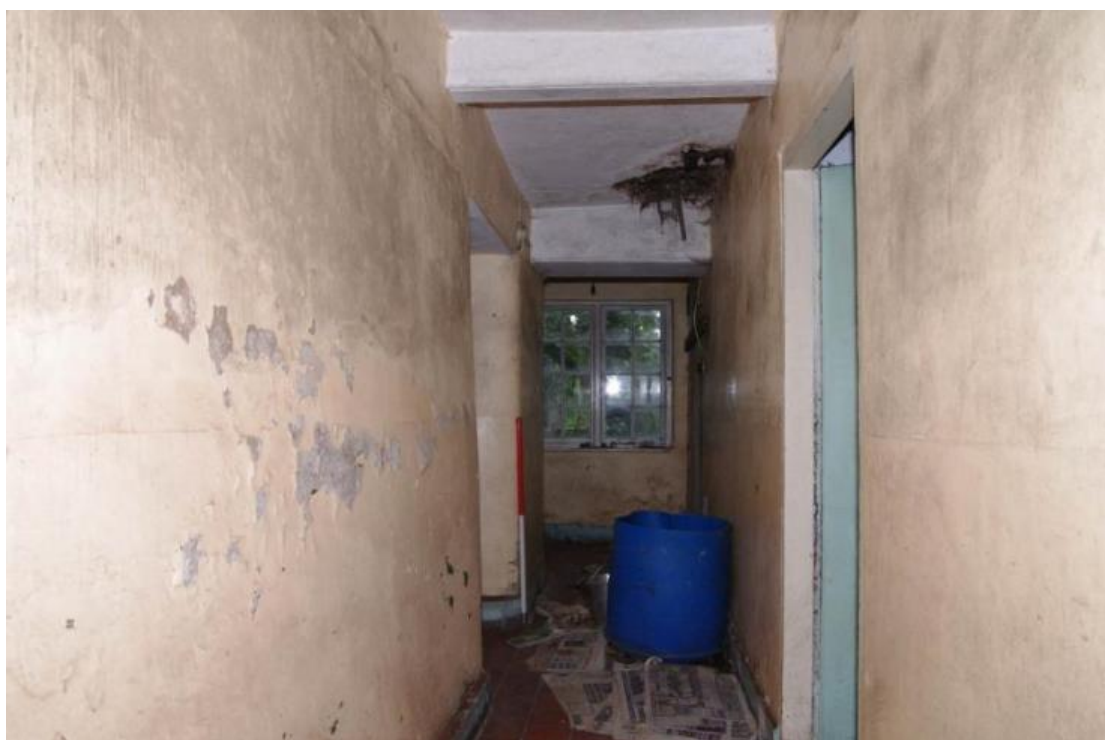
Figure 115 Room 6 corridor on west side of house Looking south. 1m scale. Outside door to right of window. Access to house on left
