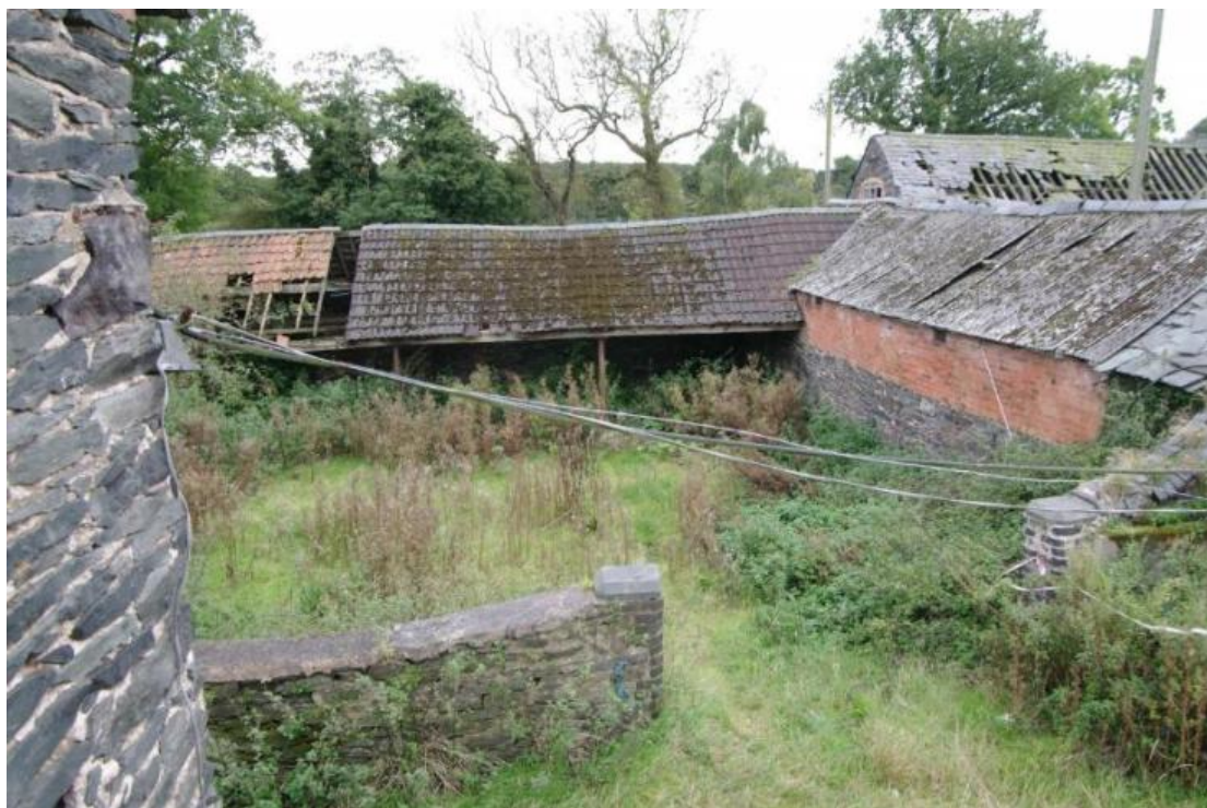
Figure 58 View of east yard Looking south-east towards Building E. Building F on left, D on right
