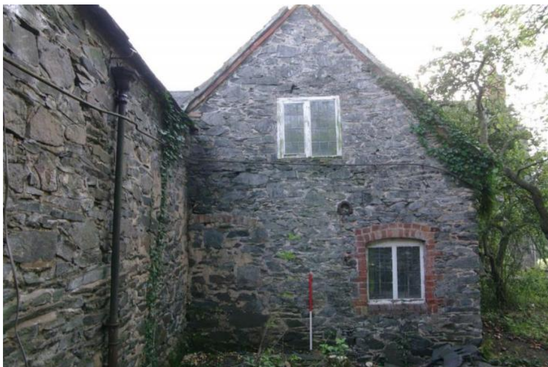
Figure 107 West-facing elevation of buildings attached to rear of main house Looking east. 1m scale. Note blocked window to left of scale
