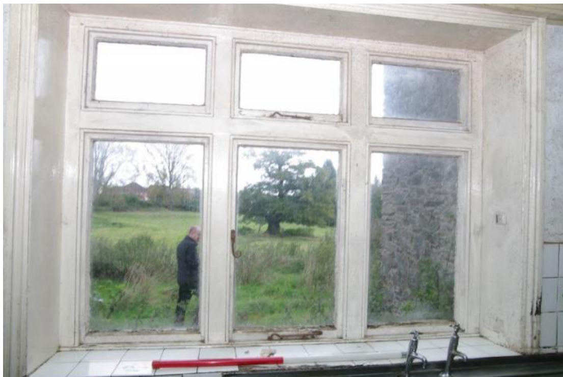
Figure 114 Room 5 window detail Looking east. 1m scale. North facing gable of main house can be seen through window
