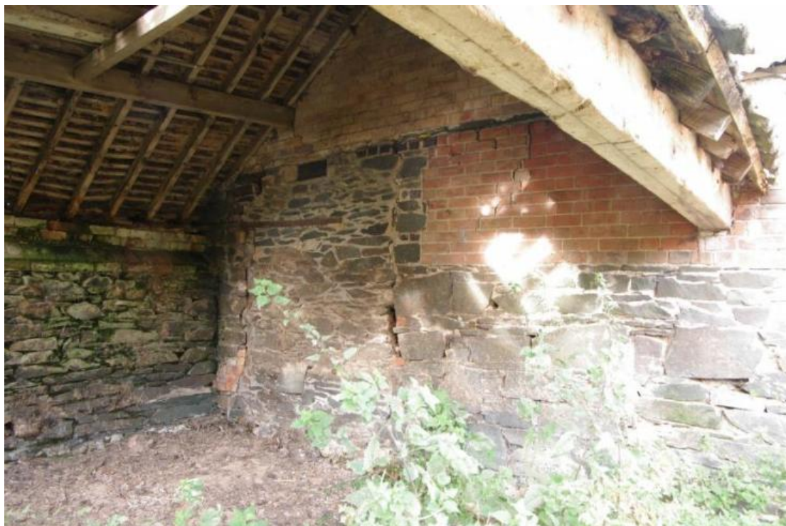
Figure 55 Building D east-facing elevation, south end inside Building E Looking south-west. South wall of Building E on left
