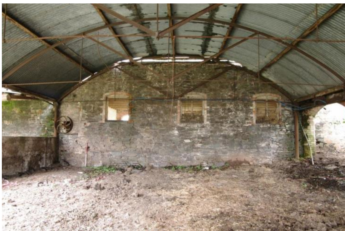
Figure 26 Building B north end of east-facing elevation Looking west. 1m scale. Building A on right. Note drive wheel extending out from a blocked window
