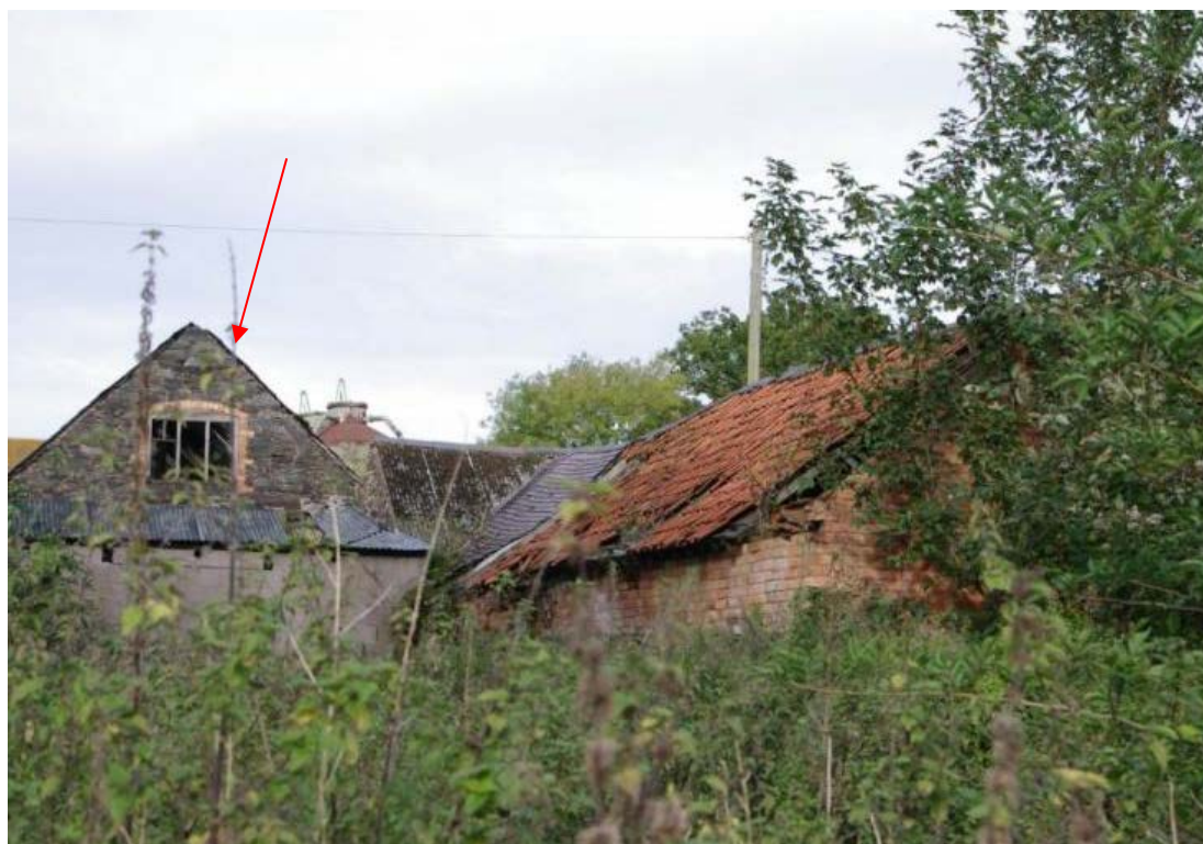
Figure 43 Building C east facing gable end Looking west. Building C arrowed. Note modern lean-to built against gable end. Pan tiles of Building E on right
