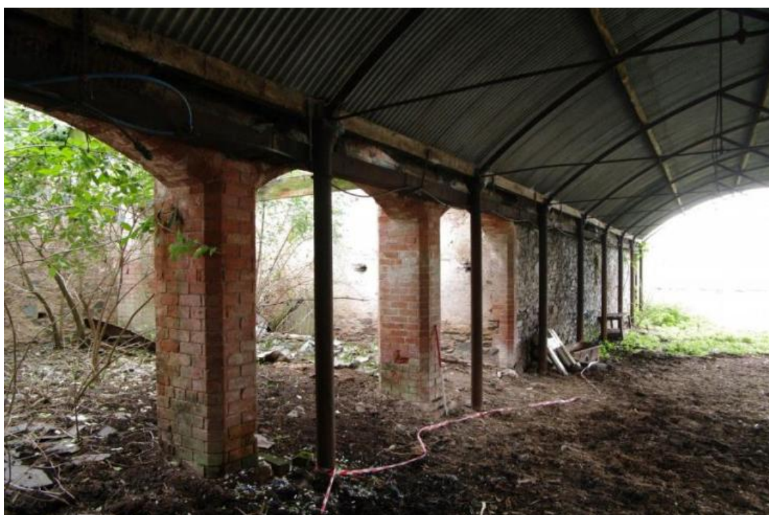
Figure 16 Building A south-facing elevation Looking north-east. 1m scale. Building A has no roof at this point hence the trees growing inside. Photo taken from inside the open barn filling the yard space
