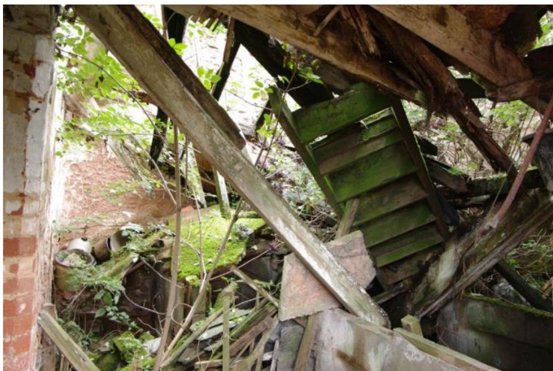
Figure 83 Inside western end of Building G Looking north-east from doorway. Note wooden stairs within collapsed material
