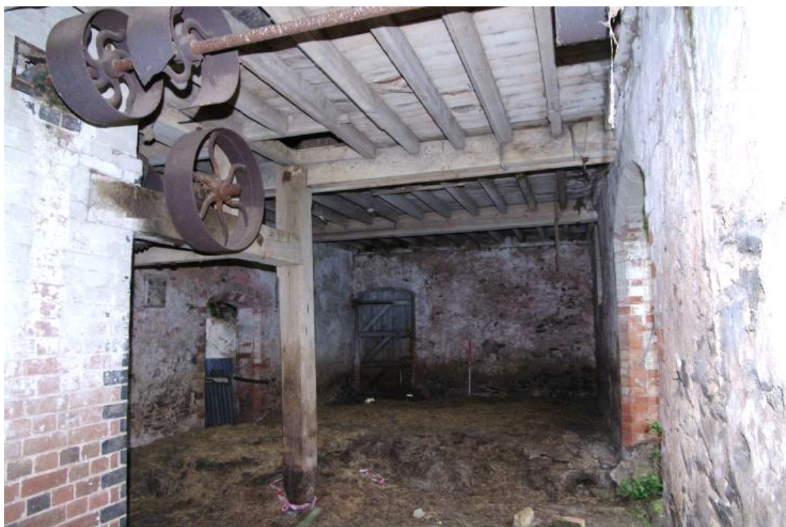
Figure 27 Building B ground floor south room Looking south. 1m scale. Door on left leads in Building C, far door leads outside to south-facing elevation. Door on right leads to west-facing elevation
