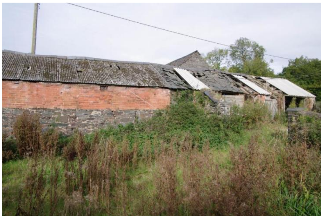
Figure 54 Building D east-facing elevation Looking north-west. Gable of Building A can be seen above the ridgeline of D
