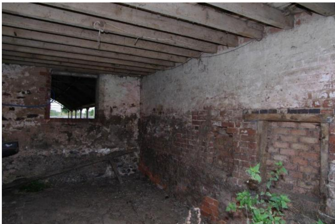
Figure 33 Building B room north of southern room Looking east. Blocked windows into south room on right
