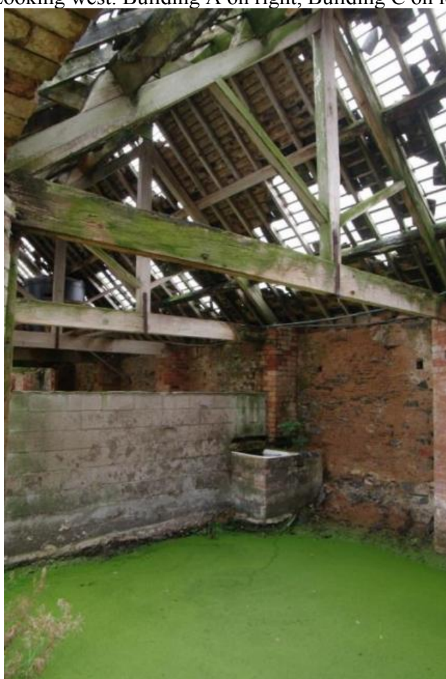
Figure 18 Inside Building A Looking south-east. Note later inserted dividing wall and trough plus the flooded floor
