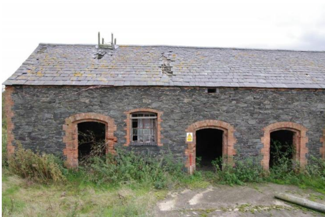
Figure 20 Building B north end of west-facing elevation Looking east. 1m scale. Note remnant of roof vent on ridge
