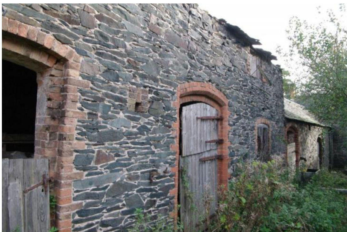
Figure 78 Building G south facing elevation Looking north-east. Note joint in stonework above doorway
