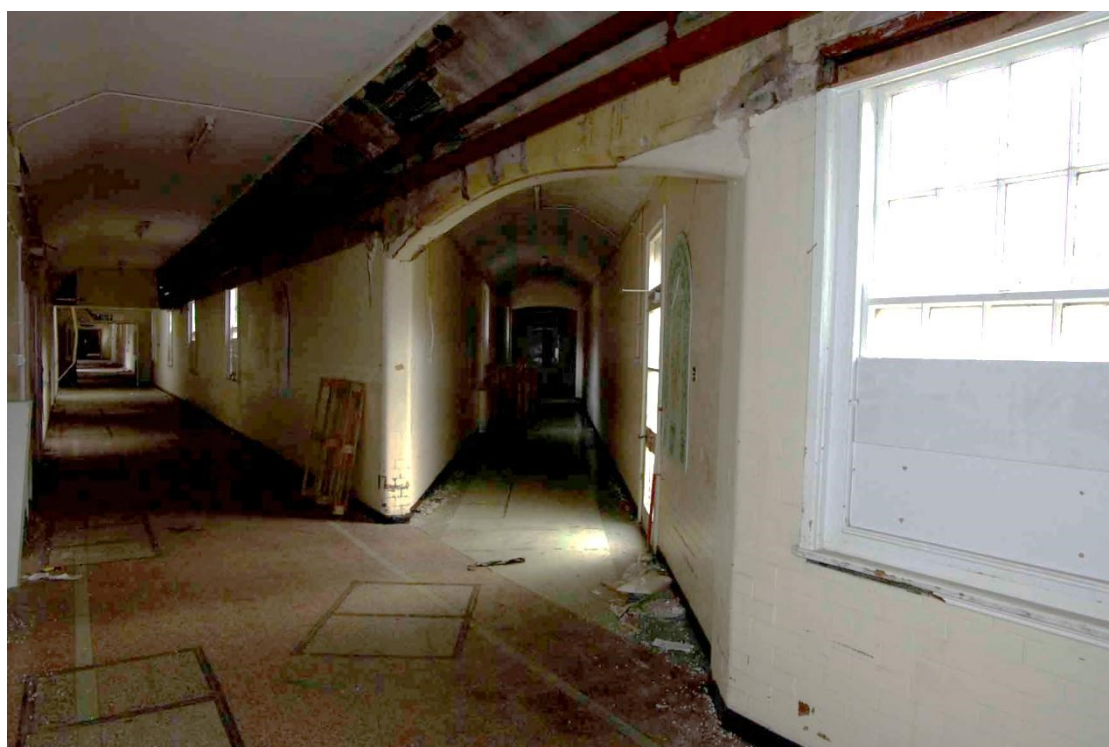
Figure 42 Main corridor and angled junction to the Daisy Peake Building Looking south-east. Main corridor on left of picture
