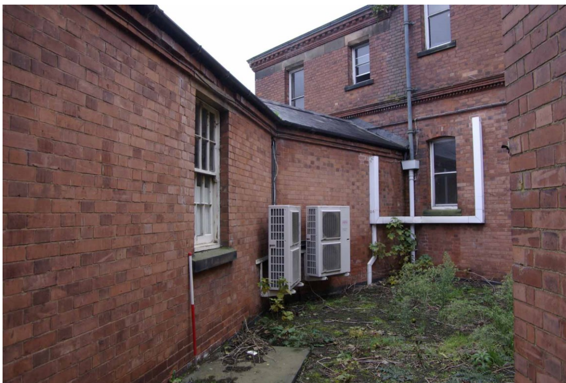
Figure 25 South facing elevation of main corridor at eastern end Looking north-east, 1m scale. The two storey building is the east end of the Daisy Peake Building.
