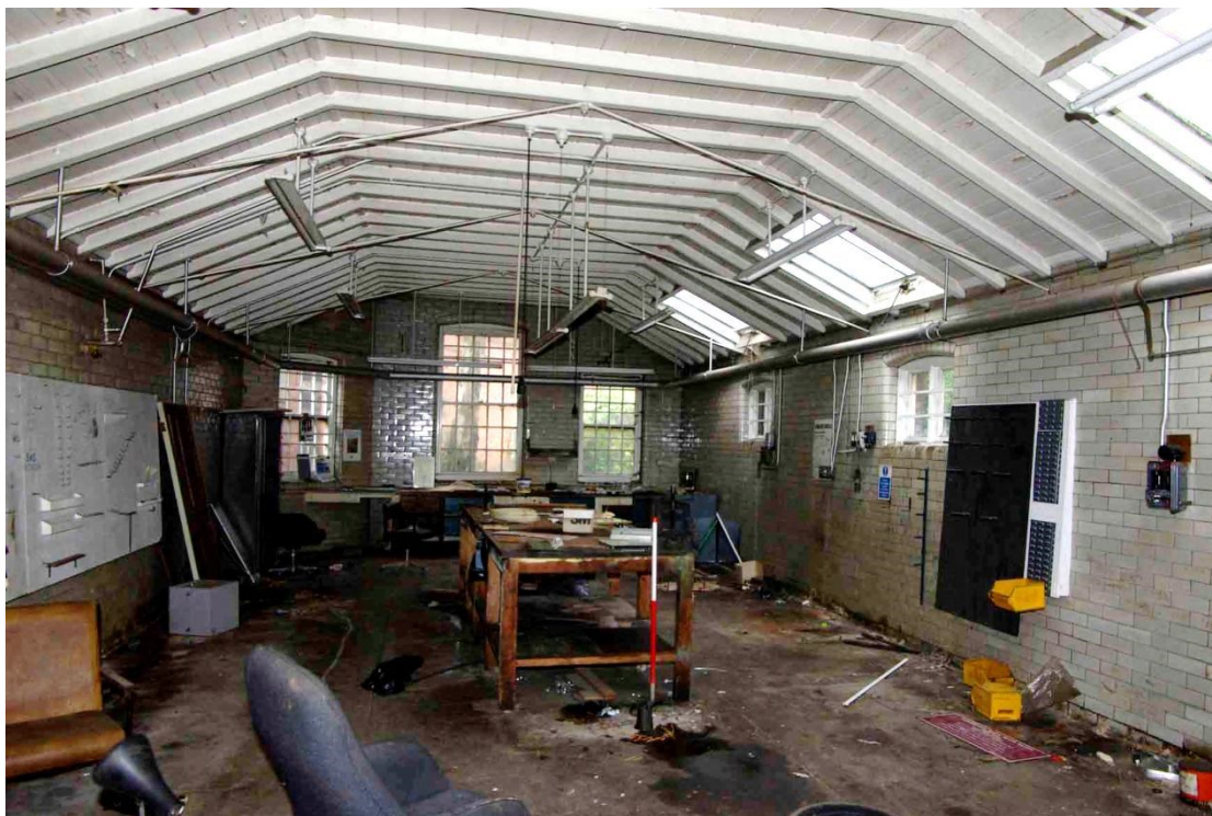
Figure 75 Accumulator room GF9 Looking west, 1m scale. Note angled corner in south west corner
