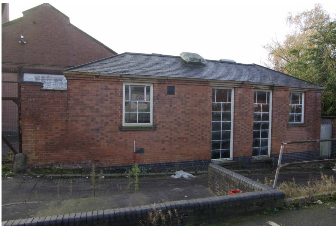
Figure 76 Building (pump room?) at north end of engineering workshop Looking south, 1m scale
