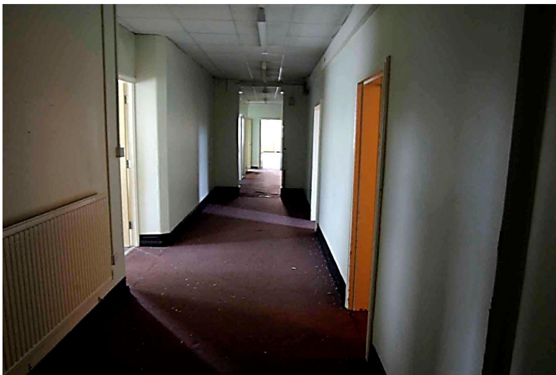
Figure 100 Ground floor corridor into Daisy Peake Building at east end Looking north. Note chamfered door jambs on left leading into former conservatory
