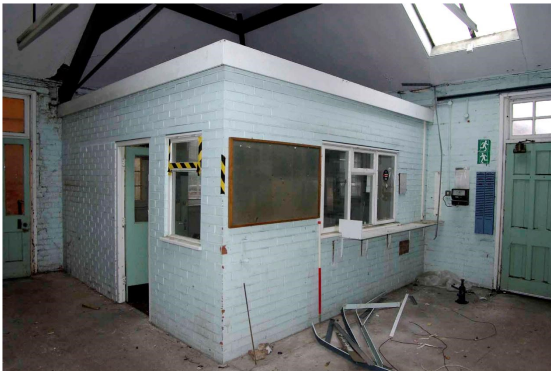
Figure 73 Inserted office at north end of engineering workshop Looking north-west, 1m scale. Door to accumulator room on left
