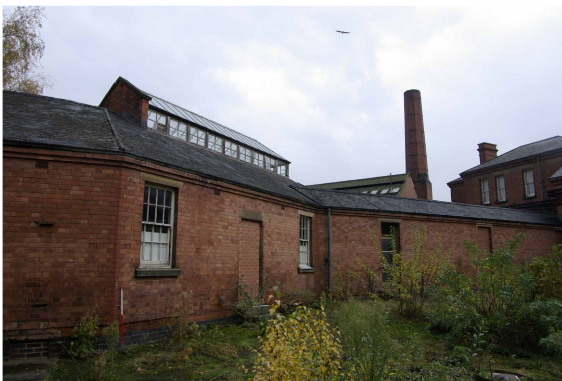
Figure 28 South facing elevation of main corridor to west of angled corridor to Daisy Peak Building Looking north-east, 1m scale.
