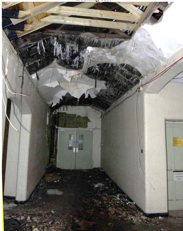
Figure 21 Main corridor to north of recreation hall Looking north west. East corridor of food processing area to right of picture
