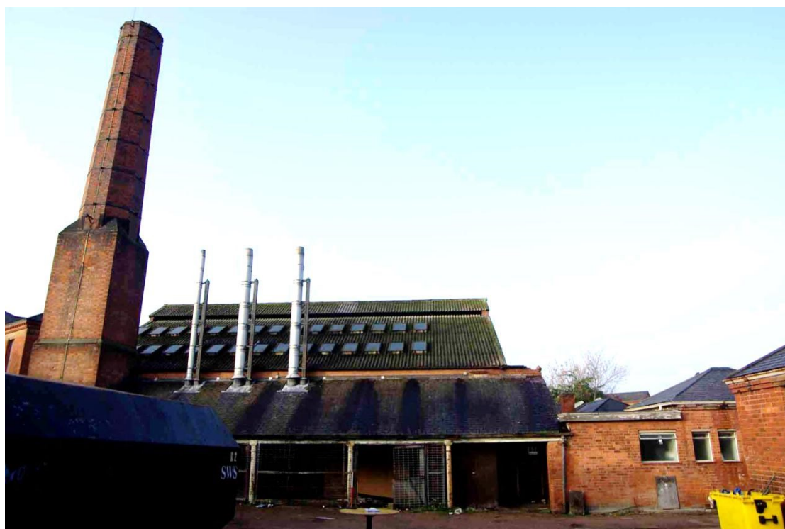
Figure 68 Boiler house east facing elevation Looking west, 1m scale. Washroom to right of lean-to. WS3 on extreme right of picture.
