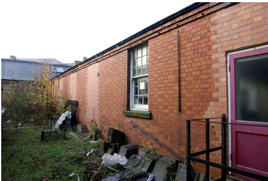
Figure 56 East facing elevation of WS2 Looking south-west, 1m scale. Note blocked windows. Outside wall of Room GF7 on left of photo
