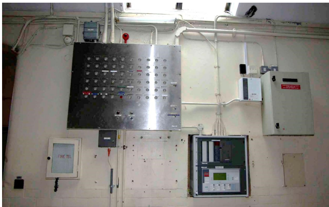
Figure 45 Fire alarm and control panel on main corridor Looking north
