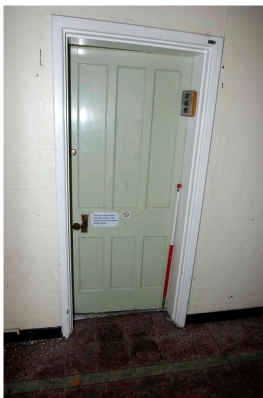
Figure 47 Doorway to Room GF1, Director of Nursing's room Looking south-west, 1m scale
