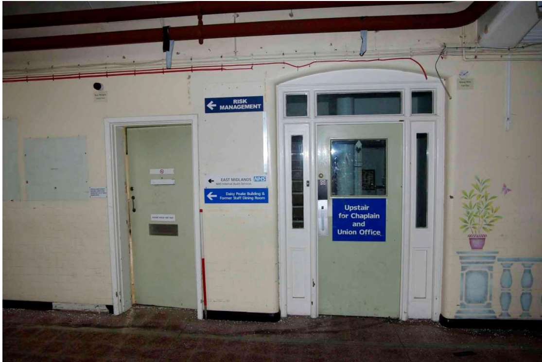
Figure 50 Doors from main corridor to GF2 and stairs Looking south-west, 1m scale
