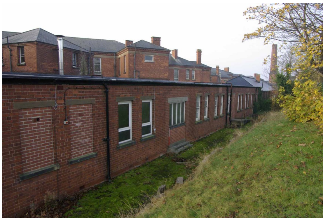
Figure 33 North facing elevation of WRVS canteen Looking south-west, 1m scale. Blocked doorway and steps are to the right of the ranging pole
