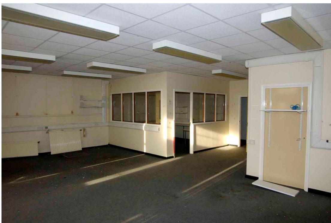
Figure 101 De Montfort ward dayroom Looking north-west, 1m scale. Inserted rooms centre and right
