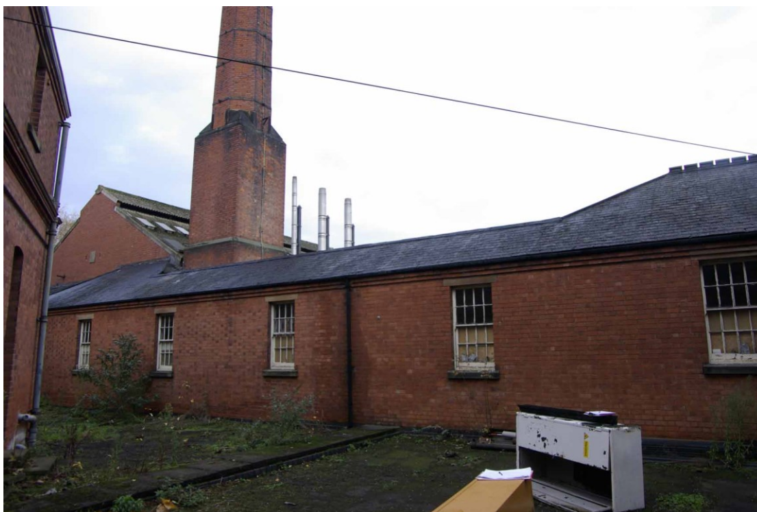
Figure 27 South facing elevation of main corridor east of boiler house Looking north-west. Photo taken on opposite side of corridor to Fig. 24
