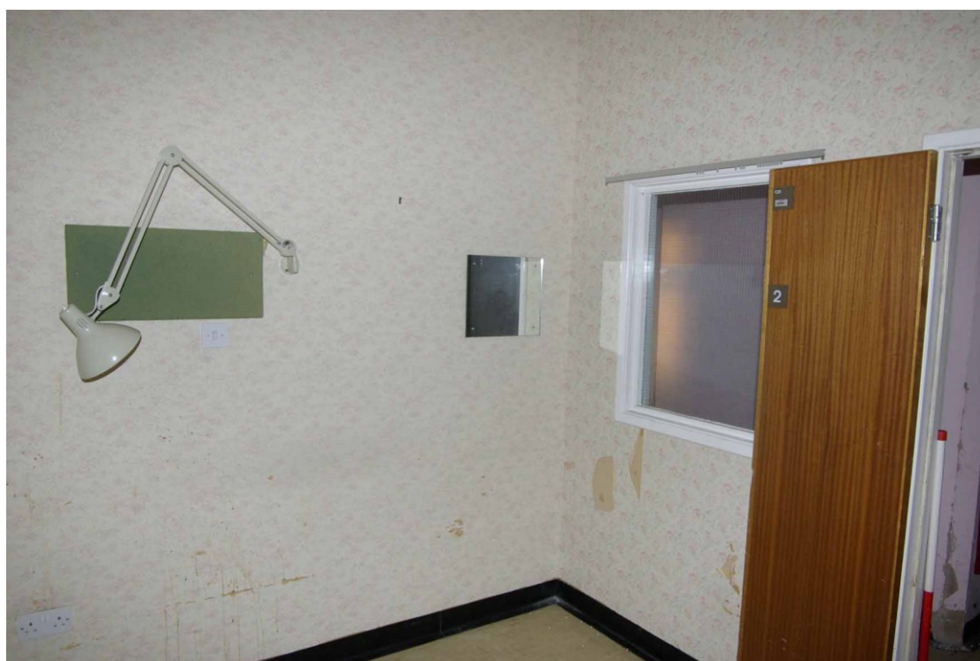
Figure 114 Interior view of an inserted room in the Cropston ward Looking north-west, 1m scale
