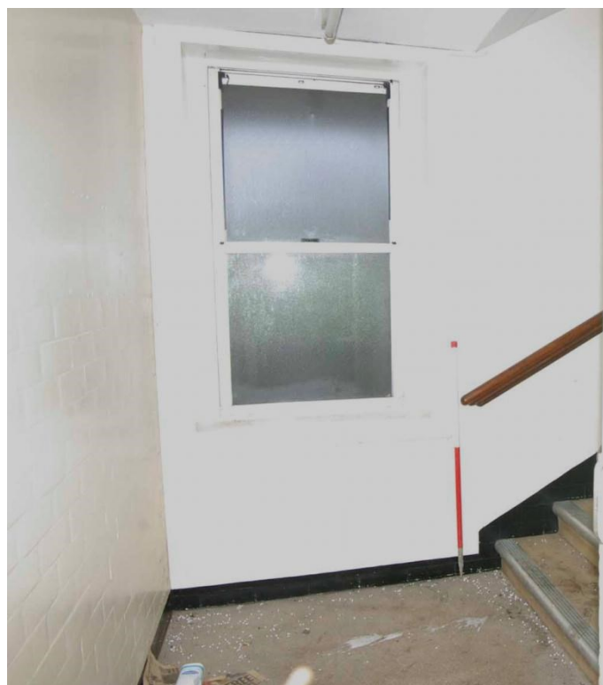
Figure 30 Stairs from east end of main corridor up to Daisy Peake Building Looking north, 1m scale. Note painted over wall tiles and modernised sash window
