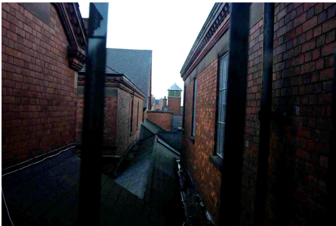
Figure 120 Passive ventilator seen from first floor of Daisy Peake Building Looking west over main corridor roof. Recreation hall gable end is in centre of photo
