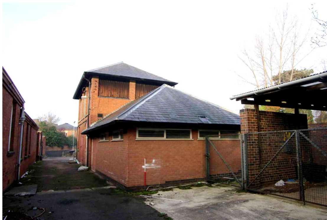
Figure 64 Single storey building attached to eastern side of WS4 Looking north-west, 1m scale. Workshop WS3 on left of photo
