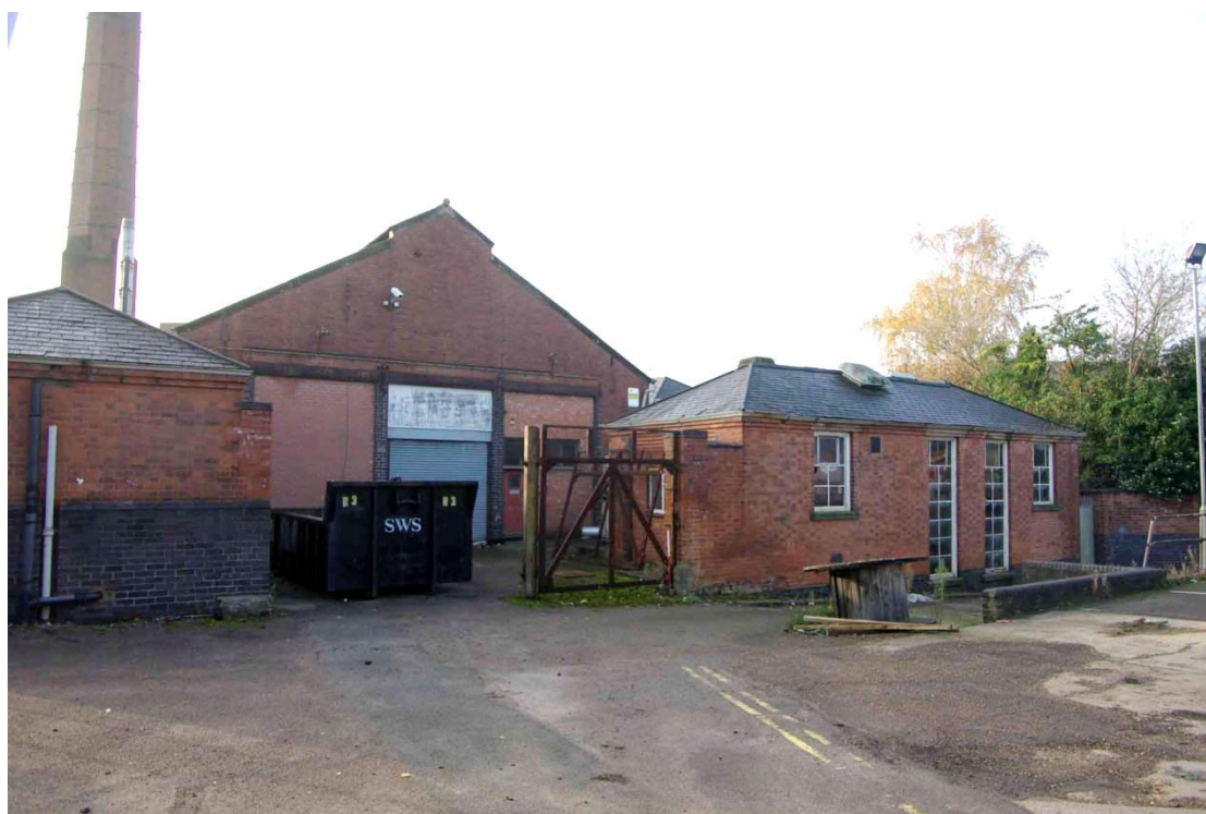
Figure 69 Boiler house north facing elevation Looking south-west, 1m scale. Note north wall of washroom on left of picture
