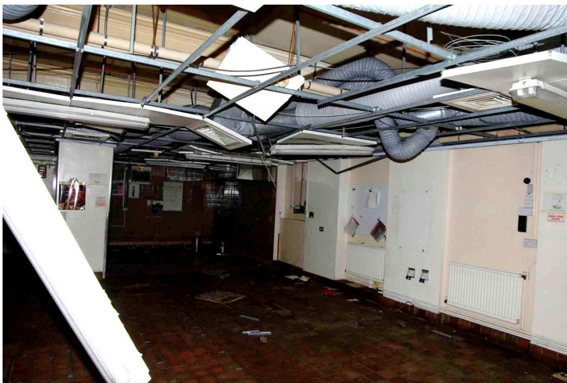
Figure 78 Staff cafeteria Looking north-east, 1m scale. Note moulded beams above false ceiling
