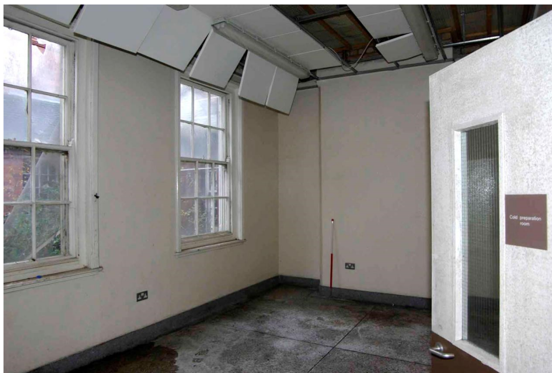
Figure 88 Cold food preparation room GF20 Looking south-west, 1m scale. Windows look out into enclosed light well courtyard
