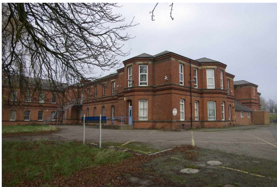
Figure 89 Eastern end of Daisy Peake Building. De Montfort and Newarke wards Looking north-west. Note ground floor infilled entrance on right of picture. Fosse and Belgrave wards on left of photo. Lift shaft mechanism on extreme right of buildings
