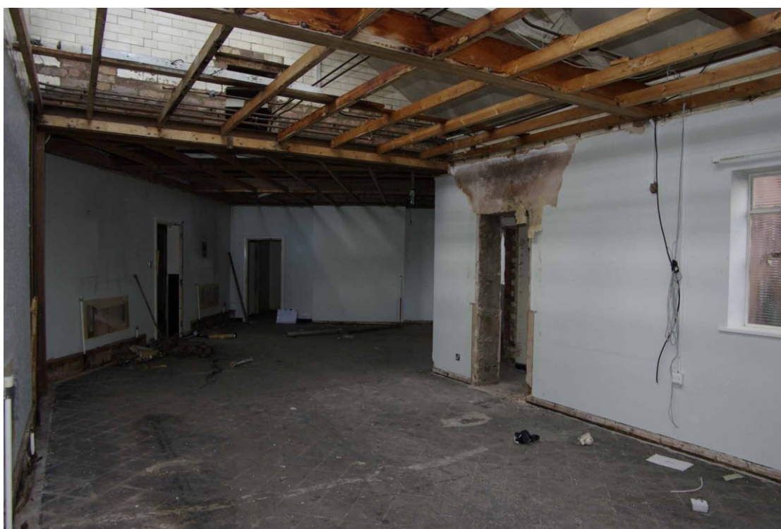
Figure 40 Room GF10 Looking north west, 1m scale. Knocked through wall was located at the end of the false ceiling
