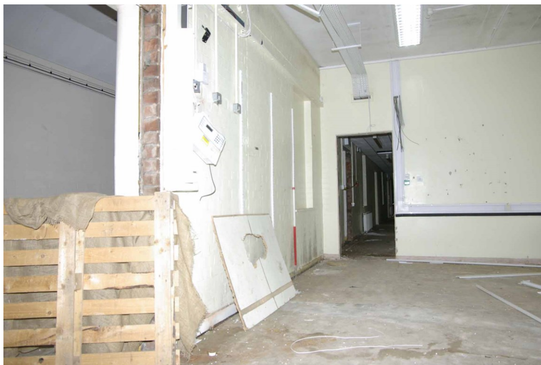
Figure 31 Original outside north wall of main corridor Looking south west, 1m scale. Blocked window can be seen to right of ranging pole. Photograph taken in the WRVS canteen looking towards the plasterboard partitions of the 1940s extension. Doorway to main corridor on extreme left of picture
