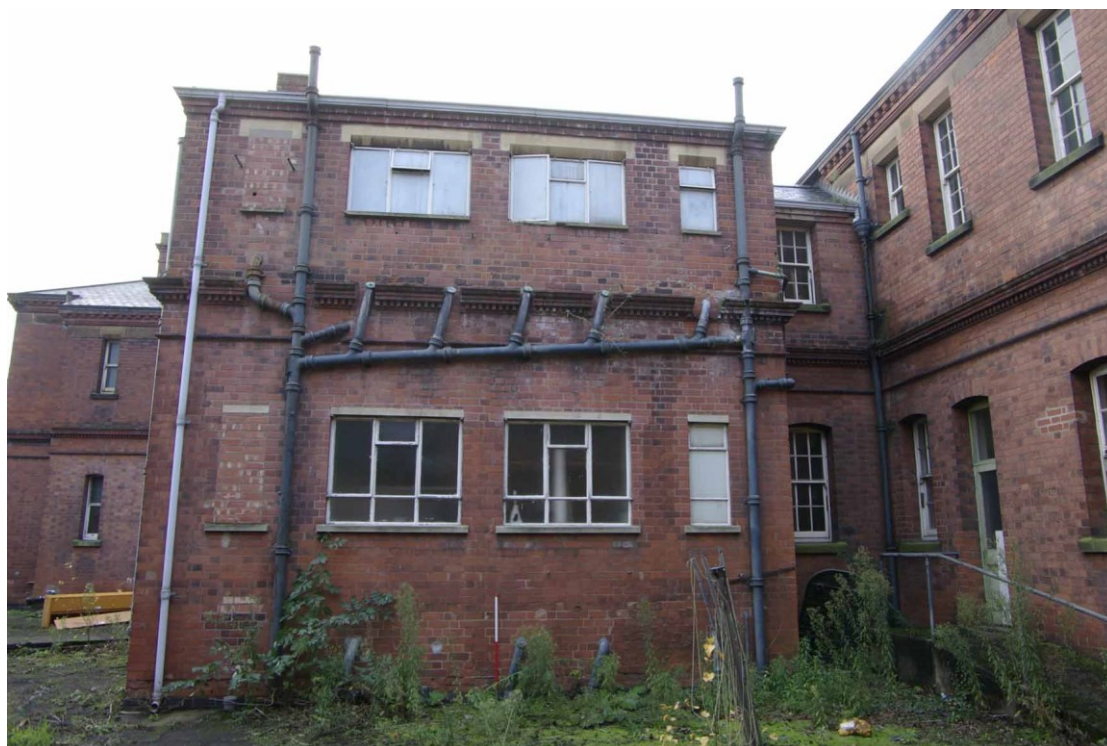
Figure 97 Toilet block behind Grace Dieu and Fernie wards Looking east, 1m scale
