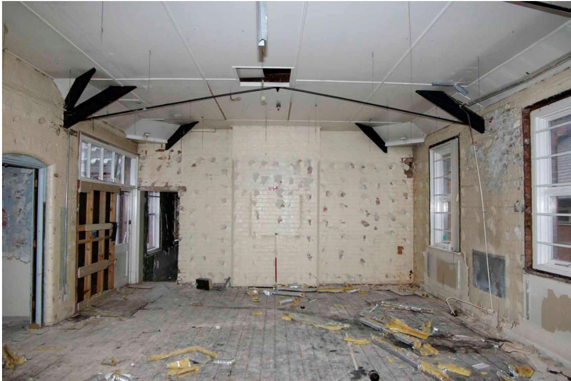
Figure 60 East end of workshop WS3 Looking west, 1m scale. Doorway to western part of WS3 to left of chimney breast
