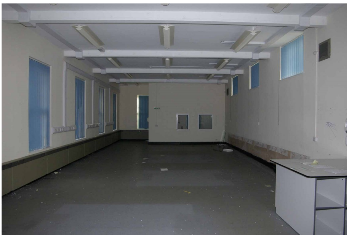
Figure 111 Beaumanor ward (west) Looking south-east. Note high windows on right above blocked veranda
