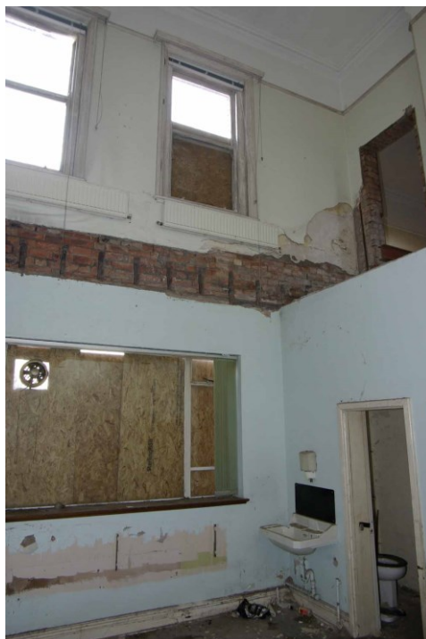
Figure 52 Room GF4 ground and first floors Looking south-west through hole in sealed doorway
