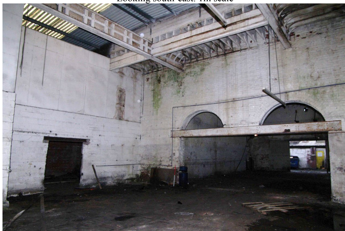
Figure 66 Room G5 Looking north-west into booking hall G6. 1m scale. Modern inserted wall on left. Compare the truncated arches with the 1967 view in Figure 32 above
