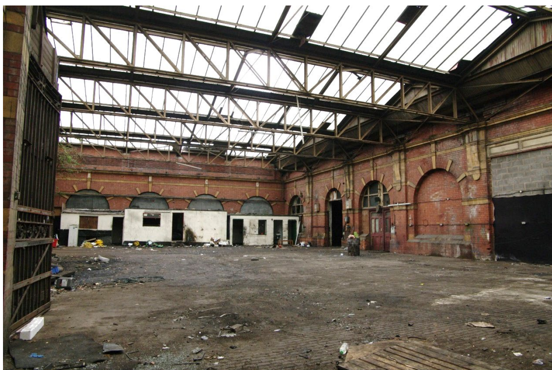
Figure 42 Portico area G7 Looking south. Blocked entrance to booking hall (G5) on right
