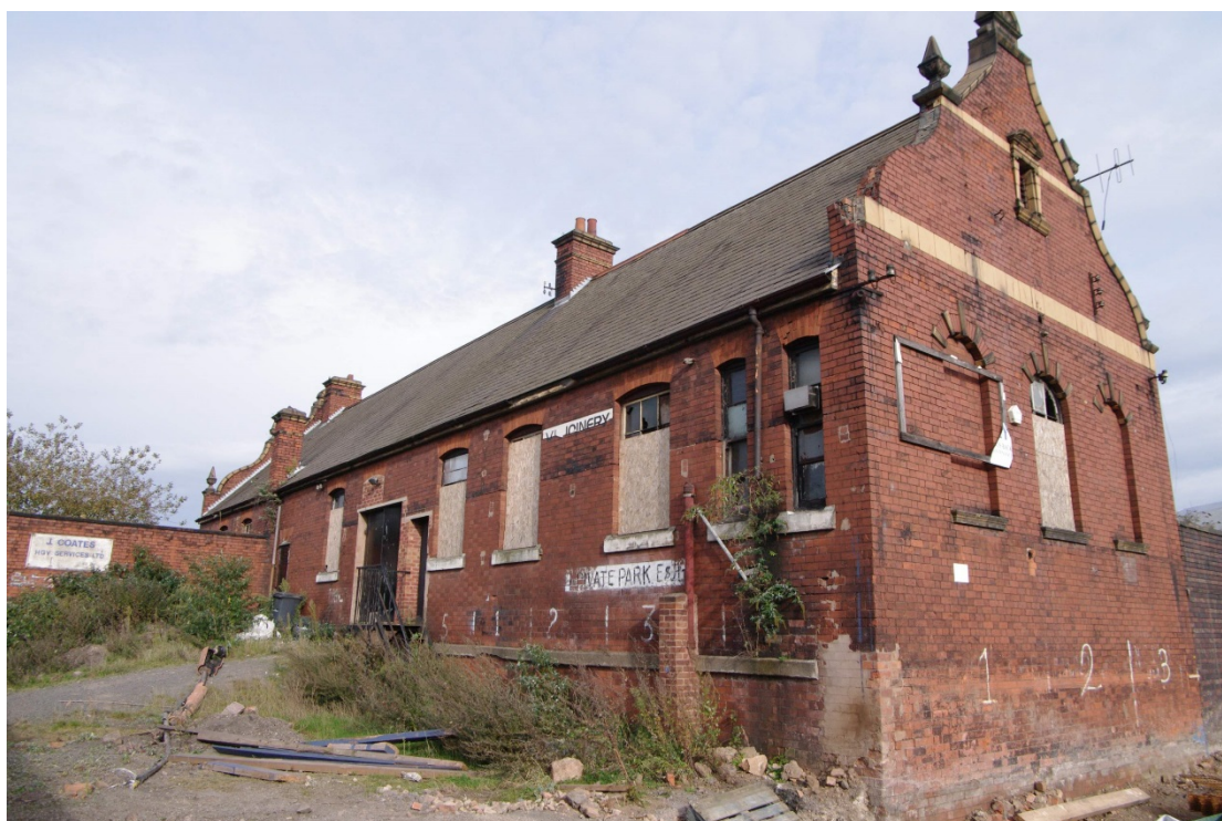
Figure 99 Parcels office west-facing elevation, south end Looking north-east. The cement line beneath the painted numbers represents the former platform level
