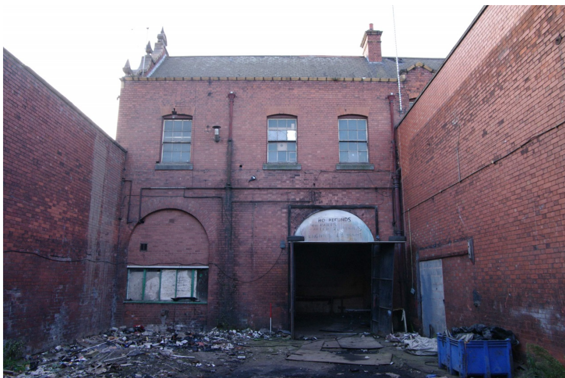
Figure 91 Parcels office east-facing elevation seen from parcels yard Looking west towards entrance to G8. 1m scale
