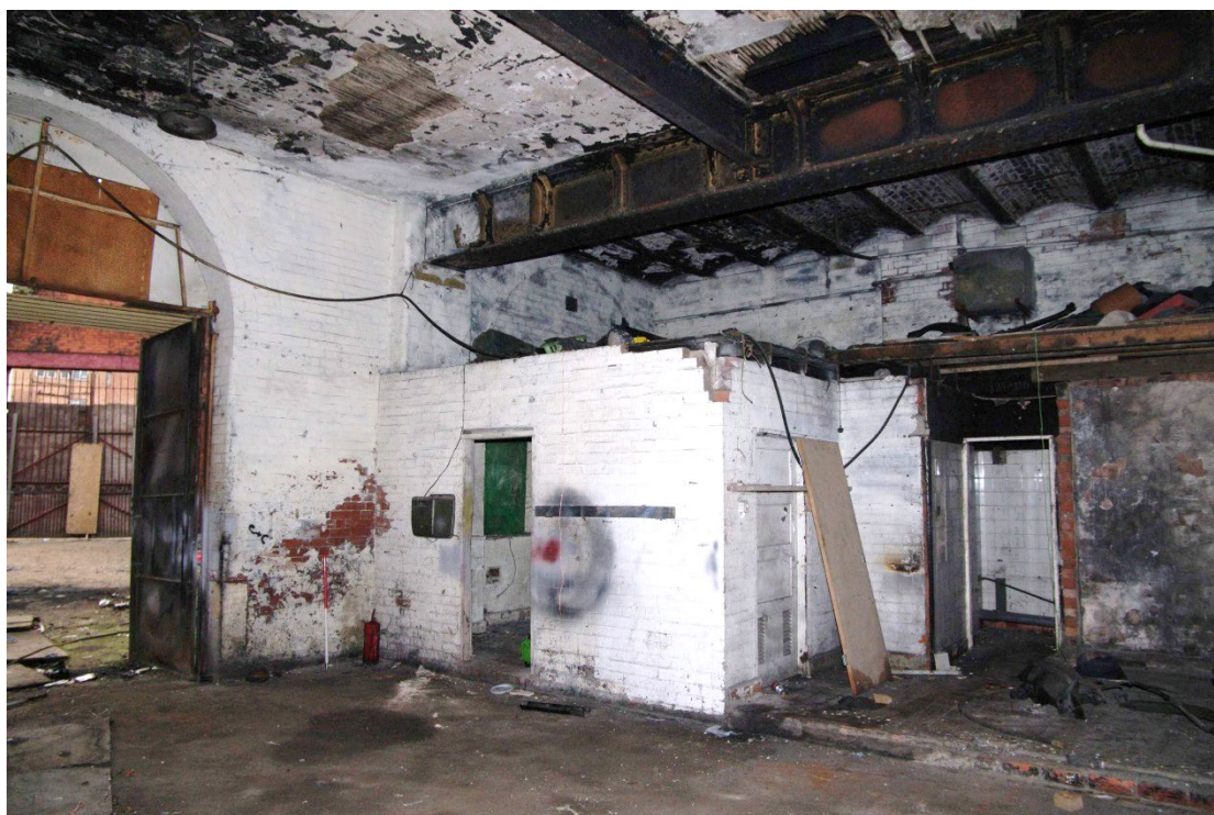
Figure 73 Parcels office ground-floor Room G8 Looking south-east. 1m scale. Parcels yard on left. Note vaulted brick ceiling on right
