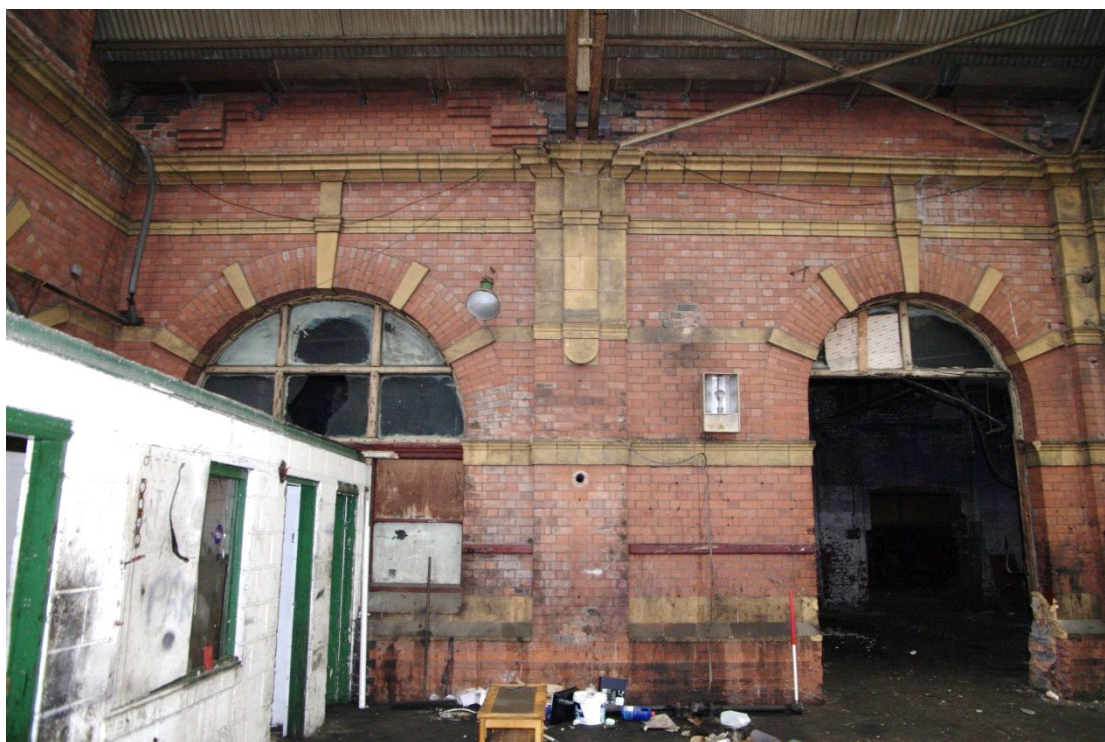
Figure 47 Portico area G7 west wall, southern end bays, entrances to G9. Looking west. 1m scale. Note partially smashed masonry at base of opening to right of scale
