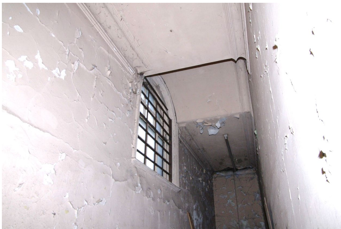
Figure 106 Parcels office Room F1 window and ceiling Looking north-east. Note moulded cornice details
