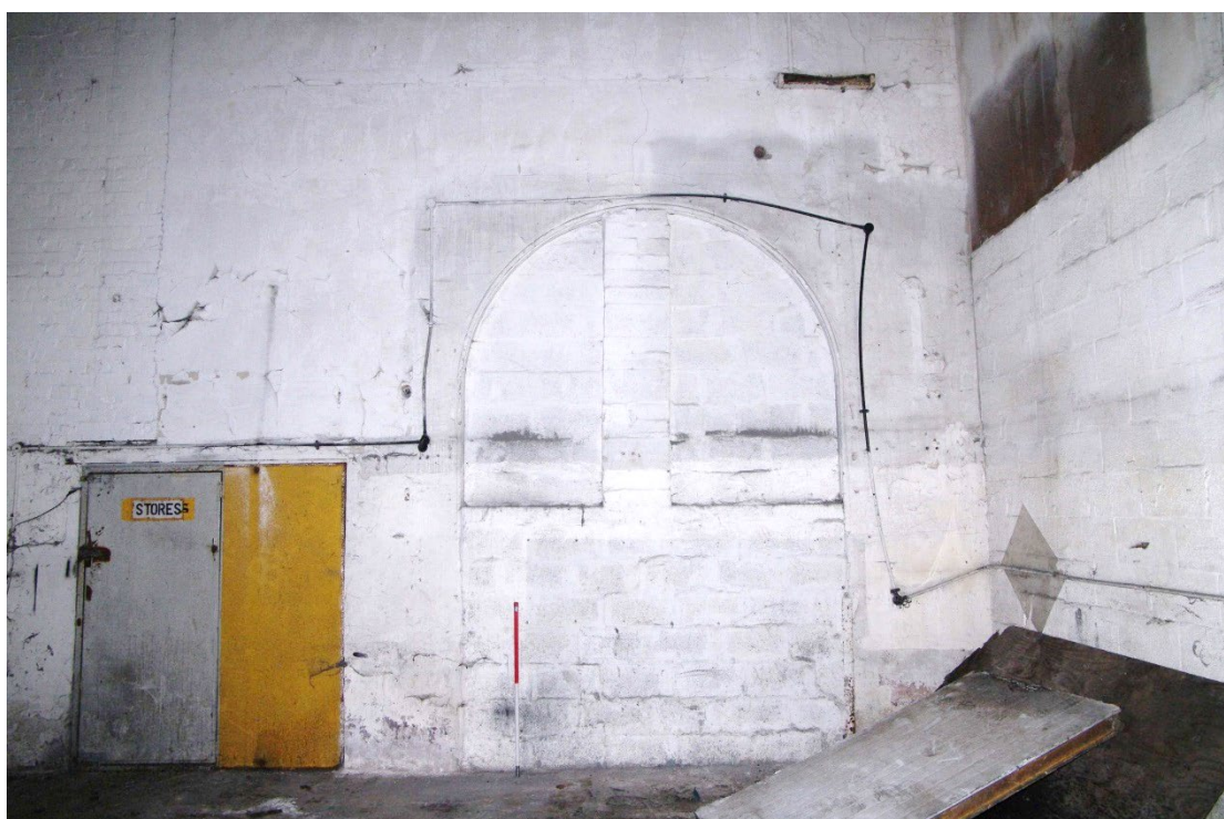
Figure 68 Room G5, blocked archway to G9 on south wall Looking south. 1m scale. Door on left leads to a space beneath the parcels office stairs. Modern inserted wall on right
