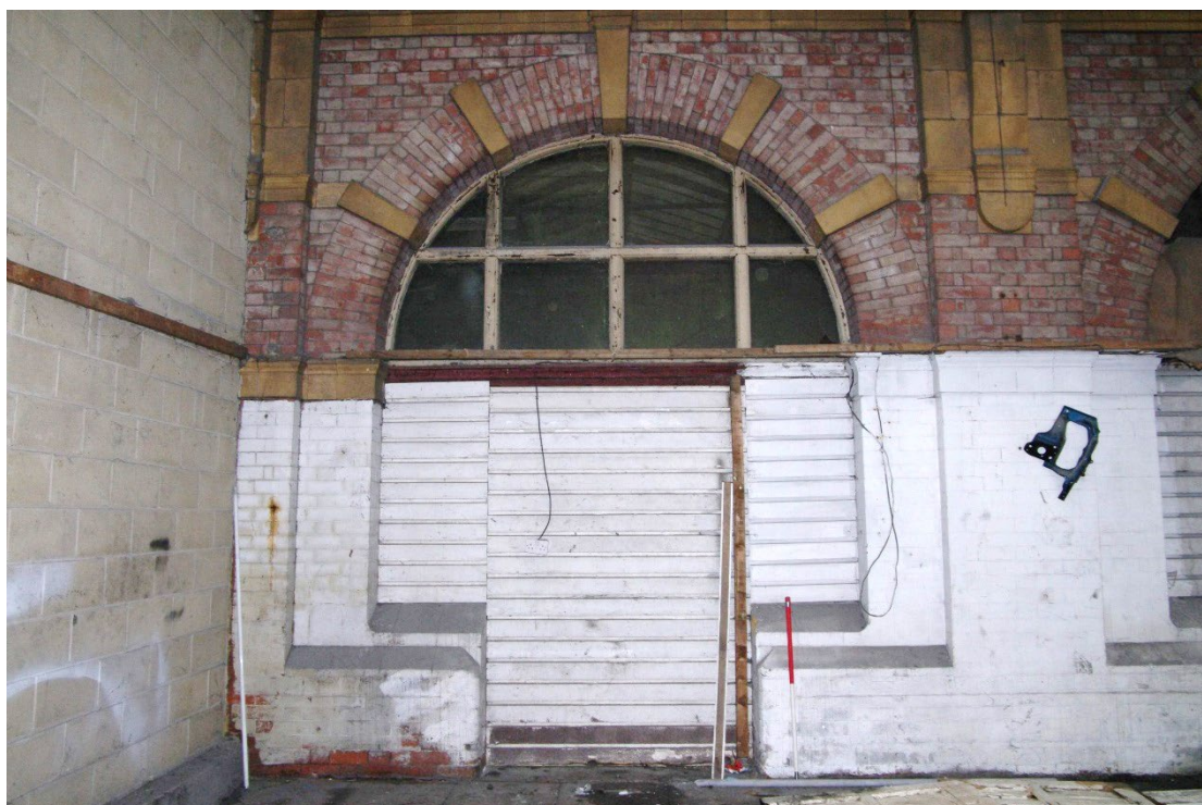
Figure 41 Portico area G1 west wall entrance to booking hall (G6) Looking west. 1m scale
