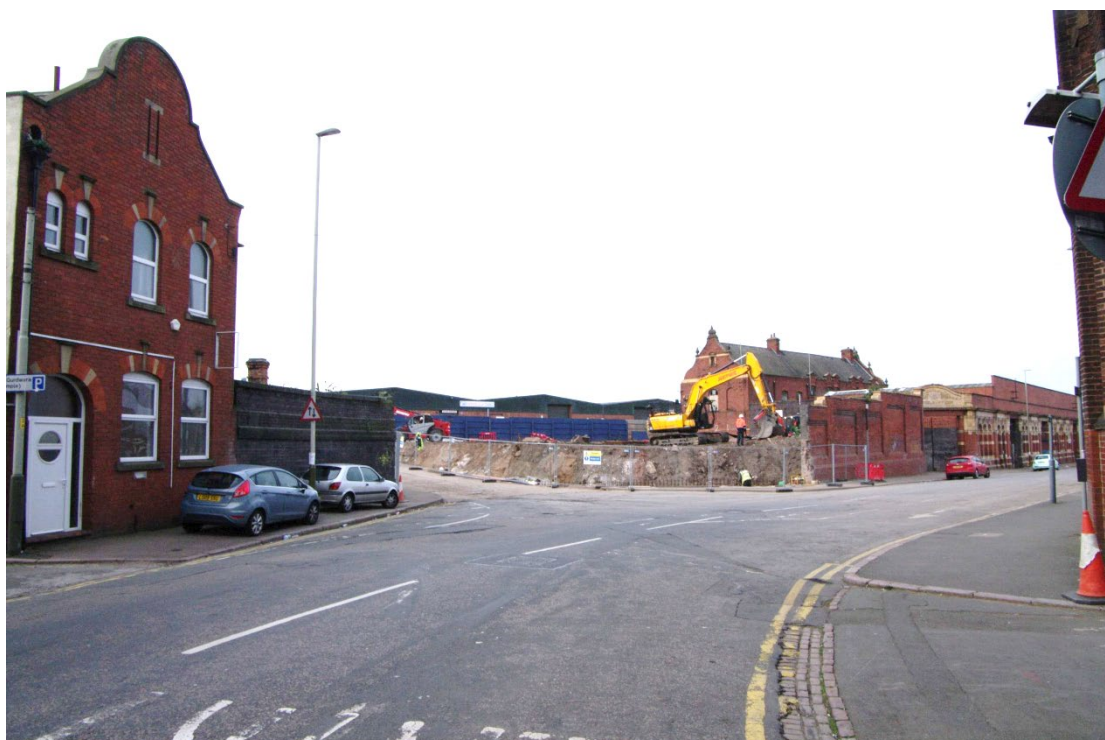
Figure 3 Great Central Street looking north Portico and surviving two storey parcels office on right behind the excavator.
