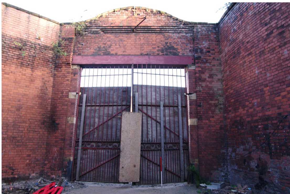
Figure 21 Parcels office yard gates Viewed from the inside looking south-east. 1m scale
