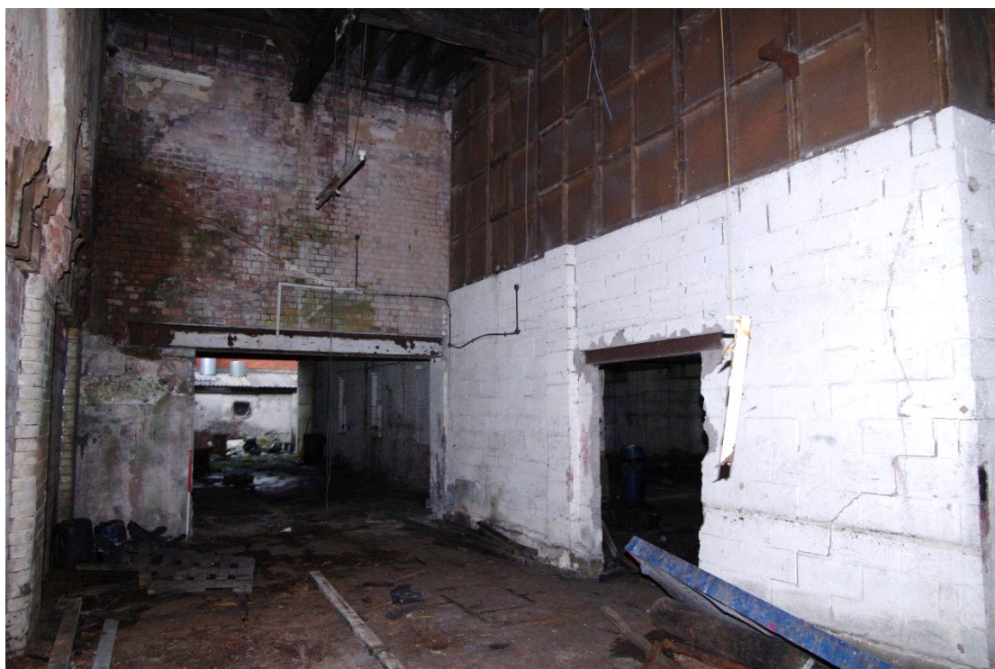
Figure 60 Room G4 Looking north-east through modern opening into G3. 1m scale. Modern partition wall on right. Brackets over arch to the subway entrance are just visible on the left
