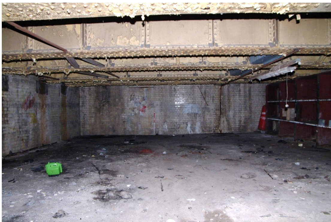
Figure 88 Parcels office Room G11 Standing in Room G10 looking west. 1m scale
