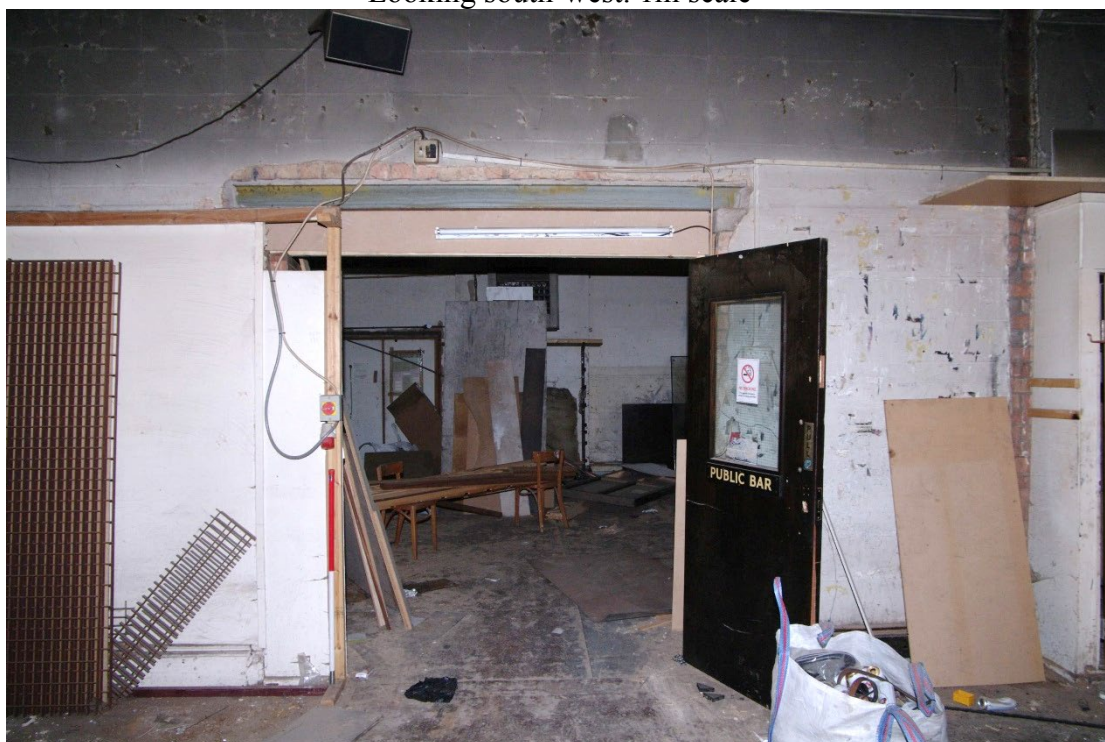
Figure 113 Parcels office Room F2 south wall Looking south at modern doorway to F3. 1m scale. Note modern surround to doorway on right of picture
