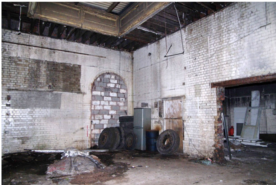
Figure 83 Parcel's office Room G10 Looking north-east. 1m scale. Doorway to G9 on right
