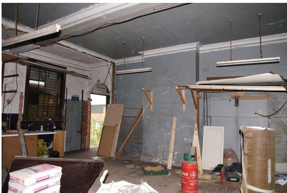
Figure 117 Parcels office Room F4 Looking north-west towards doorway to F3. 1m scale
