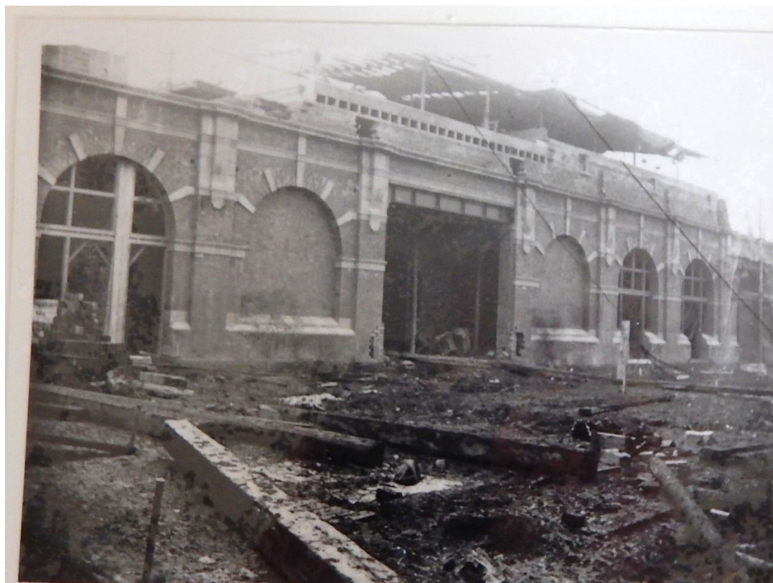
Figure 46 West wall of portico under construction 1897 Looking north-west towards booking hall entrance (centre) Newton collection. ROLLR
