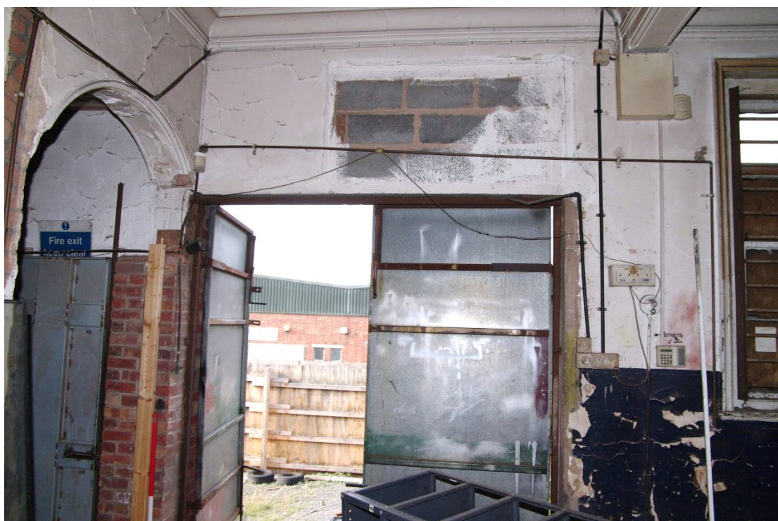
Figure 116 Parcels office Room F3 modified door on west wall Looking west. 1m scale. Note breeze block infill of former window
