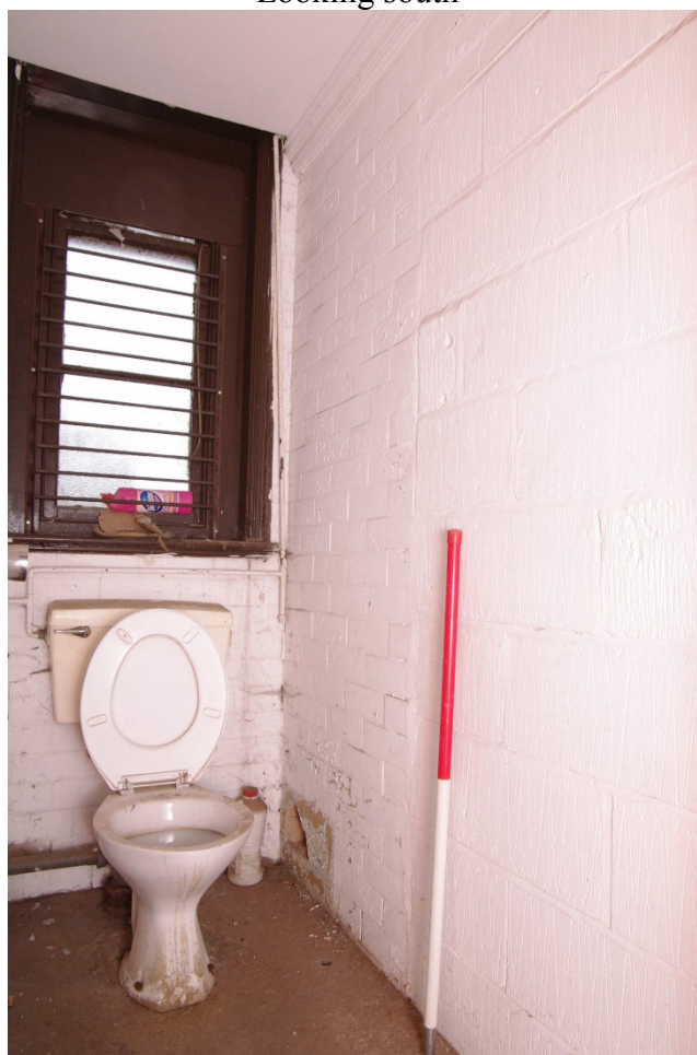
Figure 125 Parcels office Room F7 cubicle Looking west. 1m scale. Note blocked doorway on right
