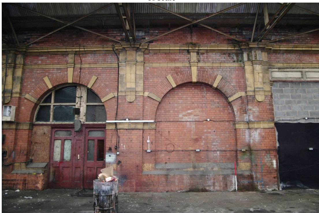
Figure 48 Portico area G7 centre bays Looking west. 1m scale. Doorway to parcels office stairs on left. Entrance to booking hall (G5) on right
