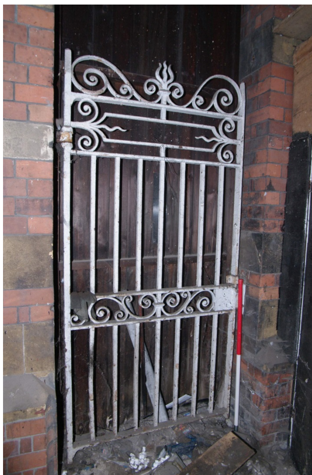
Figure 25 Pedestrian gateway on east-facing elevation of portico Looking south-east from inside the portico. 1m scale
