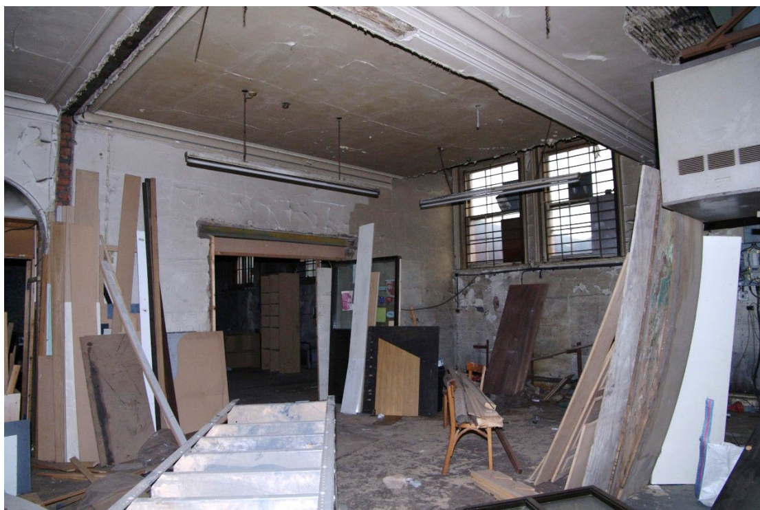
Figure 114 Parcels office Room F3 Looking north-east towards doorway to F2. 1m scale
