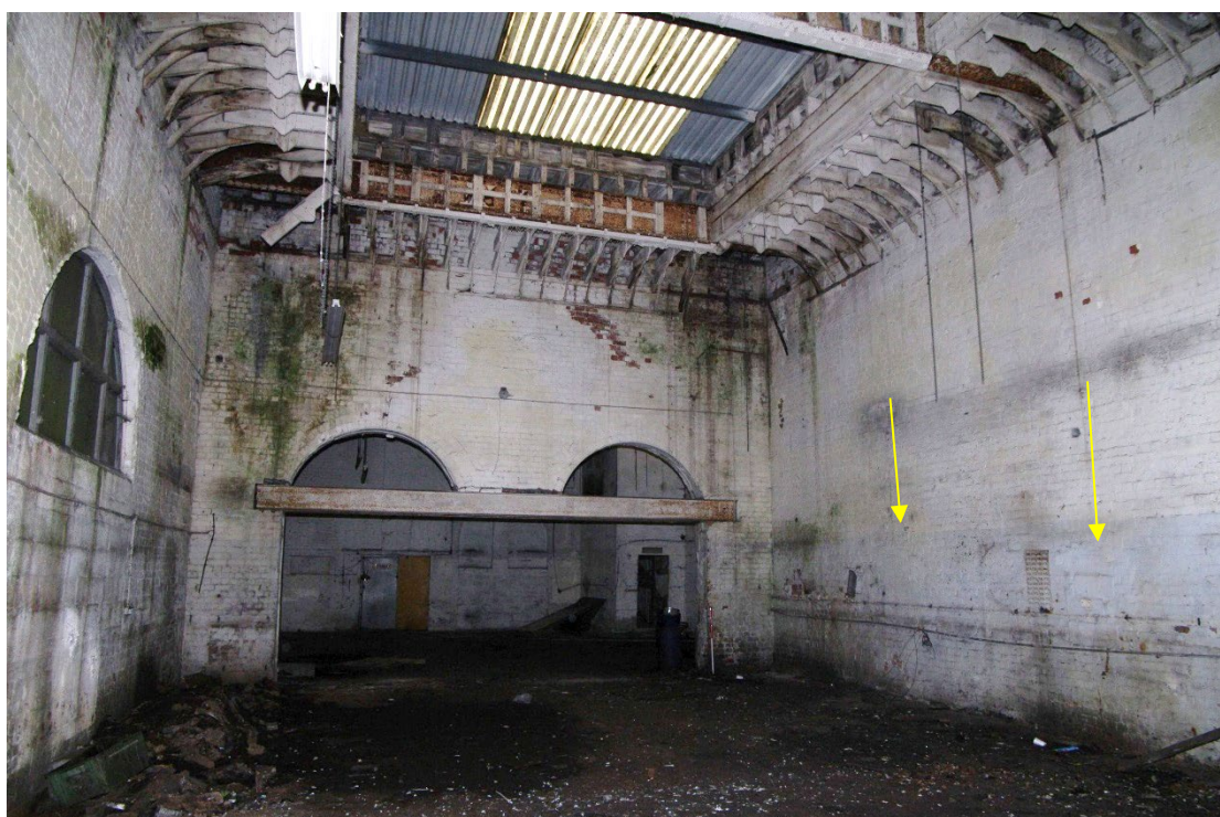
Figure 70 Booking hall, Room G6 Looking south-west. Arrows show blocked ticket booth hatches
