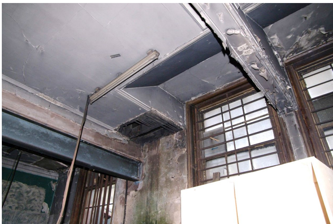
Figure 110 Parcels office Room F2 east wall window Looking north-east. Note new steel support
