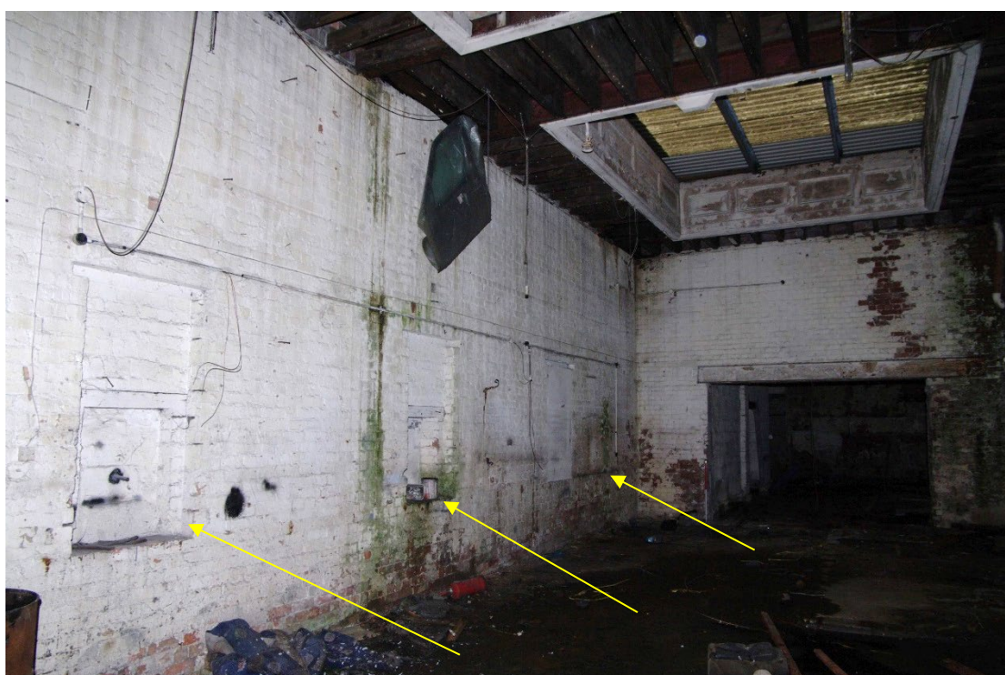
Figure 56 Room G3, ticket office Looking south-east. Note blocked hatches (arrowed) on left-hand wall and modern opening on the end wall
