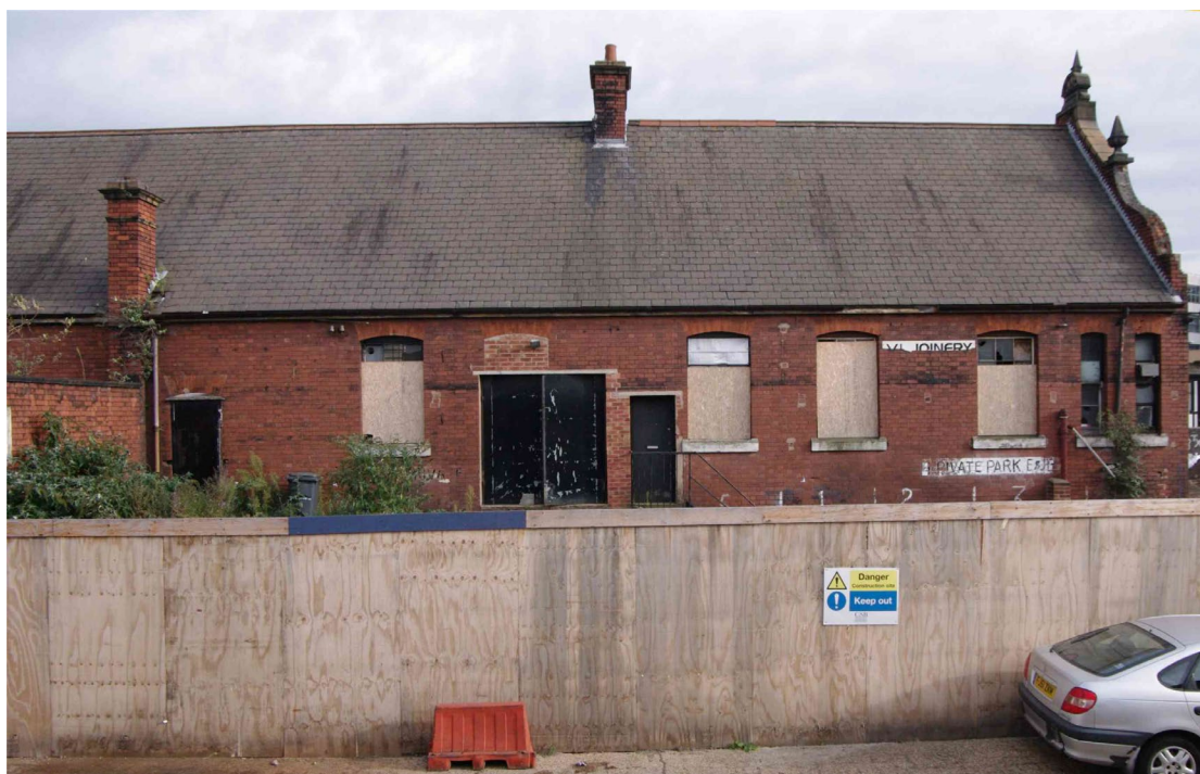
Figure 96 Parcels office west-facing elevation, south end Looking east. The top of the wooden hoarding is approximately the height of the former platform level
