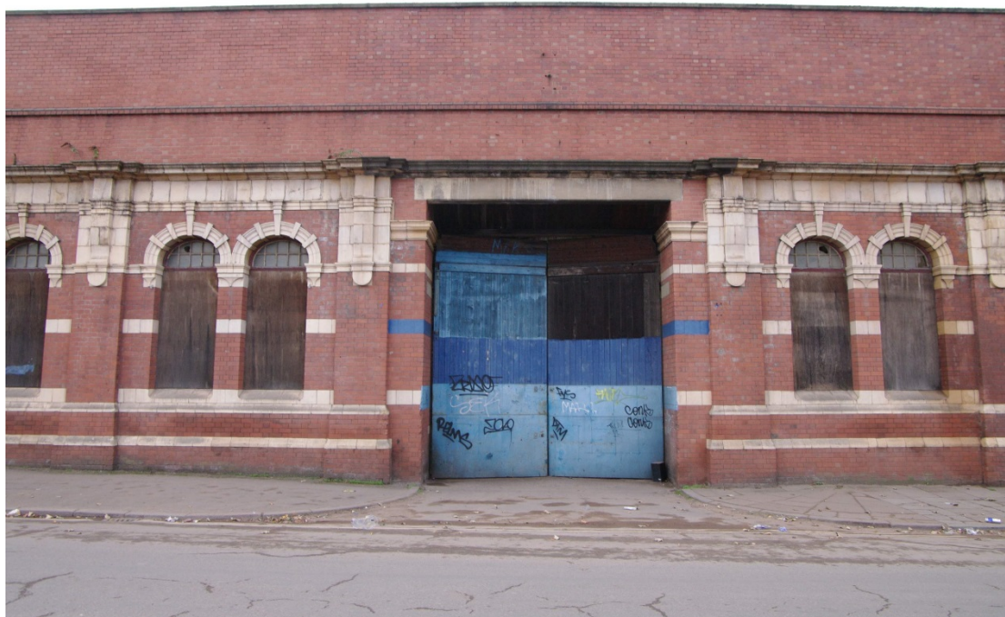
Figure 26 East-facing elevation of portico, centre vehicle entrance Looking west. Note the concrete lintel which replaced a large archway beneath the demolished clock tower
