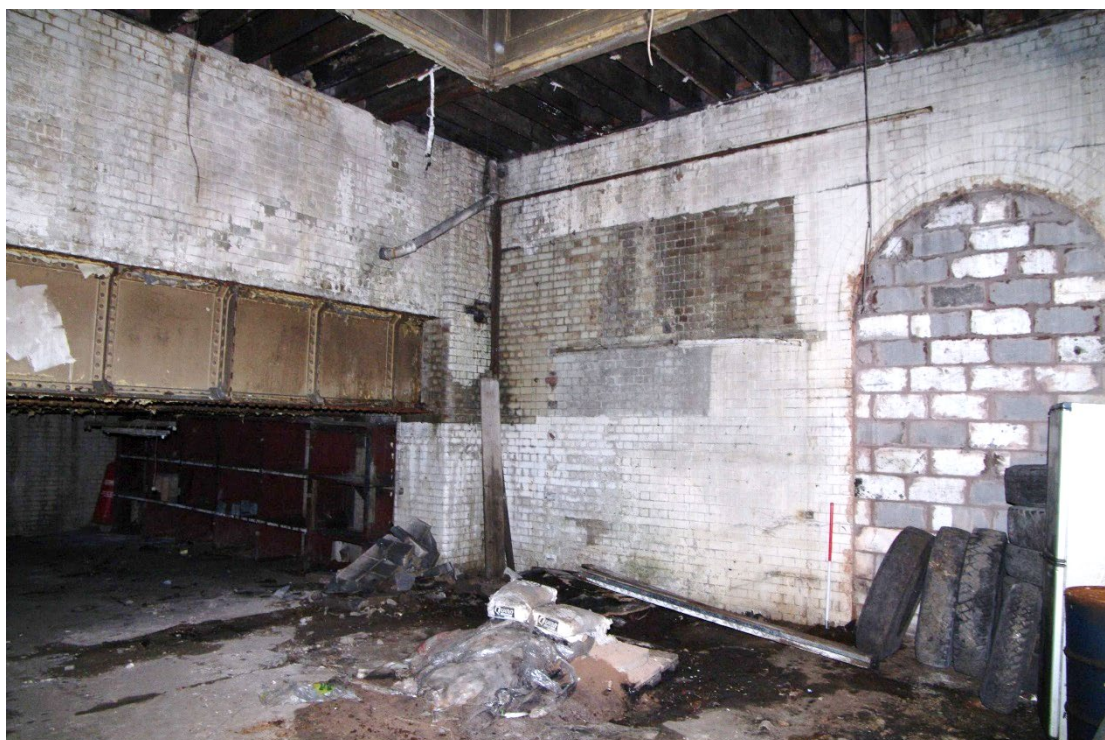
Figure 84 Parcel's office Room G10 Looking north-west. 1m scale. G11 on left below girder
