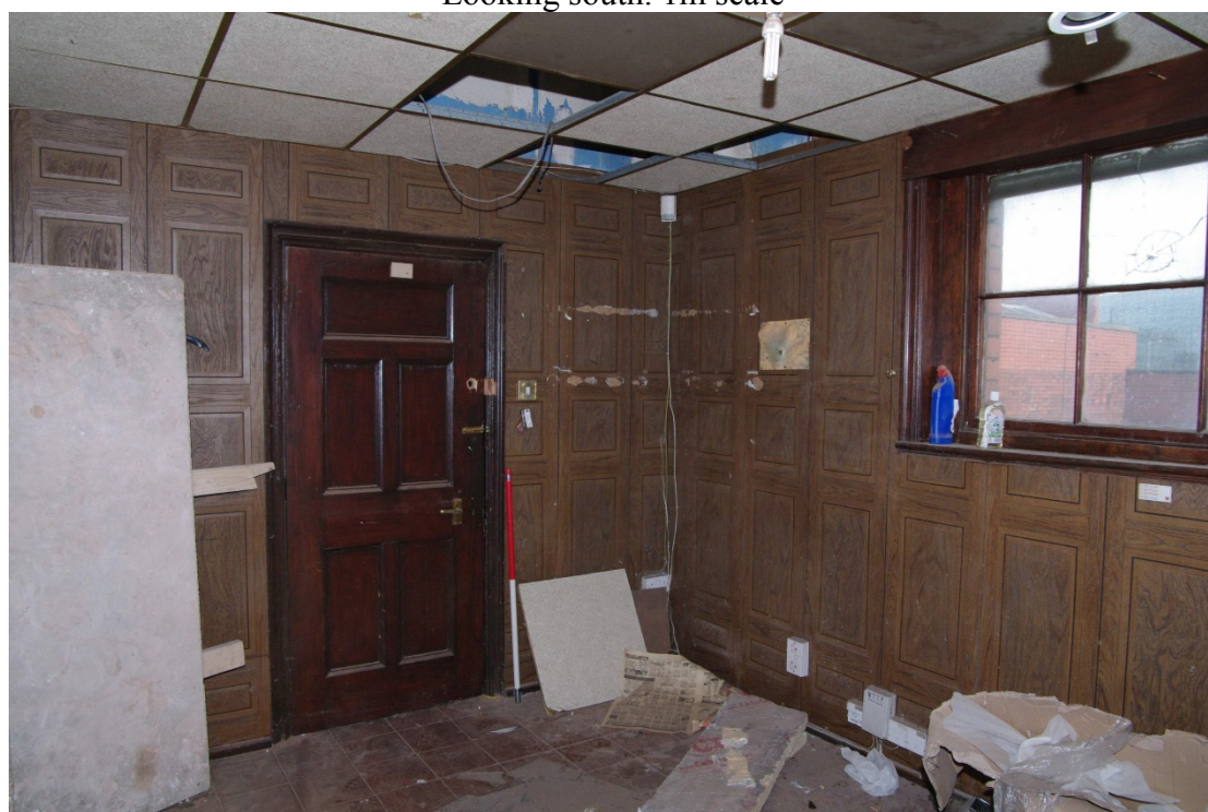
Figure 121 Parcels office Room F5 Looking north-east. 1m scale. Note false ceiling cutting sash window
