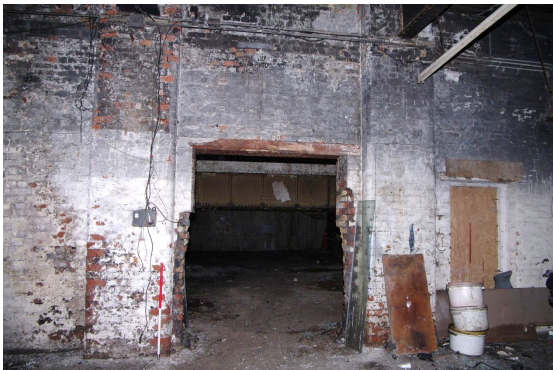
Figure 81 Parcels office Room G9 west wall Looking west into Room G10. 1m scale
