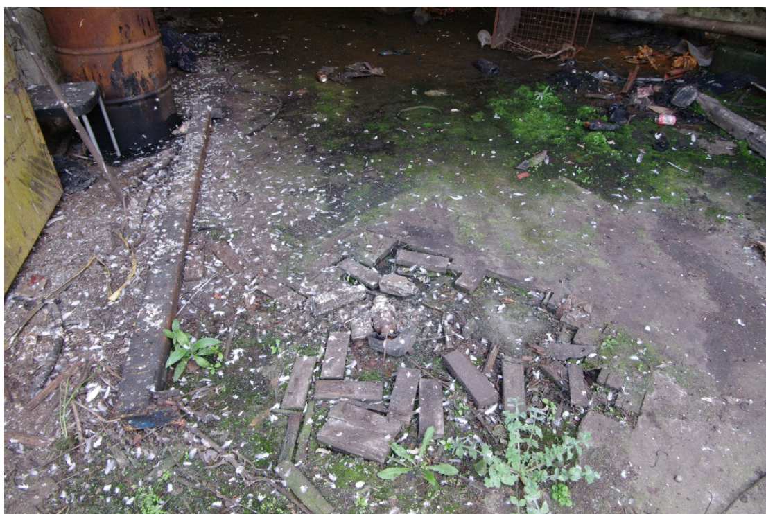
Figure 59 Room G3, woodblock floor Looking west close to doorway to yard G2
