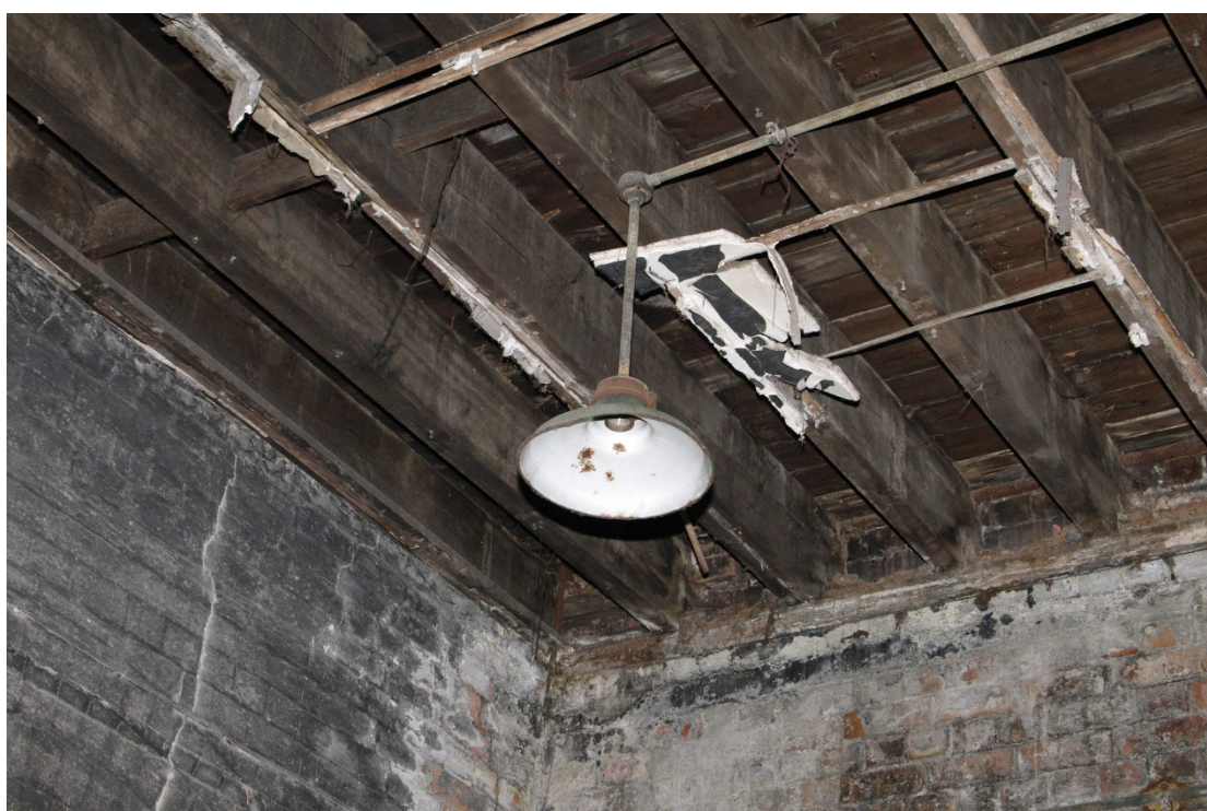
Figure 82 Parcels office Room G9, light fitting Looking towards south-western corner of the room
