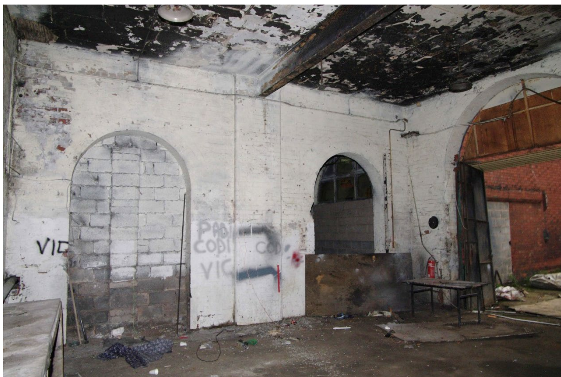
Figure 74 Parcels office ground-floor Room G8 north wall Looking north-east towards doorway to G9. 1m scale
