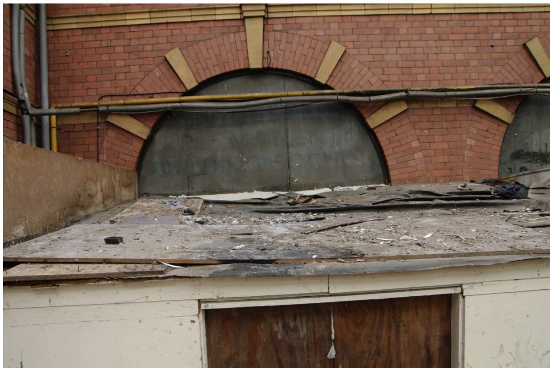
Figure 45 Portico area G7 advertisement in blind arch Looking south. Advertisement on the grey panel reads “LEICESTER PERMANENT BUILDING SOCIETY”
