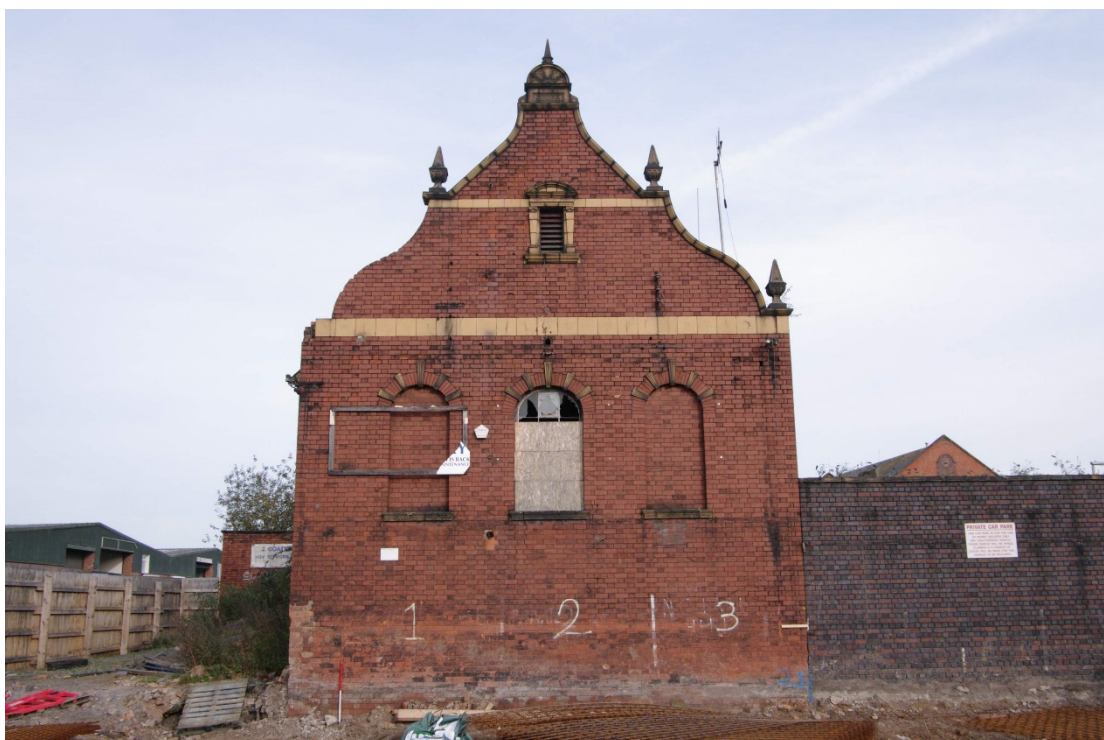
Figure 94 Parcels office south-facing elevation Looking north. 1m scale. Former platform area to left
