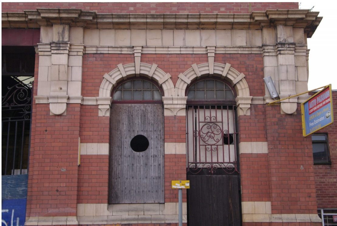
Figure 24 East-facing elevation of portico, pedestrian entrance gate detail Looking west at north end of elevation
