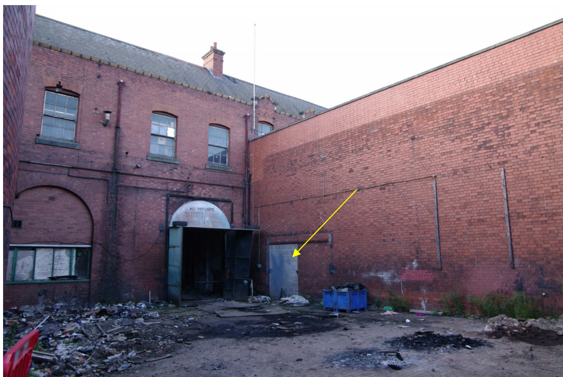
Figure 31 South-facing elevation of the portico Looking north-west from inside the parcels yard. Note blocked doorway into portico (arrowed) and rebuilt parapet. Arches lead into G8.
