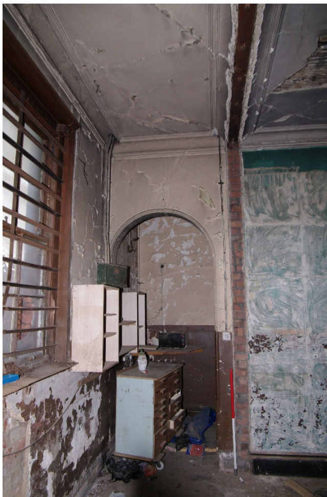
Figure 108 Parcels office Room F2 Looking north at scar left by corridor partition. 1m scale
