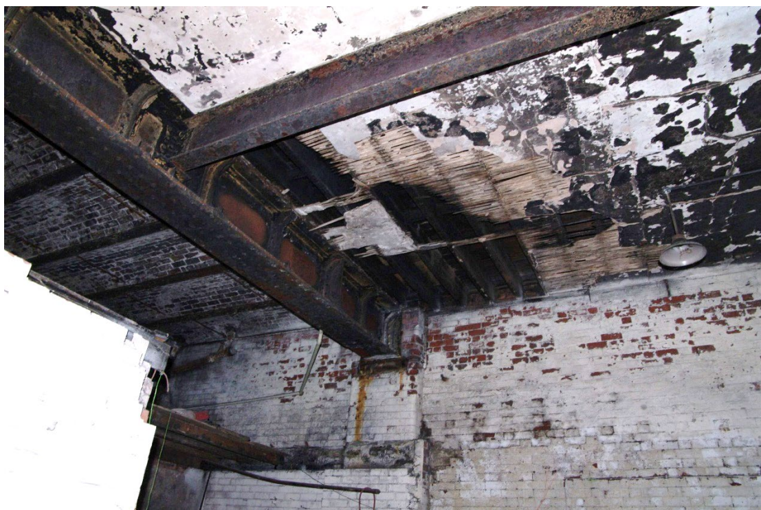
Figure 75 Parcels office ground-floor Room G8 fire damage Looking towards south wall. Note vaulted ceiling on left
