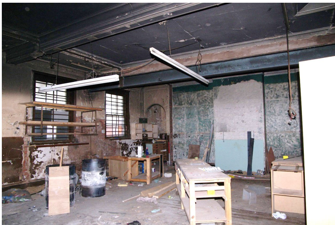
Figure 107 Parcels office Room F2 Looking north-west. Archway to F1 in corner. Note scar left by removed partition
