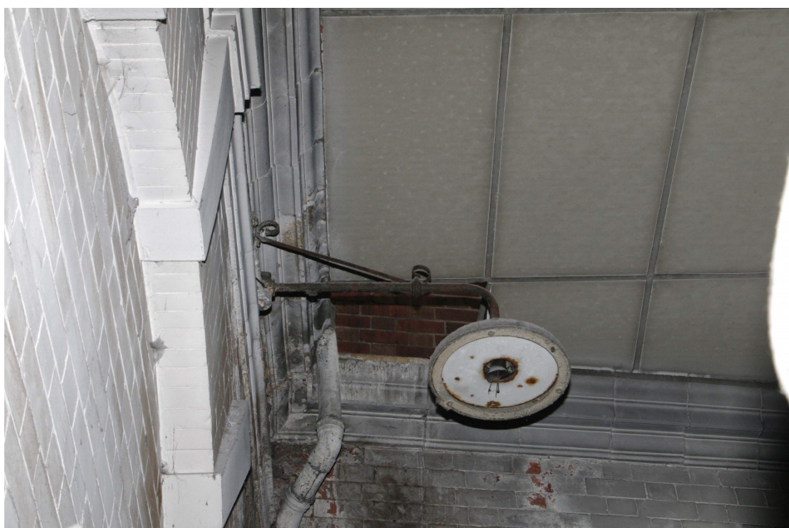
Figure 40 Portico area G1 light fitting on north wall Looking east
