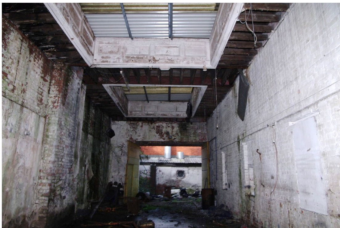
Figure 58 Room G3, ticket office Looking north towards modified doorway to yard G2
