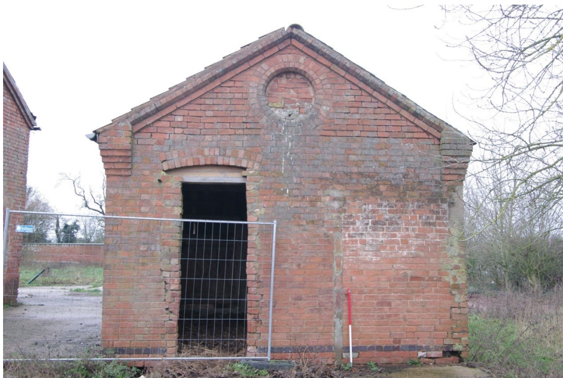
Figure 109 East to west barn, east facing elevation Looking west. 1m scale. Note scar of former structure to left of scale
