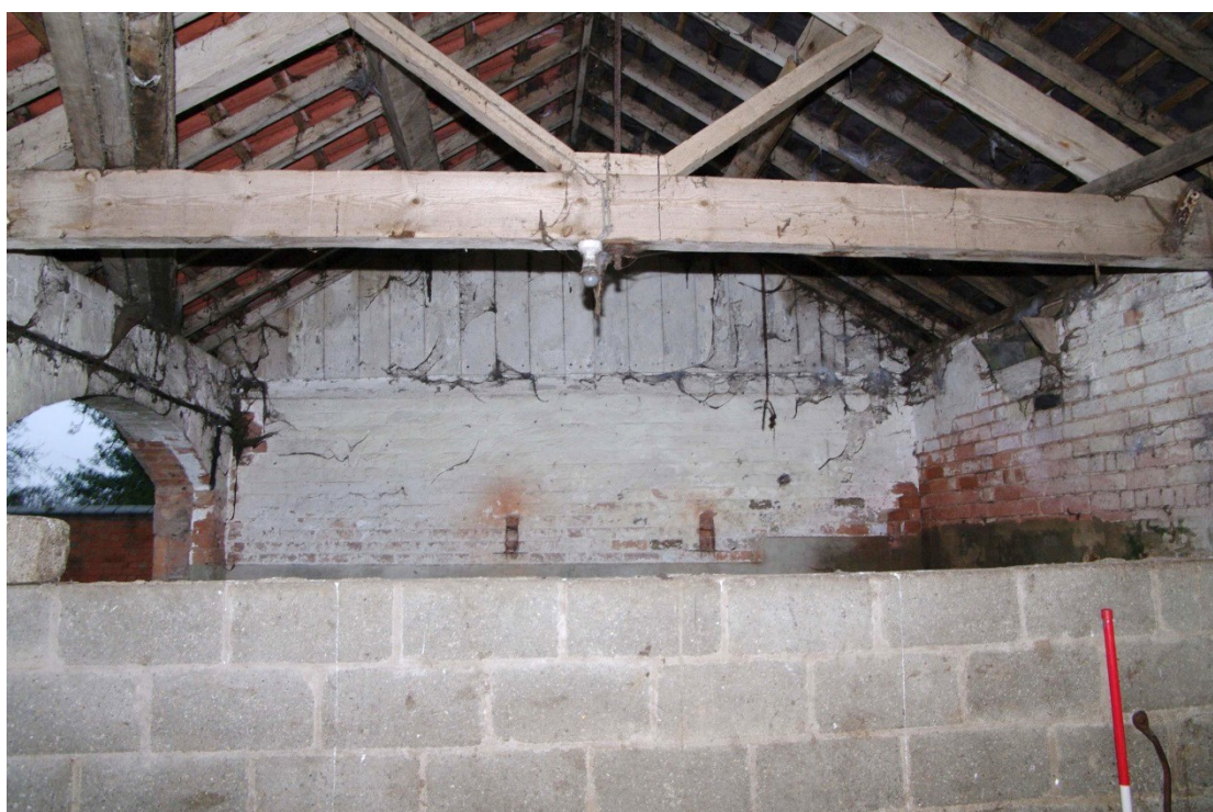
Figure 117 East to west barn. Room 2 Looking west. 1m scale. Note brick and boarded dividing wall to Room 1
