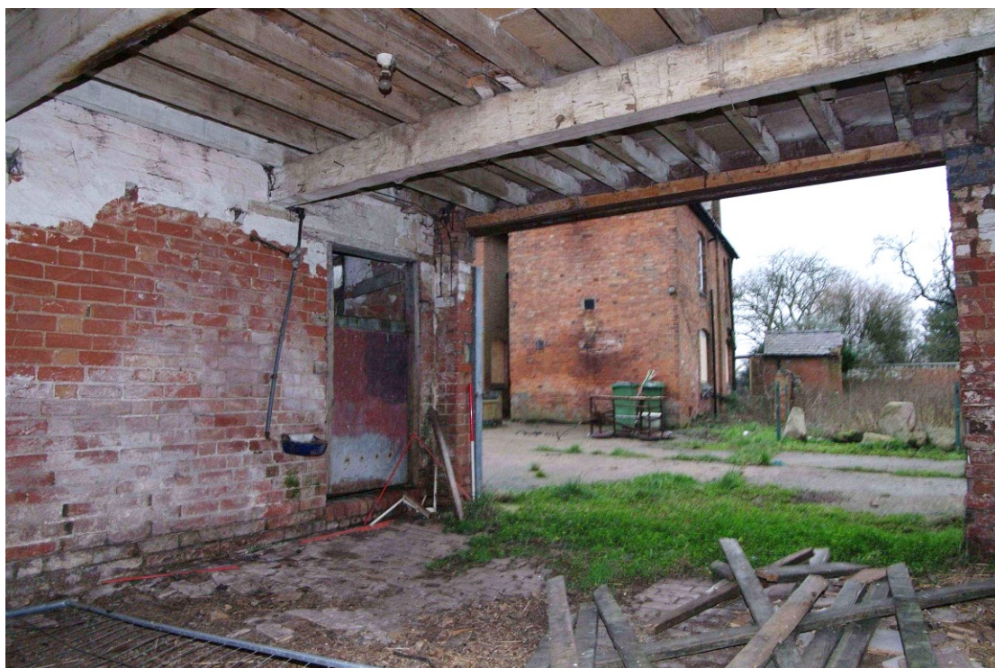
Figure 97 North to south barn. Room 2 Looking south-west. 1m scale. Doorway to Room 3 on left
