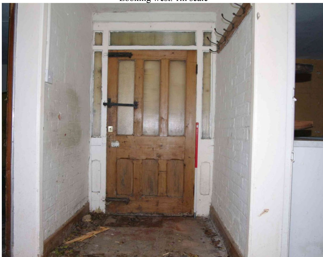
Figure 25 Rear door on east facing elevation from inside Looking east. 1m scale
