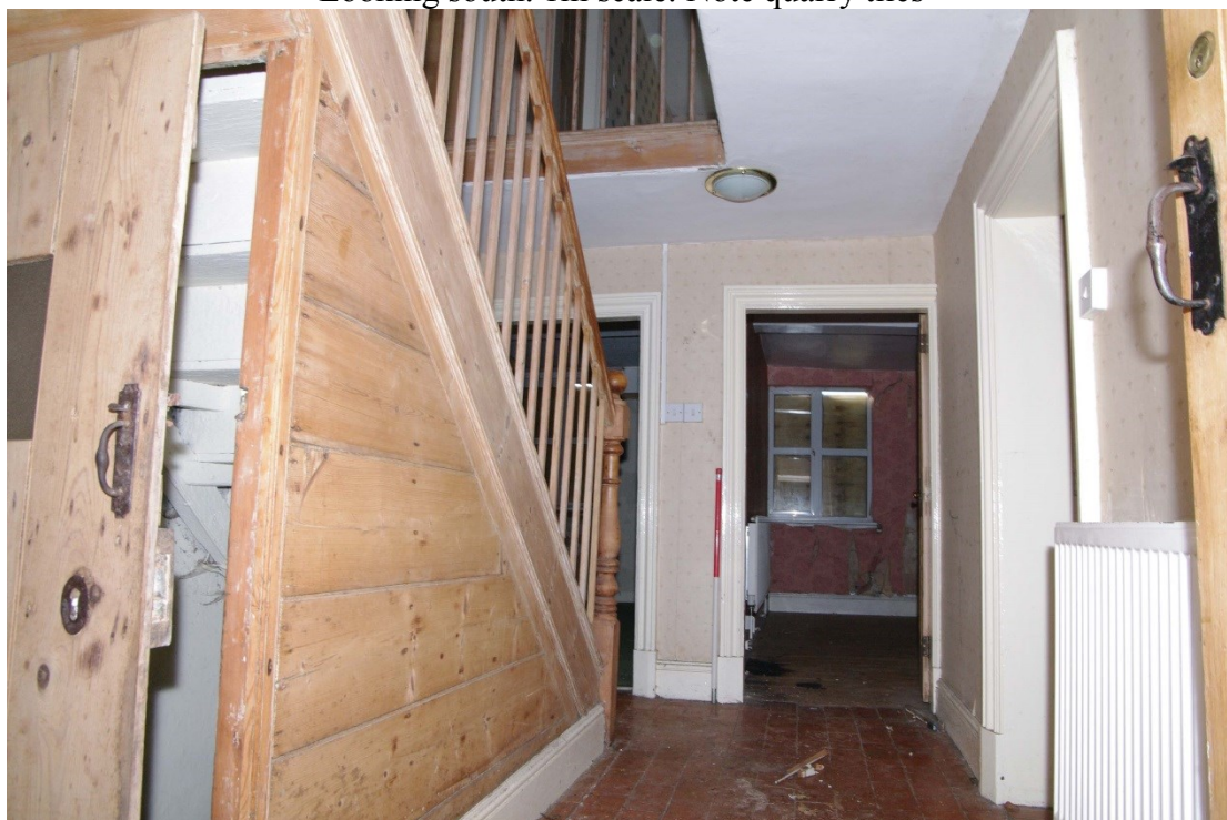
Figure 36 Hallway door frames into Rooms 2, 3 and 5 Looking west. 1m scale. Door to cellar on left, Room 5 on right
