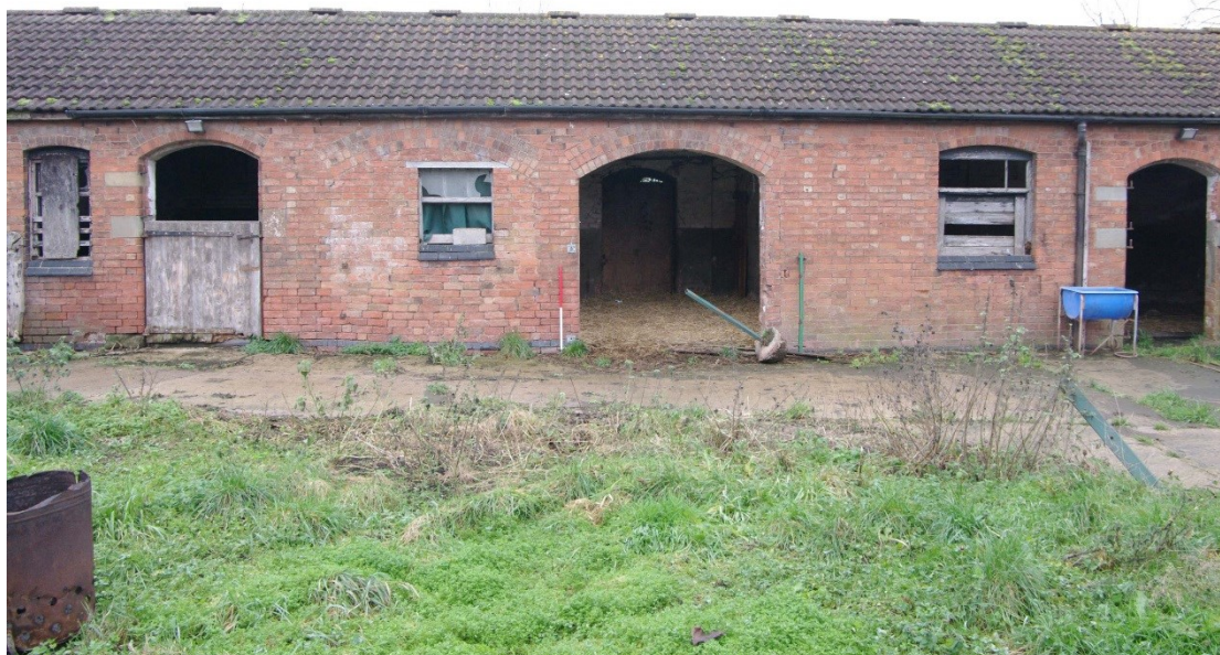
Figure 107 East to west barn. South facing elevation, centre section Looking north. 1m scale. Note blocked arch to left of scale
