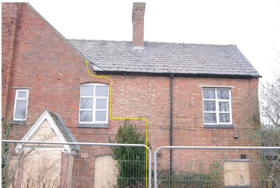
Figure 18 South facing elevation, rear range Looking north. Yellow line indicates rebuilding line
