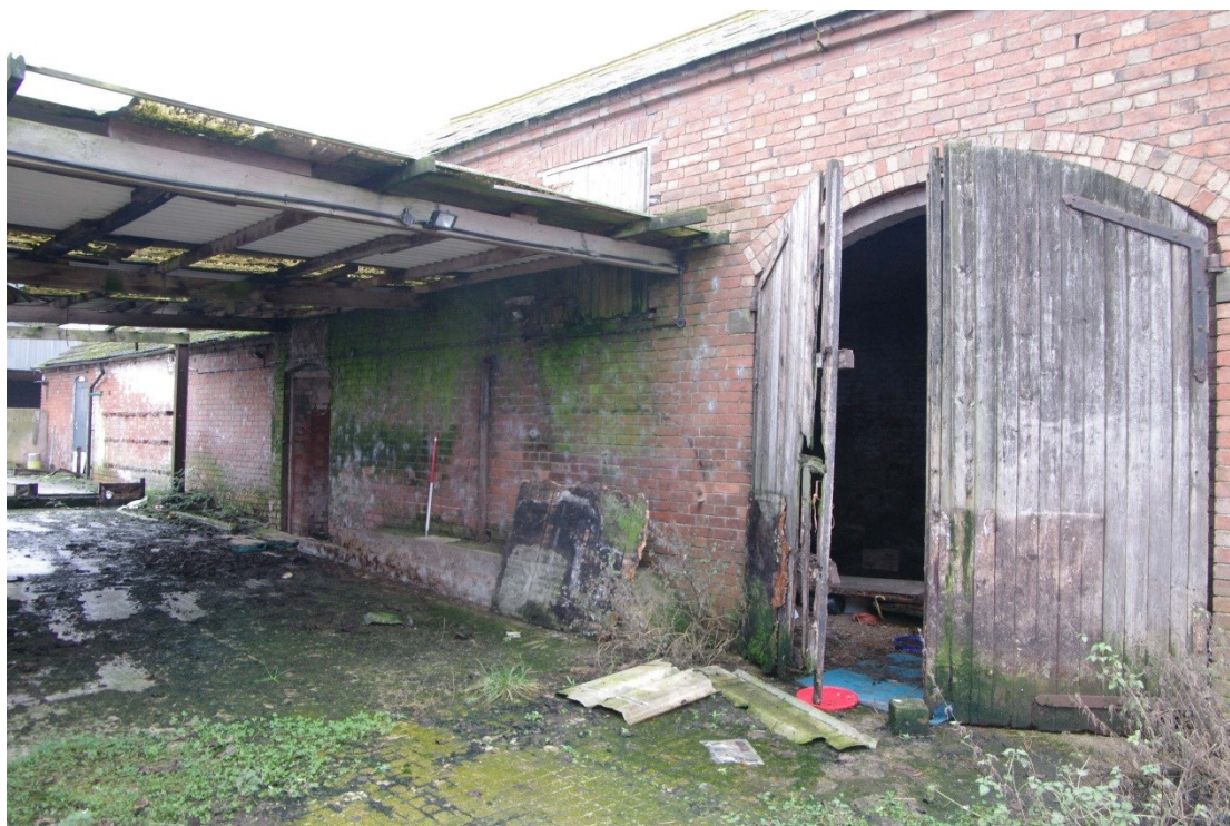
Figure 90 North to south barn. East facing elevation, middle of range. Looking south-west. 1m scale
