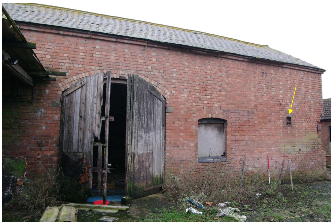
Figure 91 North to south barn. East facing elevation, northern end Looking north-west. 1m scale. Bearing box arrowed
