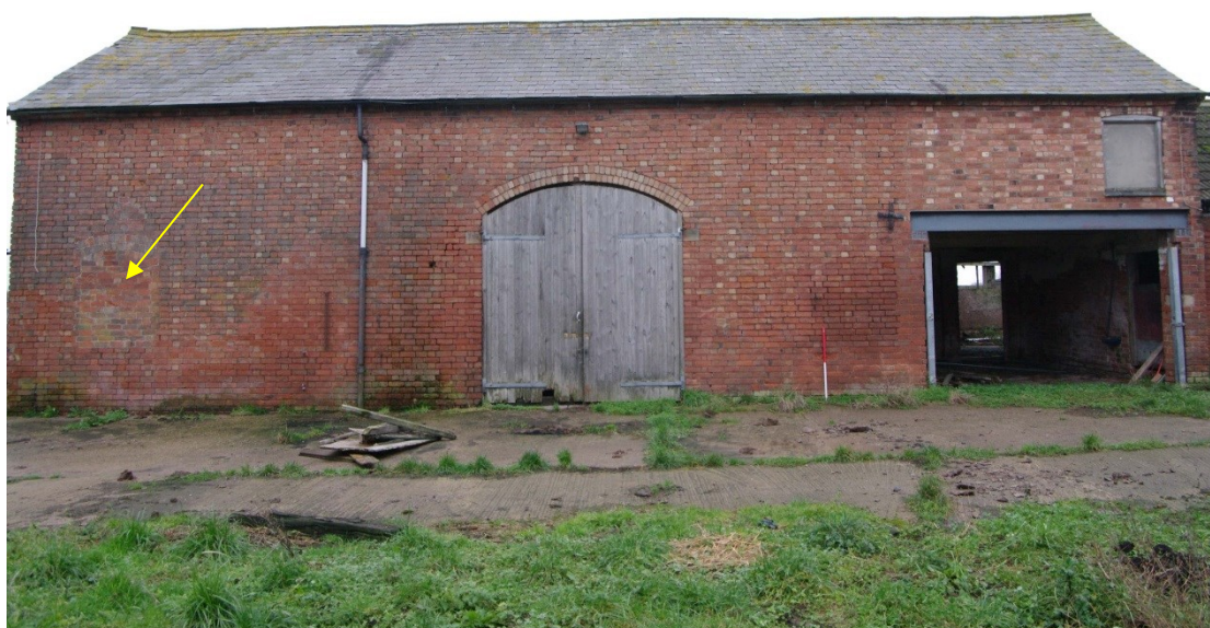
Figure 83 North to south barn. West facing elevation of north end of range Looking east. 1m scale. Arrow points to blocked window. Note rebuilt brickwork above steel lintel on right
