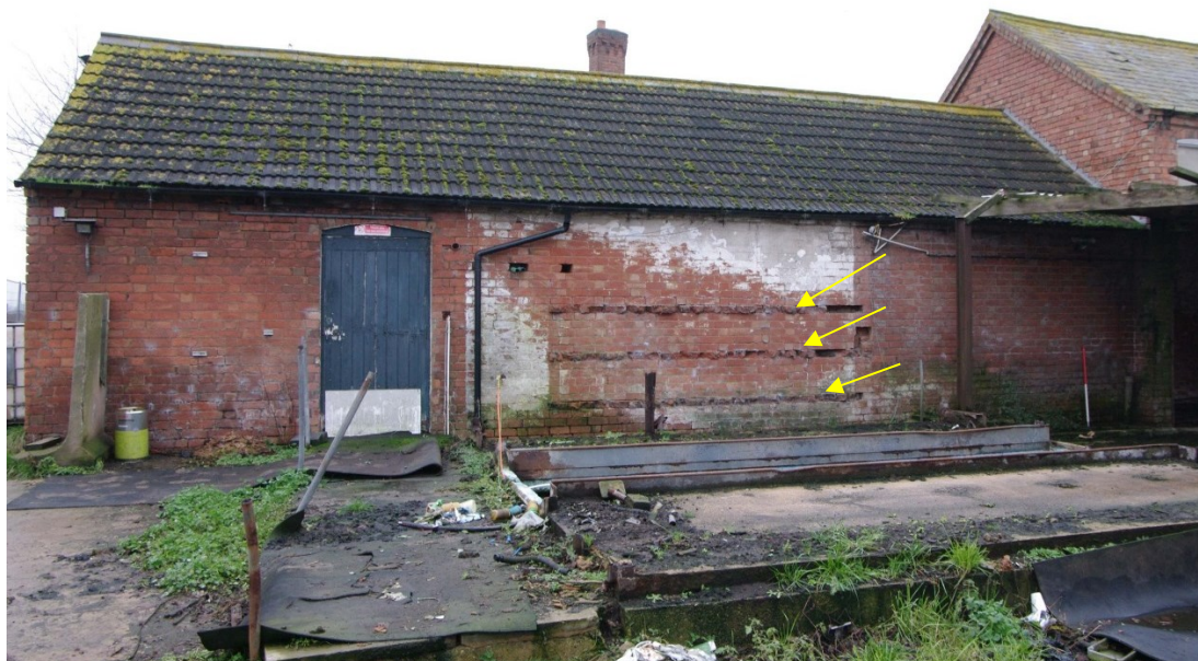
Figure 88 North to south barn. East facing elevation, south end of range. Looking west. 1m scale. Arrows point to broken brickwork projections
