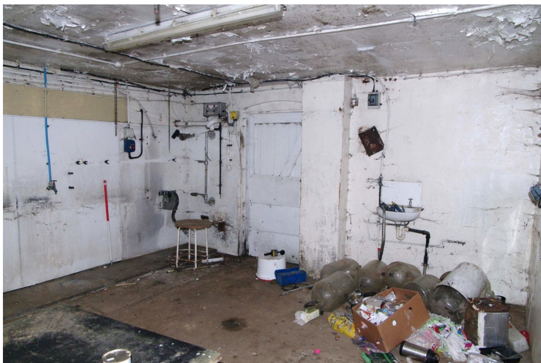
Figure 102 North to south barn. Room 4 Looking north-east. 1m scale. Note glass milk receptacles on floor
