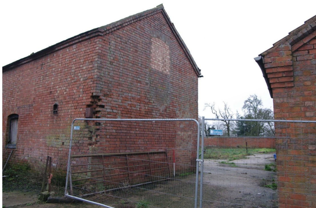
Figure 92 North to south barn. North facing gable end Looking south-west. 1m scale. Blocked doorway to right of scale. Compare brickwork decoration of both ranges
