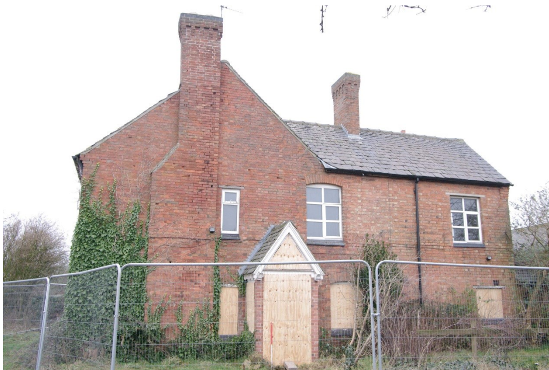
Figure 14 Farmhouse south facing elevation Looking north-east. 1m scale. Note single storey part of range on far right of photo
