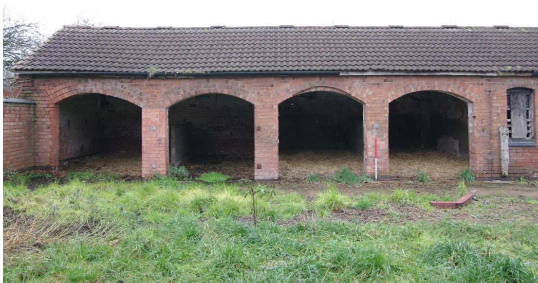
Figure 106 East to west barn. South facing elevation, western end Looking north. 1m scale
