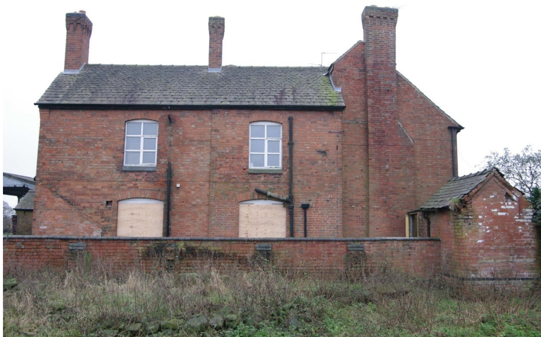
Figure 26 Farmhouse north facing elevation Looking south over foldyard wall. Privy on right of picture
