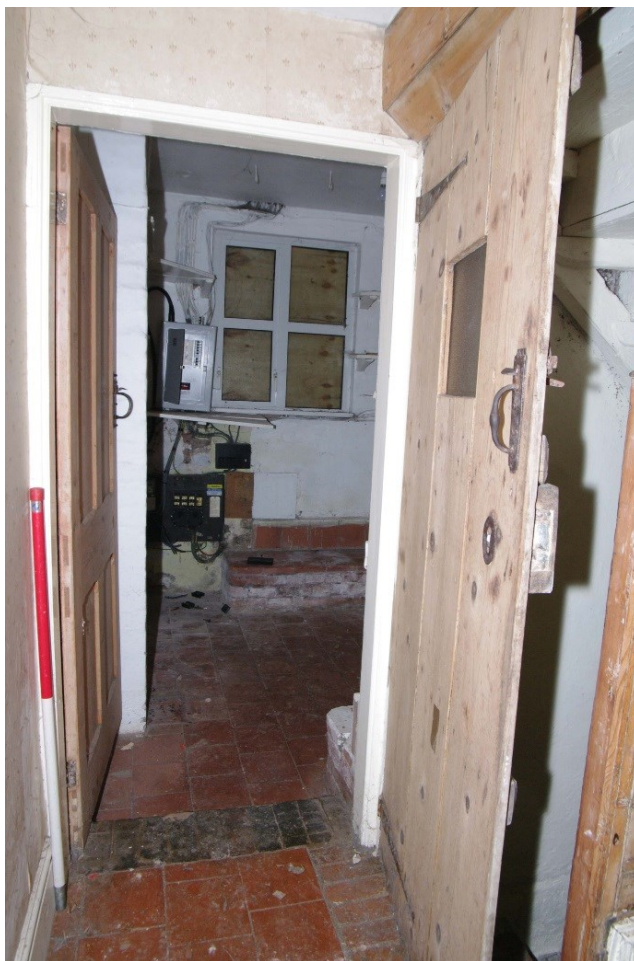
Figure 43 Doorway to Room 3 Looking south from hall. 1m scale. Door down to cellar on right
