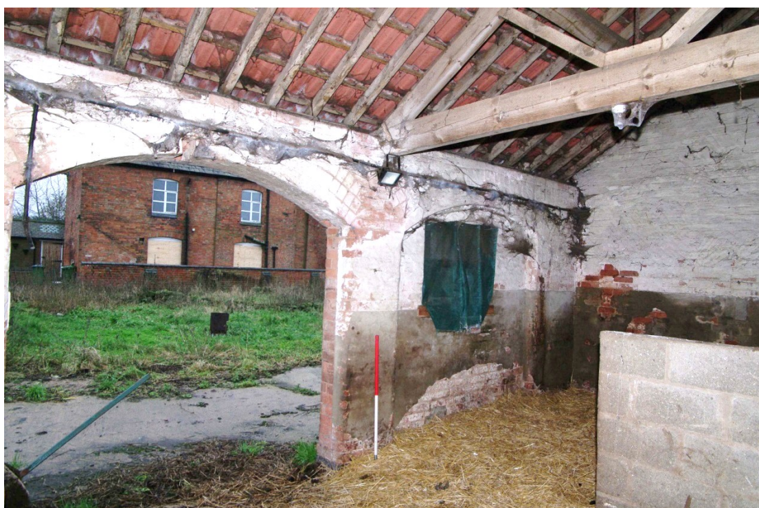
Figure 119 East to west barn. Room 4 Looking south-west. 1m scale. Note blocked arch to right of scale
