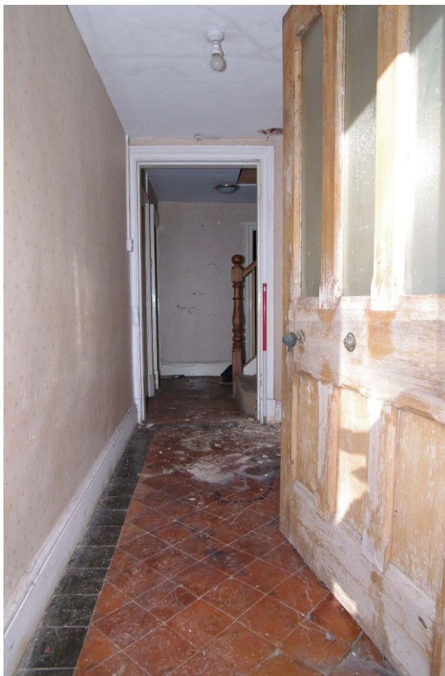
Figure 33 Ground floor hallway from front door Looking north towards foot of stairs. 1m scale
