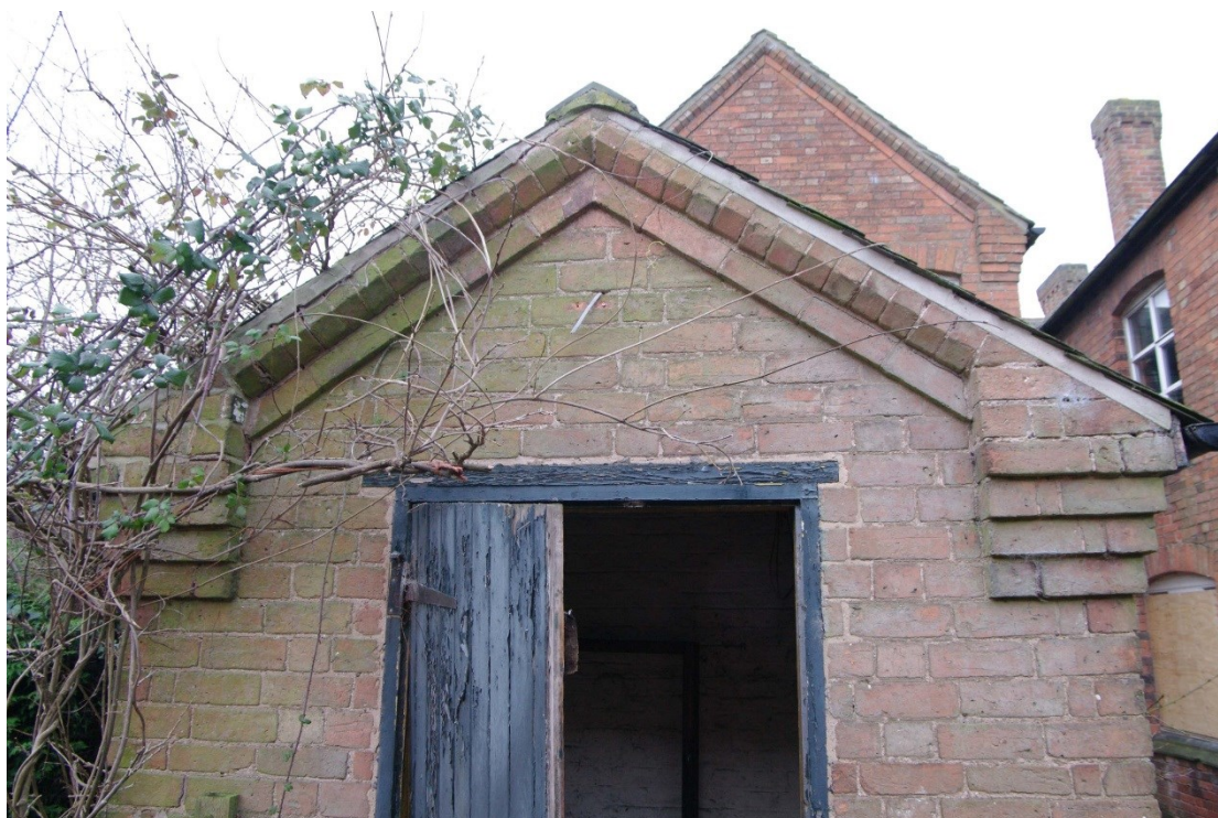
Figure 22 East facing elevation detail of brickwork decoration Looking west at gable of single storey rear range. Note the same decoration on the two storey range and chimney stacks
