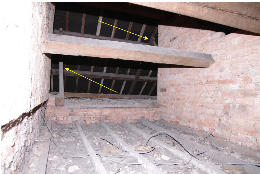
Figure 72 Roof structure of main farmhouse Looking west from hatch over staircase. Pegged supports arrowed
