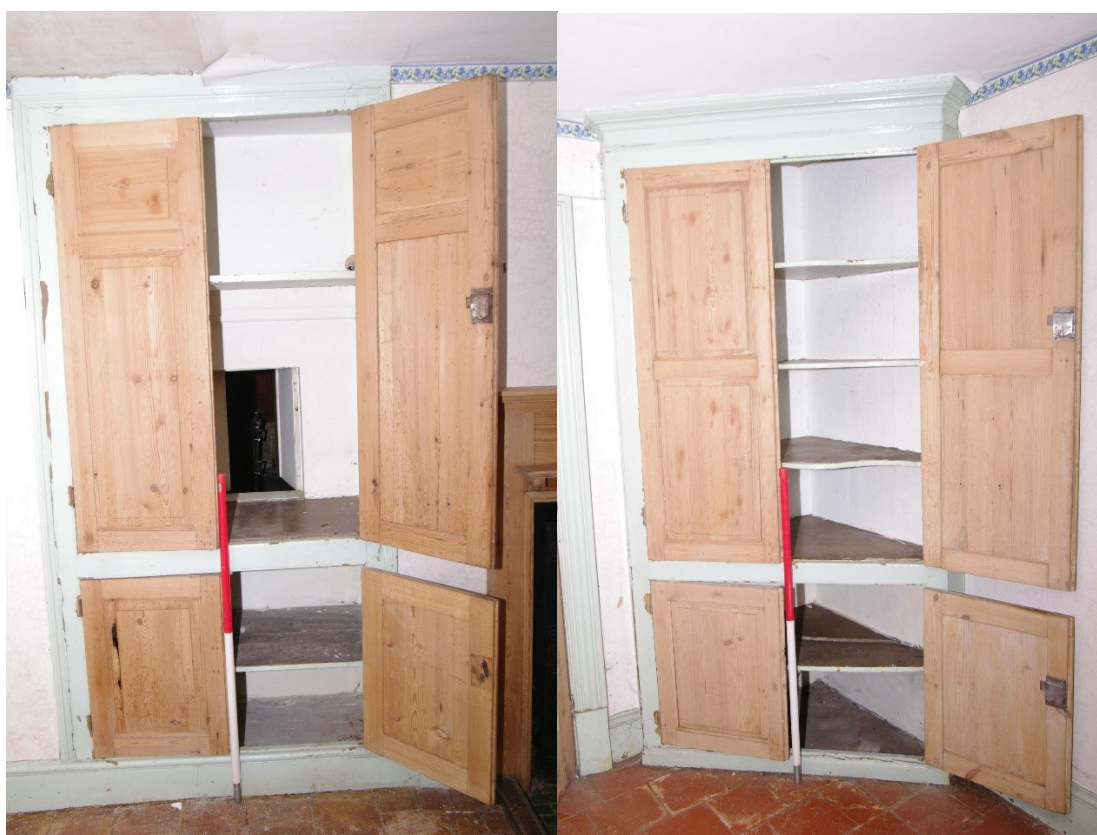
Figure 48 Room 5 fitted cupboards Left: north-east corner of room, Right: south-west corner of room.
