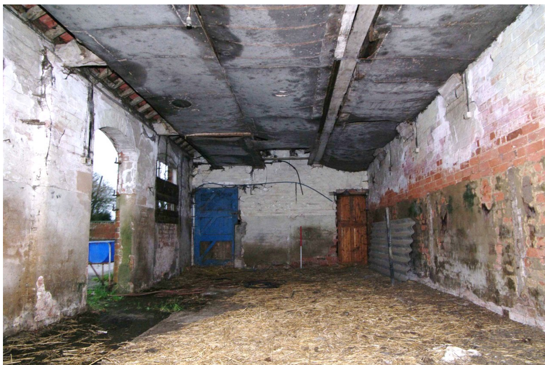
Figure 121 East to west barn. Room 5 Looking west towards doors to Room 4. 1m scale
