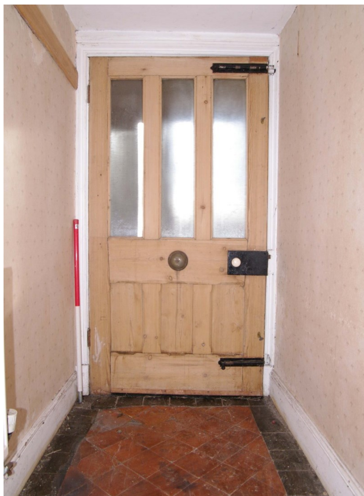
Figure 35 Main doorway on south facing elevation Looking south. 1m scale. Note quarry tiles
