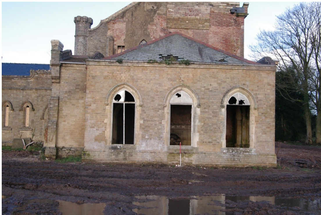
Figure 8 South facing elevation of morning room Looking north. 1m scale. Note scarring on first floor of main house following removal of the morning room first floor
