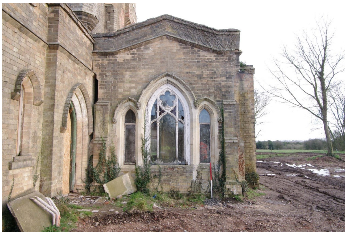
Figure 11 West facing elevation of morning room Looking east. 1m scale. Note joint with main building on left hand side
