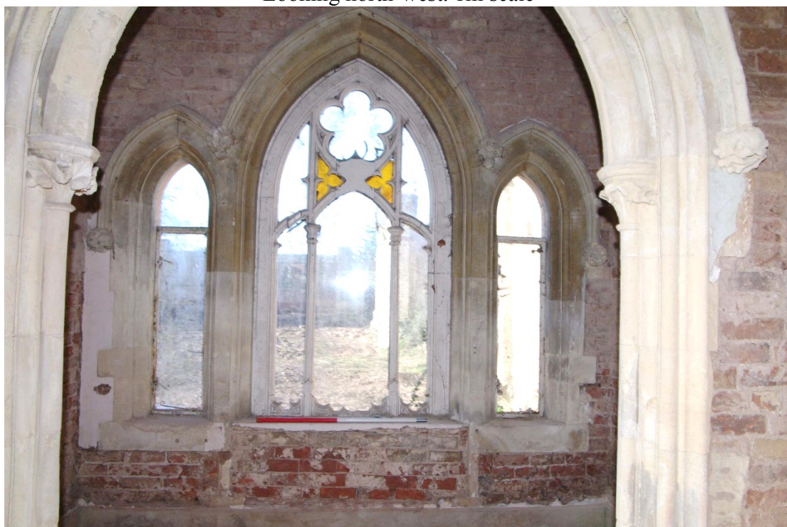
Figure 30 West wall lancet window detail Looking west. 1m scale. Noted patched brickwork under centre window
