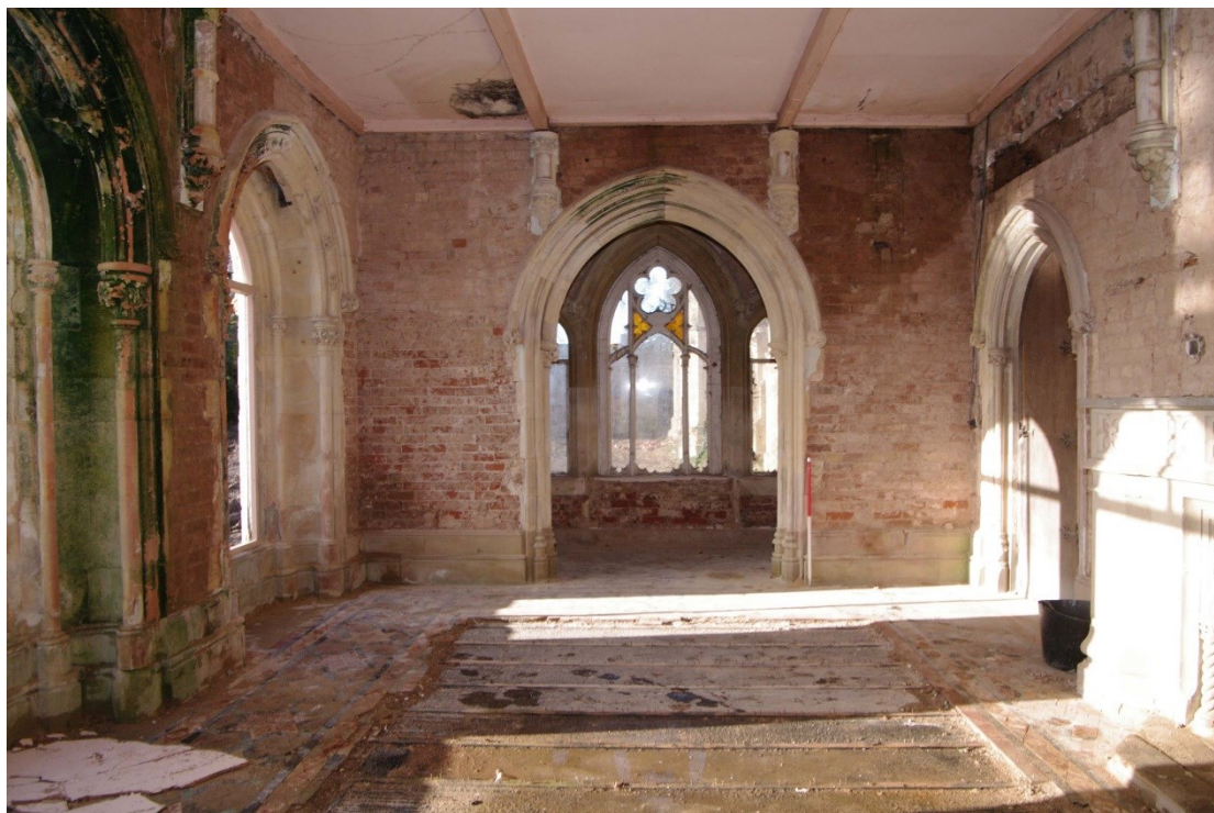
Figure 13 Morning room general view Looking west. 1m scale. Arched doorway into main house on right
