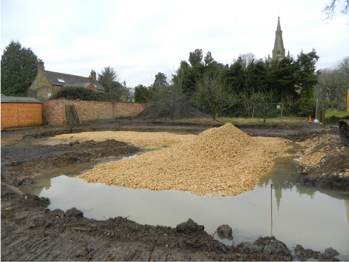
Figure 9: Terram in place covered by gravel prior to excavating the foundations. Looking west
