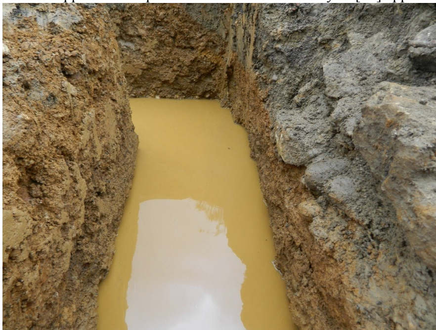
Figure 28: Looking south. Western foundation trench with wall [50] on the right, and no lower courses of wall [21] evident on the left
