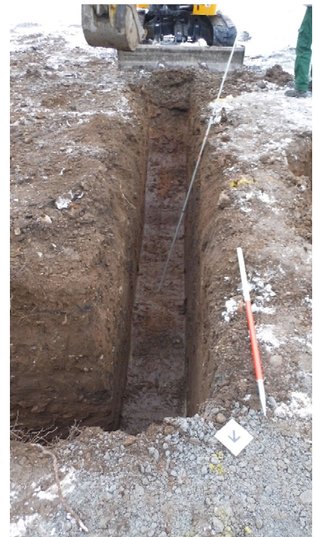
e. South facing view of west trench footings of garage (Scale: 1.00m)
