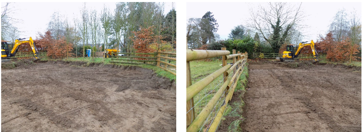
Figure 5. Ground reduction on the southern end of the assessment area prior removal of trees.
