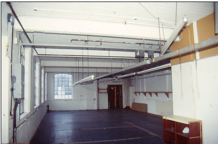
Plate 9. Frontage range (Block A), first floor interior looking E, Shilton Road to left (C30)
