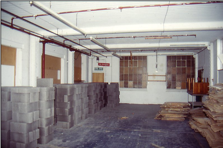
Plate 20. First floor interior of Block C, looking N towards rear elevation of Block A (C33)
