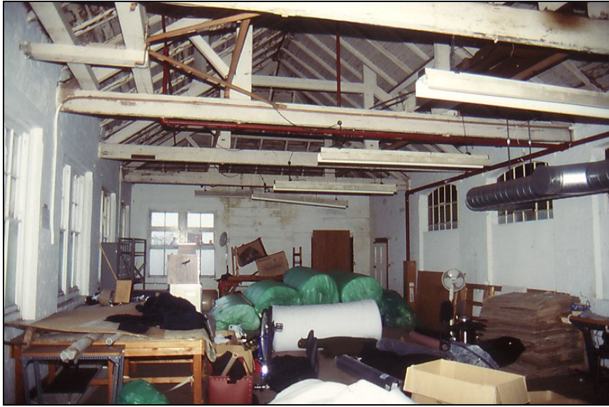
Plate 10. Frontage range (Block A), second floor interior looking E, showing queen-post roof structure (C35)
