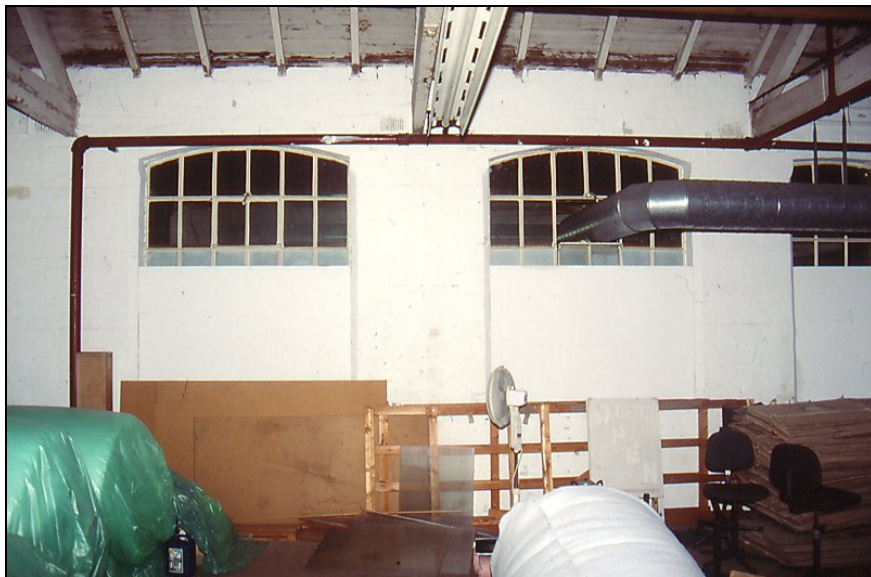
Plate 11. Original second floor windows in S (rear) elevation of Block A, now overlooking Block C (C39)
