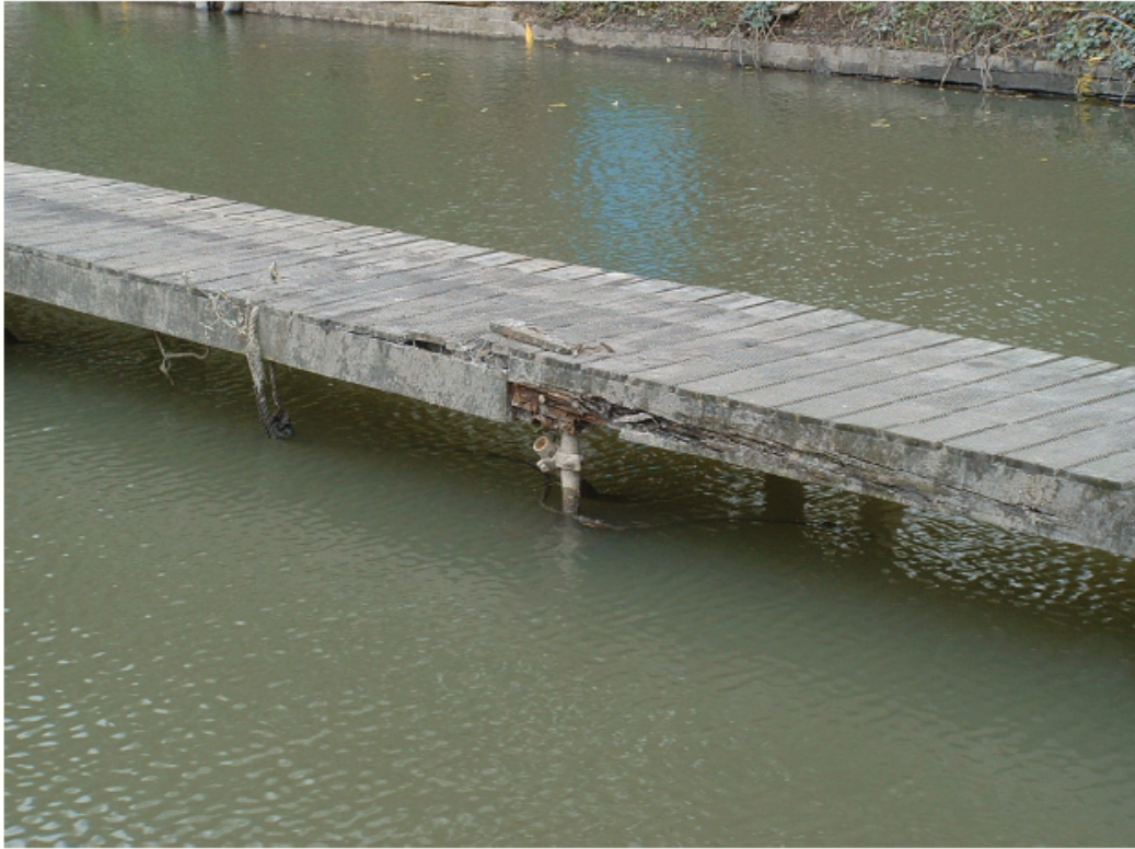
Photo 31 The timber walkway is in poor condition over the second support from the south
