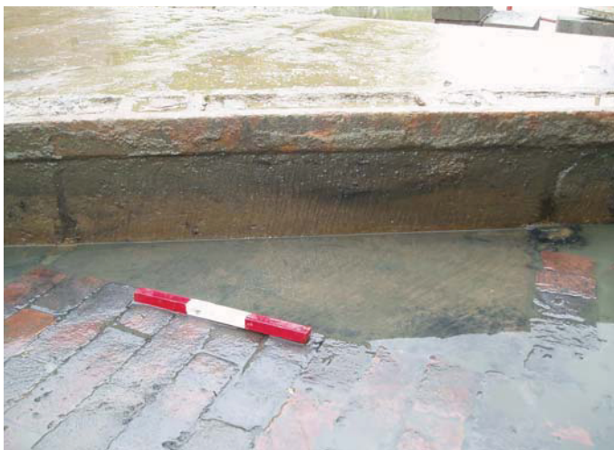
Figure 12: Iron clad rebate in Sandstone flags
