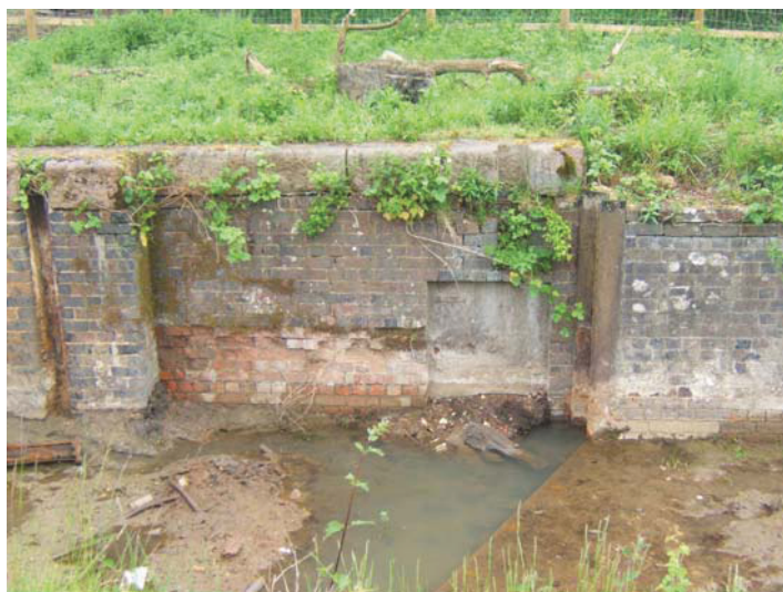
Figure 15: Chamber wall condition. May 2006
