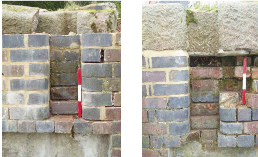
Figure 8: Recesses for Paddle Gear (damaged eastern wall to the right).
