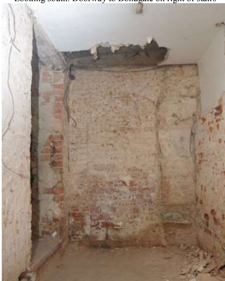
Figure 23 West wall of kitchen corridor Looking west. Note archway and stone to right of arch
