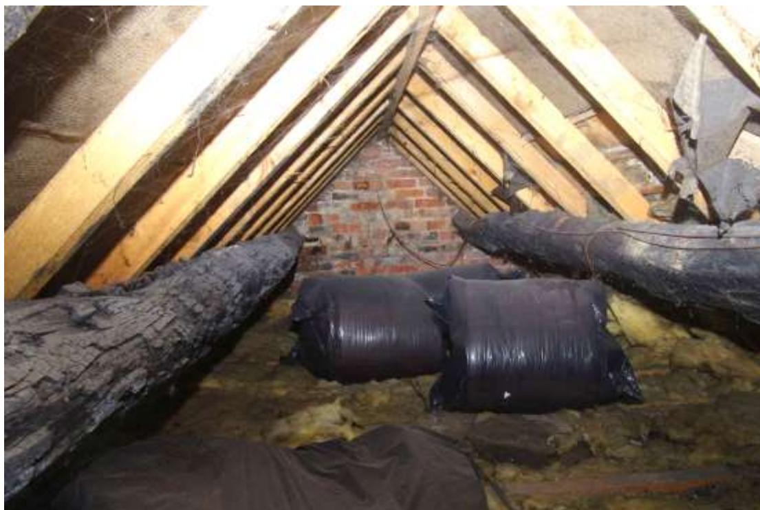
Figure 31 Roof space above Bedroom 18 Looking north. Note charring on left-hand purlin
