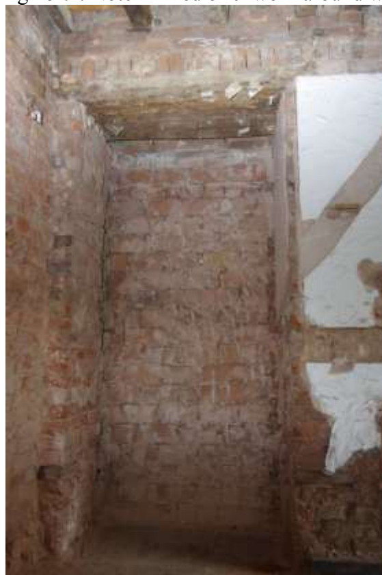
Figure 17 Lounge 1, blocked doorway to north of chimney breast Looking east. Compare with Figure 14
