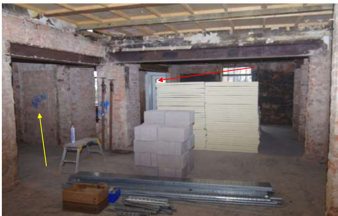
Figure 15 View of corridor wall stubs from lounge 3 Looking west. Lounge 2 behind stack of plasterboard. Original front door arrowed. Blocked doorway into Lounge 1 shown with yellow arrow
