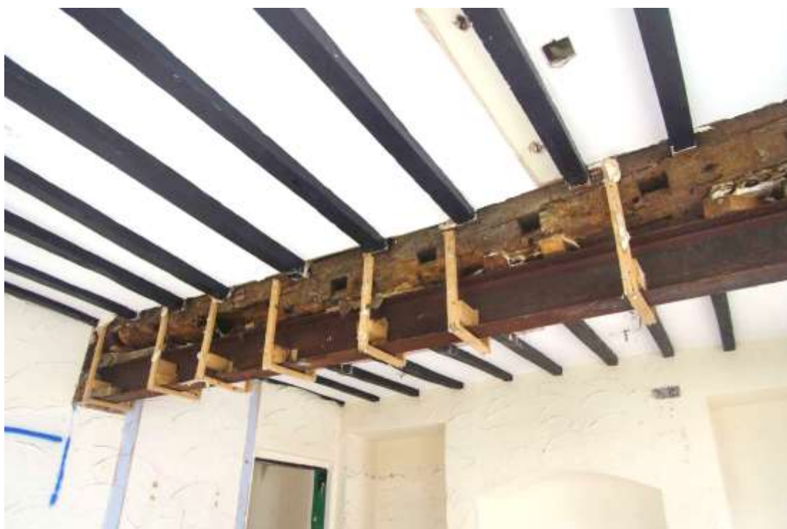
Figure 26 Supported timber beam with redundant sockets Looking north-east from the SW corner of Bedroom 16 towards fireplace in Bedroom 17 following the removal of the partition wall
