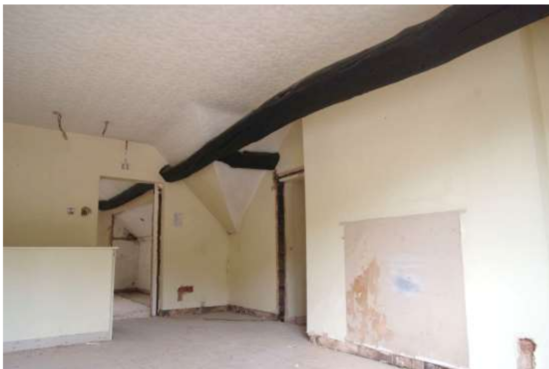
Figure 28 Second floor, former lounge Looking north-east. Stairs on left, bedroom in centre, toilet on right
