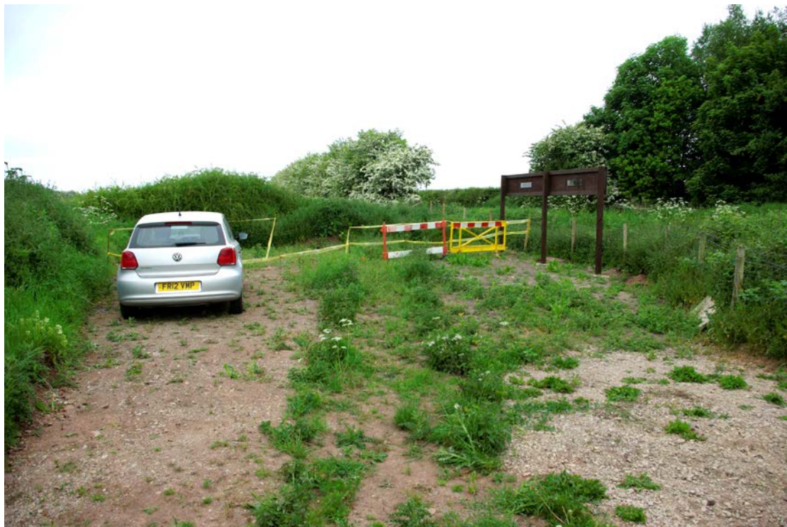
Figure 3 Ilott Wharf cleared area Looking north-west. Bosworth Road on right behind the brown sign. The brickwork exposed by the machine was protected behind the temporary barriers
