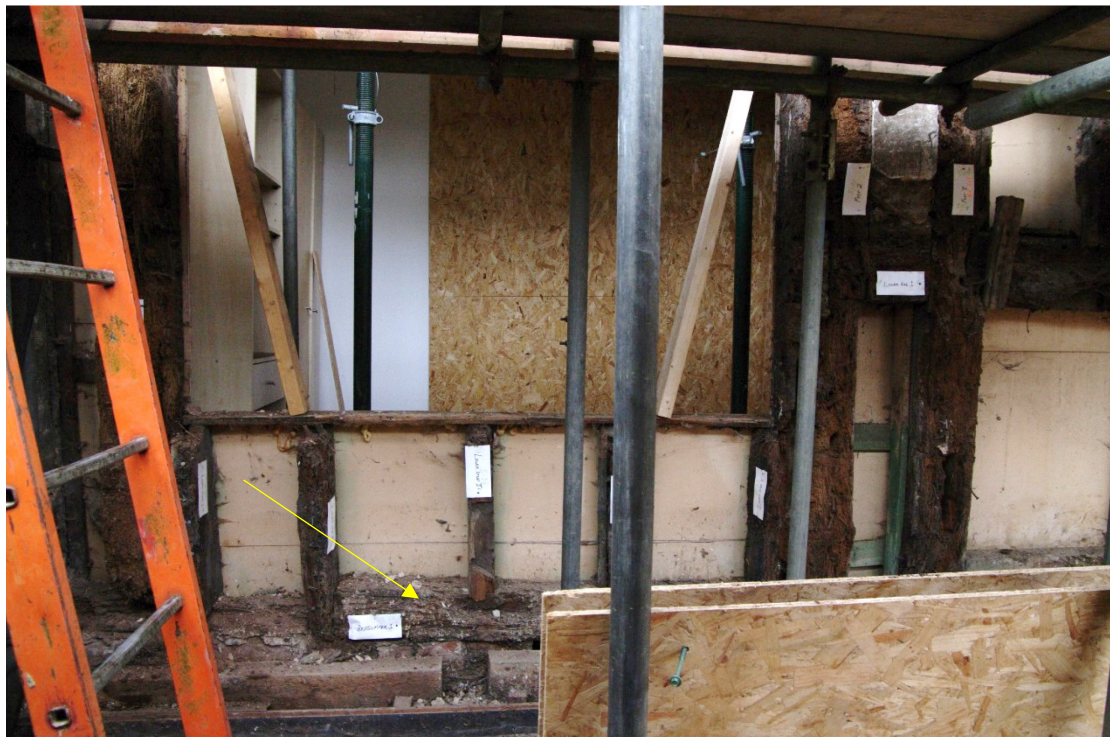
Figure 5 First floor, bressumer beam 1 Beam arrowed. Note Georgian window opening cutting across earlier timbers
