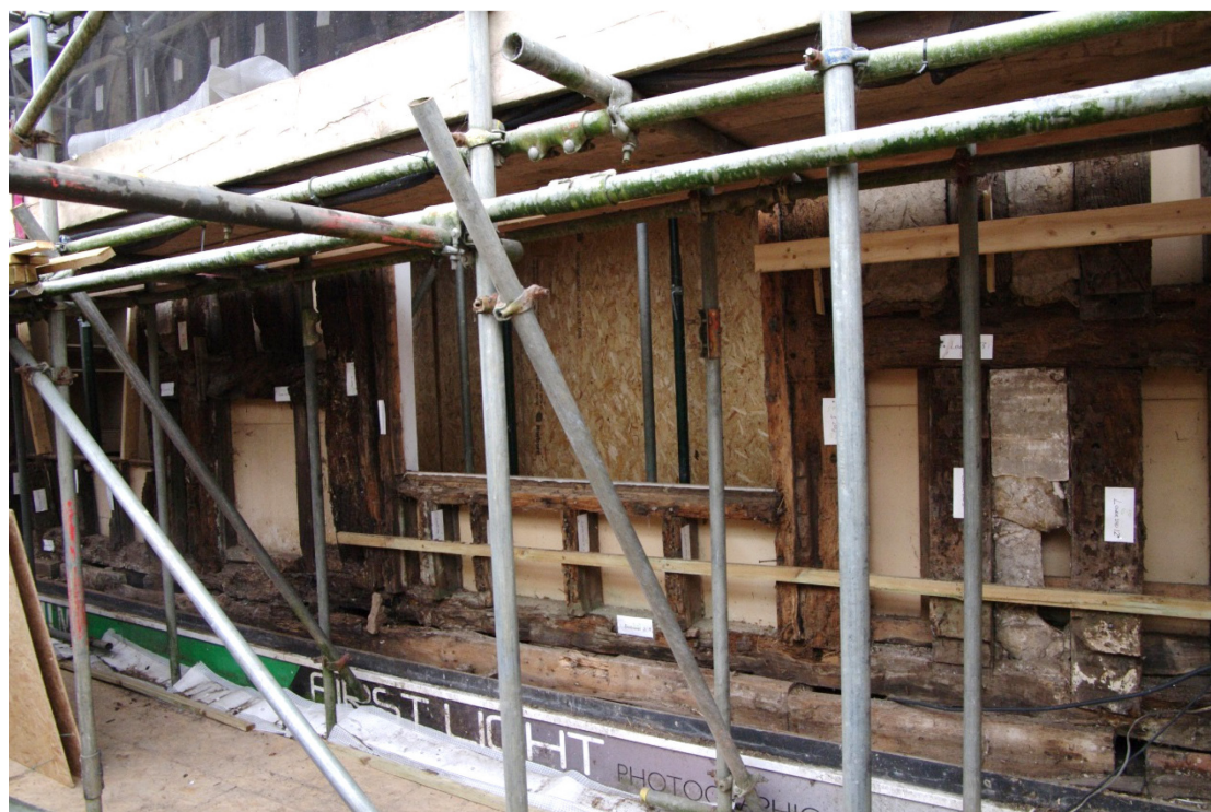
Figure 4 Top of ground floor north elevation with shop sign attached Note also the joints in the bressumer beam 1 behind the shop sign (right side of picture). Viewed from scaffolding
