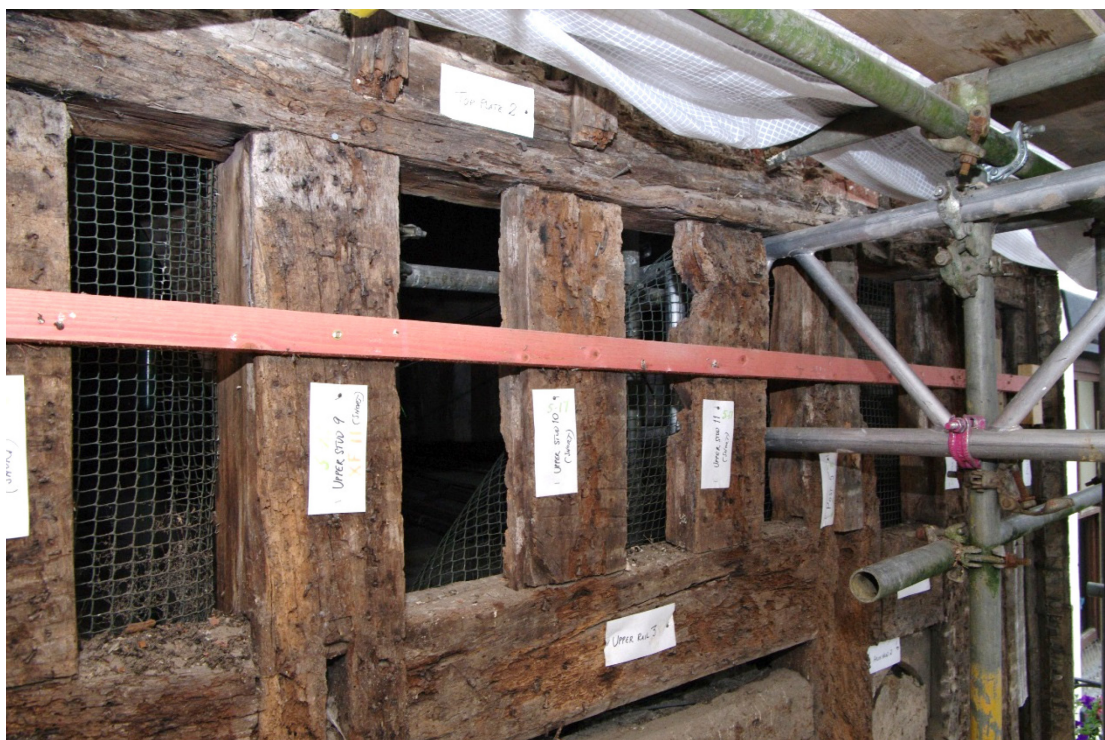
Figure 8 Timber-work near eaves above inserted window Noted pegged joint above closest stud
