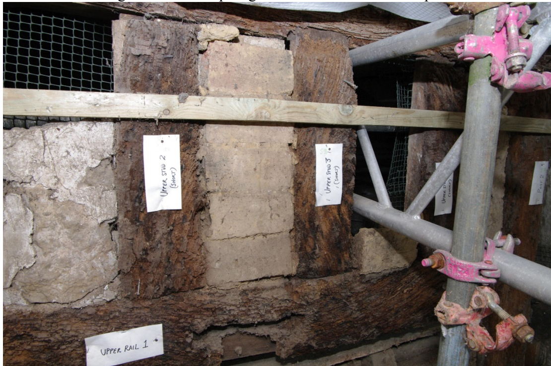
Figure 13 Brick infilled panel close to top eastern corner of frontage The brick infilled panel is the centre panel
