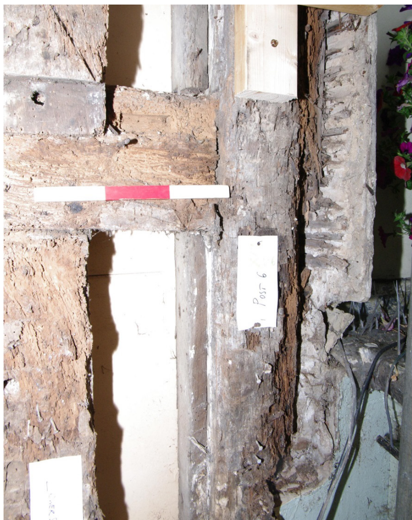
Figure 14 Stub of lath and plaster west wall Adjacent property (Number 5) to right of picture
