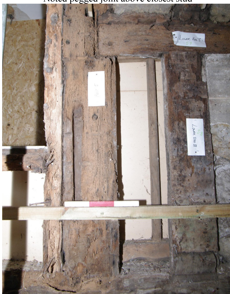
Figure 9 Redundant mortice from probable earlier window Mortice is above the 0.3m scale. Inserted Georgian west window on left
