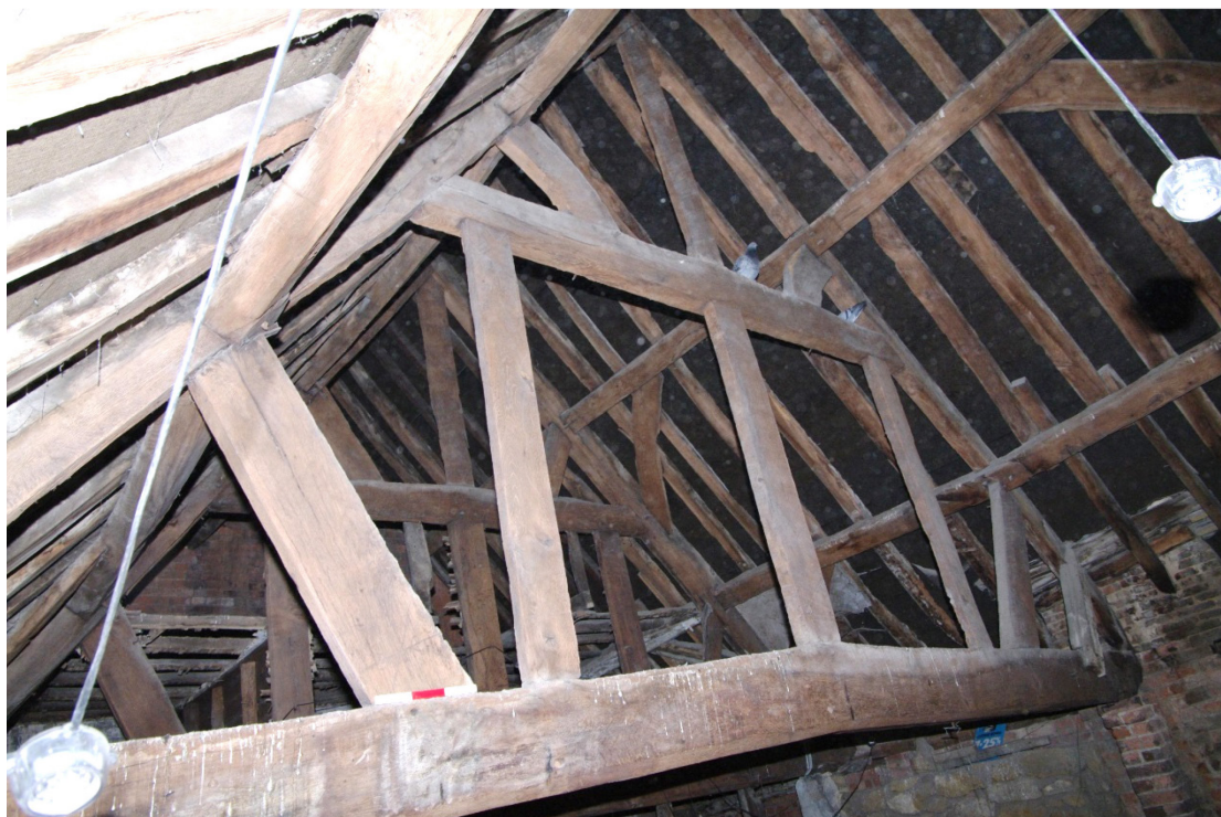
Figure 17 Truss 2 seen from western side Looking south-east. Truss 1 can be seen behind Truss 2
