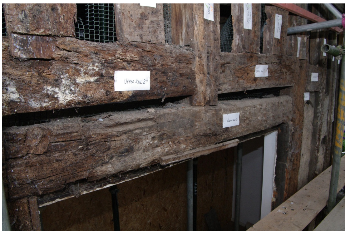
Figure 7 Top of western inserted window Note truncated post supported by inserted lintel beneath Rail 2
