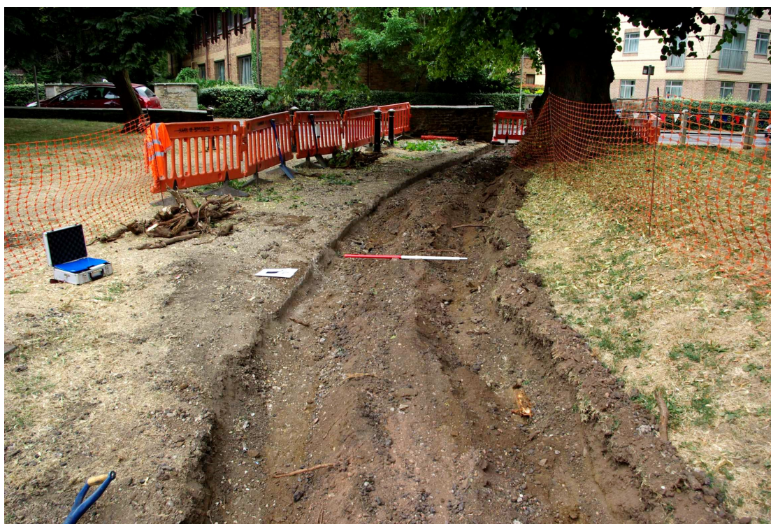
Figure 10 Pathway Stage 1, final excavated level Looking west towards Church Street. 1m scale
