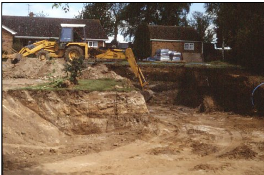
Plate 3. Northern limit of excavation. Redeposited material and sealed topsoil can be seen in left hand section.
