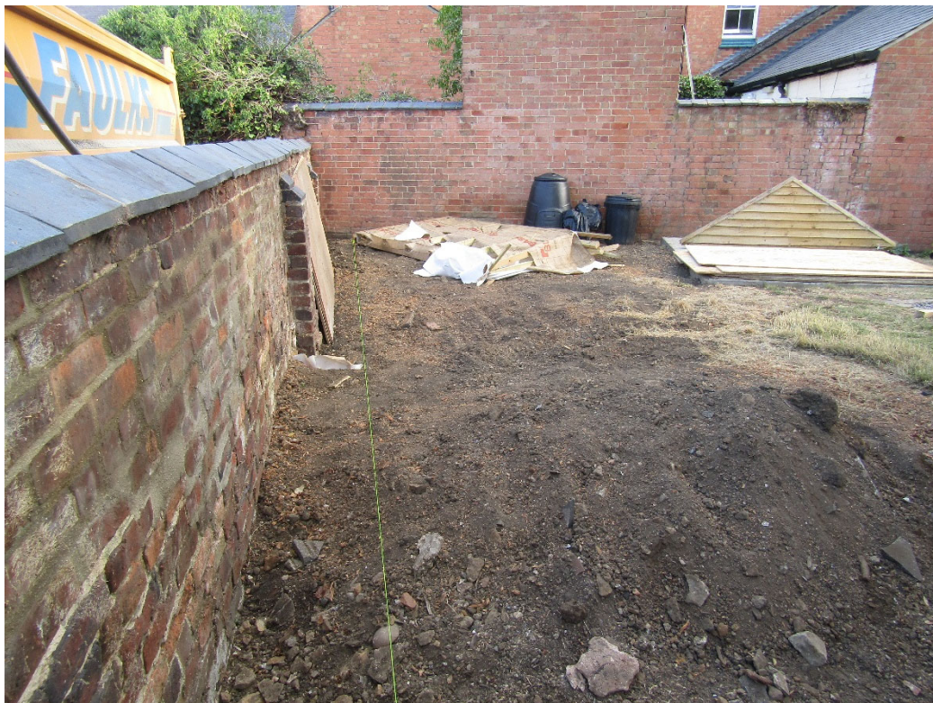
Figure 4: Area prior to excavation looking north. Visible in the photograph is the existing concrete shed base to be removed.
