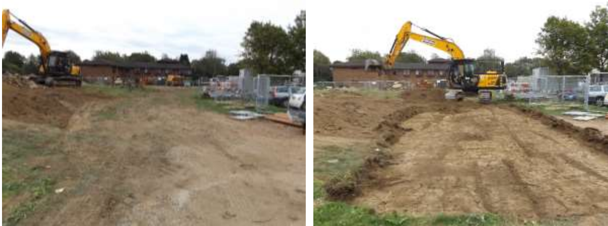
Figures. 4 & 5. The removal of the topsoil and made ground with mechanical excavator
