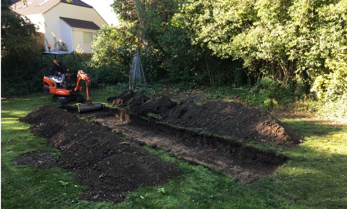
Figure 4: Looking south-west across the application area, with the mechanical digger working at Trench 1.
