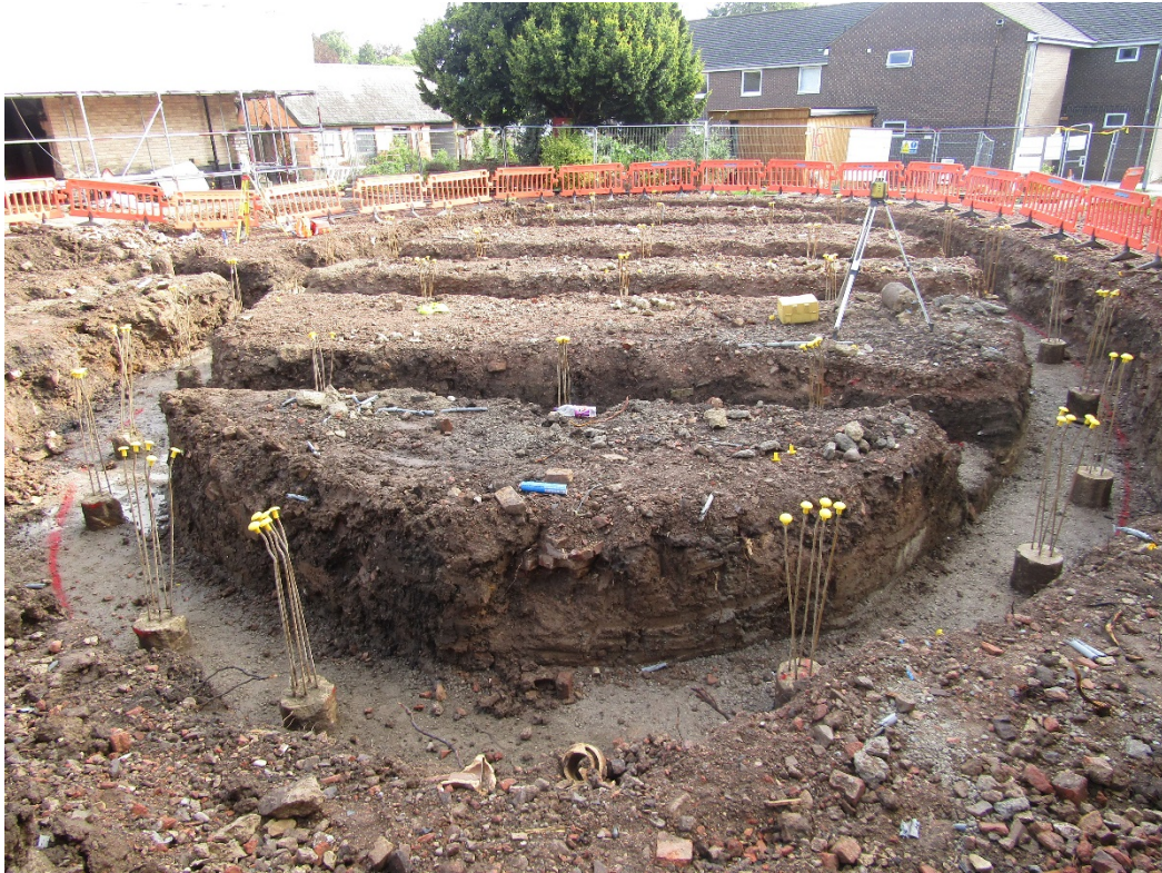
Figure 7: Lower area with foundation trenches opened and layered with concrete in the base. Looking north-east.
