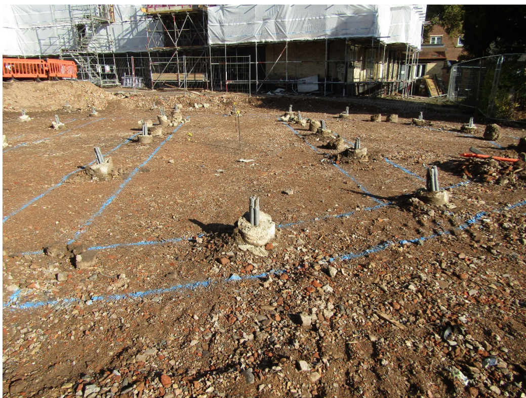
Figure 4: Lower area of site prior to excavations with pilings in situ, looking north.
