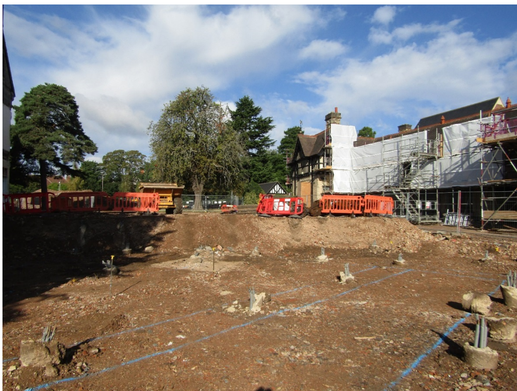
Figure 3: Site looking west, showing pilings and area of made ground under orange barriers.
