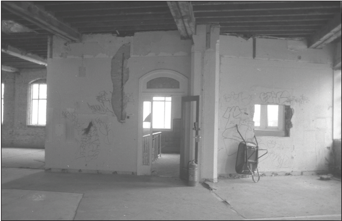
Plate 12 Deacon St range, east end looking north. Office (to the right) and stairwell (straight ahead)
