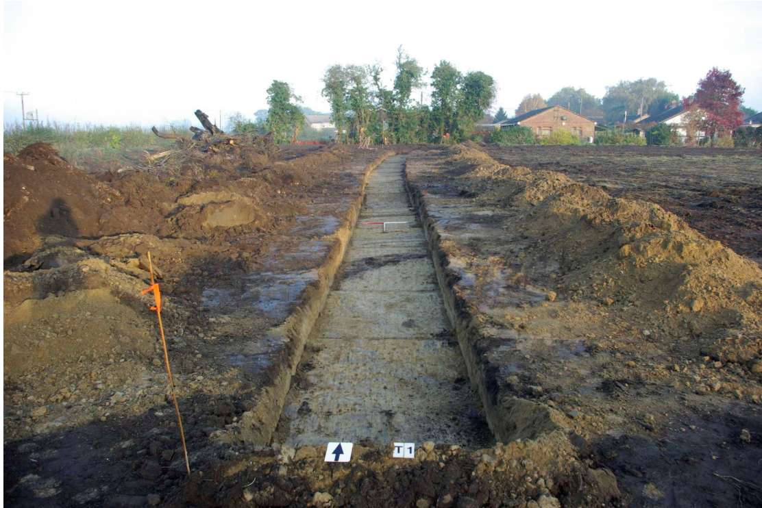
Figure 11 Trench 1 1m scales. Root disturbance seen as a dark band in the foreground
