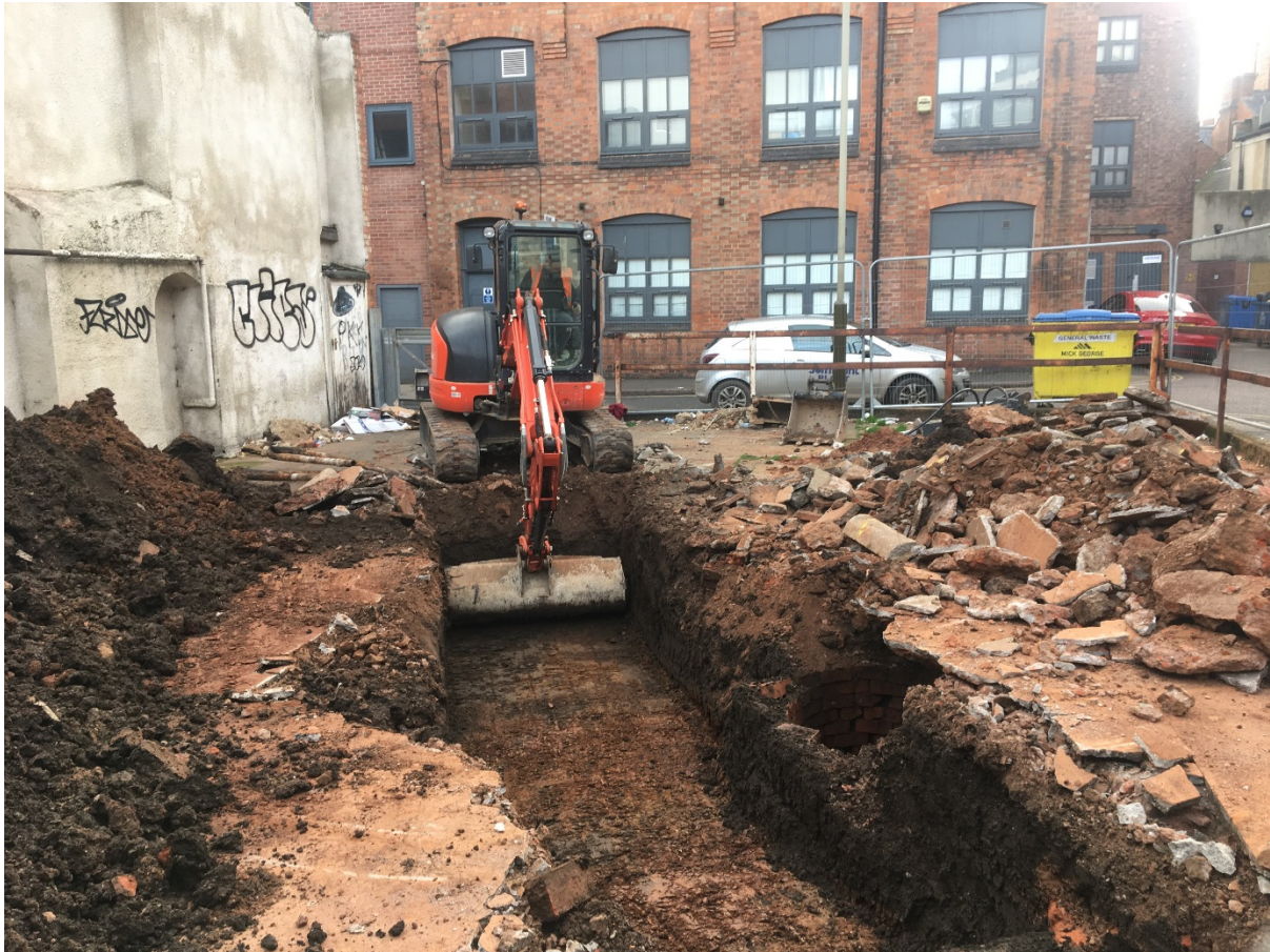
Figure 2: Looking south-east across the development area, with the mechanical digger excavating Trench 1.
