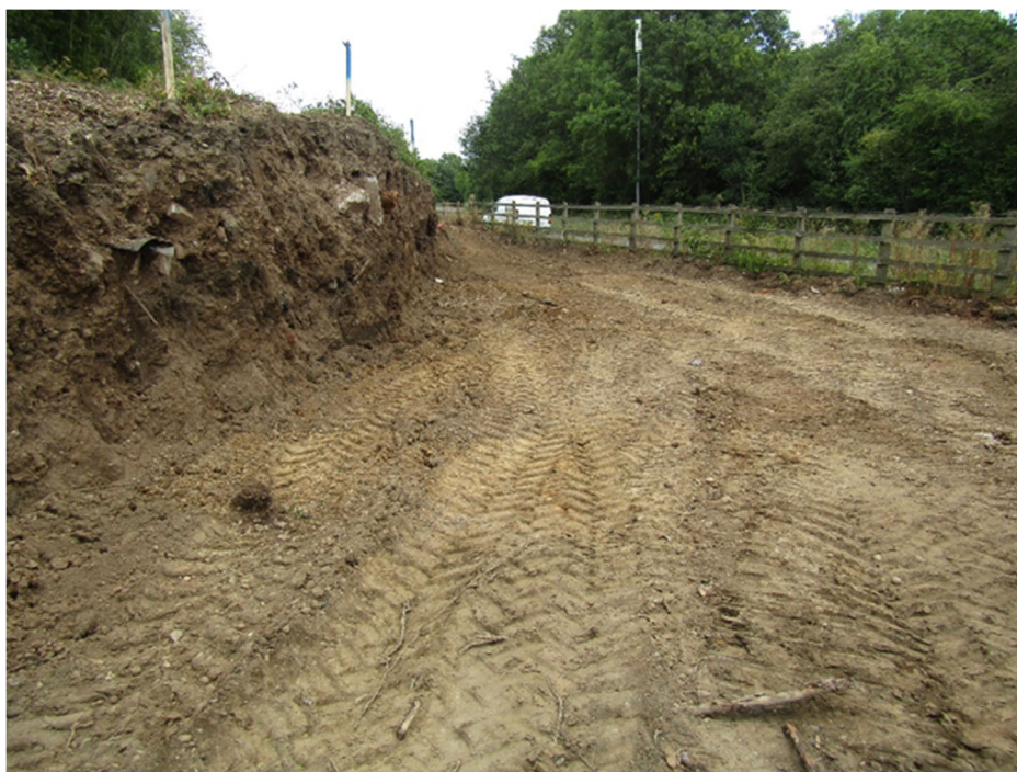
Figure 9: Area 2a east of bridleway looking east prior to stripping after the partial removal of the bund.
