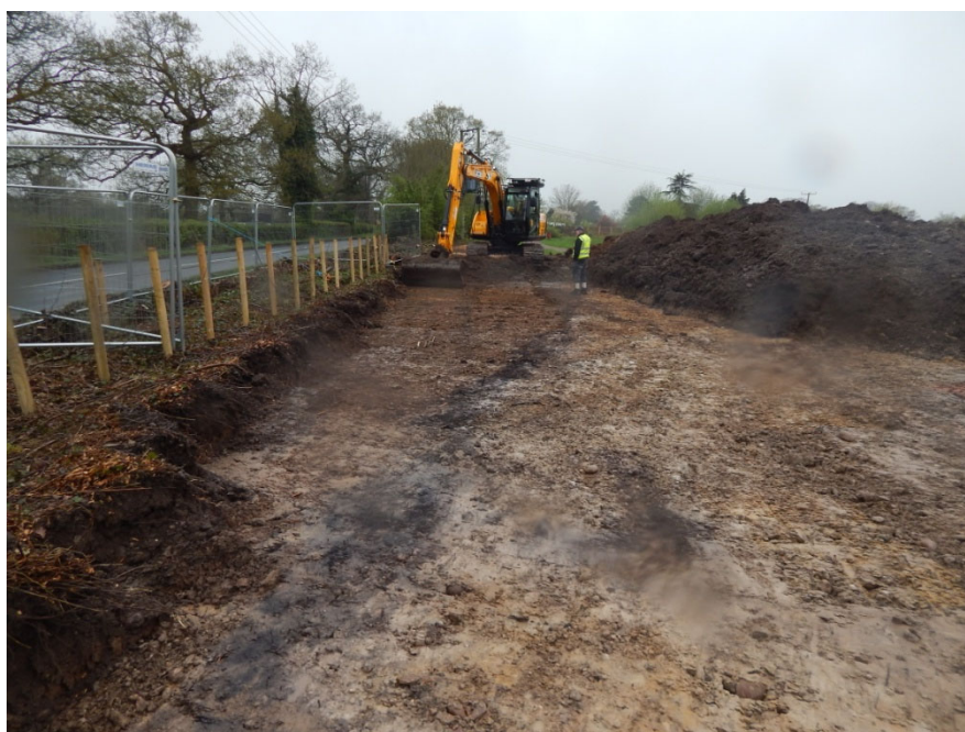
Figure 8: Top-soil stripping in progress along Kineton Road showing possible trackway of Post- medieval date. Looking west.
