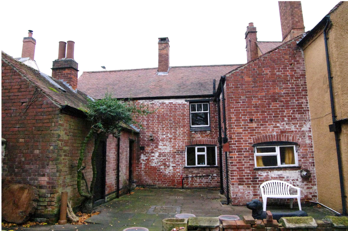
Figure 14 Proposed location of new single storey extension Looking north-west. Store and wash house on left. 1m scale
