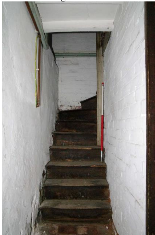
Figure 23 Stairs to west of scullery up to first floor Looking south-west. 1m scale
