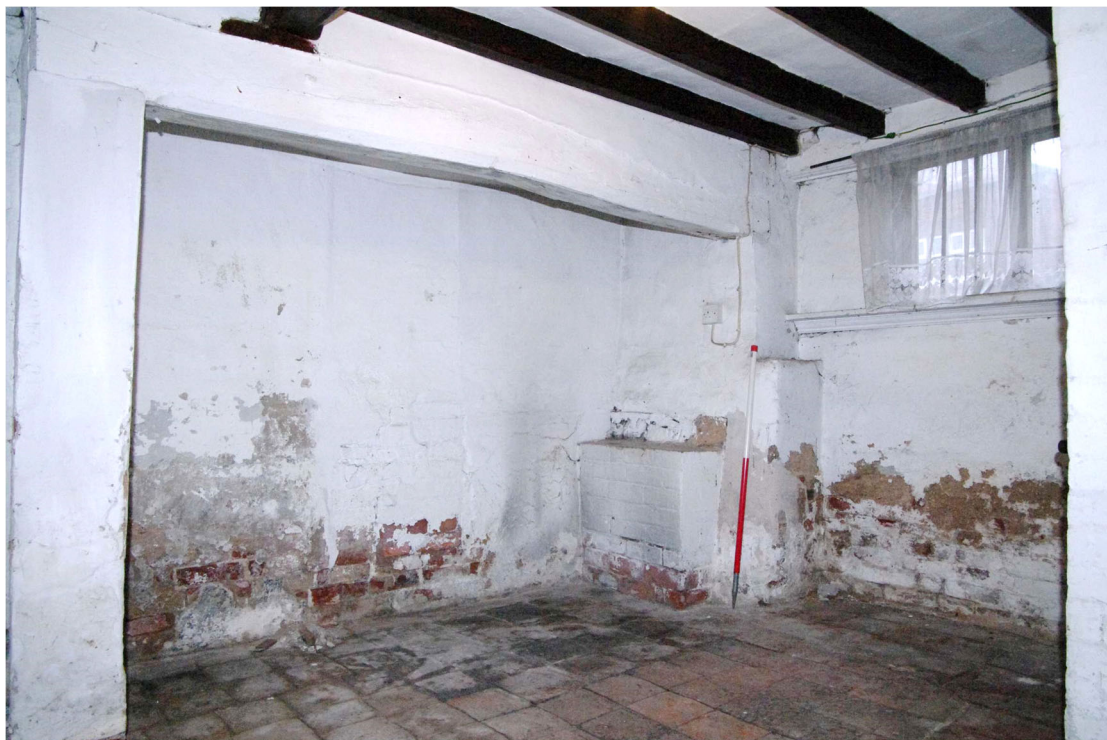
Figure 24 Scullery fireplace Looking west. 1m scale. Window to Main Street on right.
