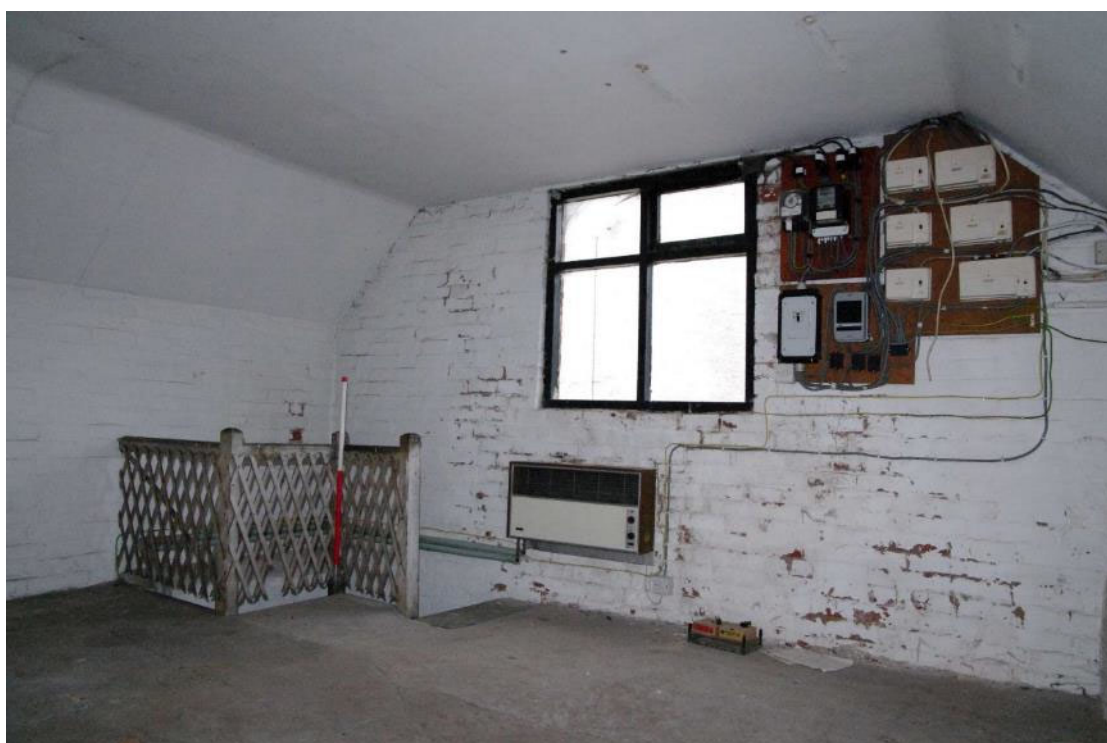
Figure 42 First floor western room Looking south towards stairs (see Fig. 23). 1m scale
