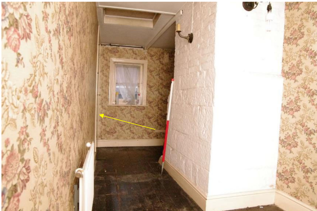
Figure 44 First floor, landing and chimney stack above kitchen Looking north-west. Door to stairs shown in Fig. 27 arrowed. 1m scale
