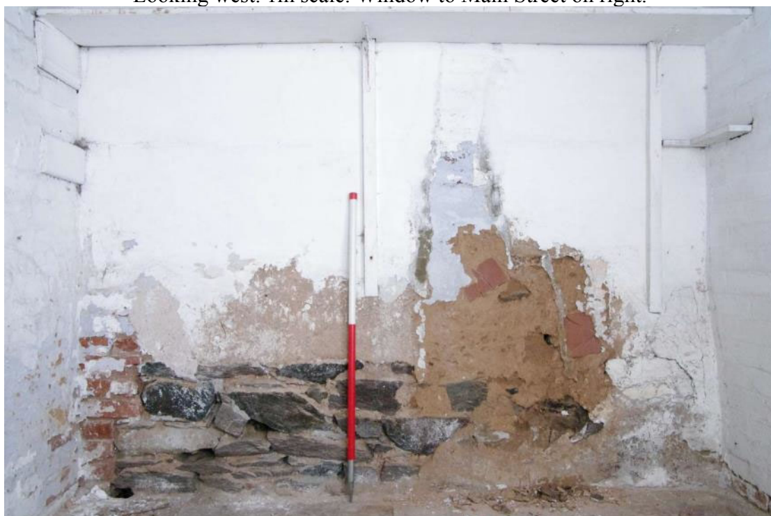
Figure 25 North-east wall of scullery Stone base, brick and mud patching. Looking north-east. 1m scale
