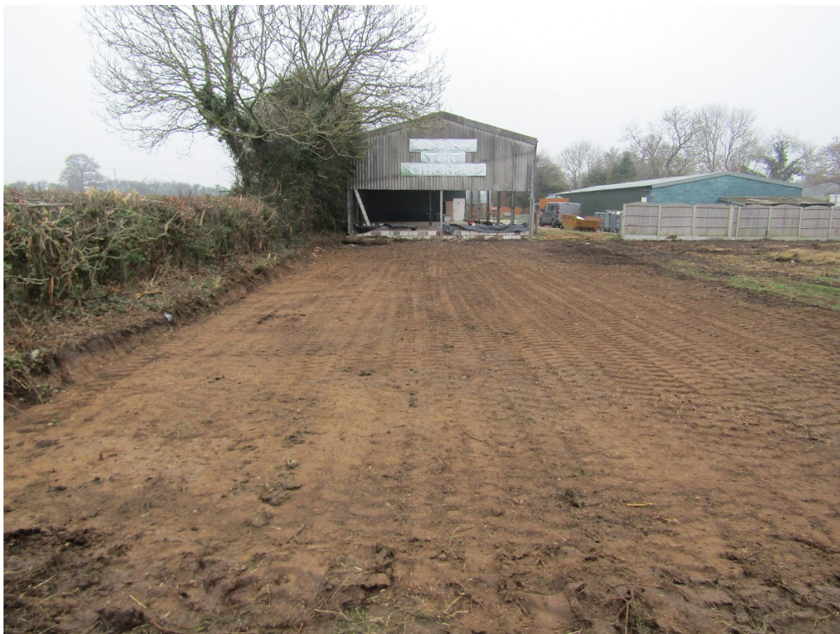
Figure 6 Completed area of groundworks. Shallow intrusion into top and subsoil visible on the left.
