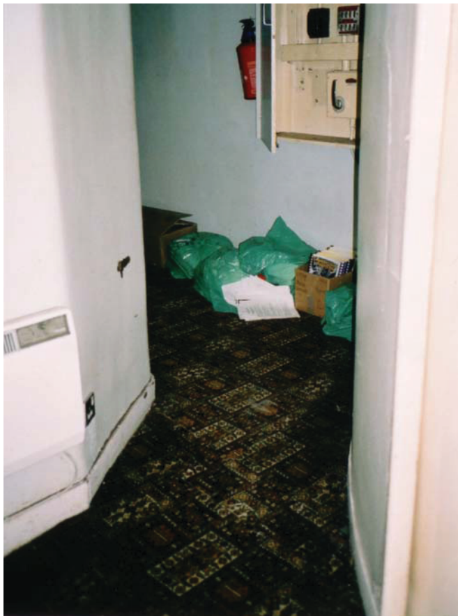
Plate 5 Second floor corridor at point where the Fire Door is to be installed. The curved section on the extreme right is the partitioning of the orchestra balcony.
