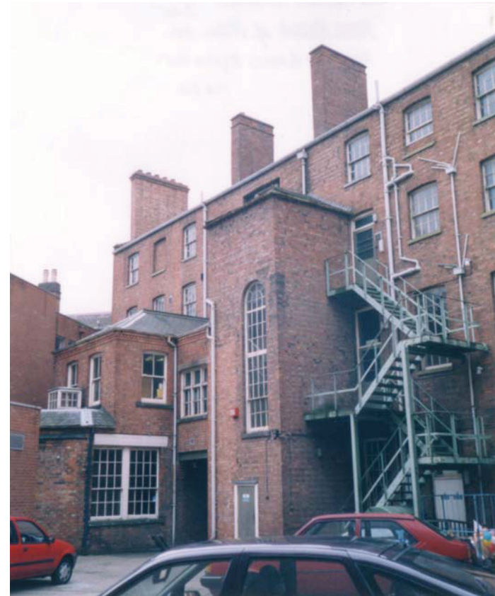
Plate 4 Rear view of the City Rooms showing the brick outshoot for the service staircase with deep sash window and later brick outshoot additions for the kitchen block and mezzanine office. Also shows the array of sash windows on this elevation.
