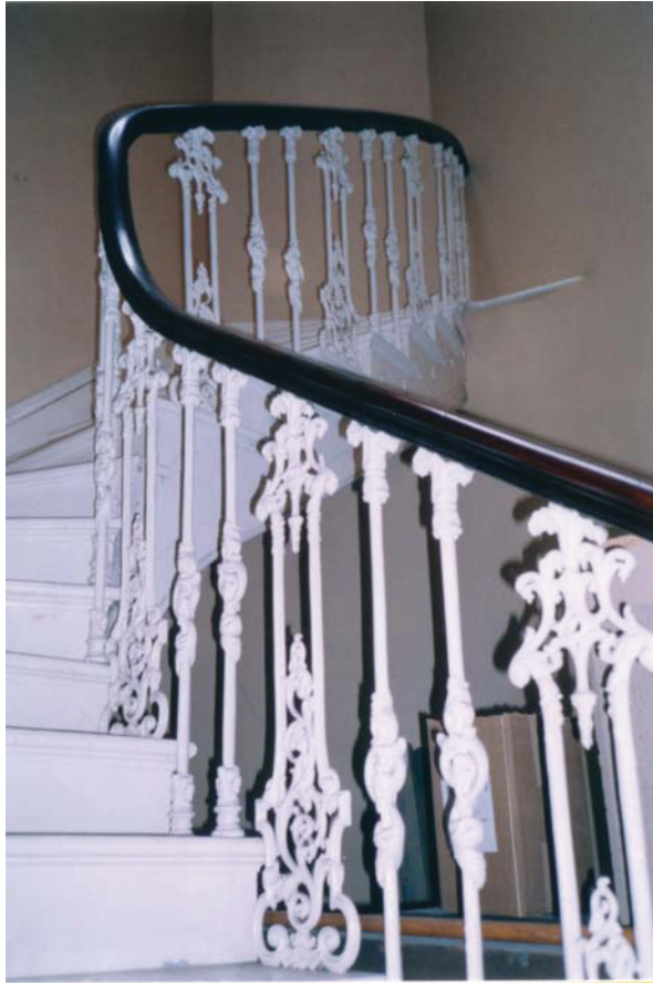
Plate 1 Cast iron balustrade with moulded handrail rising from Ground floor lobby area to blocked doorway at First Floor Level
