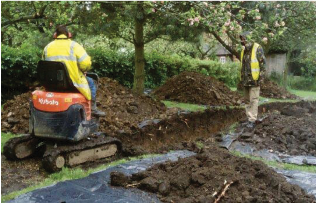
Plate 1 excavation of Trench 1. The earthwork can be seen rising and falling in the far section.
