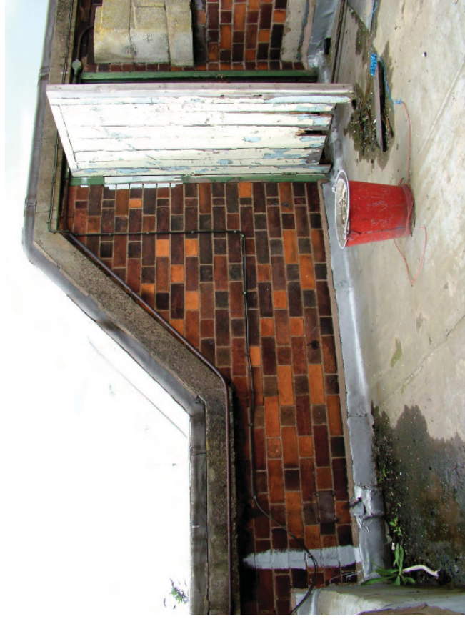
Plate 11: Lift gear housing
