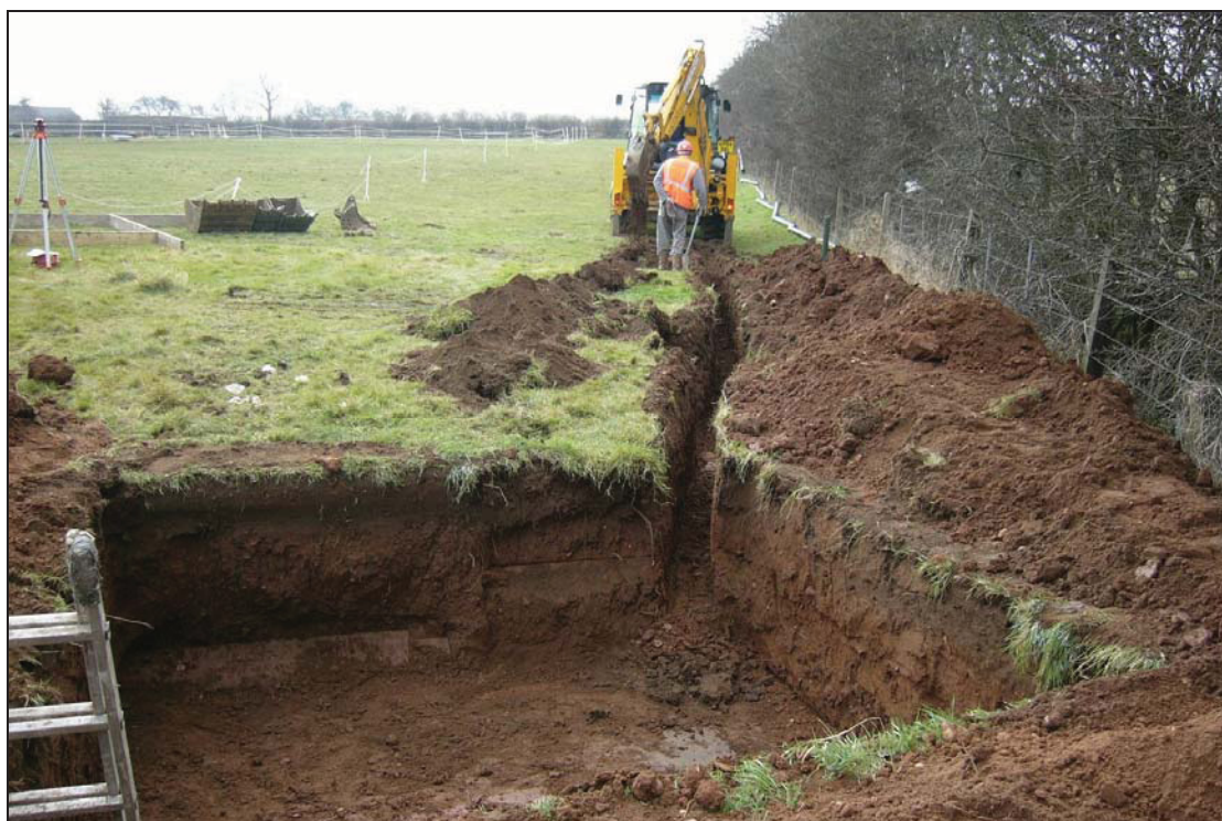
Plate 2: General view north from mast base footings trench along the cable trench
