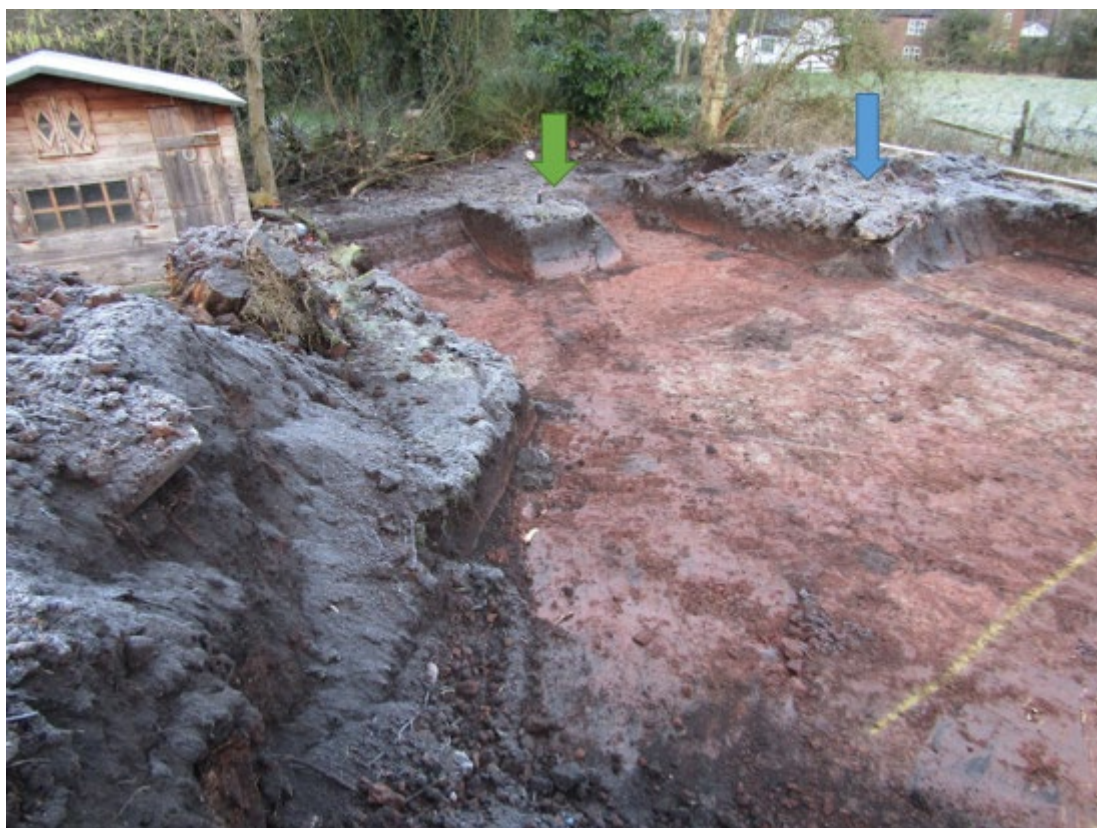
Figure 7: Site looking north-west. Area indicated by blue arrow contained asbestos. Area indicated by green arrow contained geotechnical gas collection unit.
