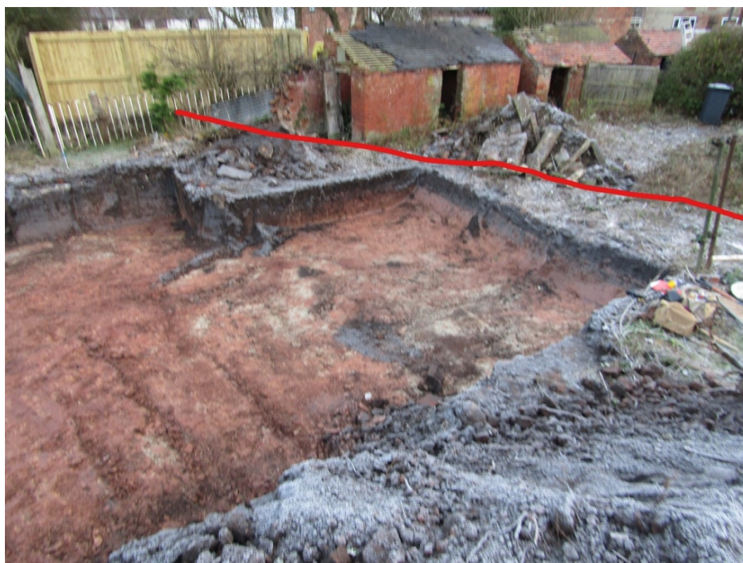
Figure 8: Site looking north-east with approximate line of overhead cable indicated in red.
