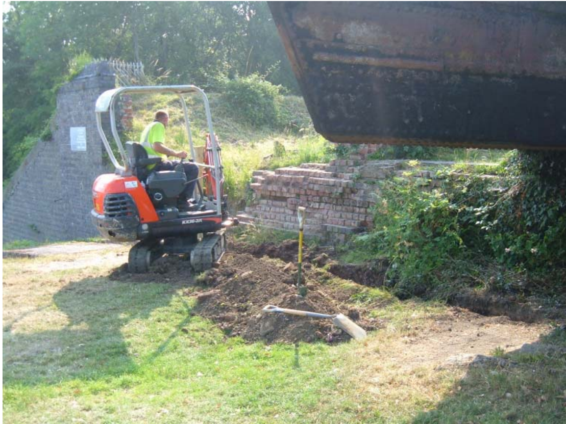
Plate 1: Work in progress on badger fence close to abutment wall, looking southeast
