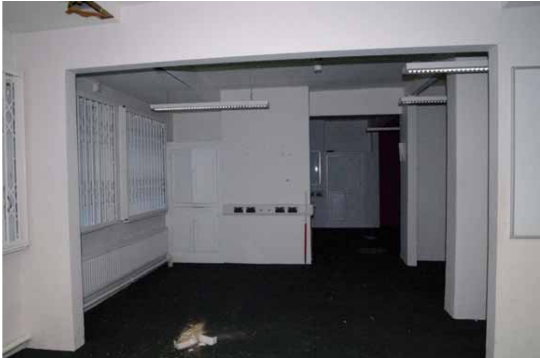
Figure 36 Rooms G3 and G4 Looking south-east showing stubs of original dividing walls. 1m scale
