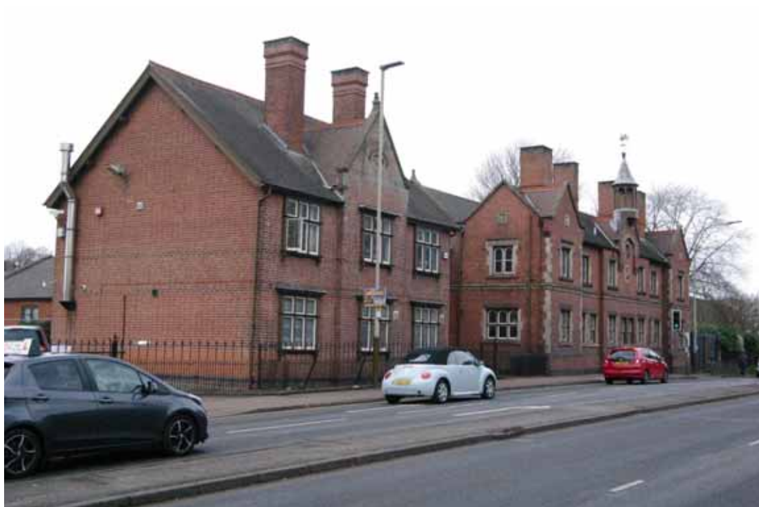
Figure 12 North-east facing elevation Looking west. 1893 block in foreground, 1856 block on right Note faint band of diaper work in brickwork
