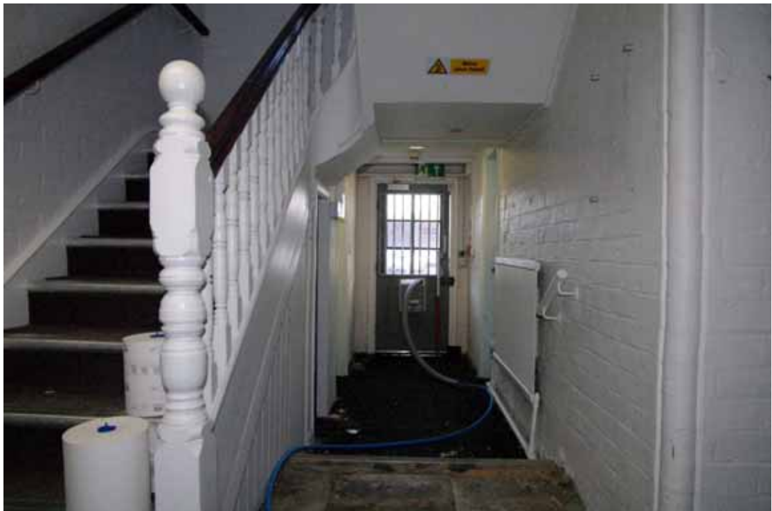
Figure 43 G9 stairs and doorway to rear of 1856 block Looking south-west. 1m scale
