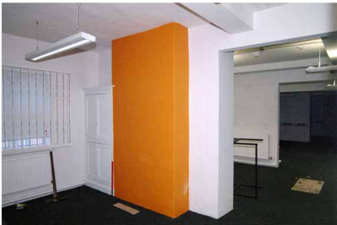
Figure 32 Ground floor Room G1 Looking east. 1m scale. Note how dividing wall has been removed to show Rooms G2, G3 and G4 to right. Original cupboard in corner by window
