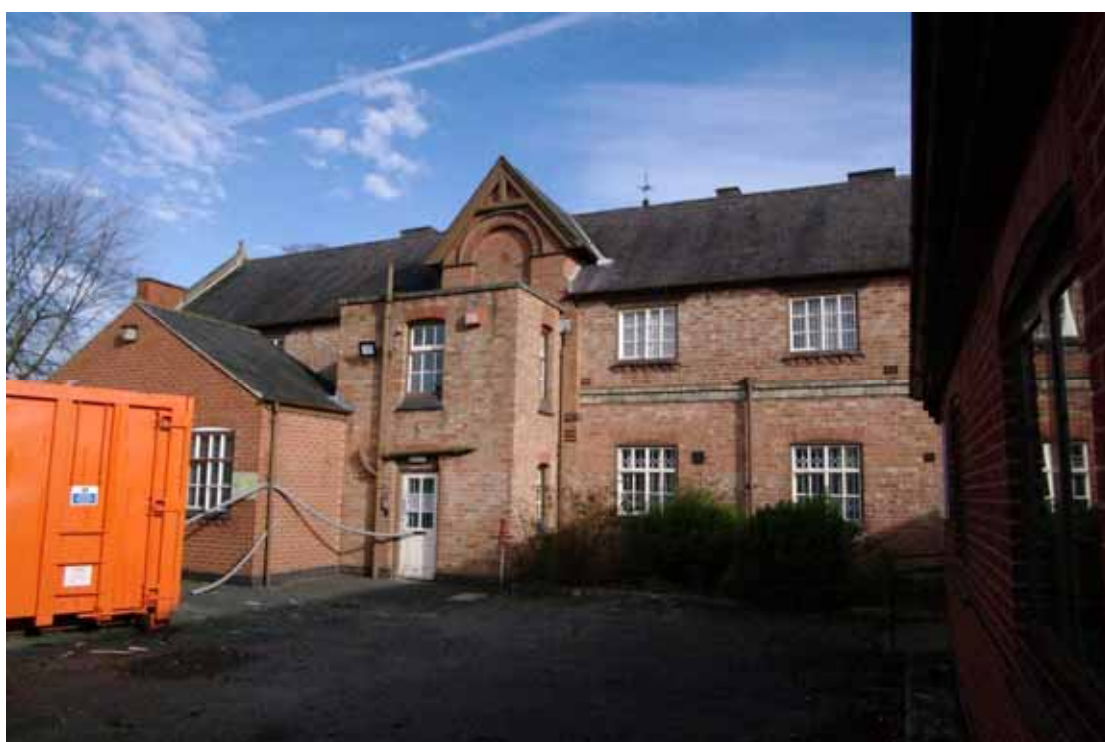
Figure 22 South-west facing elevation of 1856 block Looking north. Modern office extension on left behind skip. Modern medical extension on right. Note brick-built toilet extension of 1940s/1950s date
