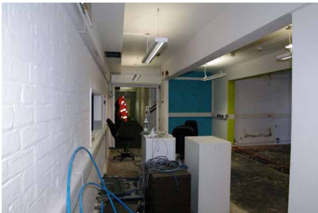
Figure 39 Corridor G9 Looking south-east. Knocked-through wall to rear rooms on right and modern office extension to right of green wall stub
