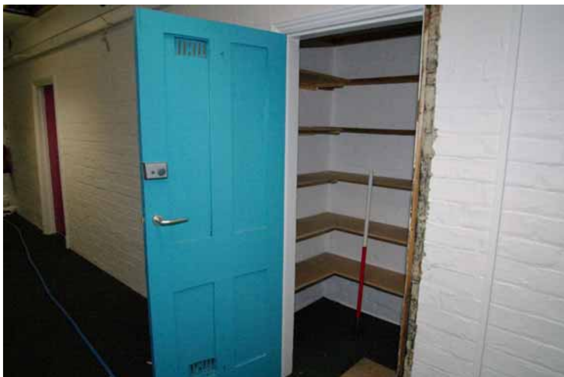
Figure 46 Store off corridor G13 Looking north. 1m scale. Note: removal of door surround has exposed original green and cream paint scheme
