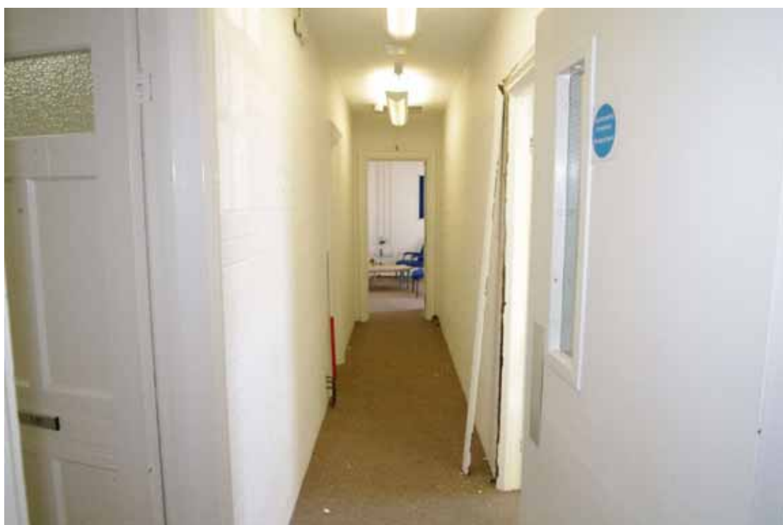
Figure 77 Corridor F21, 1883 block Looking south-east. 1m scale. Door to F17 first left
