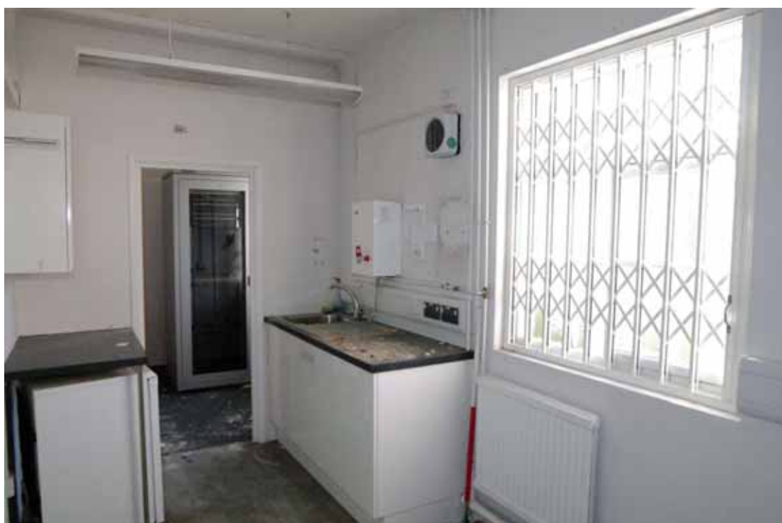
Figure 47 Room G10 Looking south to doorway to Room G11. Horizontal sliding sash window on left
