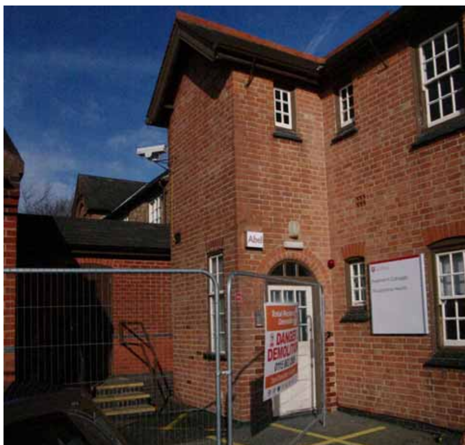
Figure 28 Toilet block on south-west facing elevation of 1893 block Looking north. Link to modern extension on left
