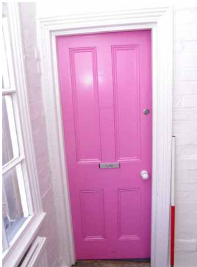
Figure 63 First floor 1856 block, door to Room F1 Looking north-east from corridor F10. 1m scale
