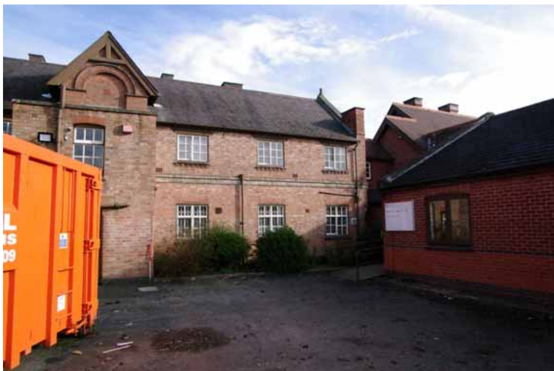
Figure 23 South-west facing elevation of 1856 block Looking north-east. Modern office extension on left behind skip. Modern medical extension on right.
