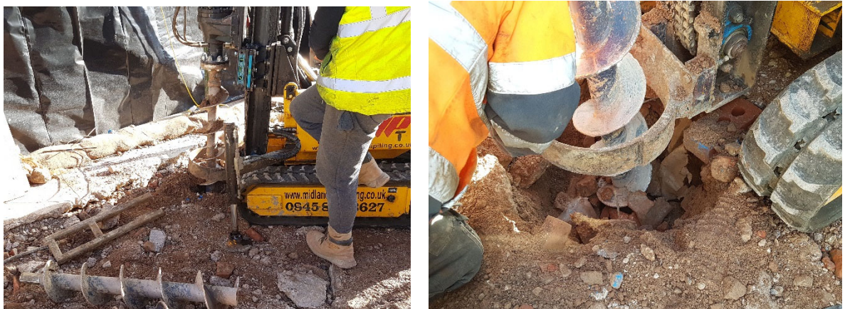
Figure 7. The drilling for the piles being monitored and the subsiding of the boreholes
