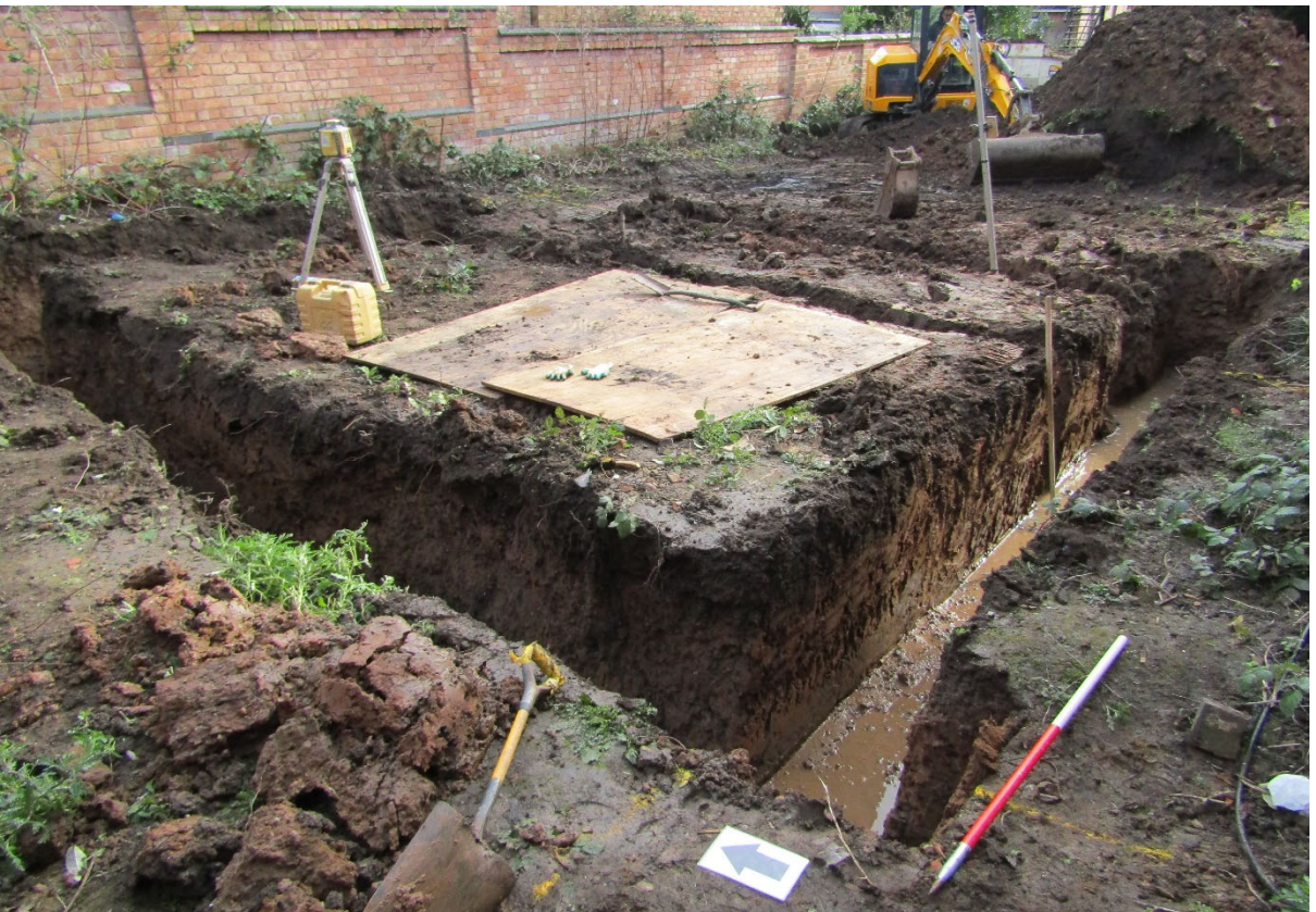
Figure 8: Foundation trenches looking north-east from south-west corner of the development (1m scale).
