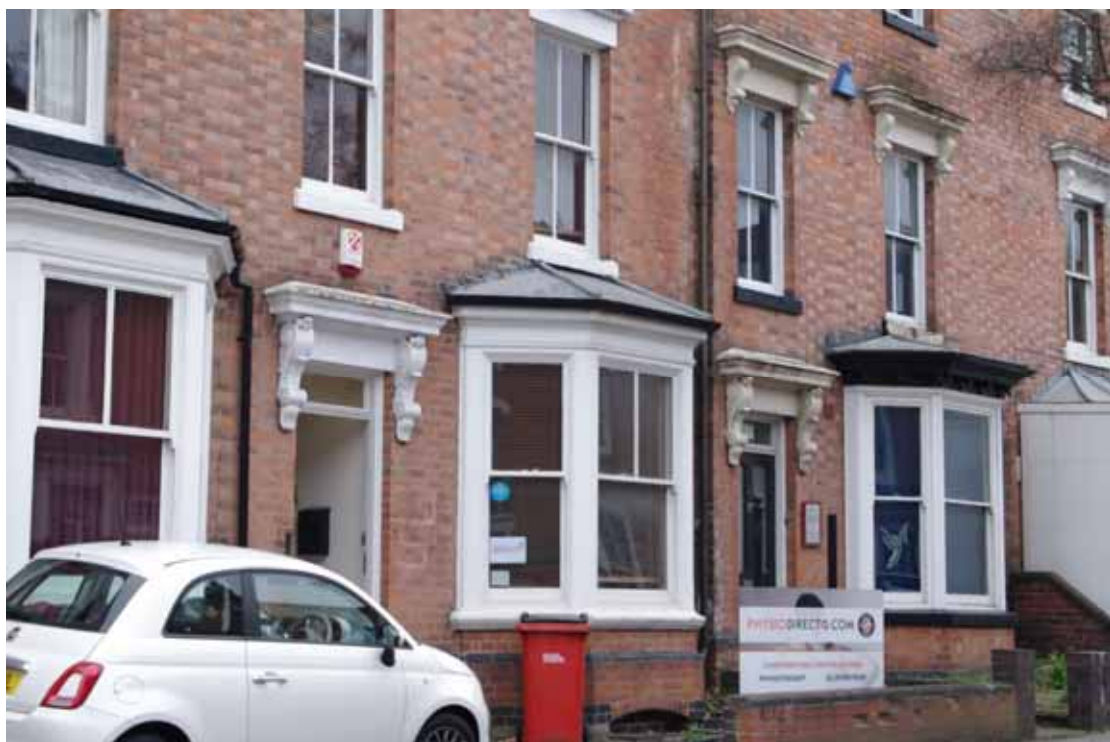
Figure 9 Ground floor bay windows of 8-10 De Montfort Street These appear to be un-modified versions of what would have existed at 12-16 Looking south
