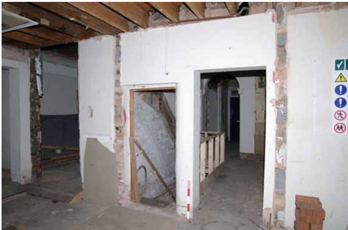
Figure 29 Ground floor rear extension behind Numbers 12 and 14 Looking west. Centre doorway leads down to cellar of Number 12
