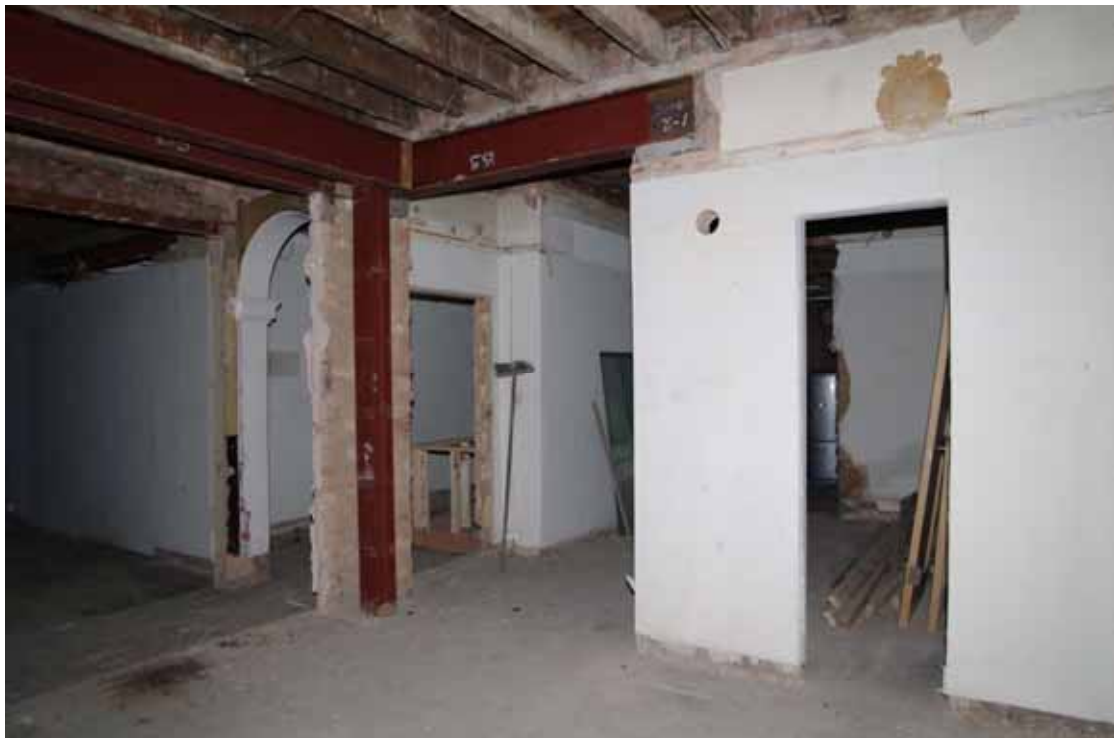
Figure 31 Number 14 ground floor front room Looking east. Modern steelworks shows where the adjoining wall to Number 12 has been removed. Note removed plaster decoration and picture rail on right of picture
