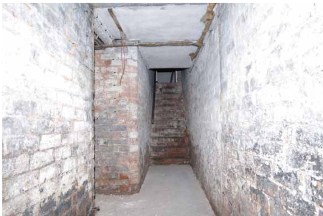
Figure 18 Stairs up to ground floor from cellar of Number 16 Looking south-east from coal cellar
