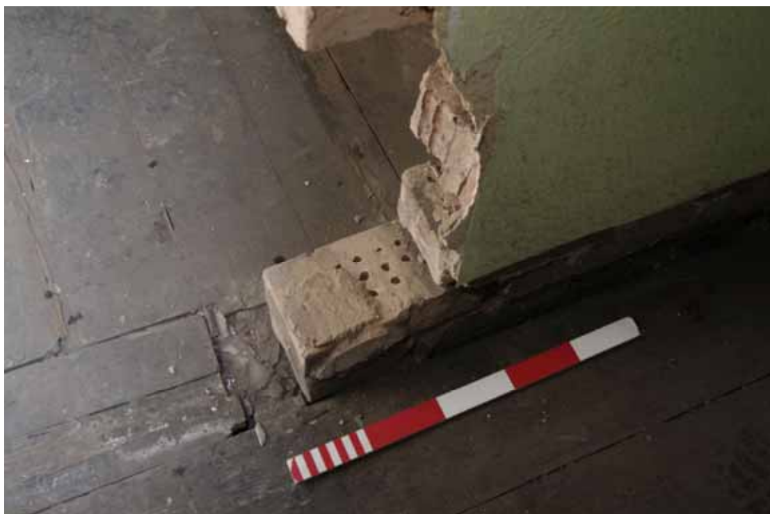
Figure 66 Number 16 second floor brick detail This type of perforated brick appears to be used throughout the terrace
