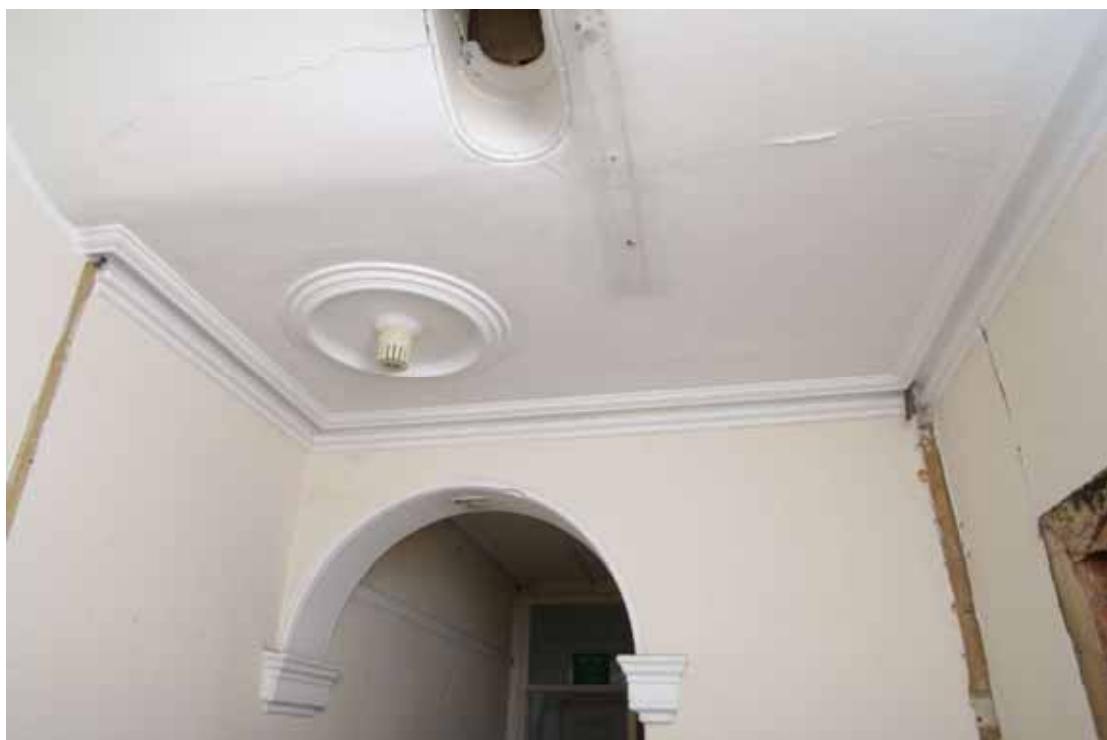
Figure 42 Number 16 ground floor plasterwork detail Looking at plaster beneath the staircase. Hallway to front door on left
