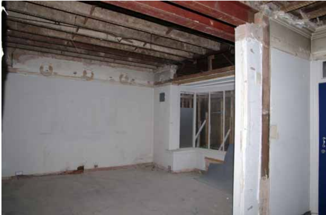
Figure 30 Number 14 ground floor front room Looking west from hallway of Number 12 through modern opening
