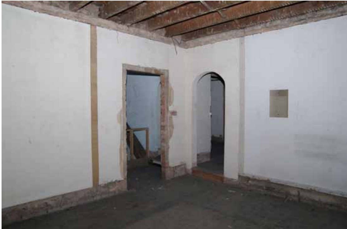
Figure 46 Number 12 first floor front room Looking south. Round-headed door is a later insert to connect with Number 14
