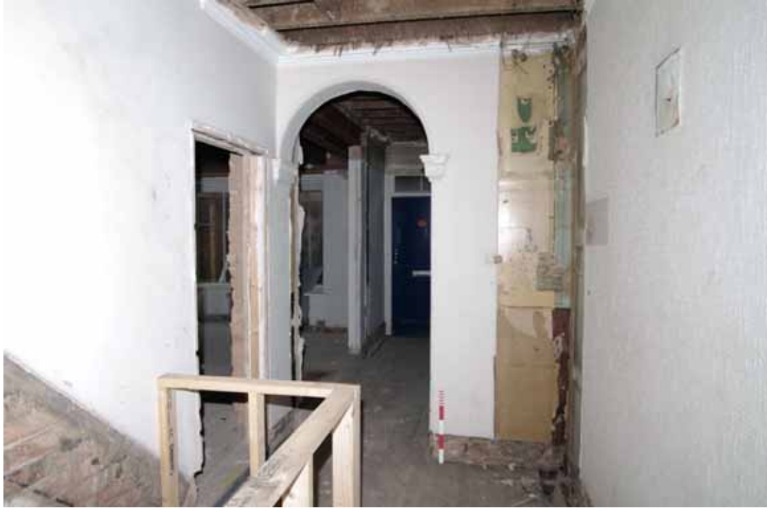
Figure 24 View into hallway of Number 12 Looking west. Openings on right are modern and connect to Number 14. Note decorative plasterwork around archway (see photo 25 below)
