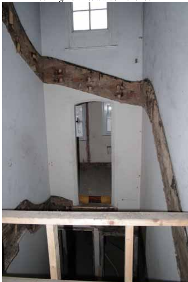
Figure 53 Number 14 removed staircase at first floor level Looking south-east towards doorway to rear toilet block
