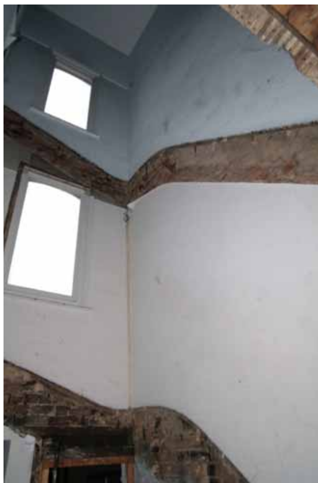
Figure 26 Removed staircase in Number 12 Looking north. Stairs were immediately above the cellar stairs
