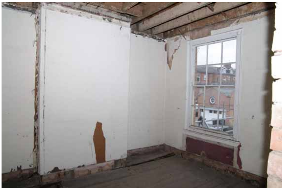
Figure 48 Number 12 first floor rear room Looking east. The stable block can be seen through the window
