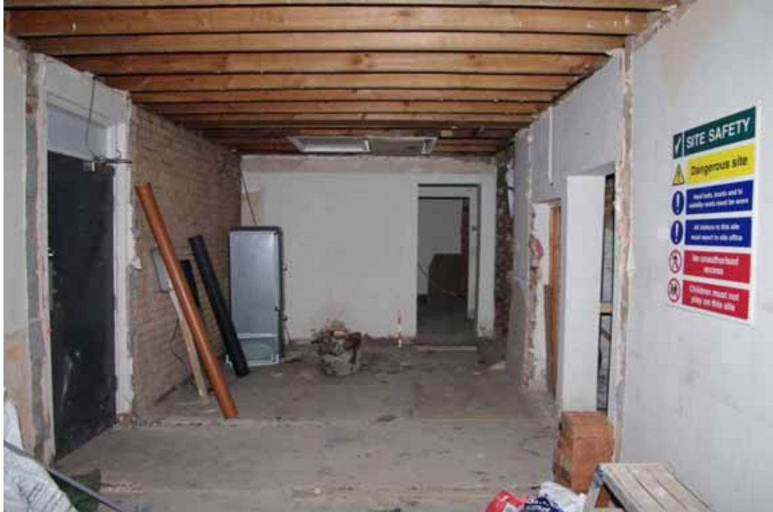
Figure 28 Ground floor rear extension behind Numbers 12 and 14 Looking south-west. This has replaced and enlarges the original rear toilet and wash house of both buildings
