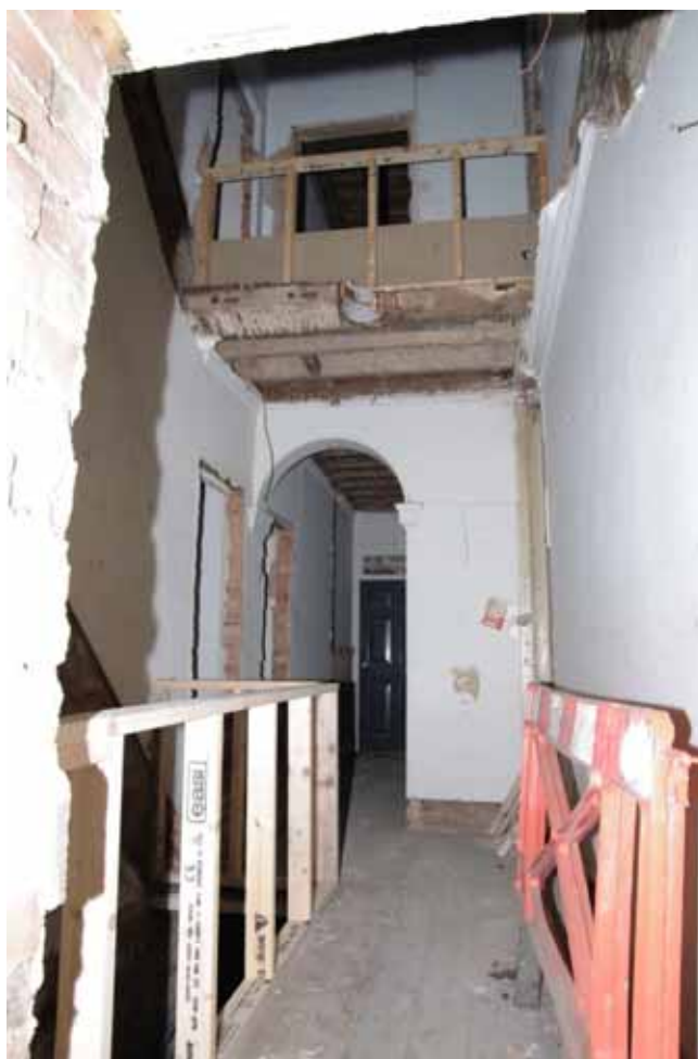
Figure 34 Number 14 hallway through to front door Looking west. Main staircase has been removed
