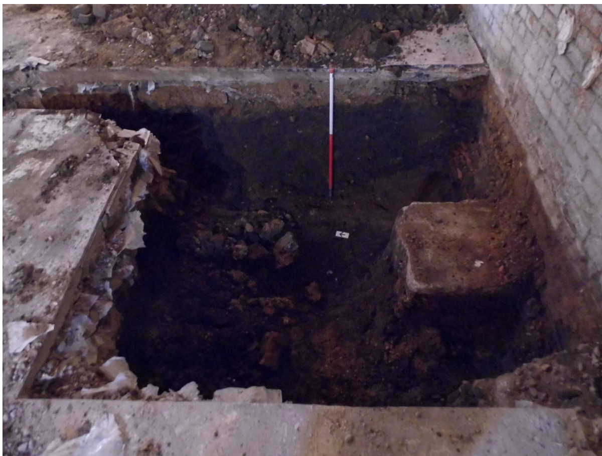
Figure 4: Deposits encountered in the lift shaft area showing the concrete block against the building wall.
