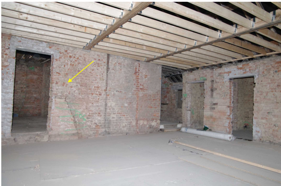
Figure 51 Room 12 Looking north-west. Note remnant of brick arch on right of left hand door Doors on right lead to Room 15, doorway in centre leads to hallway 16
