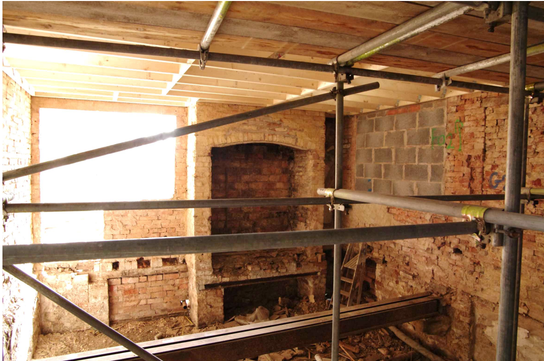
Figure 32 Room 5 Looking east. Floor level was at the top of the steel joist height
