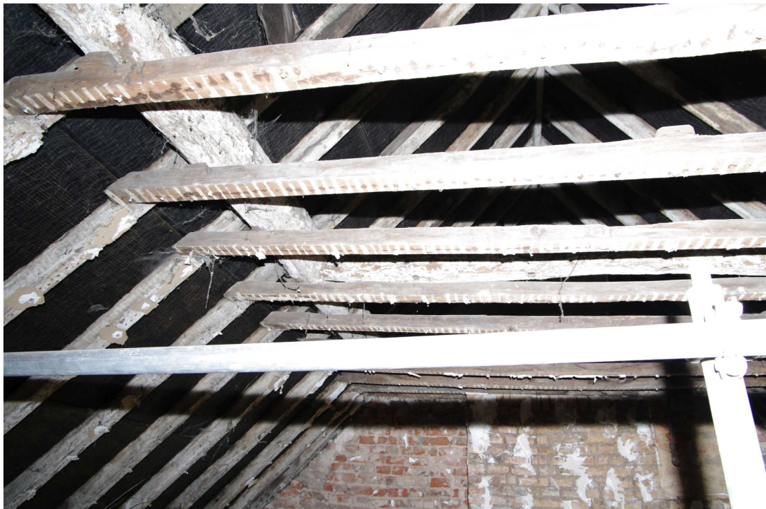
Figure 53 Room 13 roof structure Looking east. Note round section purlin and tie-beam. Tie-beam has a row of circular holes for wattles
