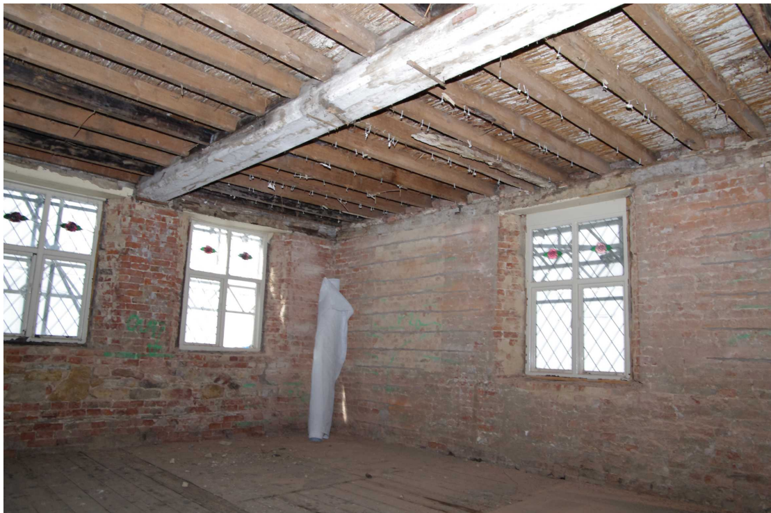
Figure 45 First floor Room 10 Looking south-west. Note blocked windows each side of window on right. These windows had been blocked by the time the illustration in Figure 5 was drawn. Note stone patching in wall on left
