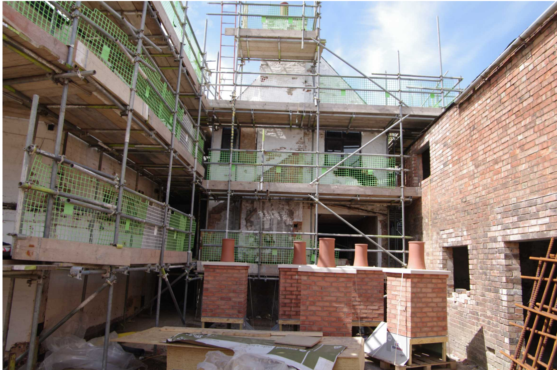
Figure 18 East facing elevation of rear northern range Looking west. Note scar of gable from demolished stable buildings
