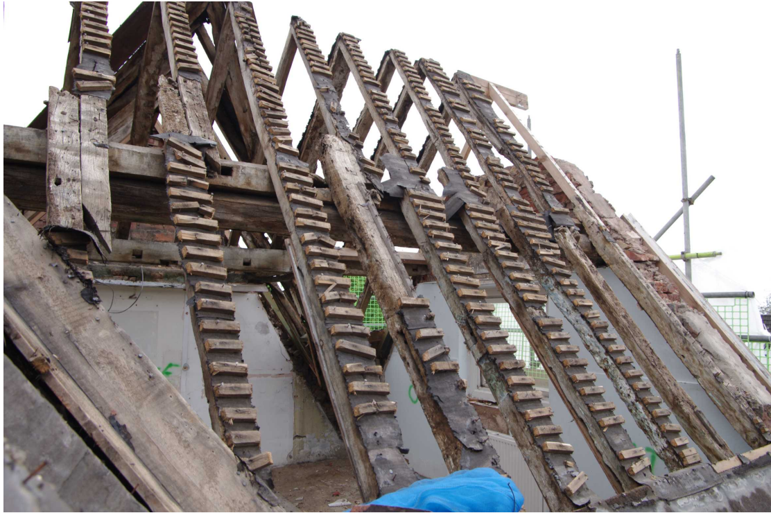
Figure 72 Outside of roof of Room 20 Looking south-east from Room 19. Note re-used timbers and patching
