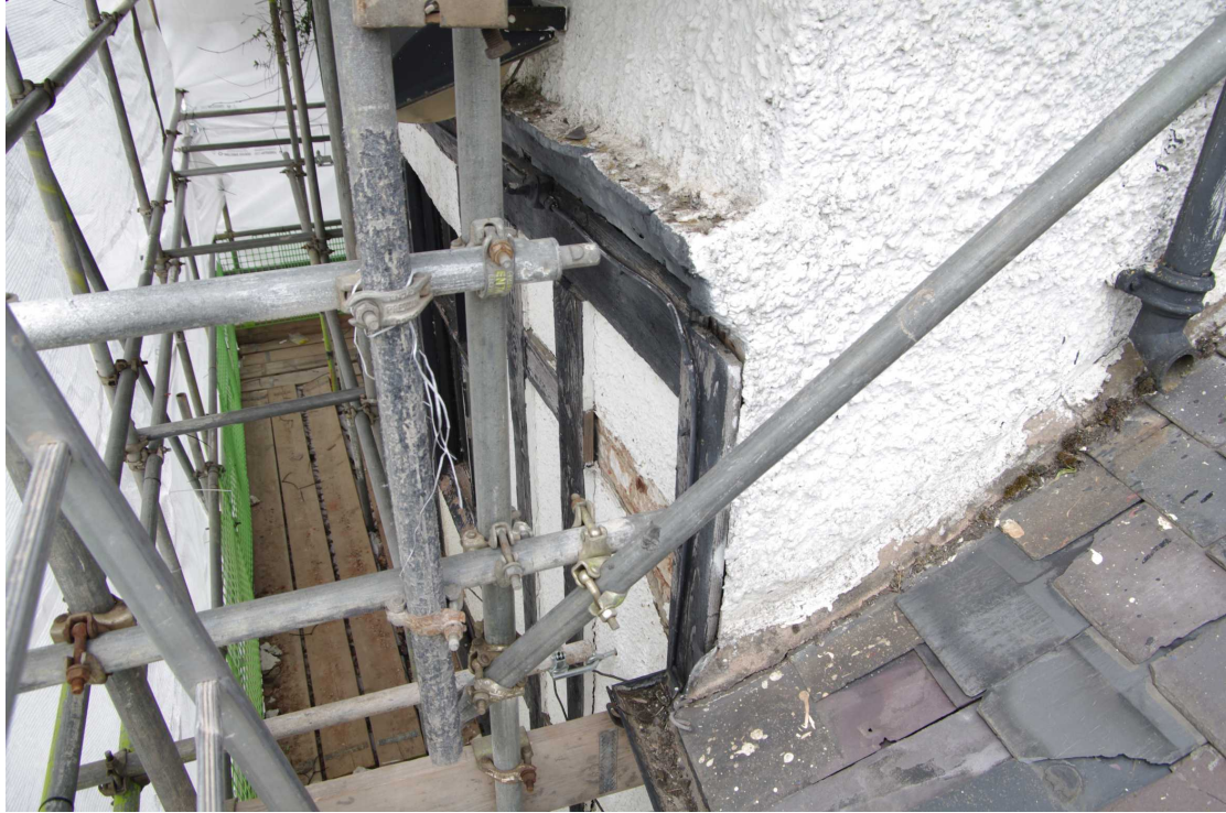
Figure 16 South facing elevation at first floor level Looking north-west. Note moulded brick string course above window
