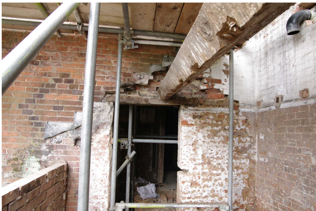
Figure 36 North wall of Room 5 from the outside in former pantry Note diaper work to left of door
