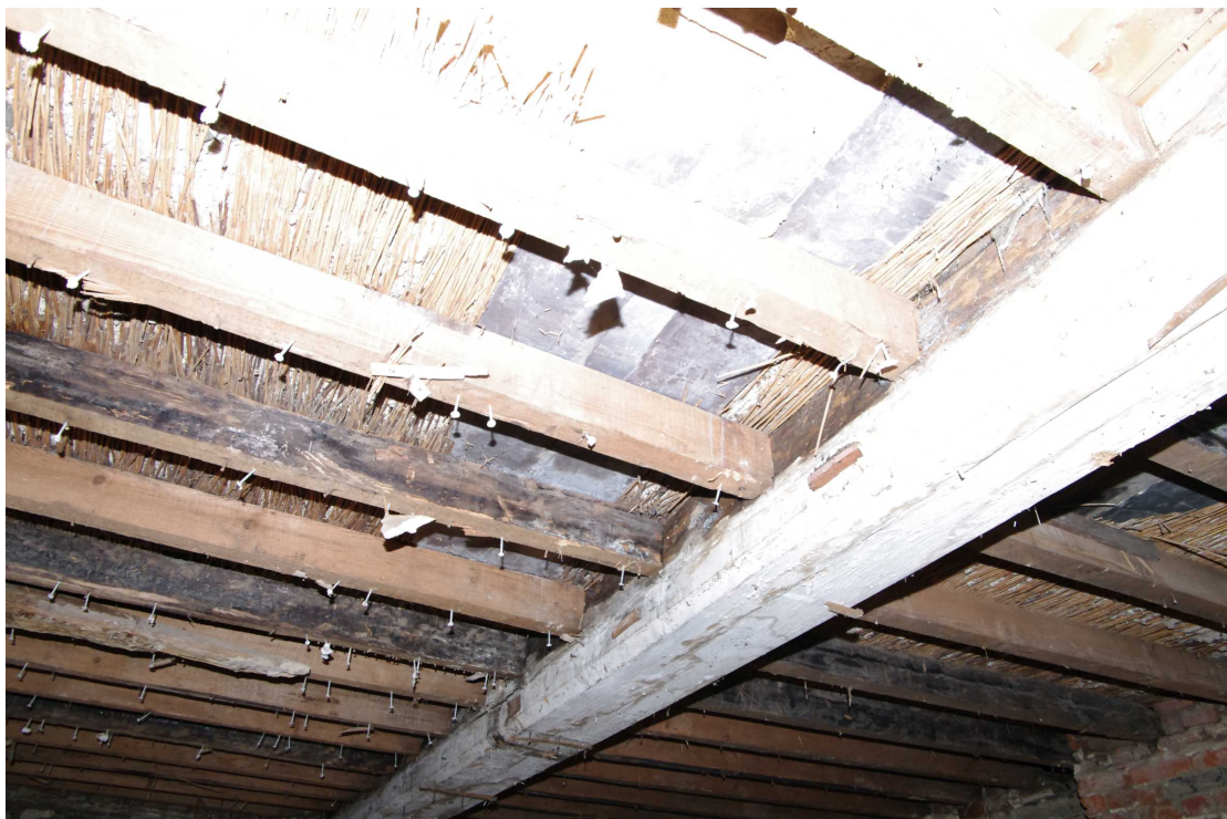
Figure 47 First floor Room 10 beam detail Note redundant sockets
