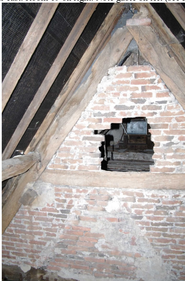
Figure 61 East gable over Room 13 seen from Room 18 Looking east. Note pegged apex and scar from earlier lower gable
