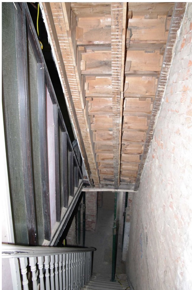
Figure 56 Stairs down to ground floor Looking east. Underside of stairs up to first floor also visible
