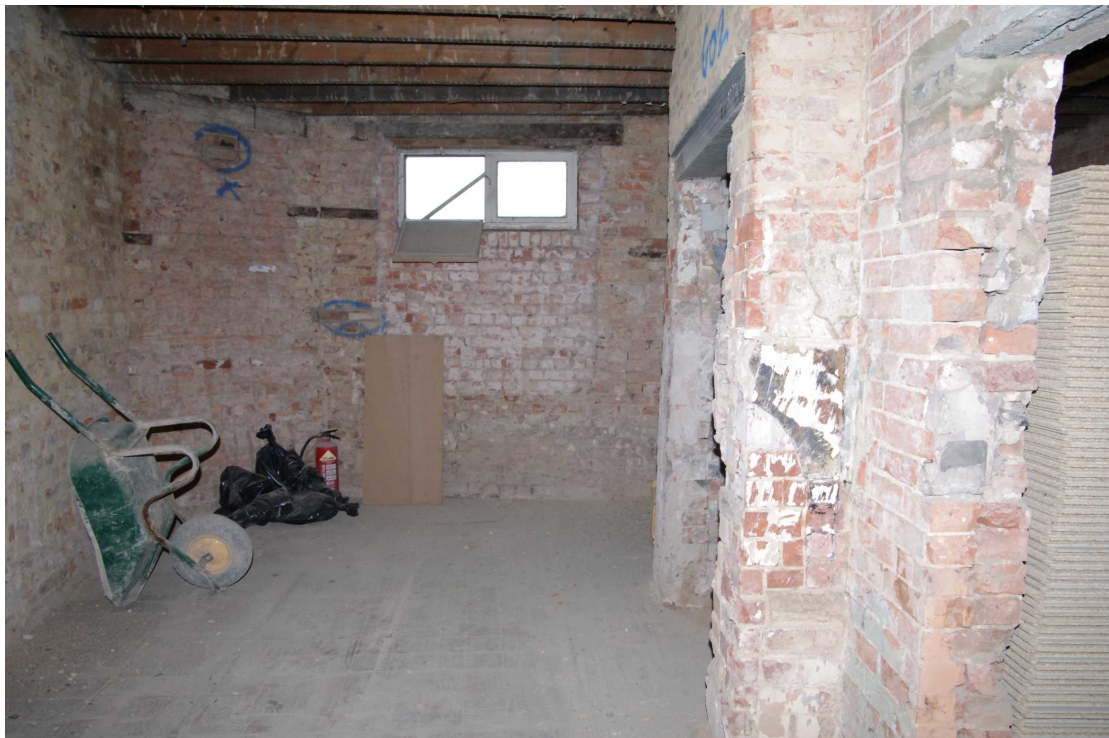
Figure 39 Ground floor Room 7 Looking north-east. Fireplace on right. Blocked doorway to right of barrow
