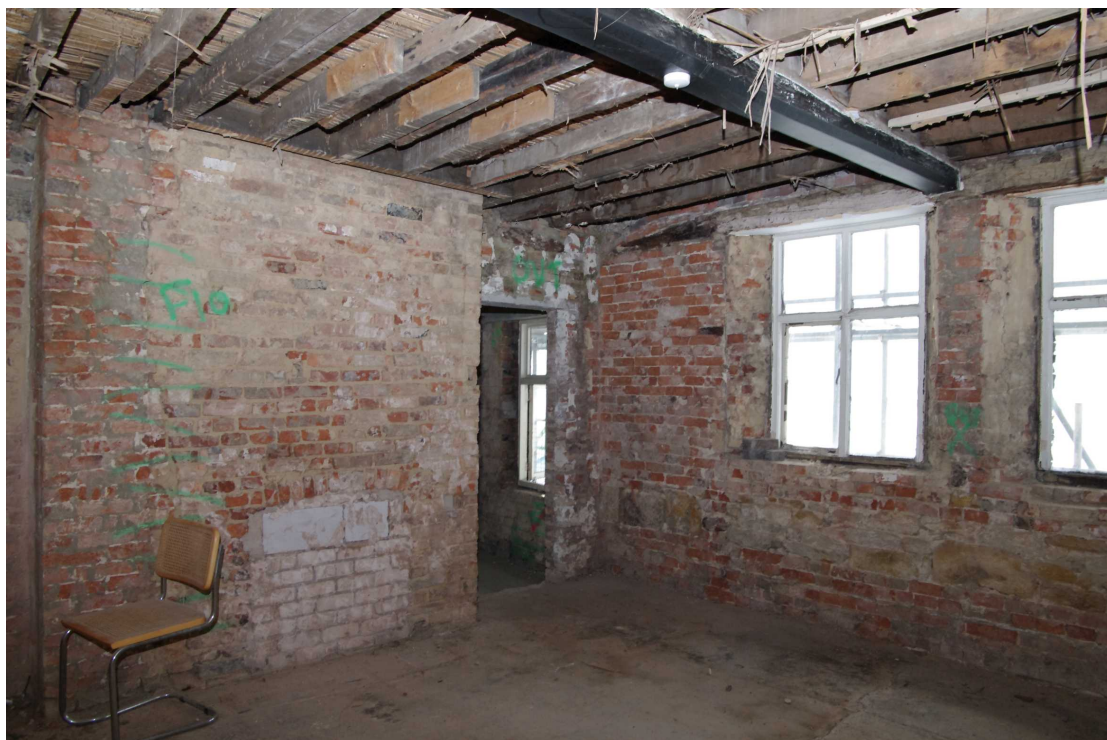
Figure 49 Room 11 Looking south-east. Note step down in floor level to Room 12 through doorway
