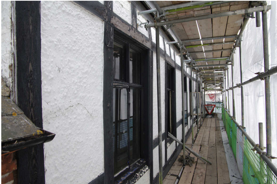
Figure 14 West facing elevation, first floor window detail Looking south. Gutter of 1 Main Street on left
