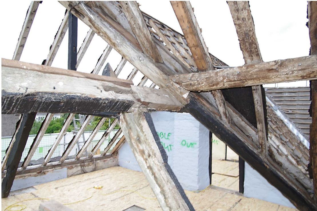
Figure 69 Room 19 roof detail Looking north-west through former slated roof. See also Figure 70 below
