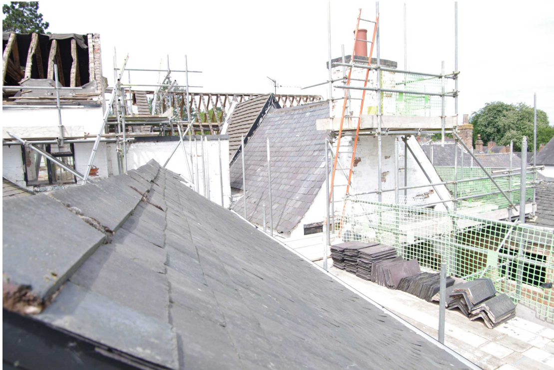
Figure 20 Roofscape of rear northern range Looking north-west. The range consists of two phases with different height gable ends
