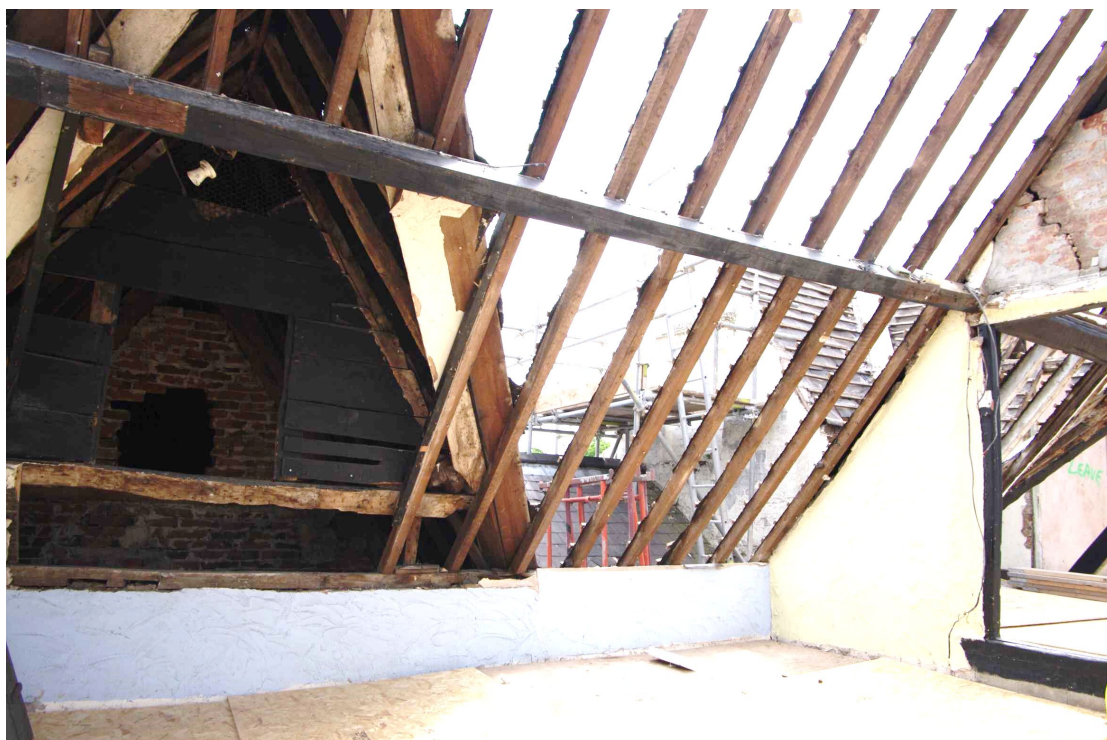
Figure 60 Room 18 Looking south-east. Room 19 on right. Note gable on left (see Figs 61 and 62)
