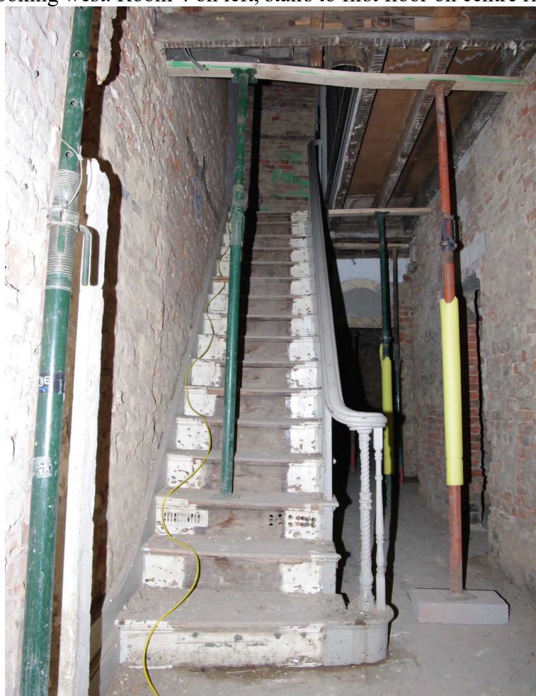
Figure 41 Stairs to first floor (Room 8) Looking west. Door to Room 2 on right
