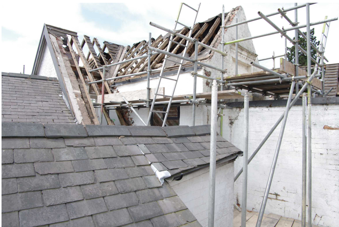
Figure 19 Roofscape of gabled southern extension Looking south-west. Note drip-mould around redundant window in gable
