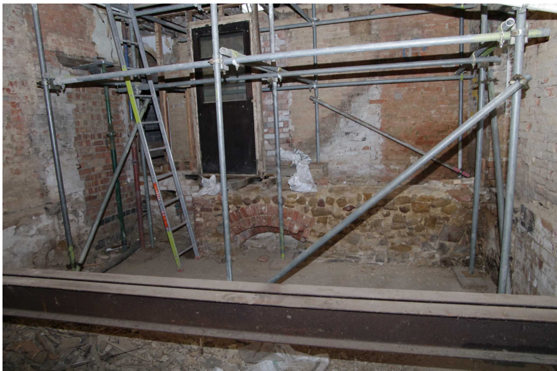
Figure 33 Room 5 base of stone wall and brick arch Looking west. This may be part of a cellar or undercroft possibly extending as far north as Main Street
