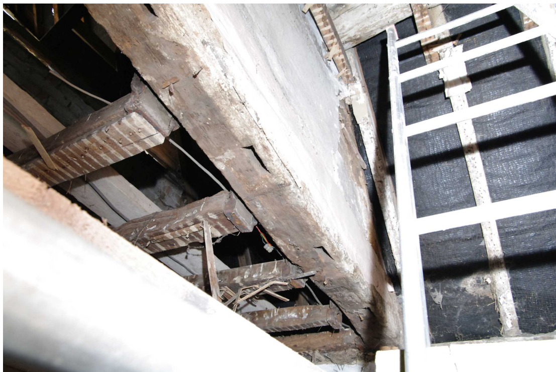
Figure 54 Room 13 underside of original gable end wall Looking north-west. See Figure 37 for external view
