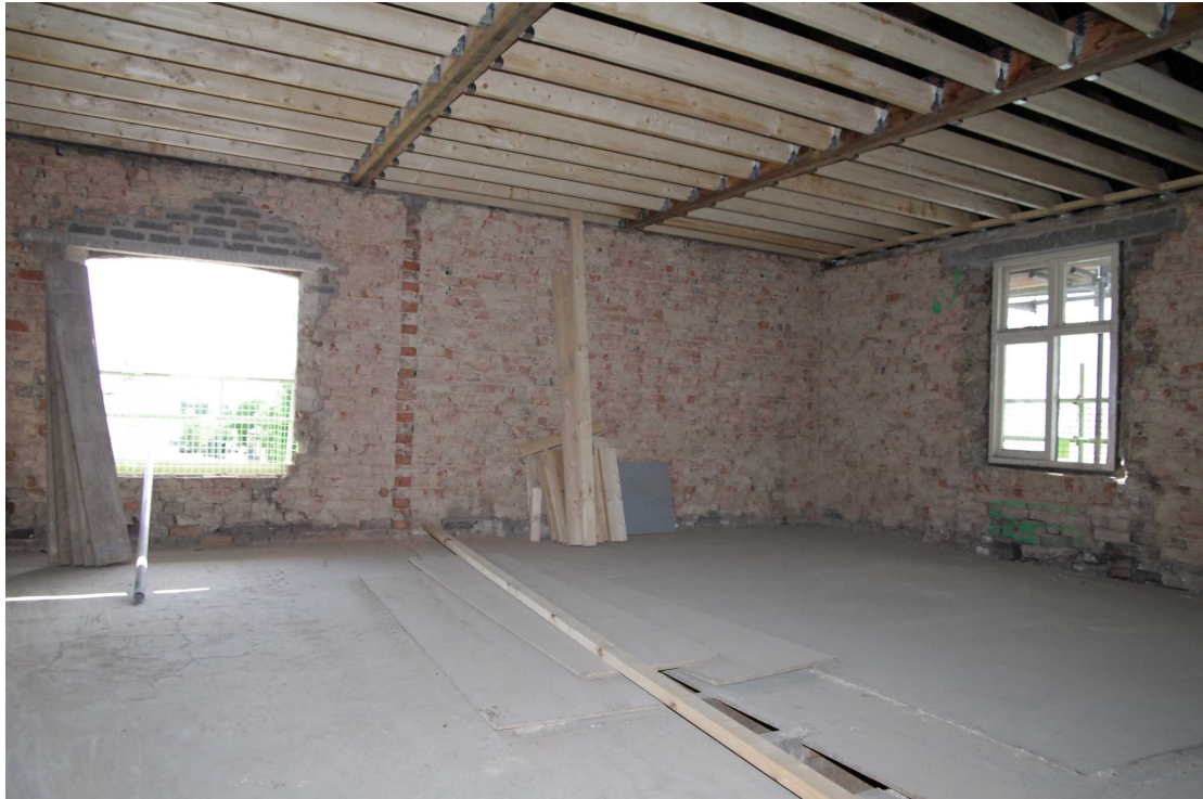
Figure 50 Room 12 Looking south-east after removal of internal walls and new ceiling insertion
