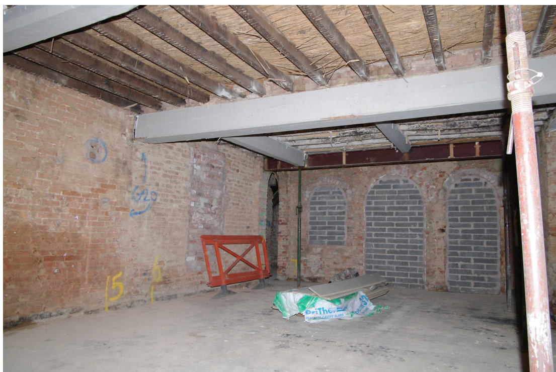
Figure 23 Northern room (1) of Main Street range Looking south-east. Chamfered beam on left, beaded beam on right
