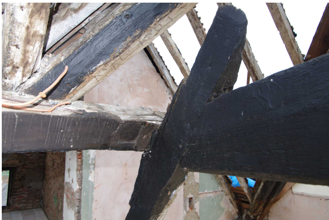
Figure 67 Room 19 joint detail of western frame Looking south-east. Note marks on underside of principal rafter
