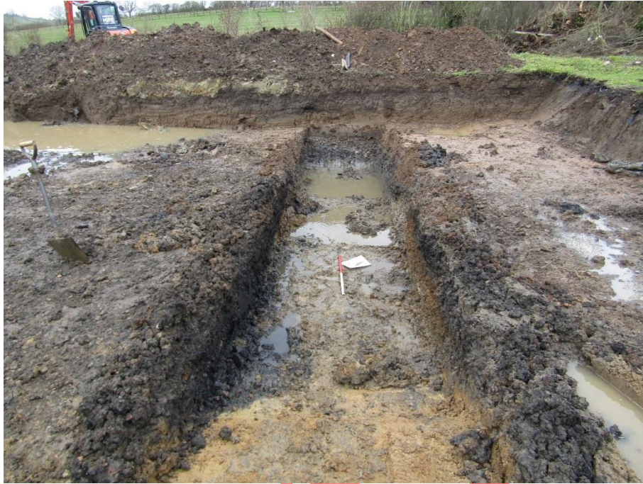
Figure 14: Sondage machined through stone deposits. Note water ingress and evidence of section collapse.
