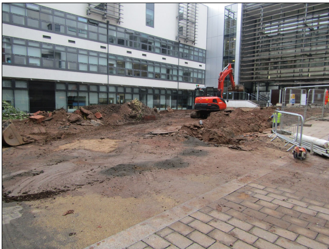
Figure 4: The site on arrival looking north, with service trench to the right.
