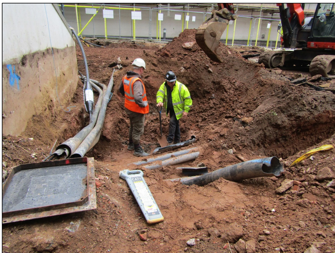
Figure 5: Exposed services up to a depth of 2m at the north-east end of the development area looking south-east.
