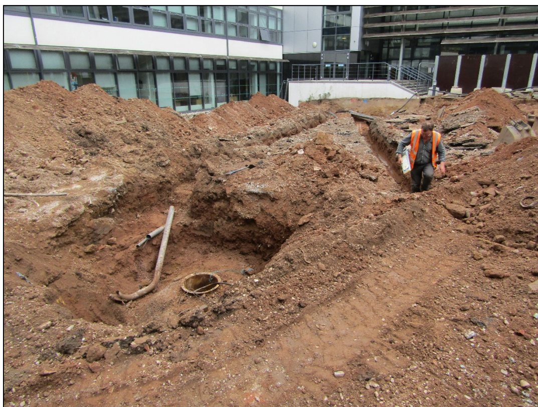
Figure 8: The development area looking north-east showing the extent of previous truncation and demolition deposits.
