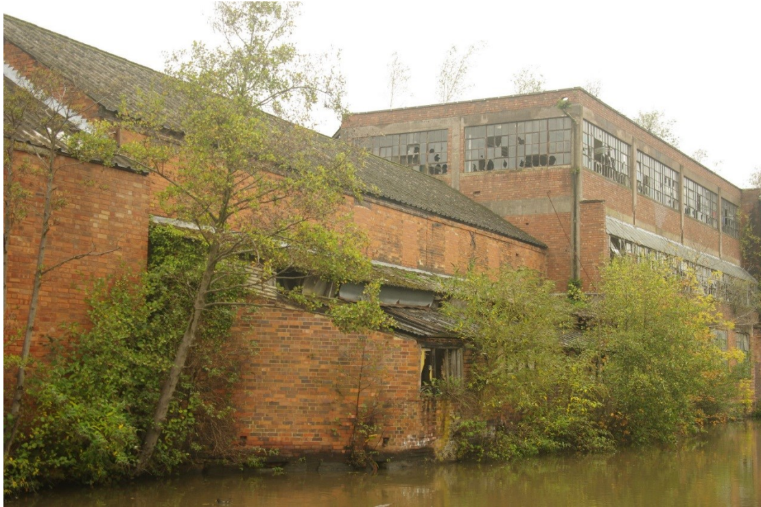
Figure 21 North-east facing elevation of Building C and lean-to Building D Looking north-west. Building F-L on right
