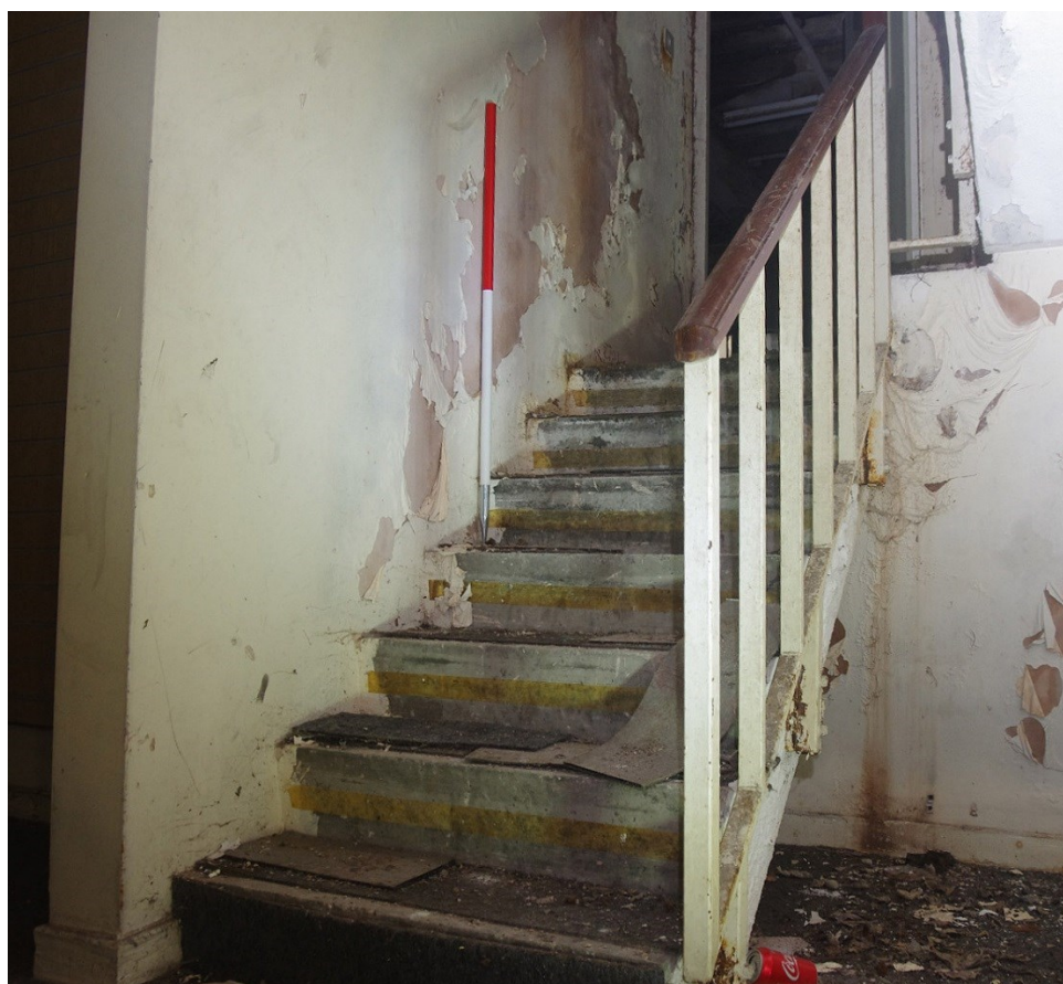
Figure 68 Rear wing R1 stairs at ground floor level Looking north. 1m scale
