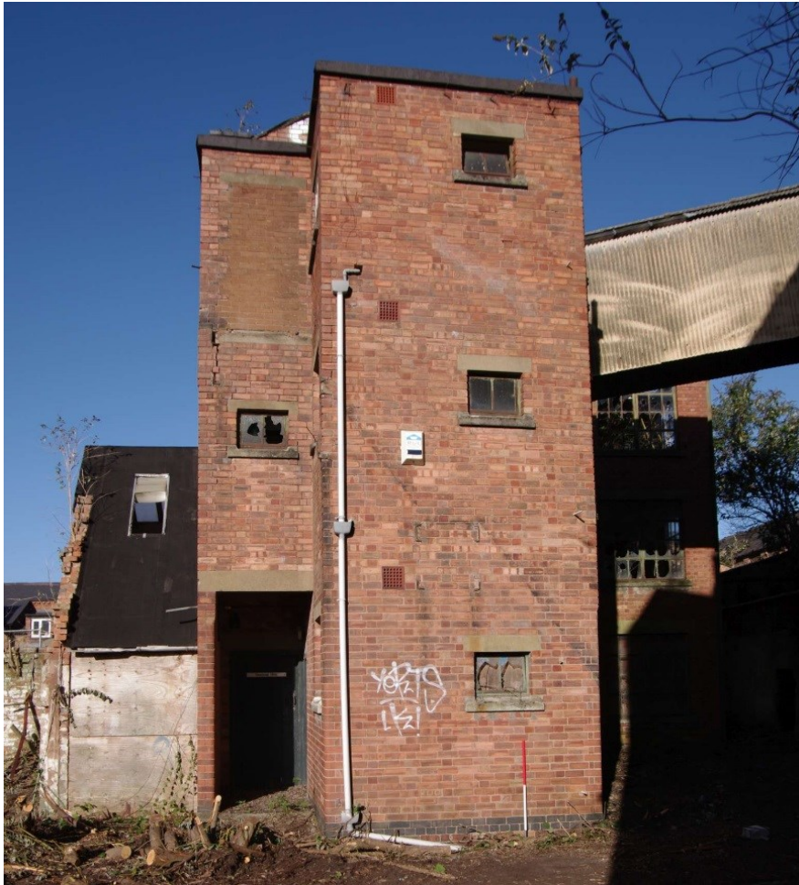
Figure 84 Building V south-east facing elevation Looking north-west. 1m scale. Note stairs and building remnant on left
