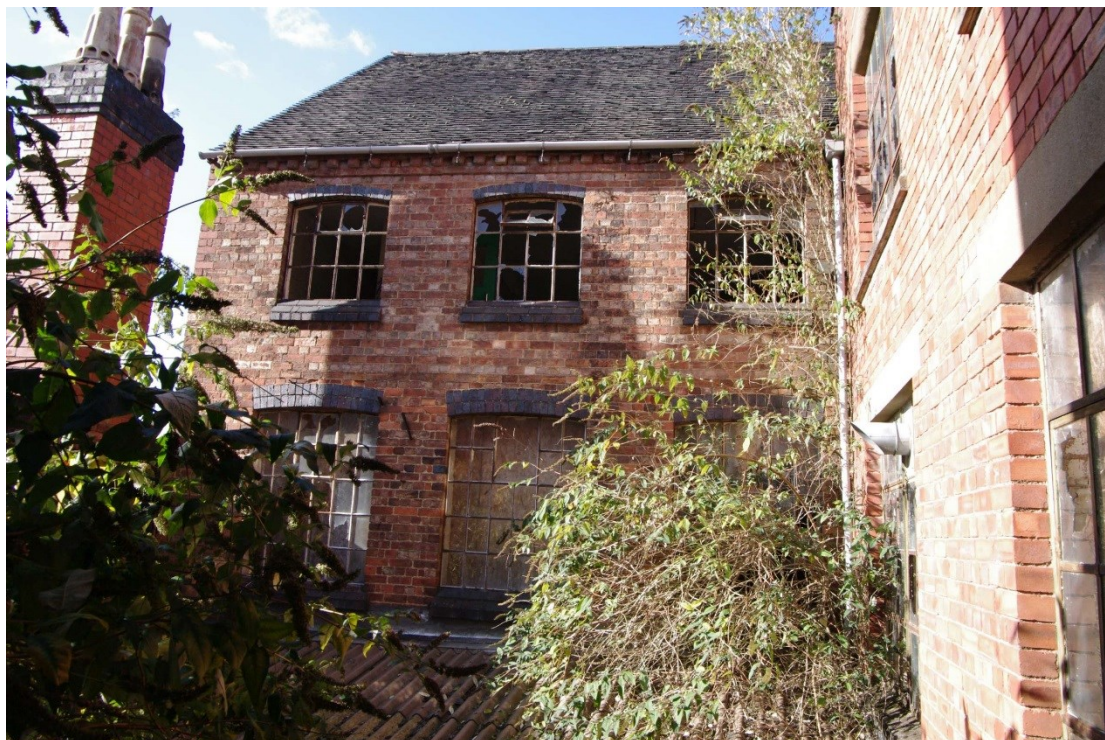
Figure 81 Building U south-east facing elevation Looking at first and second floors from Building V.
