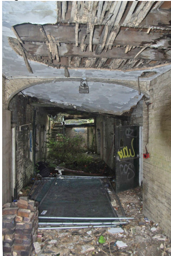
Figure 62 Passageway beneath Building R Looking south-east from Coleshill Road. R1 on left, R2 on right
