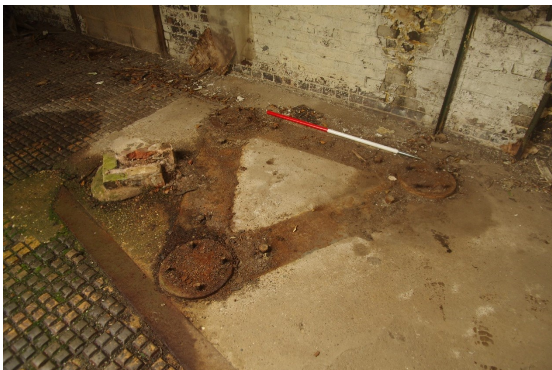
Figure 26 Building D possible machine base at southern end of room 1m scale
