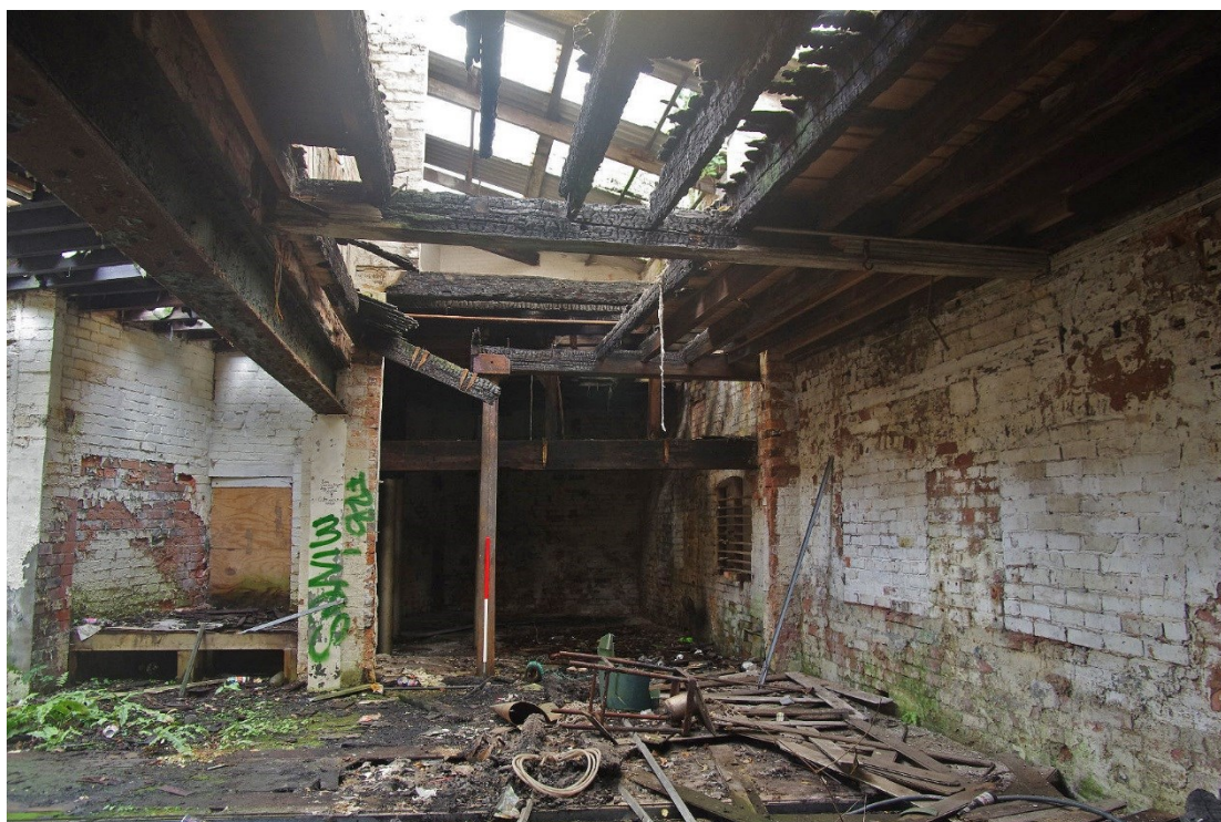
Figure 74 Rear wing R2 ground floor southernmost room Looking south-east. 1m scale. Building F-L on left
