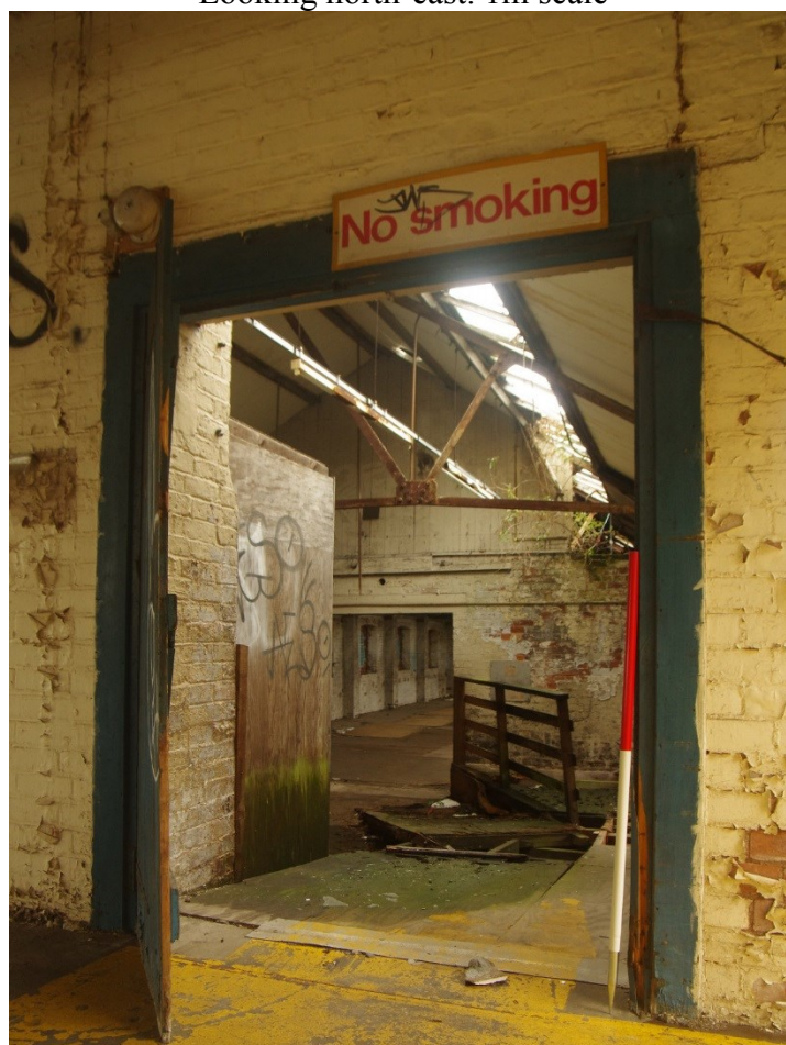
Figure 30 Building E first floor seen from Building F Looking south-west. 1m scale
