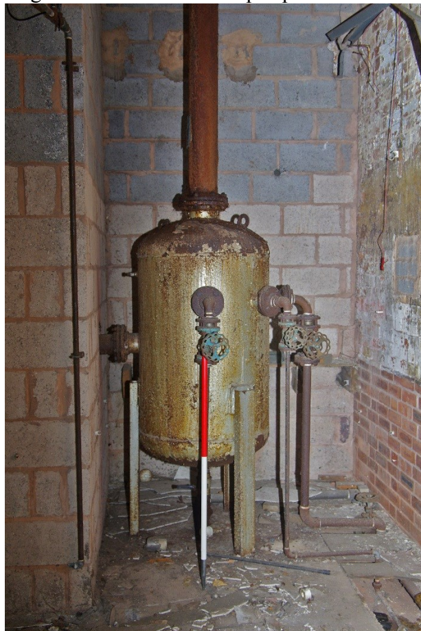
Figure 17 Boiler inside southern end of Building A/B Looking north-west. 1m scale
