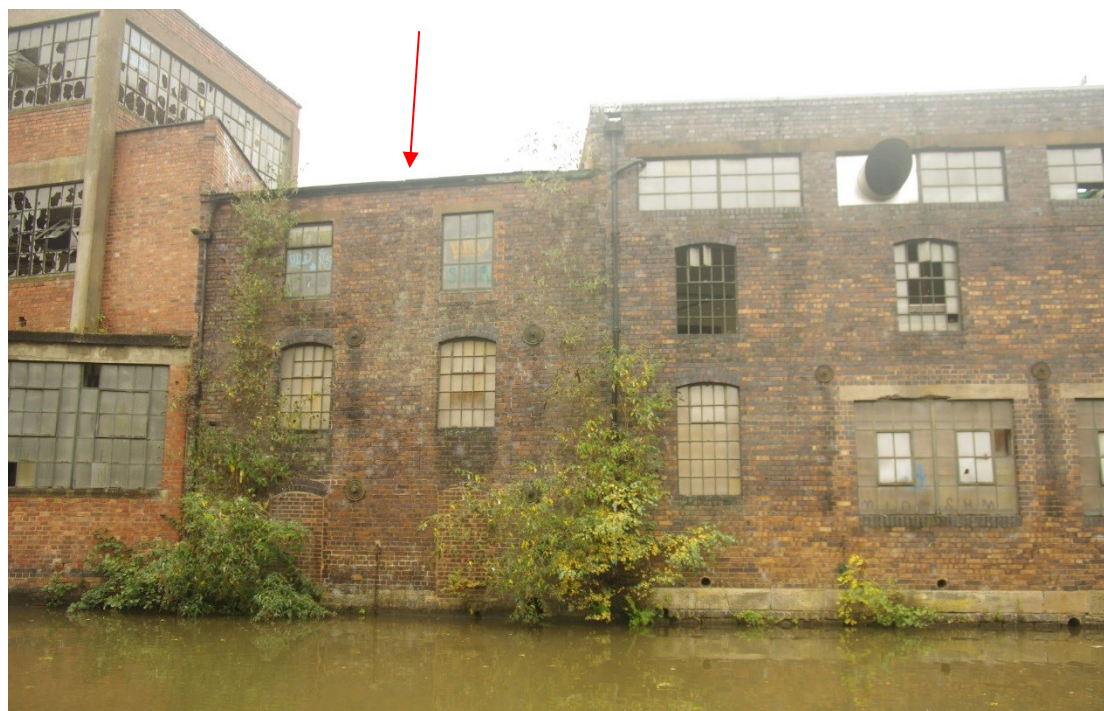
Figure 49 North-east facing elevation of Building N Building N is arrowed. Building F-L on left and O/P on right
