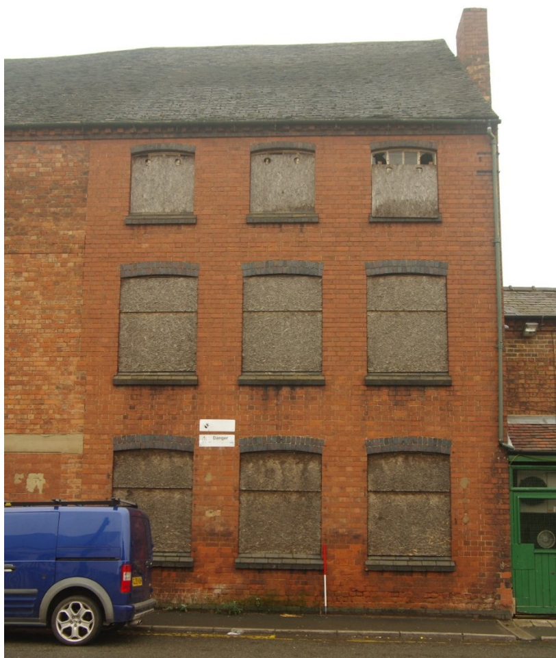
Figure 79 Building U north-west facing elevation onto Coleshill Road Looking south-east. 1m scale
