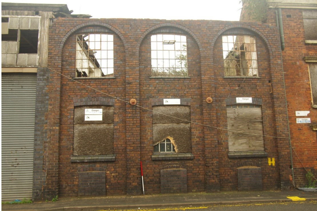
Figure 57 Building Q north-west facing elevation Looking south-east. 1m scale. Covered access to left, Building R to right
