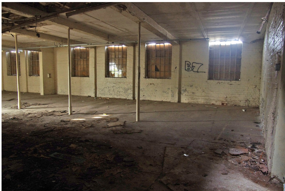
Figure 78 Building T first floor Looking north-west. The first floor of Building U is beyond the stub of wall to the left
