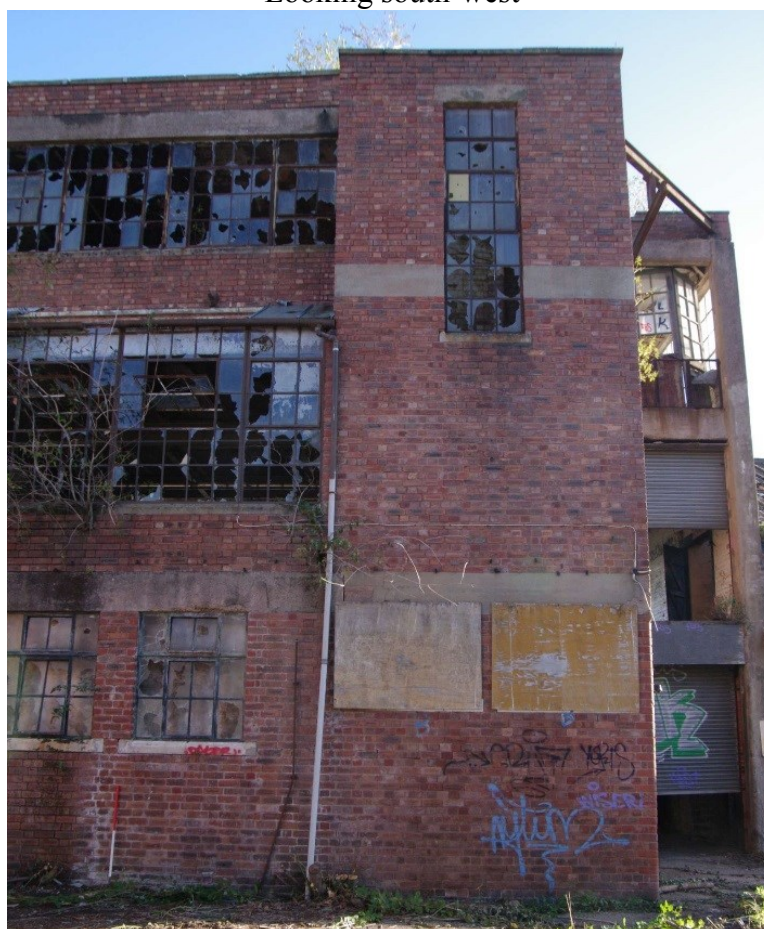
Figure 35 South-west facing elevation of Building F-L (south end) Looking north-east. 1m scale. F-L loading bays on right
