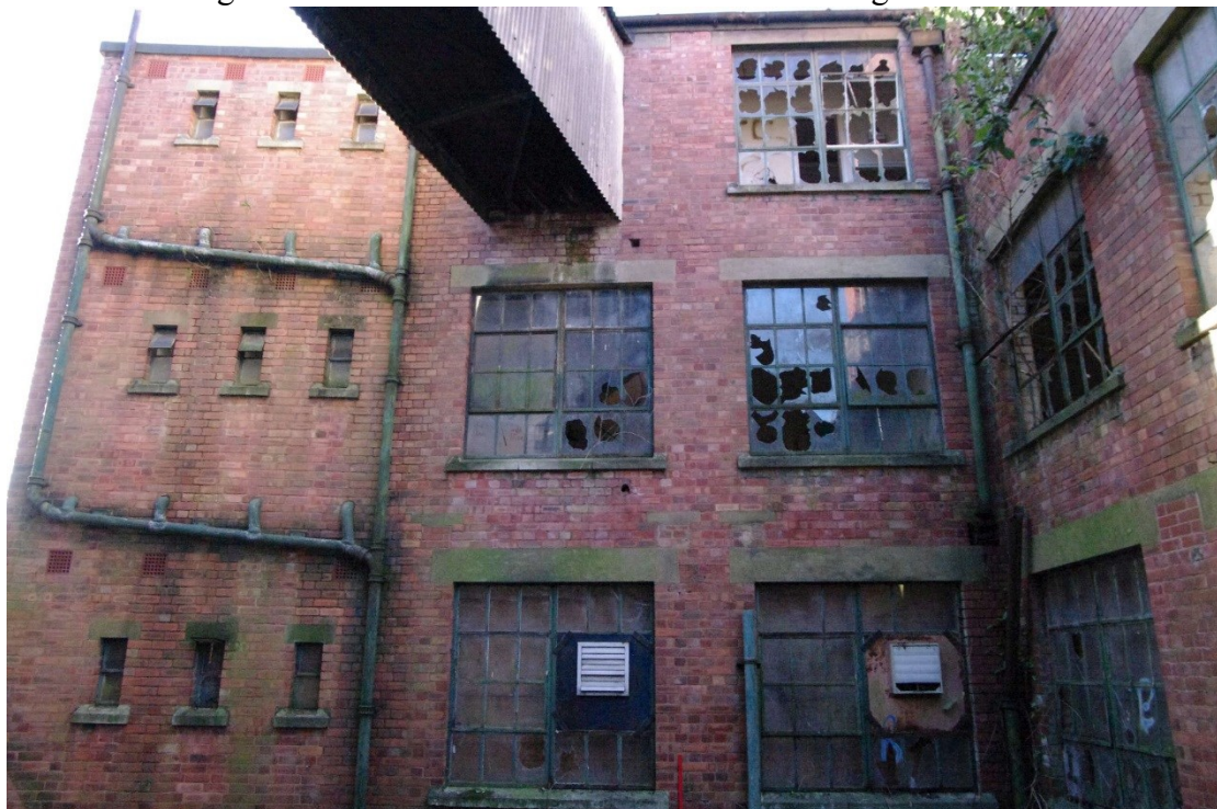
Figure 85 Building V north-east facing elevation (southern end) South-east facing elevation on right. Bridge to Building F-L top centre
