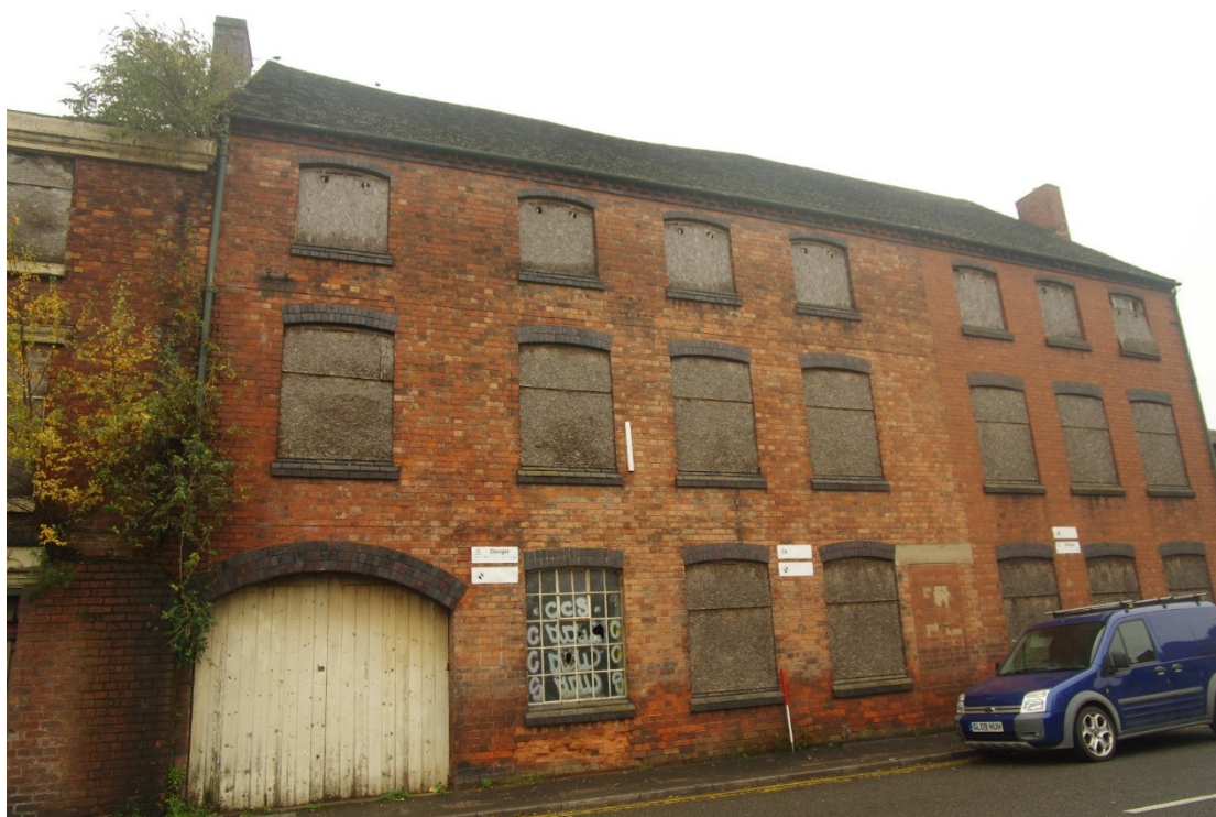
Figure 76 Building T north-west facing elevation onto Coleshill Road Looking south-west. 1m sale. Building U with darker bricks on right
