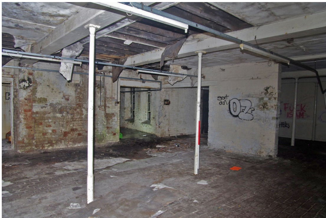
Figure 77 Building T ground floor Looking south. 1m scale. Ground floor of Building U behind wall with “OZ” graffiti. Building V through gap in wall in centre
