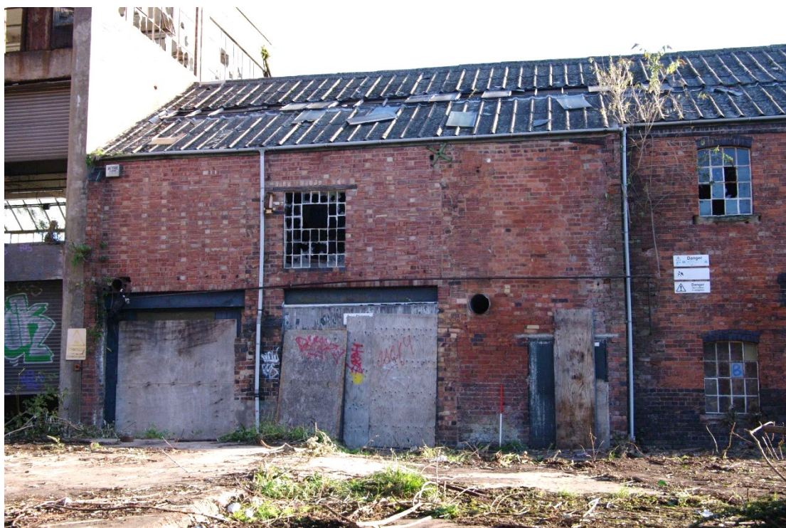
Figure 28 South-west facing elevation of Building E Looking north-east. 1m scale. Building F-L on left
