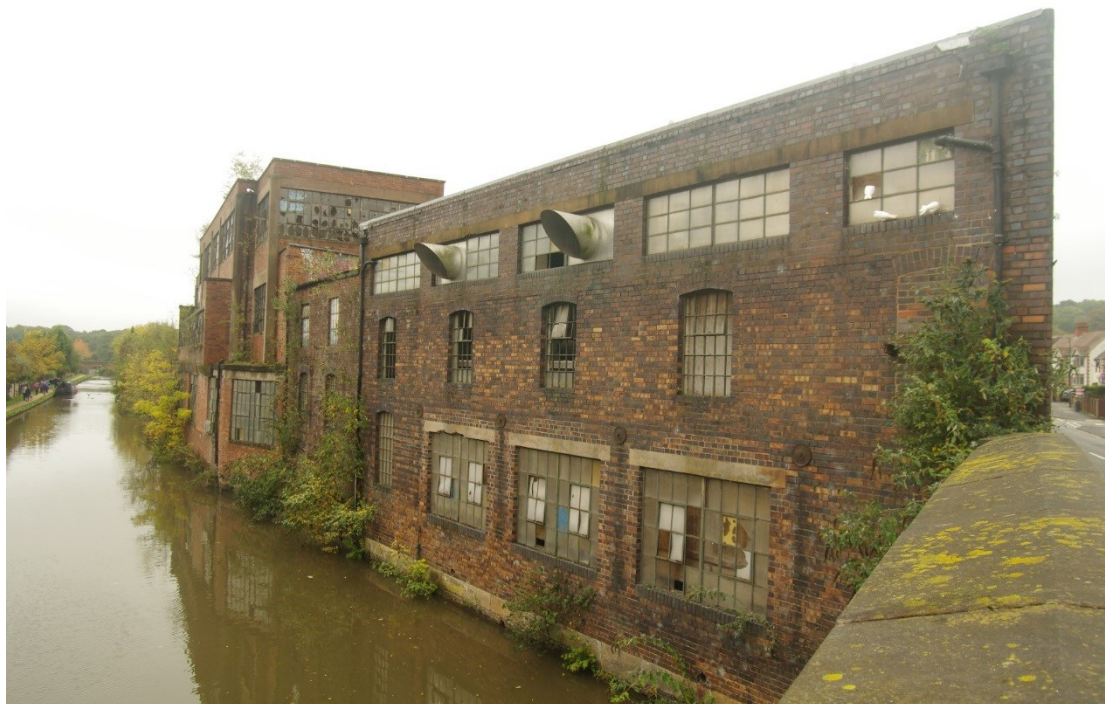
Figure 10 north-east facing elevation along canal (northern end) Looking south from Coleshill Road over bridge parapet. Building N on foreground
