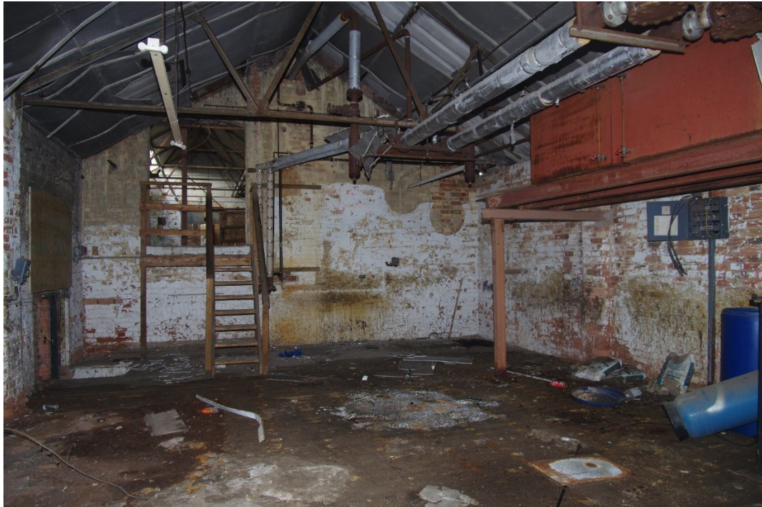
Figure 16 Inside southern end of Building A/B Looking north-west towards steps up to mezzanine floor
