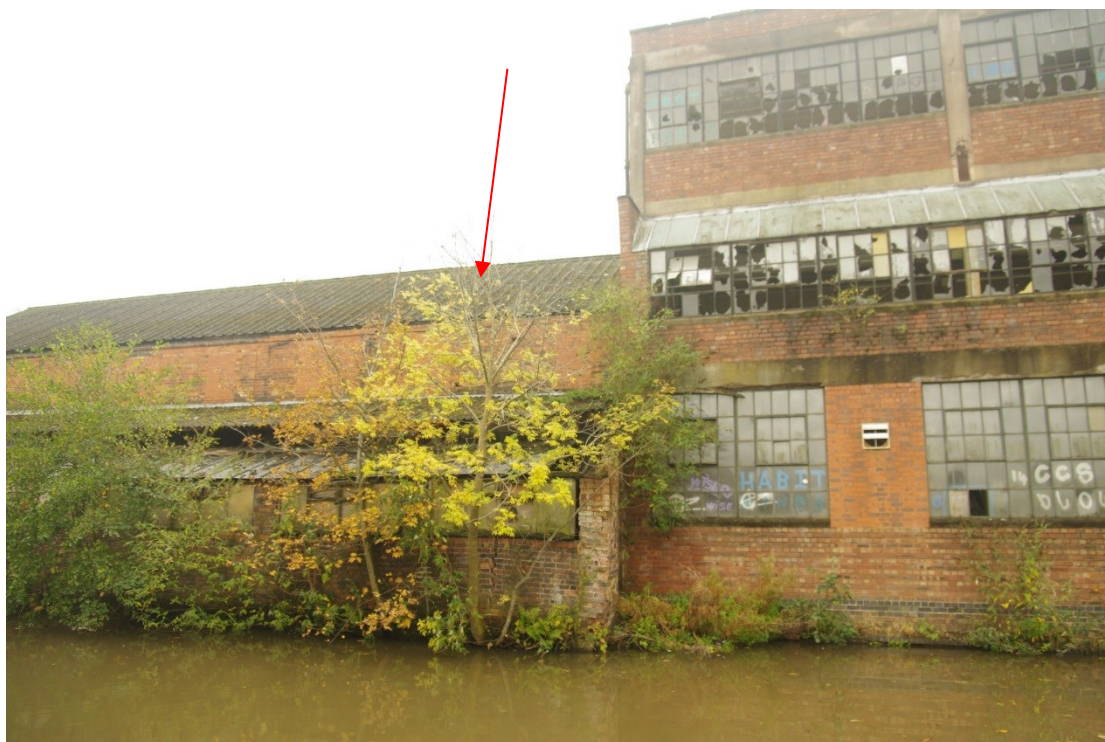
Figure 27 North-east facing elevation of Building E Joint between Building C and Building E is arrowed. Building F-L on right
