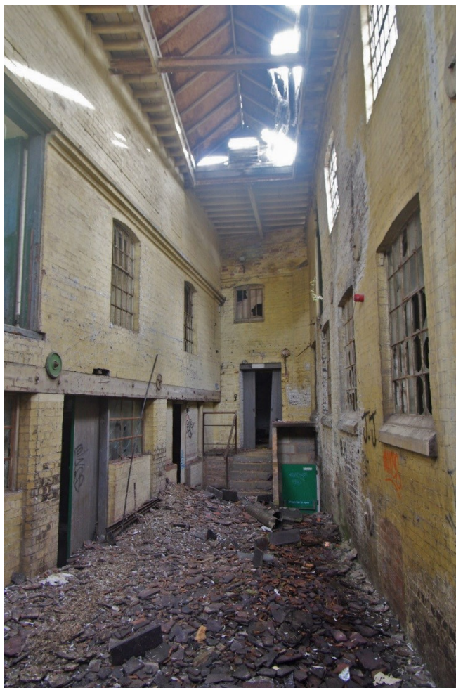
Figure 55 Building O/P south-west facing elevation Looking south-east. Building O/P on left, Building N in centre, Building Q on right
