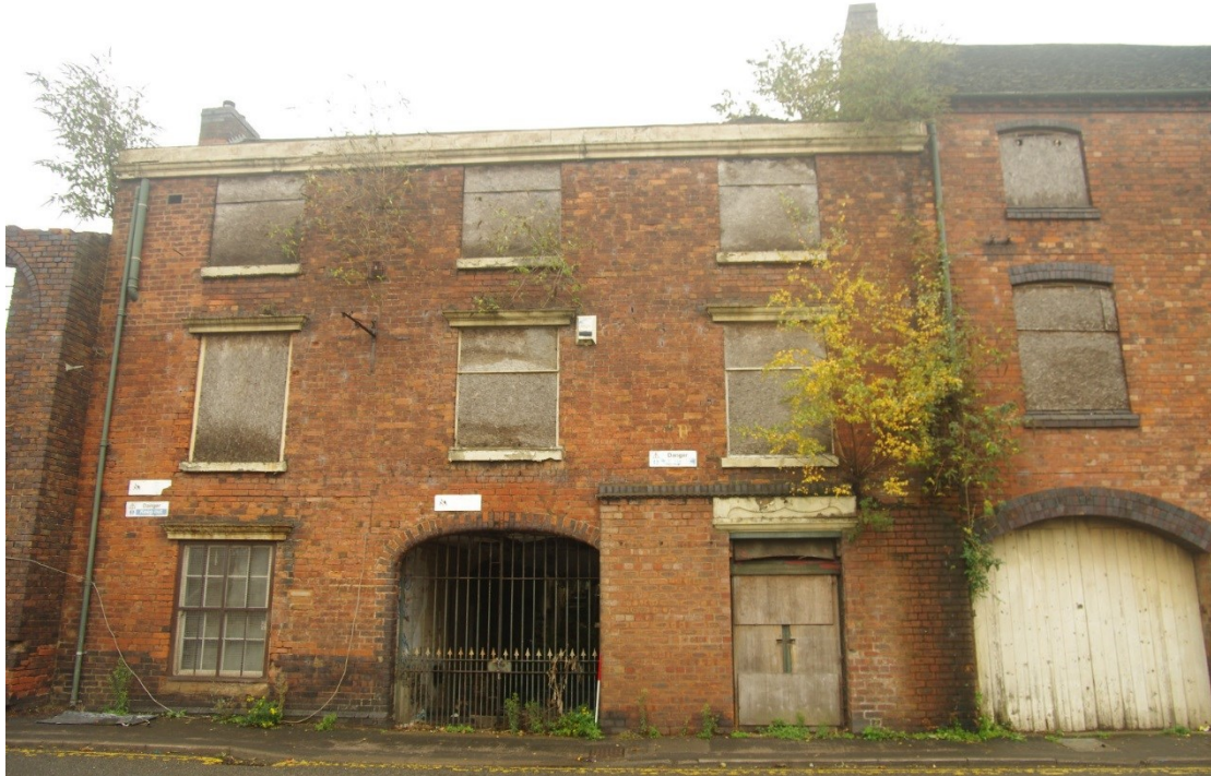
Figure 61 Building R north-west facing elevation Looking south-east. 1m scale. Building U/T on right
