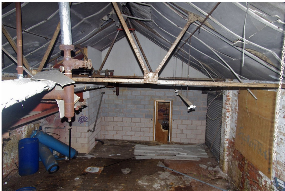
Figure 19 View from Building C onto mezzanine floor of Building A/B Looking south-east
