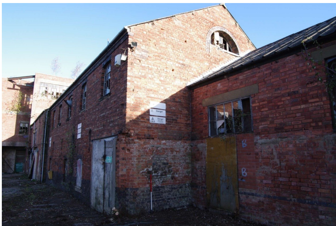
Figure 20 Building C south-east facing gable end Looking north. 1m scale. Note chamfered corner. Building A/B on right
