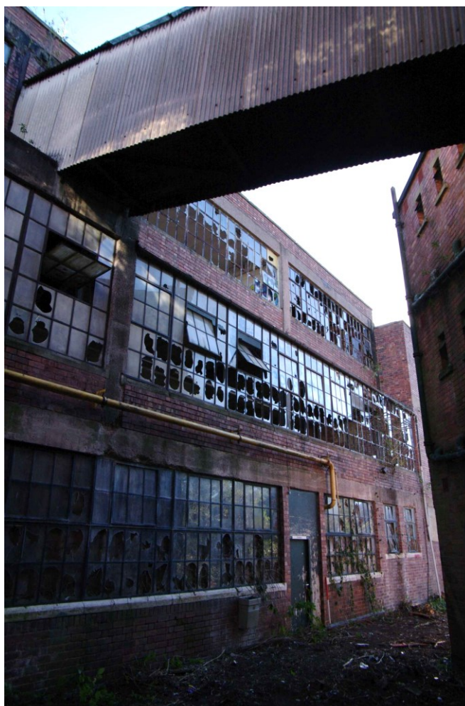
Figure 36 South-west facing elevation of Building F-L (north end) Looking east. 1m scale. Bridge leads to Building V on right
