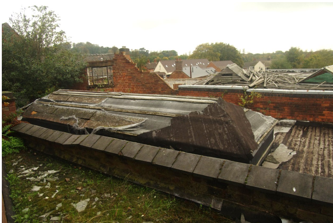
Figure 48 View across Buildings N, O/P and Q from second floor of Building F-L Looking north
