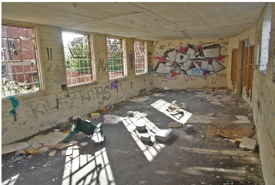
Figure 70 Rear wing R1 second floor Looking north-east from stairs of Building F-L. Plasterboard partition to rest of R1 on right.
