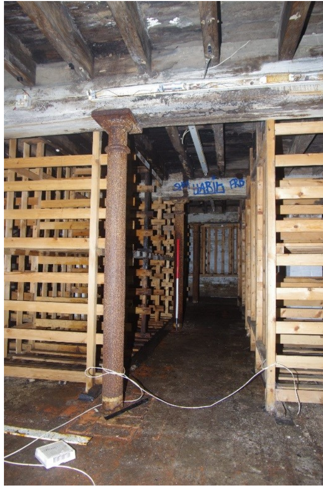
Figure 50 Building N basement/ground floor Looking north-west from Building N to space below Building Q. 1m scale
