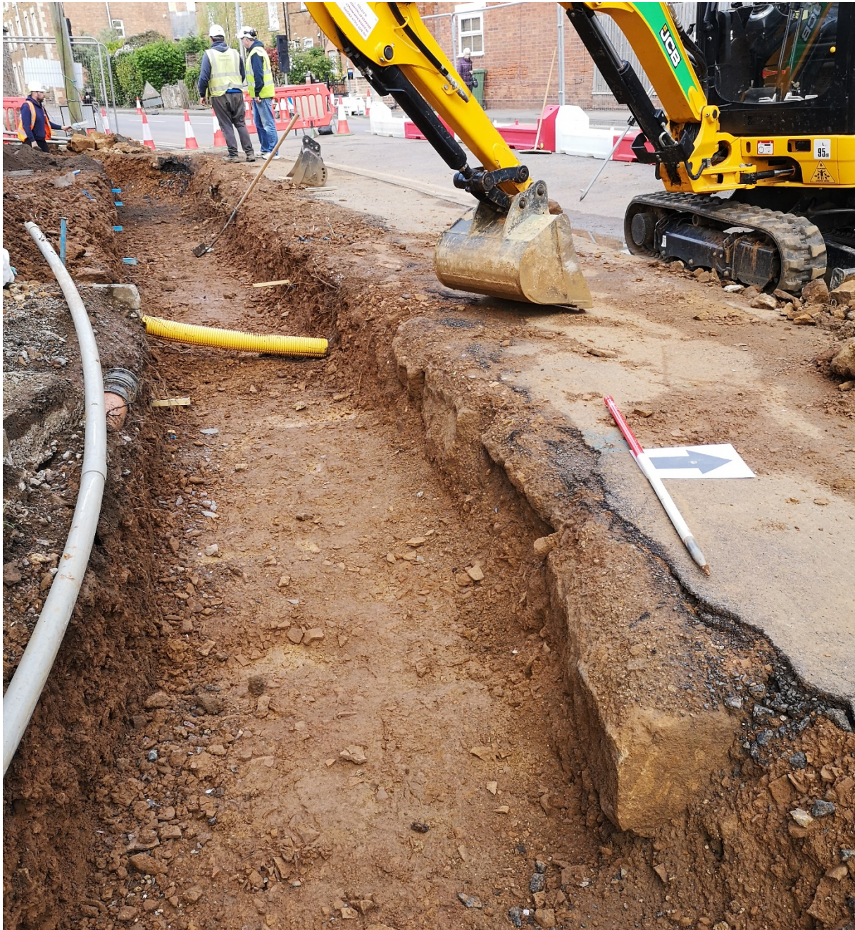
Figure 24: New footings trench after excavation. Also shows original footings beyond the line of the wall (right).
