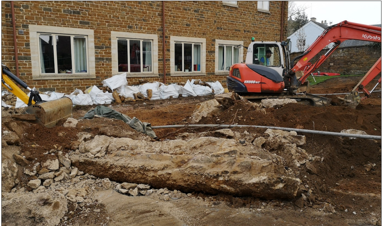
Figure 21: Large section of wall (1) previously rebuilt with a cement mortar.
