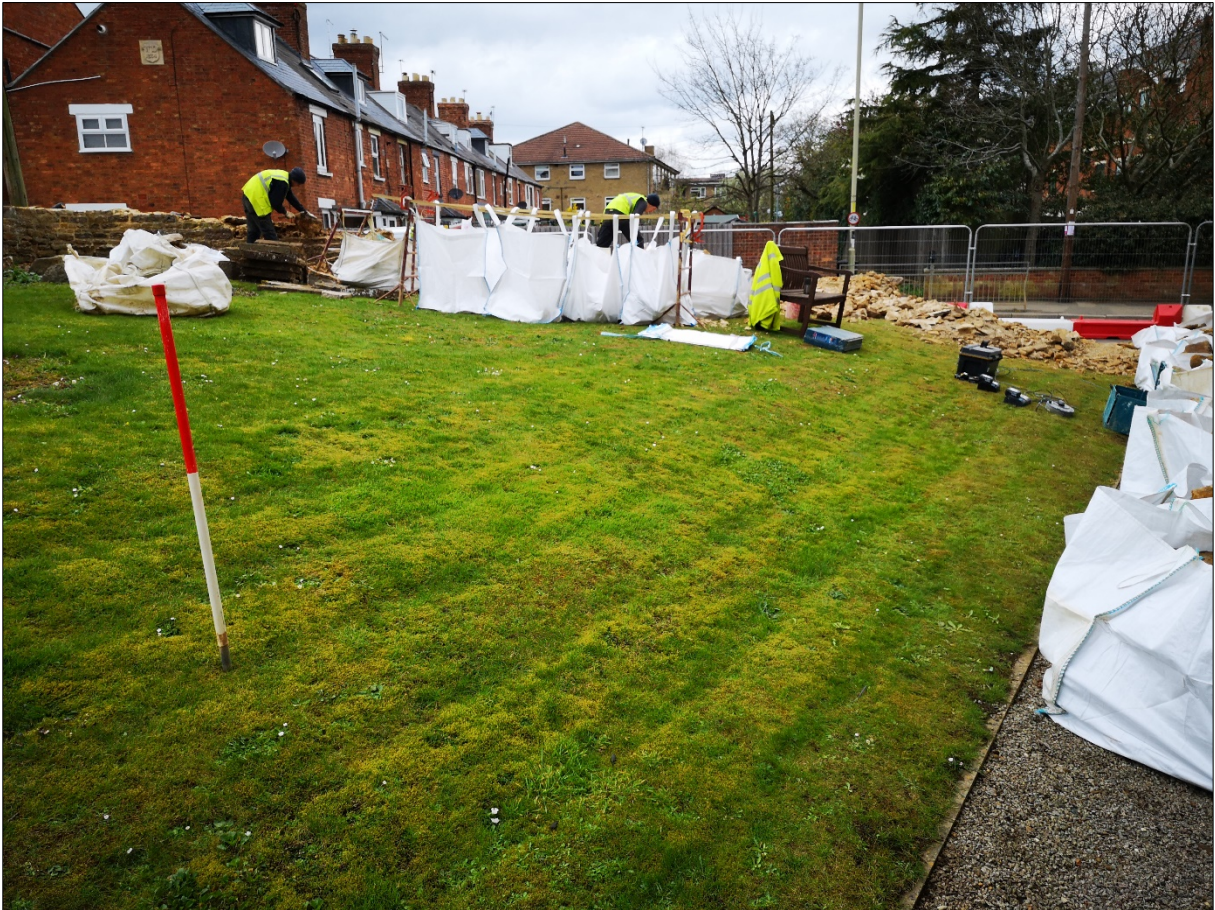
Figure 6: General view of internal area prior to works, and wall being removed (background), looking north.
