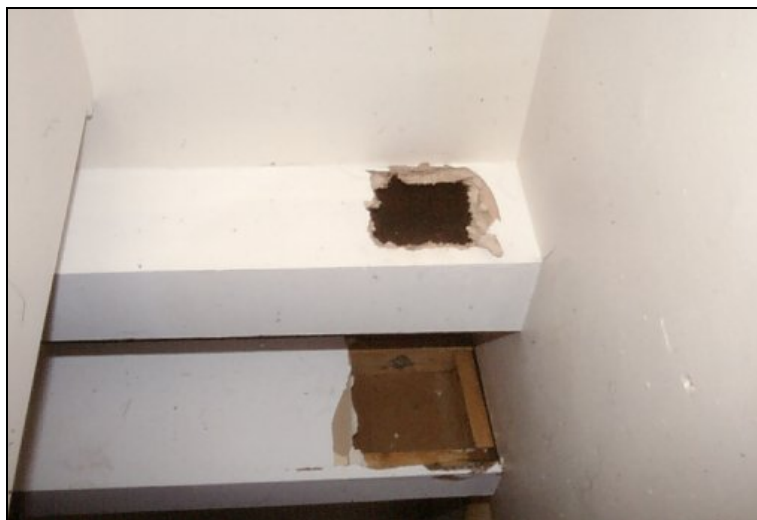
Plate 4. Area D (to rear) and E (to front) openings to investigate first floor structure
