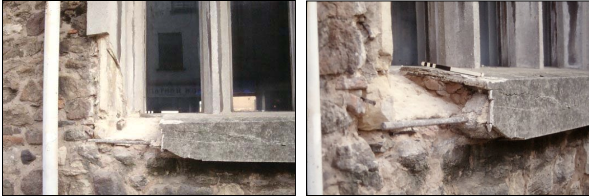
Plates 11 & 12. Two views of Area 4 opening to investigate surround of window W3
