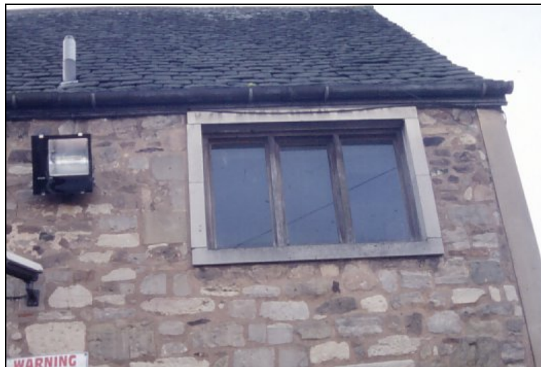
Plate 22. Window W16 east (car park) elevation showing remains of early stone window surround to left of and truncated by 1960s concrete surround
