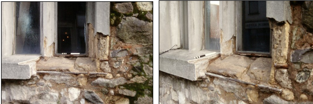
Plates 13 & 14. Two views of Area 5 opening to investigate surround of window W1
