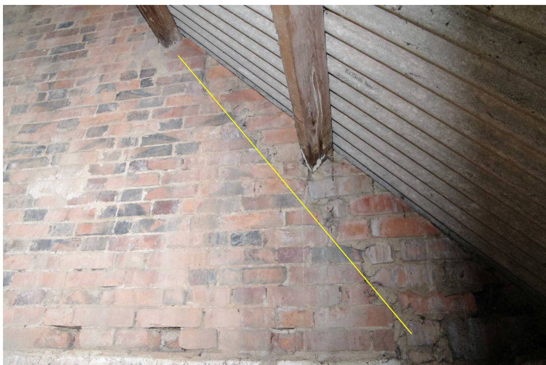
Figure 28 Saddle House rebuilt eastern gable end Looking east. Yellow line shows the original roof pitch
