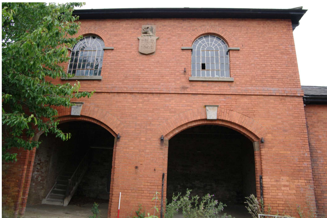
Figure 33 The Coach House south facing elevation, centre range Looking north. 1m scale
