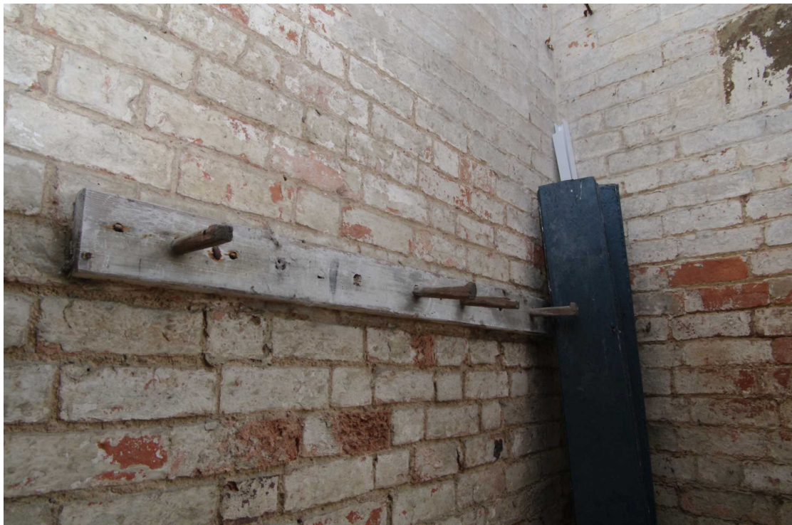
Figure 54 The Coach House ground floor east wing Wooden pegs/hooks on eastern wall (see Fig. 53 above)
