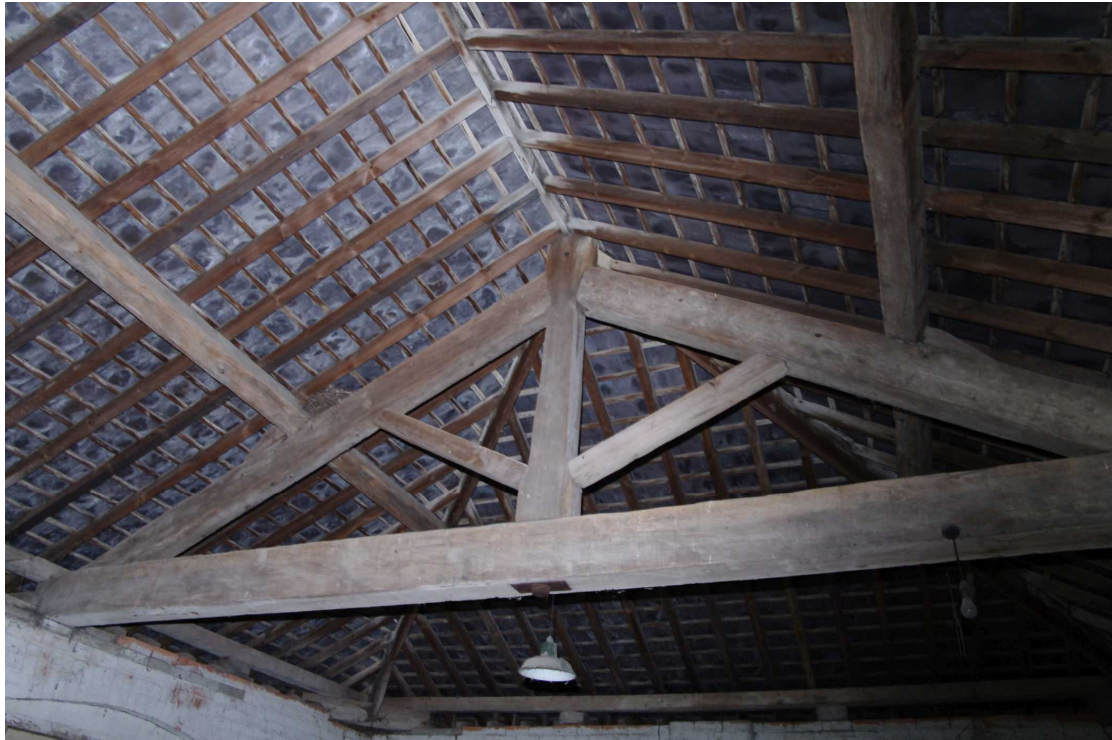
Figure 57 The Coach House first floor, roof detail Looking south-west at western truss
