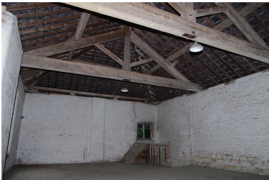
Figure 56 The Coach House first floor Looking north-west. 1m scale. Stairs in far corner
