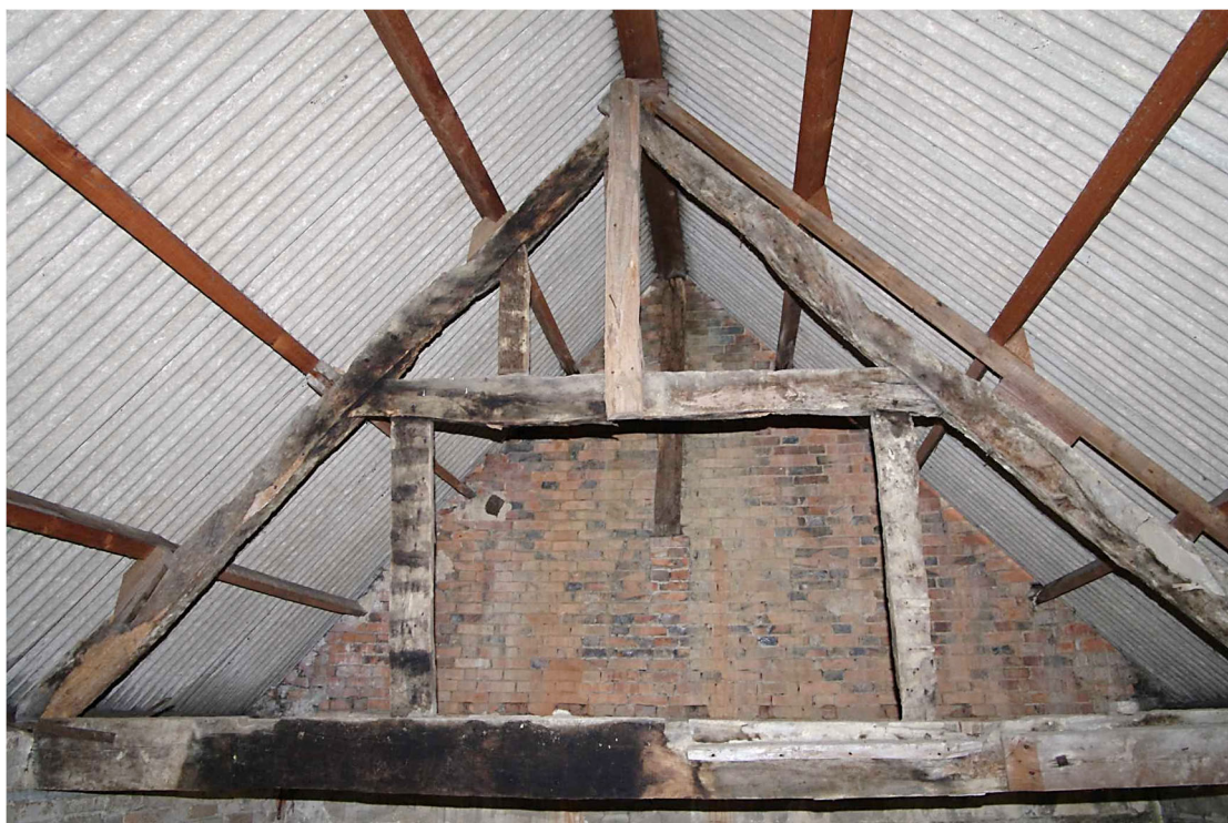
Figure 25 Saddle House roof structure Looking east. Joints are pegged with many reused timbers. There is some burning present on the truss
