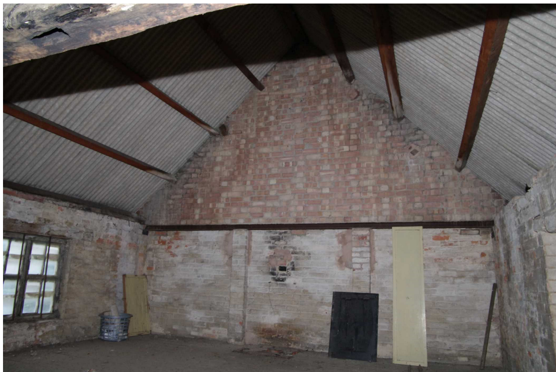
Figure 24 Saddle House first floor Looking south-west. The modern brickwork in the gable rests on a horizontal girder
