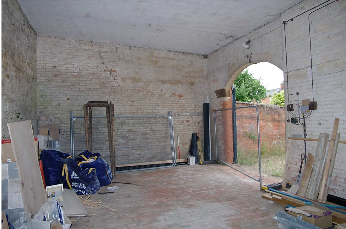
Figure 53 The Coach House ground floor east wing Looking south-east. 1m scale. Note wooden pegs above the scale
