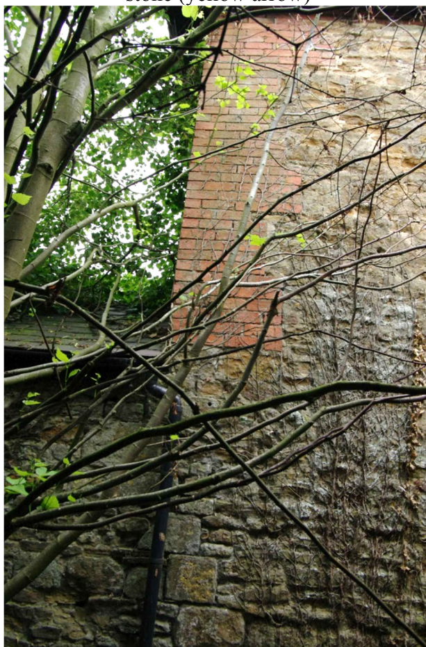
Figure 38 The Coach House east corner of north facing elevation Looking south through undergrowth which hides much of this elevation
