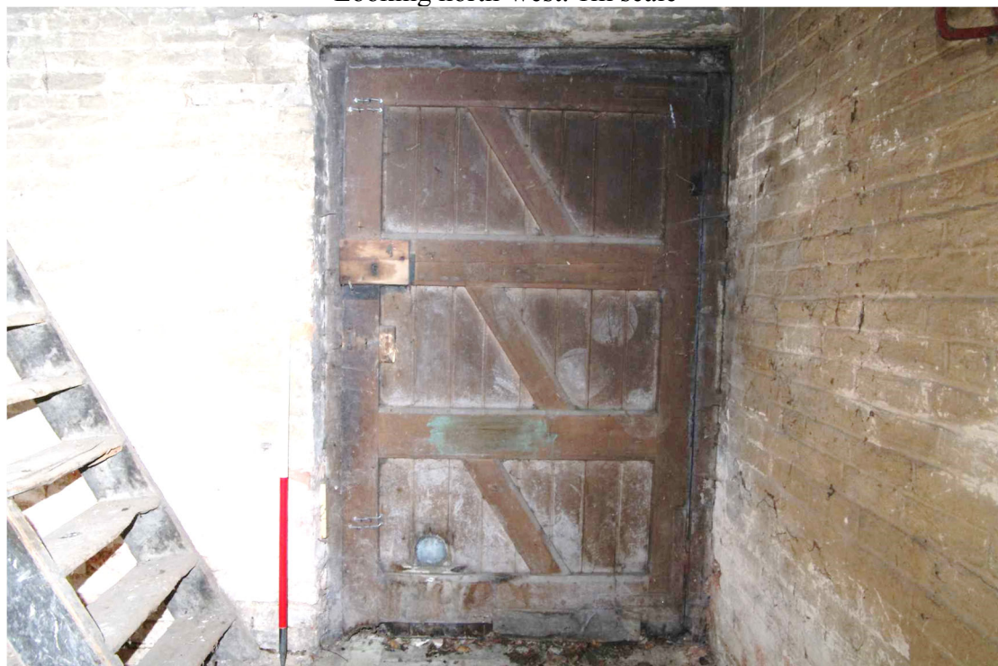
Figure 17 Saddle House ground floor eastern room. North door Looking north. 1m scale. Note wooden lock plate and L-hinges (see Fig. 18 below)
