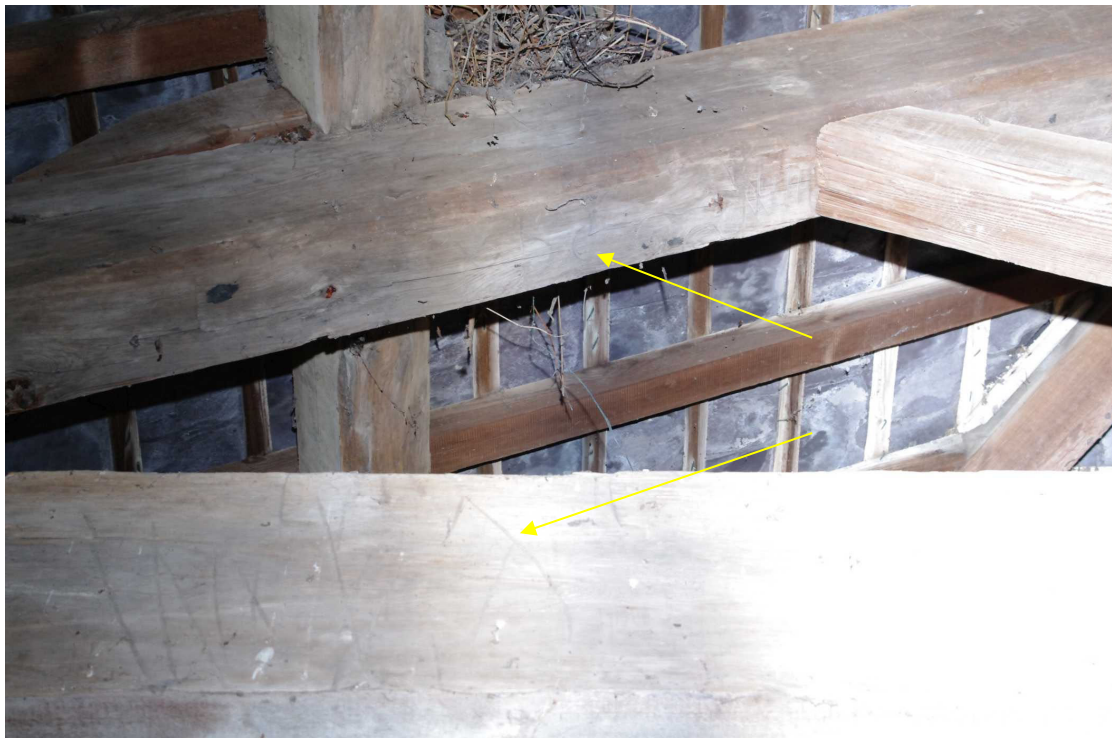
Figure 58 The Coach House first floor Rase marks or apotropaic marks on western truss
