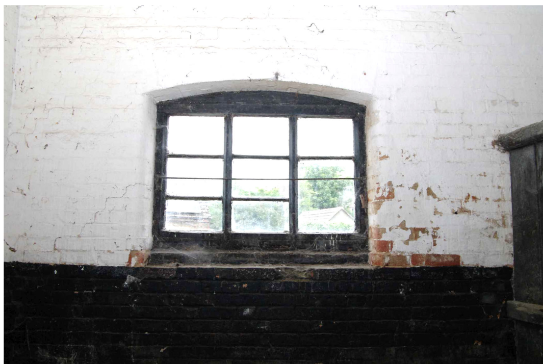
Figure 44 The Coach House ground floor west wing west window detail Looking west
