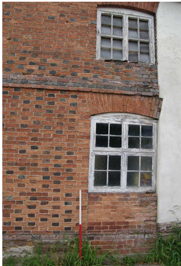
Figure 9 Saddle House south facing elevation blocked door and window detail Looking north. 1m scale
