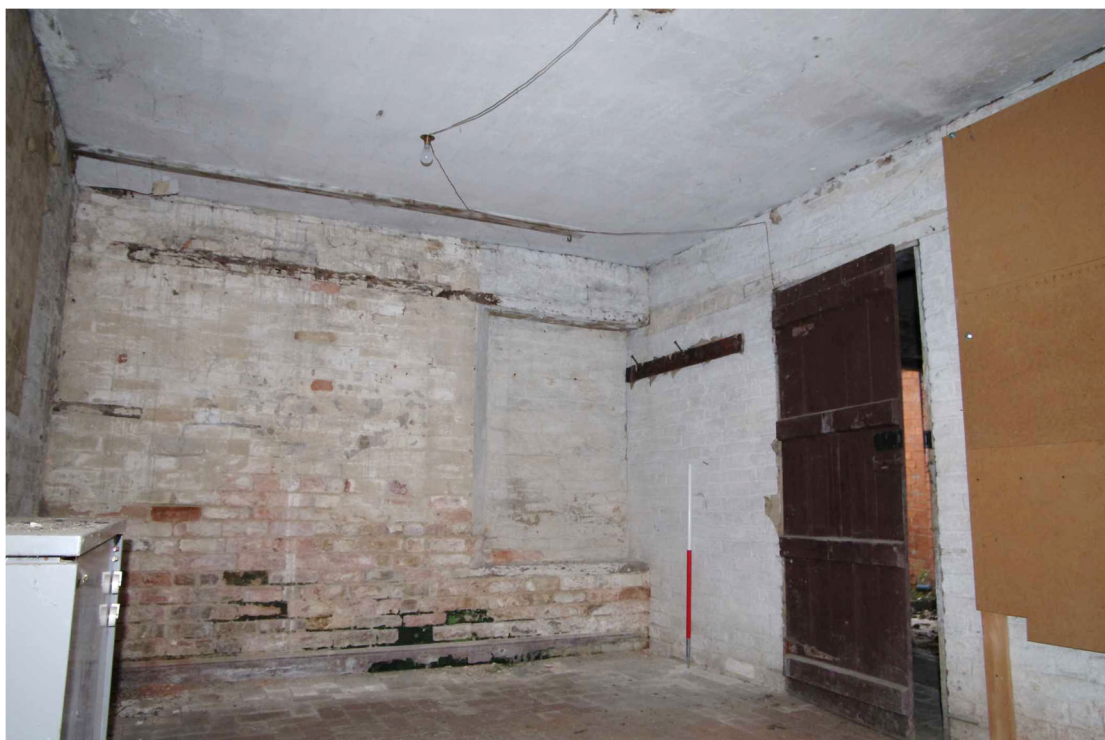
Figure 22 Saddle House ground floor western room Looking north-east. 1m scale. Note blocked window and inserted dividing wall. This room also has remnants of a skirting board and some wallpaper
