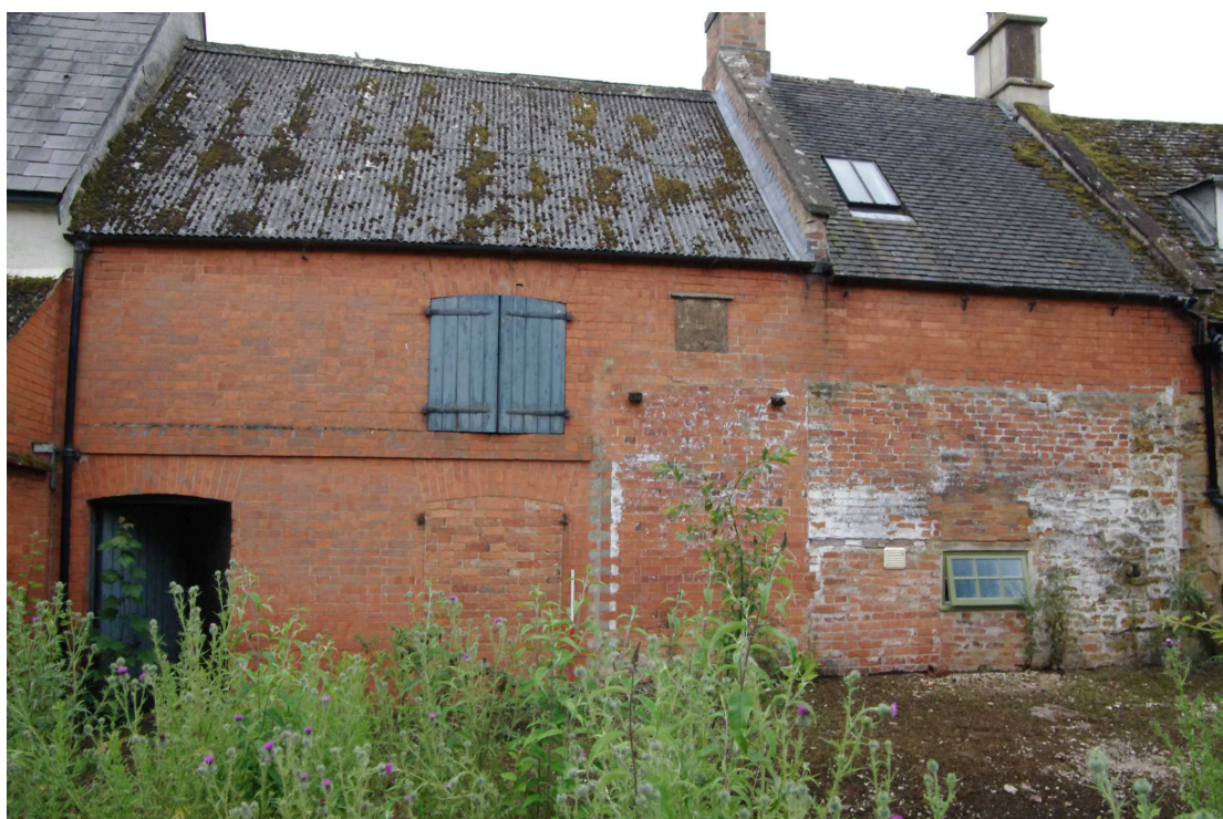
Figure 11 Saddle House north facing elevation Looking south. 1m scale. Note blocked ground floor window. The brick string course above the door stops to the right of the hayloft door. The offset date plaque to the right of the hayloft door has I.H.D. 1821 carved on it
