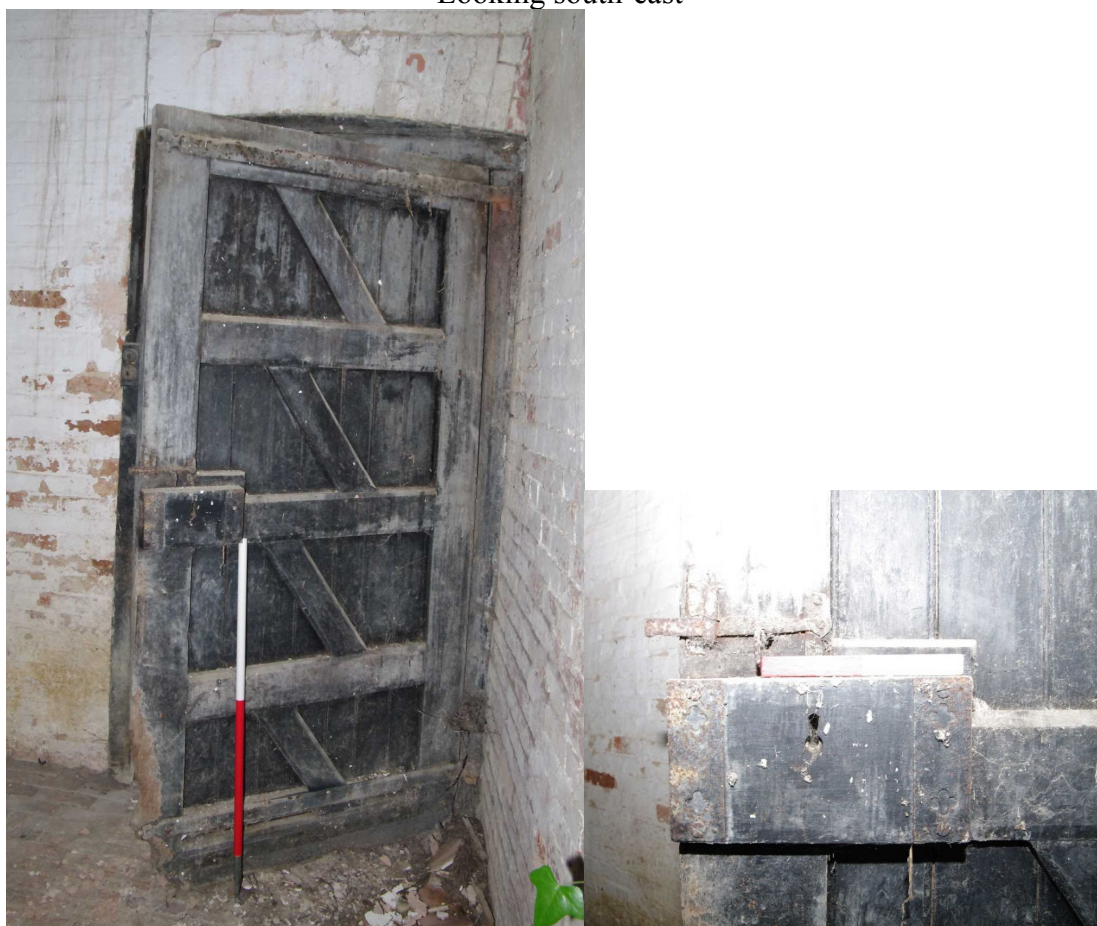
Figure 42 The Coach House ground floor west wing Looking east towards door to centre range. Left: door, 1m scale. Right: Detail of wooden lock plate with metal decoration, 0.2m scale
