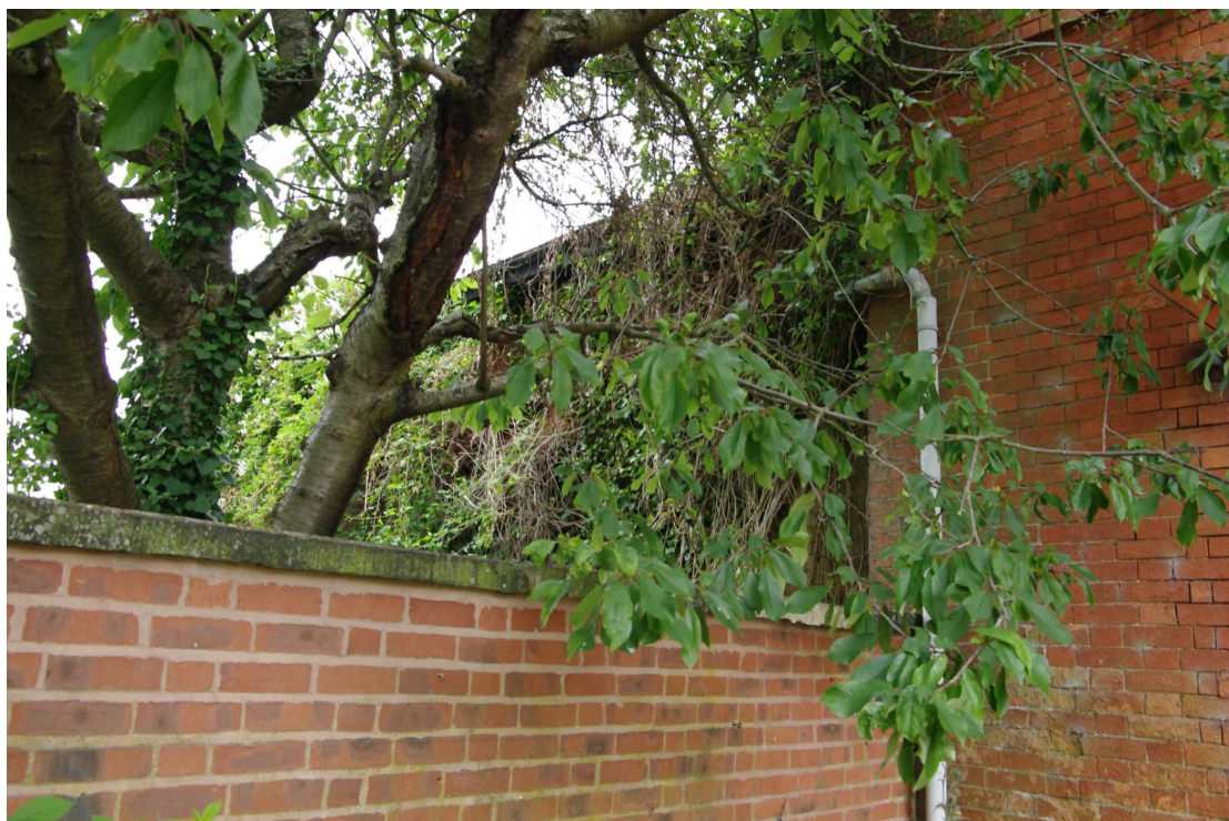
Figure 32 The Coach House south facing elevation, west wing Looking north-west over dividing wall. The west wing is covered with vegetation
