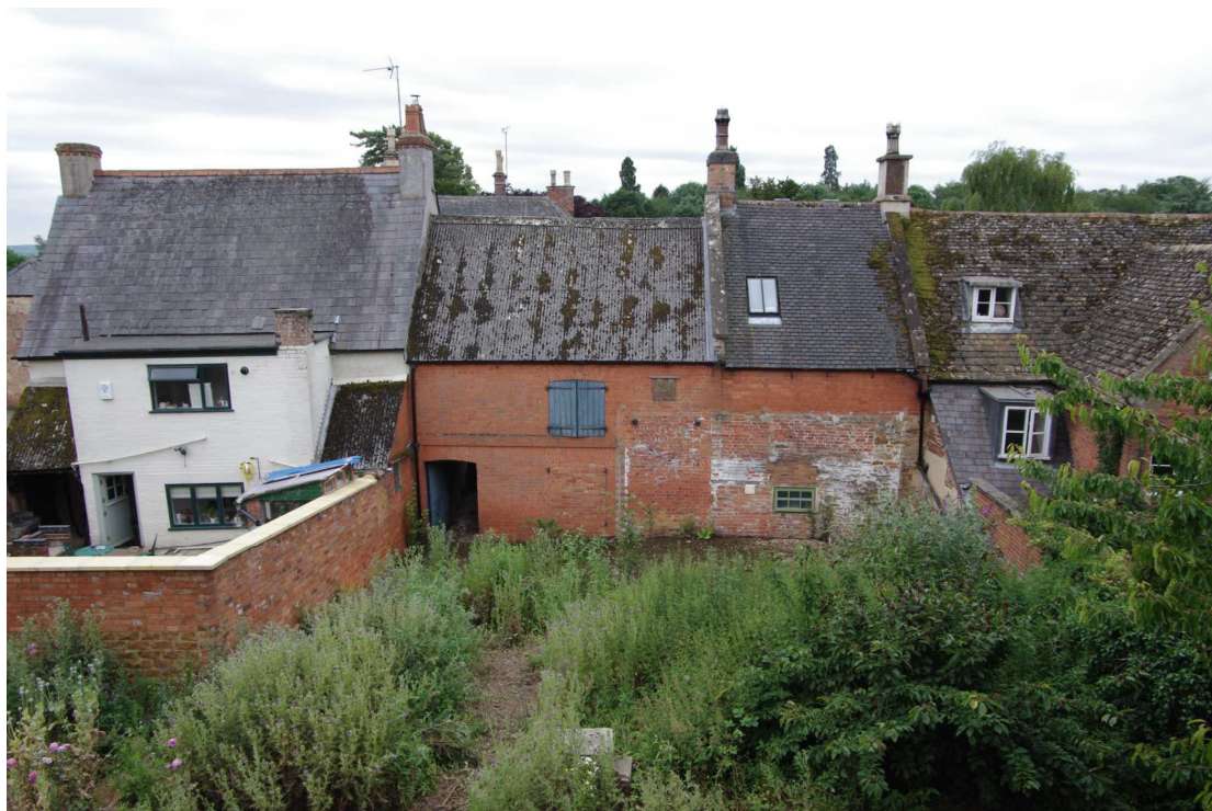
Figure 10 Saddle House north facing elevation Looking south. Saddle House has the corrugated roof. Note the different type of bricks used compared to the south facing elevation
