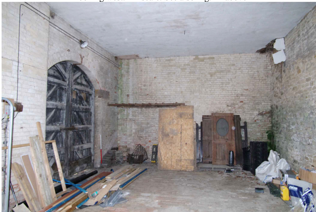
Figure 52 The Coach House ground floor east wing Looking west. 1m scale. Note hooks on ceiling for holding lights
