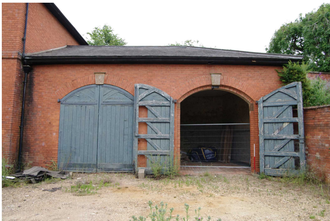
Figure 35 The Coach House south facing elevation, eastern wing Looking north. 1m scale
