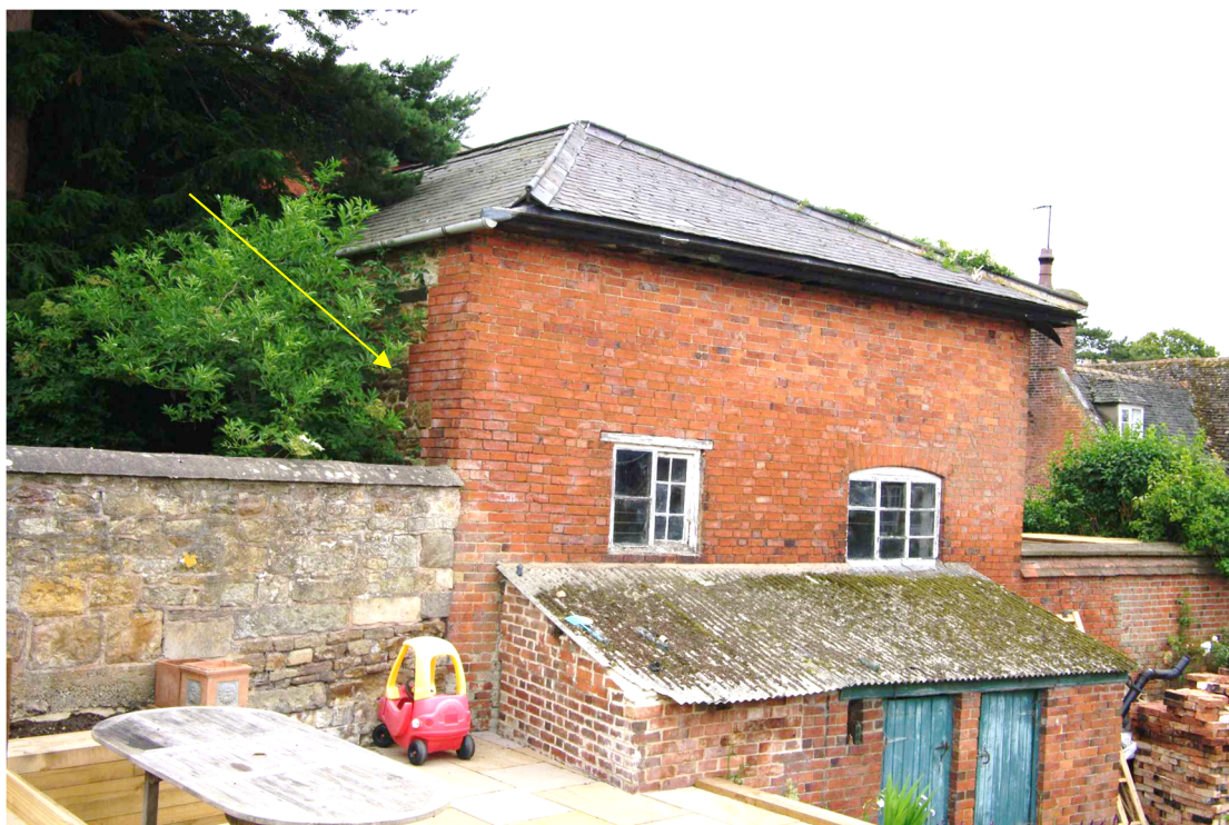
Figure 37 The Coach House west facing elevation Looking south-east. Note how the rear (north) facing elevation changes from brick to stone (yellow arrow)
