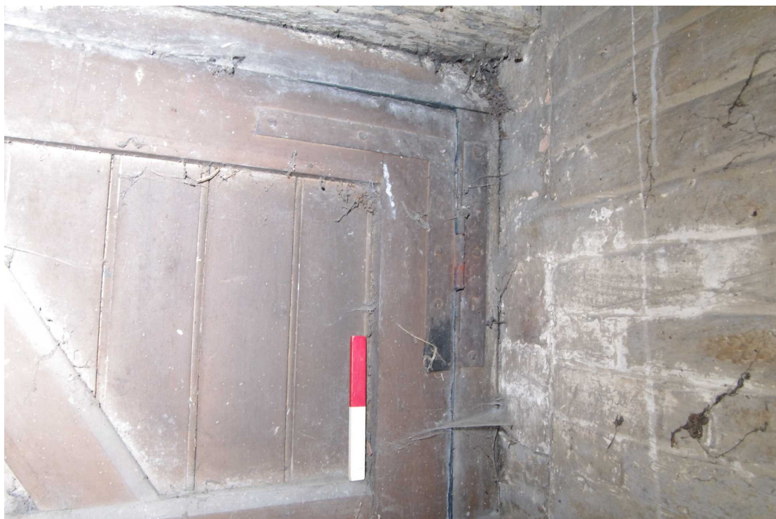
Figure 19 Saddle House ground floor eastern room L-hinges Looking north-east. 0.2m scale. Probable late 18th or early 19th century
