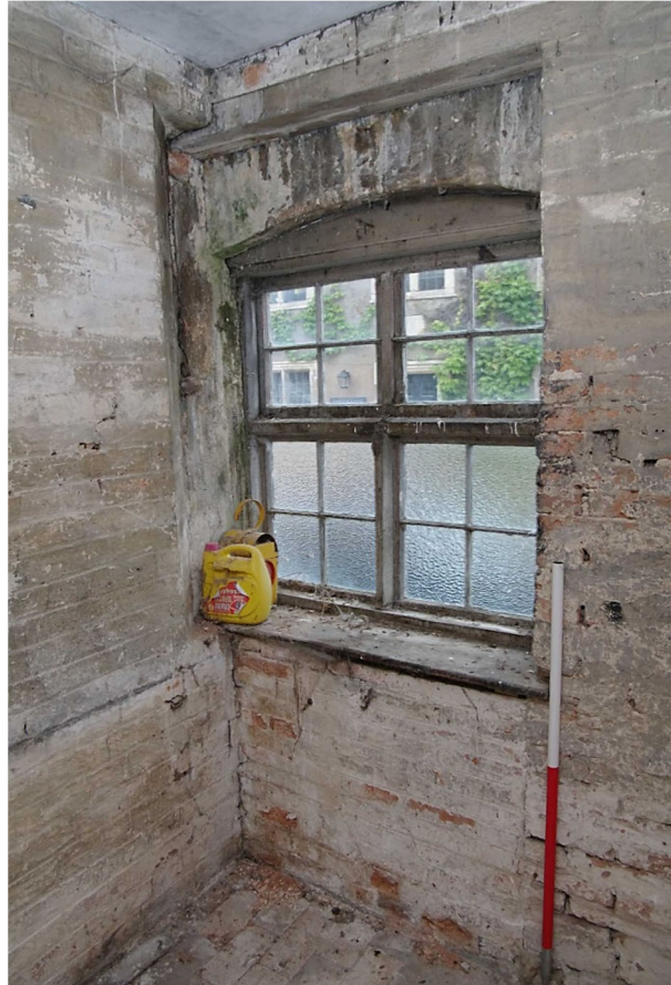
Figure 14 Saddle House ground floor eastern room. Modified doorway Looking south-east. 1m scale. Note how the left hand edge of the doorway is chamfered into the wall
