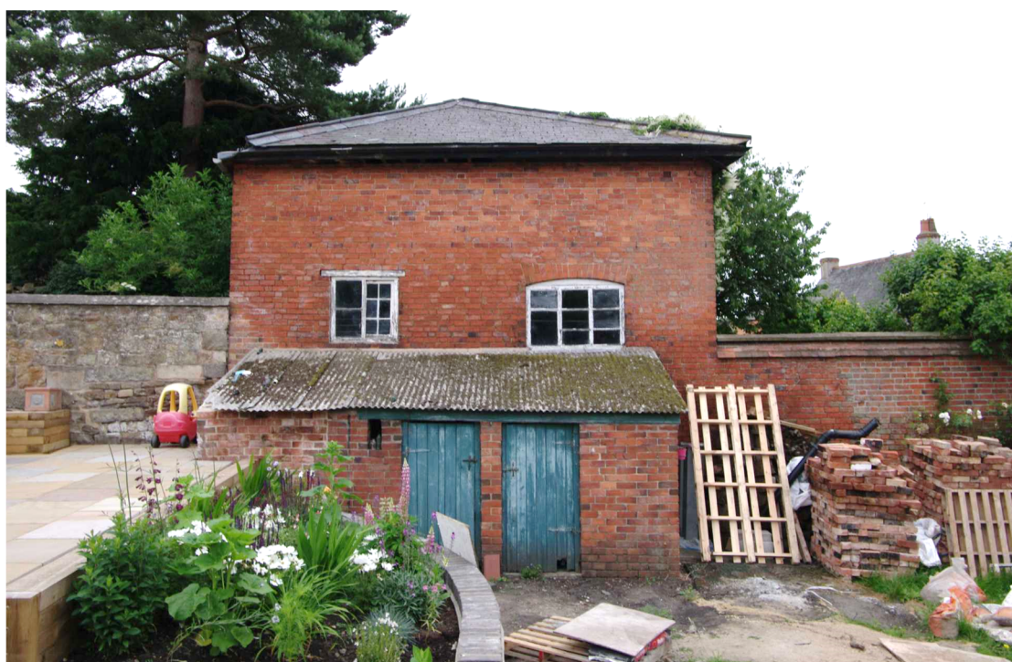
Figure 36 The Coach House west facing elevation Looking east. The lean-to outbuildings are a later addition but are still shown on the First Edition Ordnance Survey 1886 map
