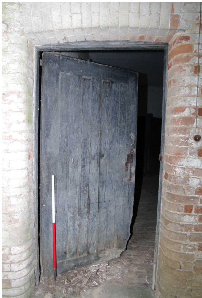
Figure 51 The Coach House ground floor middle range. Door to west wing Looking west. 1m scale. See also Fig. 42 above
