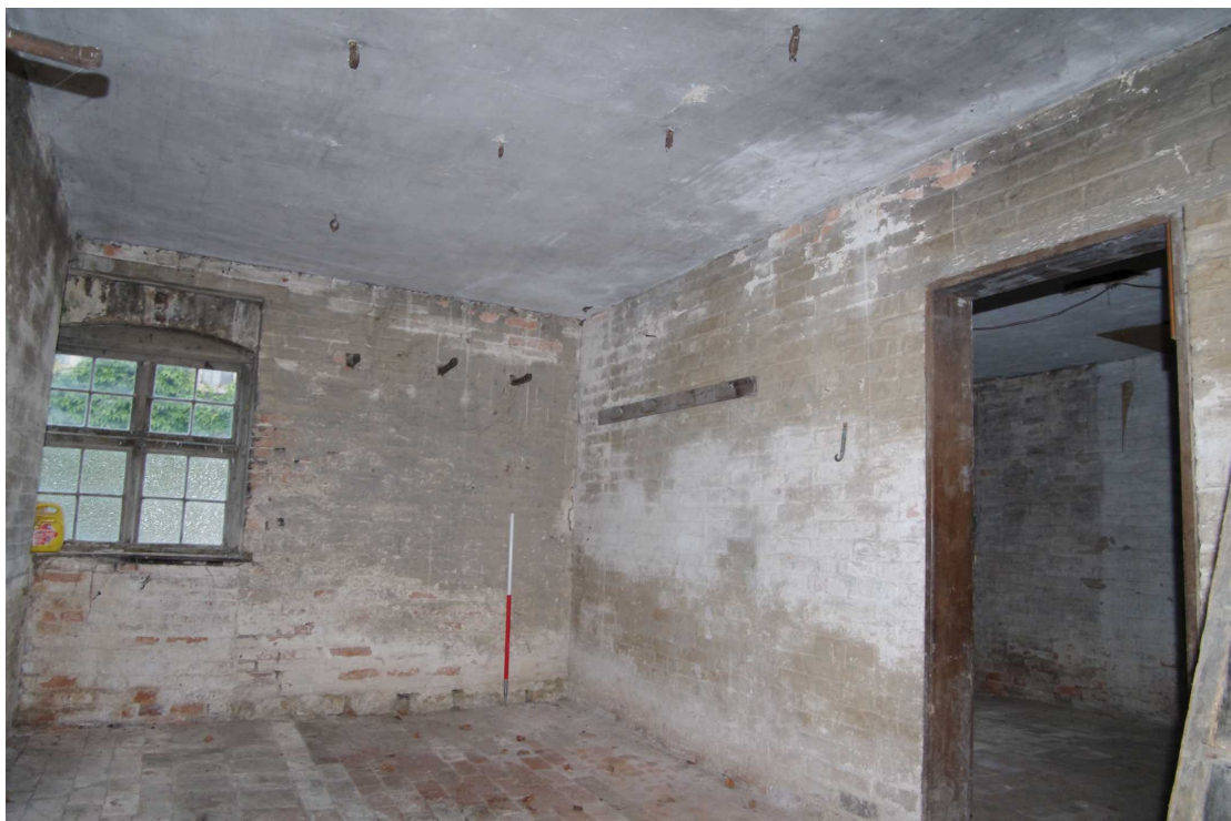
Figure 13 Saddle House ground floor eastern room Looking south-west. 1m scale. The window on the left has been modified from a former doorway onto Churchgate. Note the wooden hooks on the wall
