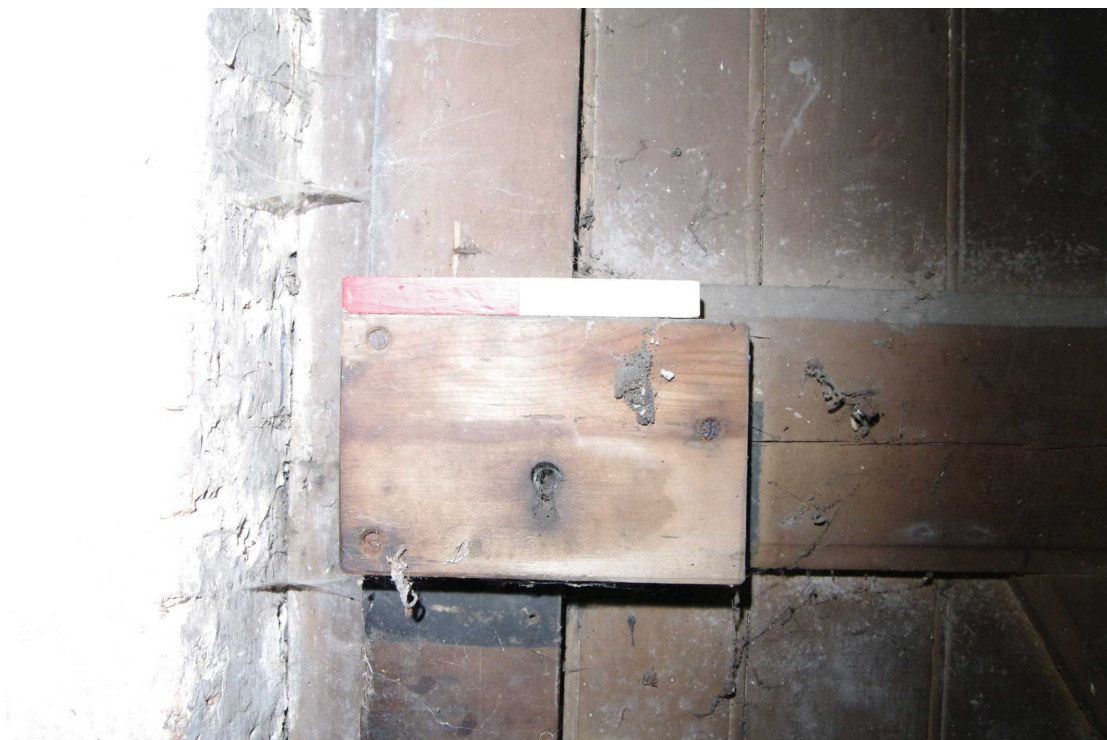
Figure 18 Saddle House ground floor eastern room wooden lock plate on door Looking north. 0.2m scale. Probable late 18th or early 19th century
