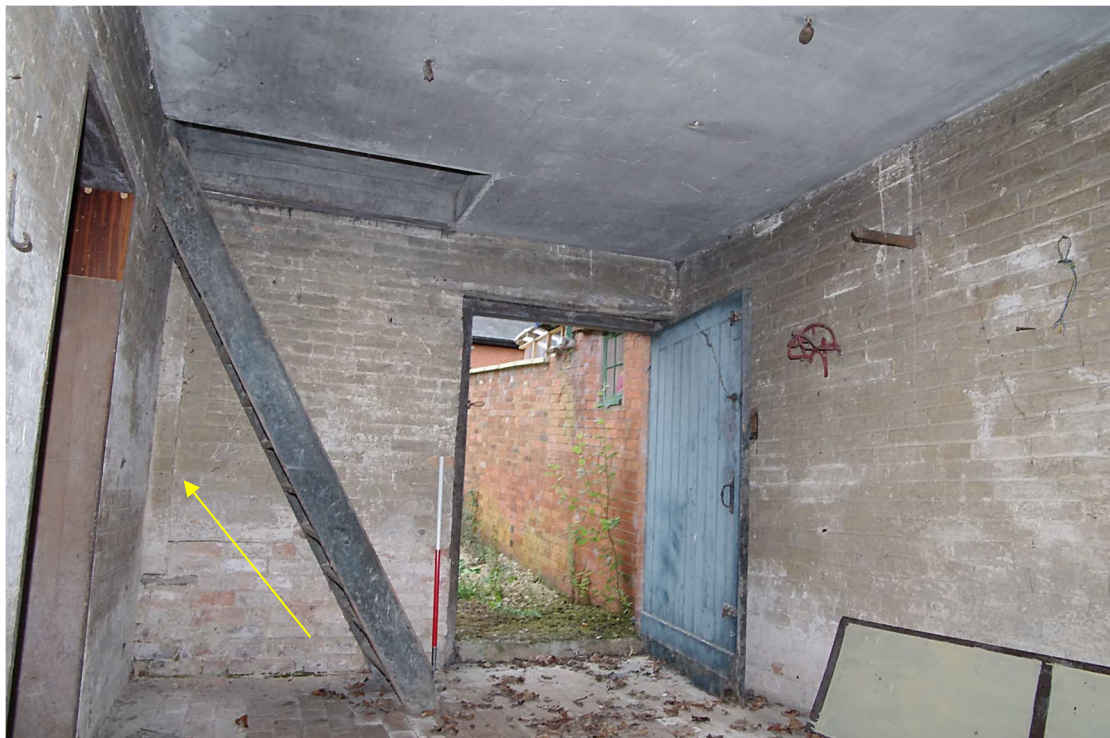
Figure 15 Saddle House ground floor eastern room Looking north-east. 1m scale. Steps lead up to first floor. The arrow points to blocked edge of window which has been partially obscured by the inserted dividing wall
