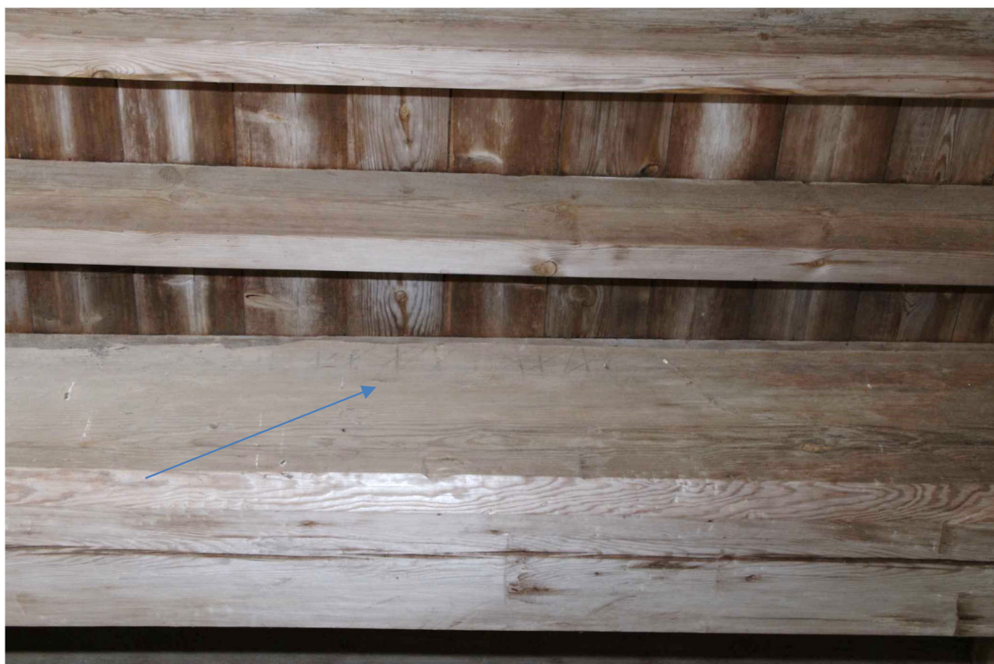
Figure 49 The Coach House ground floor middle range Rase marks or apotropaic marks on top edge of stop-chamfered beam
