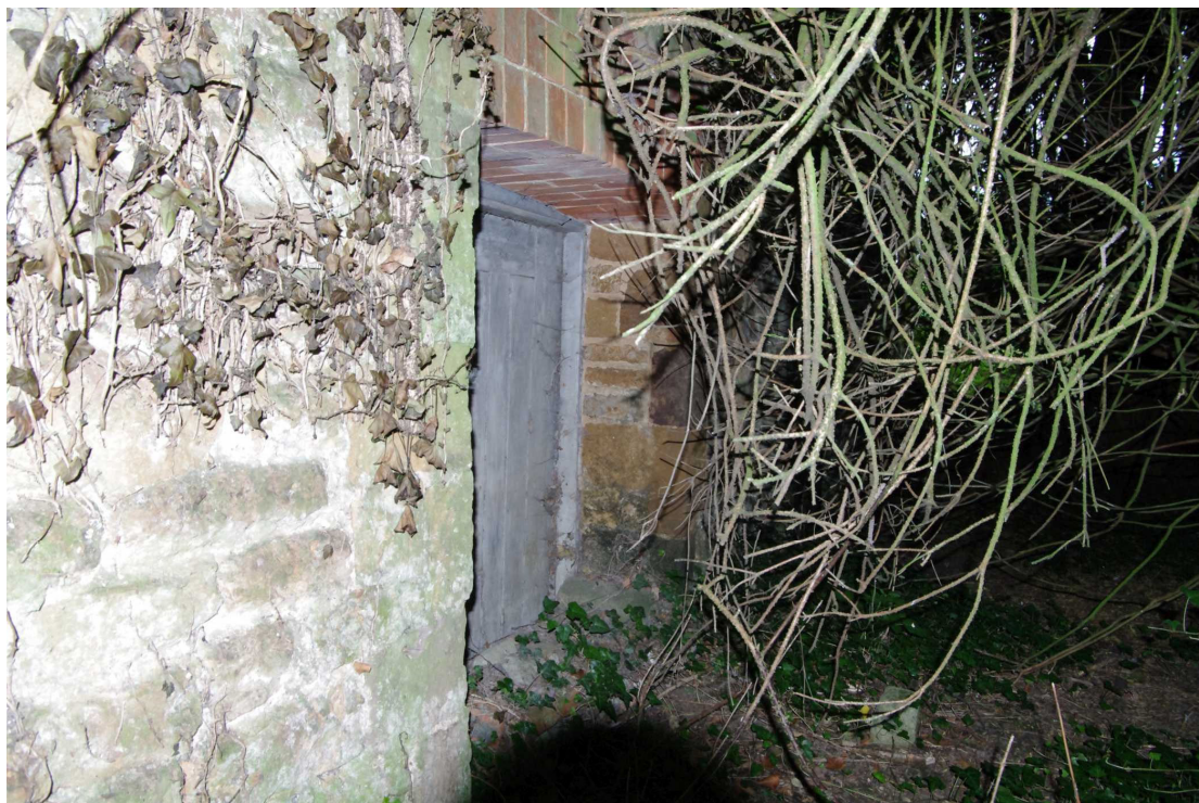
Figure 39 The Coach House north facing elevation doorway Looking south-west. The ground level on this side of the building has risen to half cover the doorway
