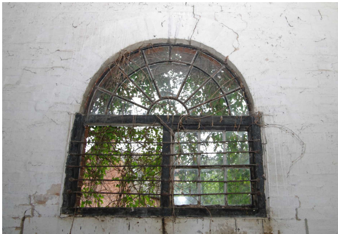
Figure 43 The Coach House ground floor west wing south window detail Looking south
