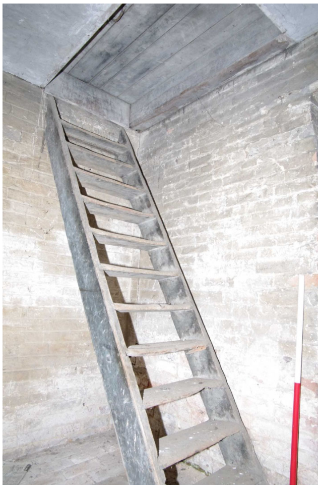
Figure 16 Saddle House ground floor eastern room stairs to first floor Looking north-west. 1m scale
