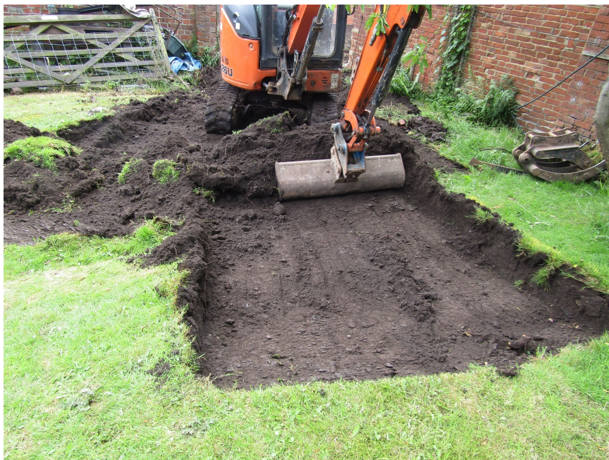
Figure 7: Work in progress on the area north of the workshop, looking south-east
